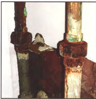
LOW PRESSURE DAMAGING LEAKS
