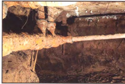
CAST IRON/ABS PIPES SEWER LINE FAILURE
