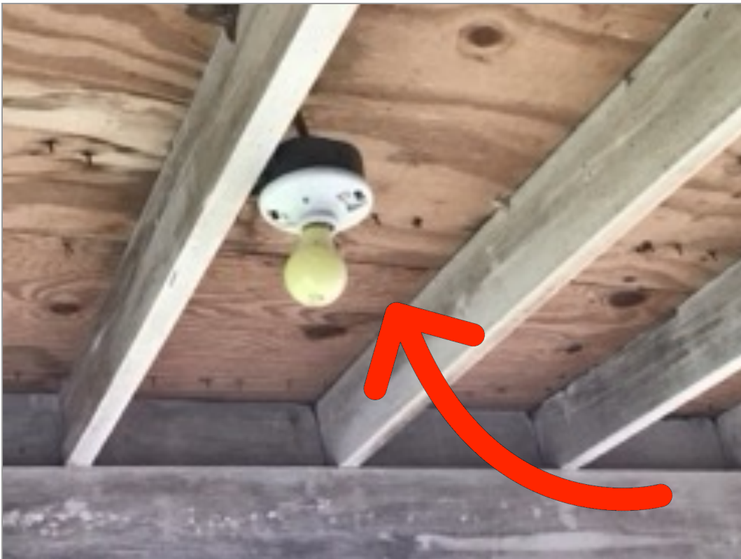
Front Exterior Light Fixtures Light did not turn on.
