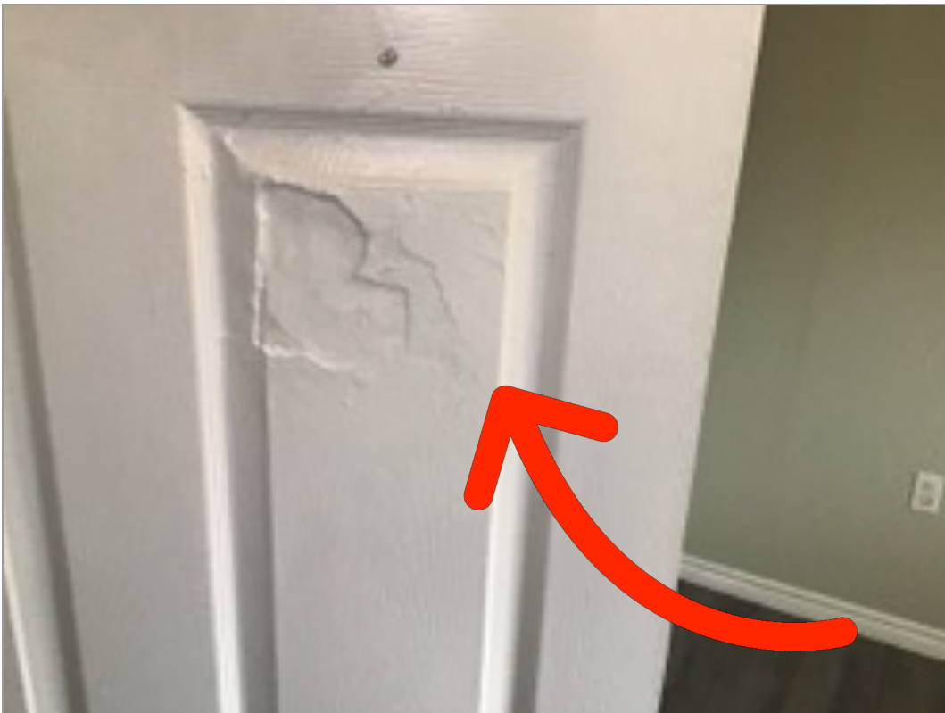
Bedroom 1 Door Door is cracked
