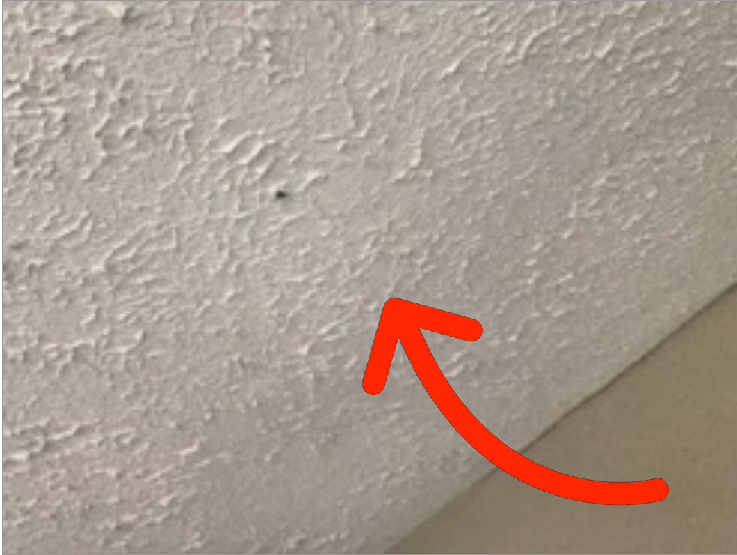
Living Room Ceiling Holes
