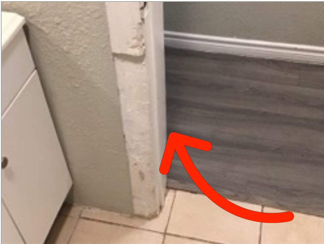
Bathroom 1 Walls/Paint Cracks in texture
