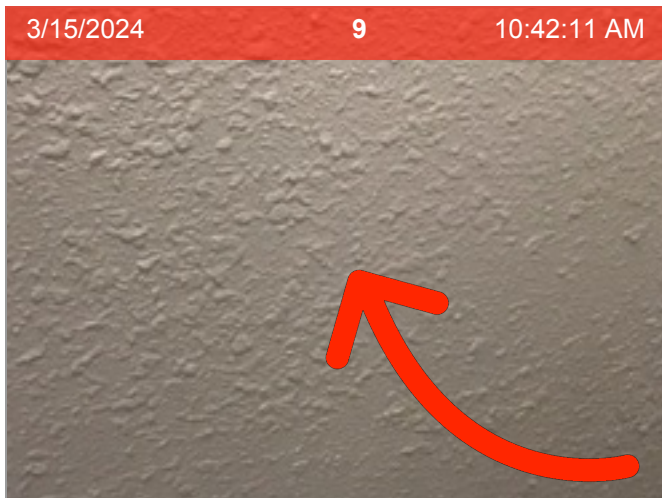
Door Stop | Missing- no wall damage noted.
