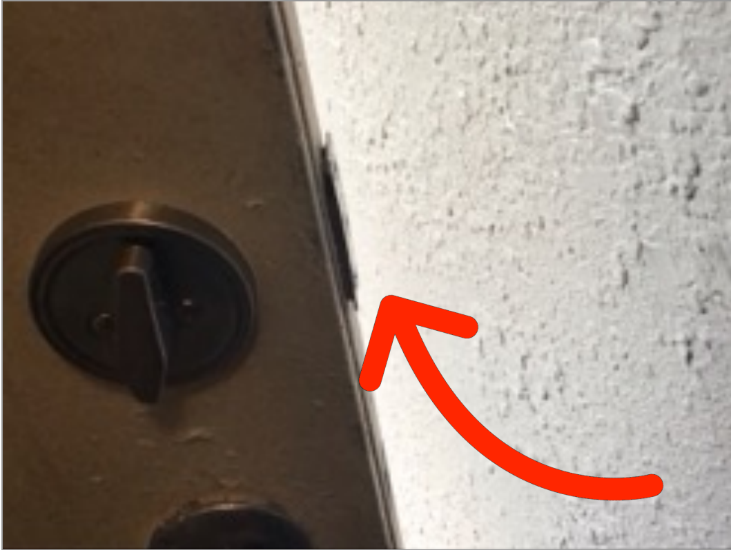
Entry Front Door Interior Hard to close door
