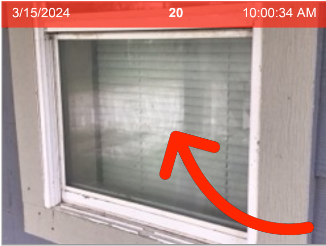
Window Screens | Screen(s) are missing
