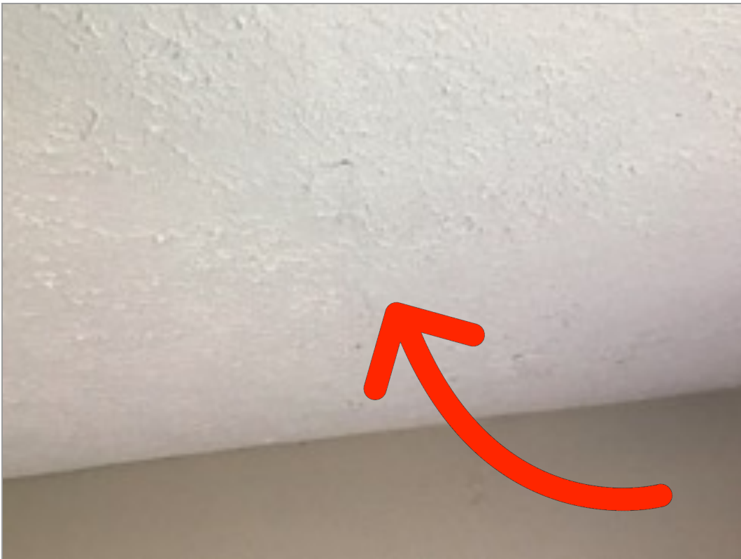
Living Room Ceiling Cracks in ceiling.
