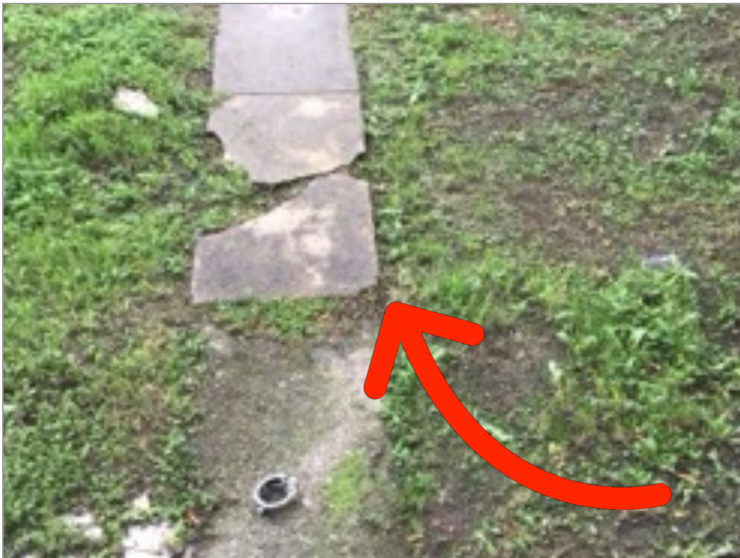
Front Exterior Walkways Cracked or uneven
