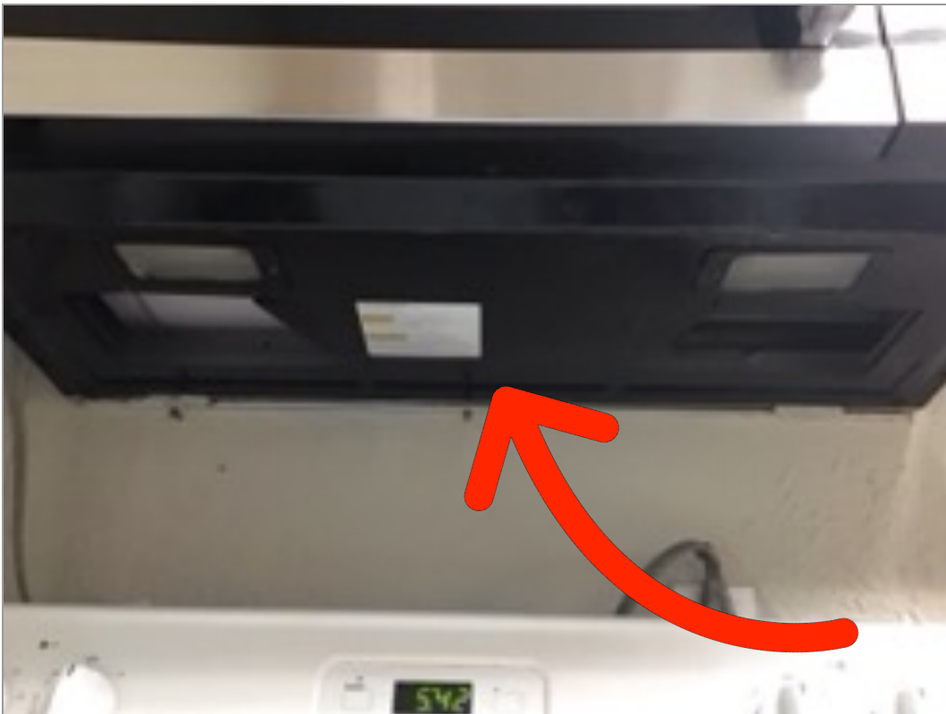
Kitchen Exhaust Fan No filters
