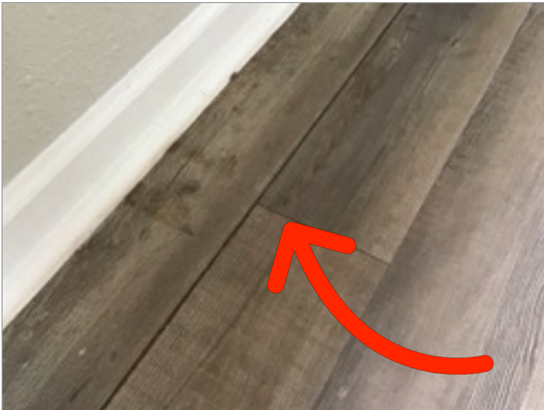
Living Room Floors Flooring is stained.
