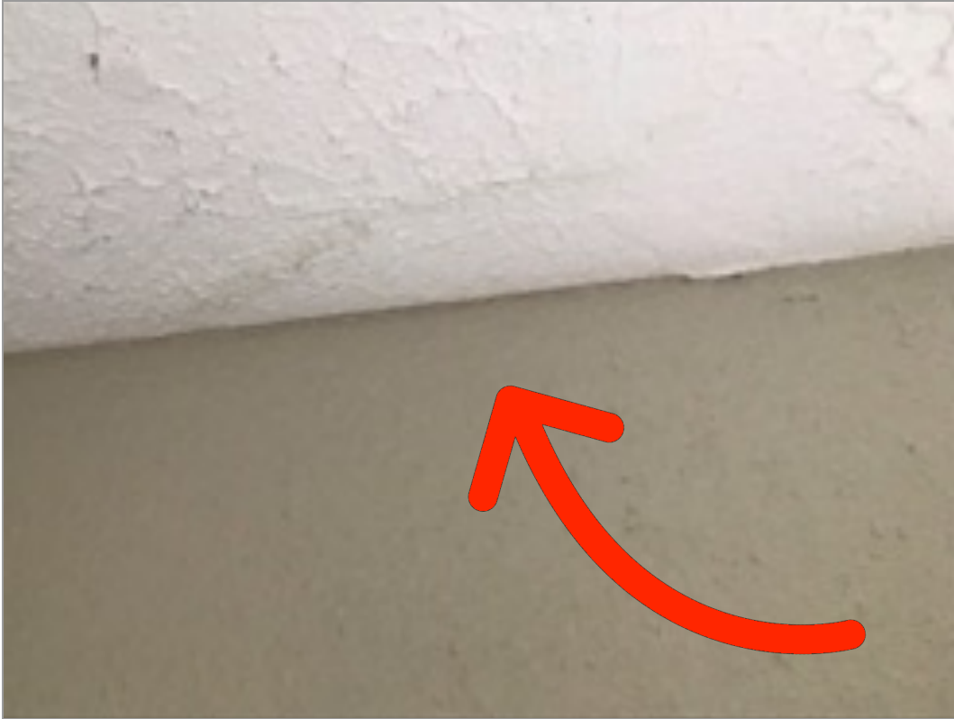
Living Room Ceiling Cracks in ceiling.
