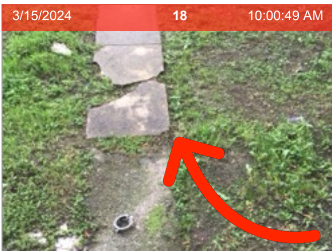
Walkways | Cracked or uneven
