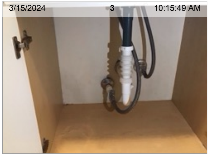
Cabinet Under Sink
