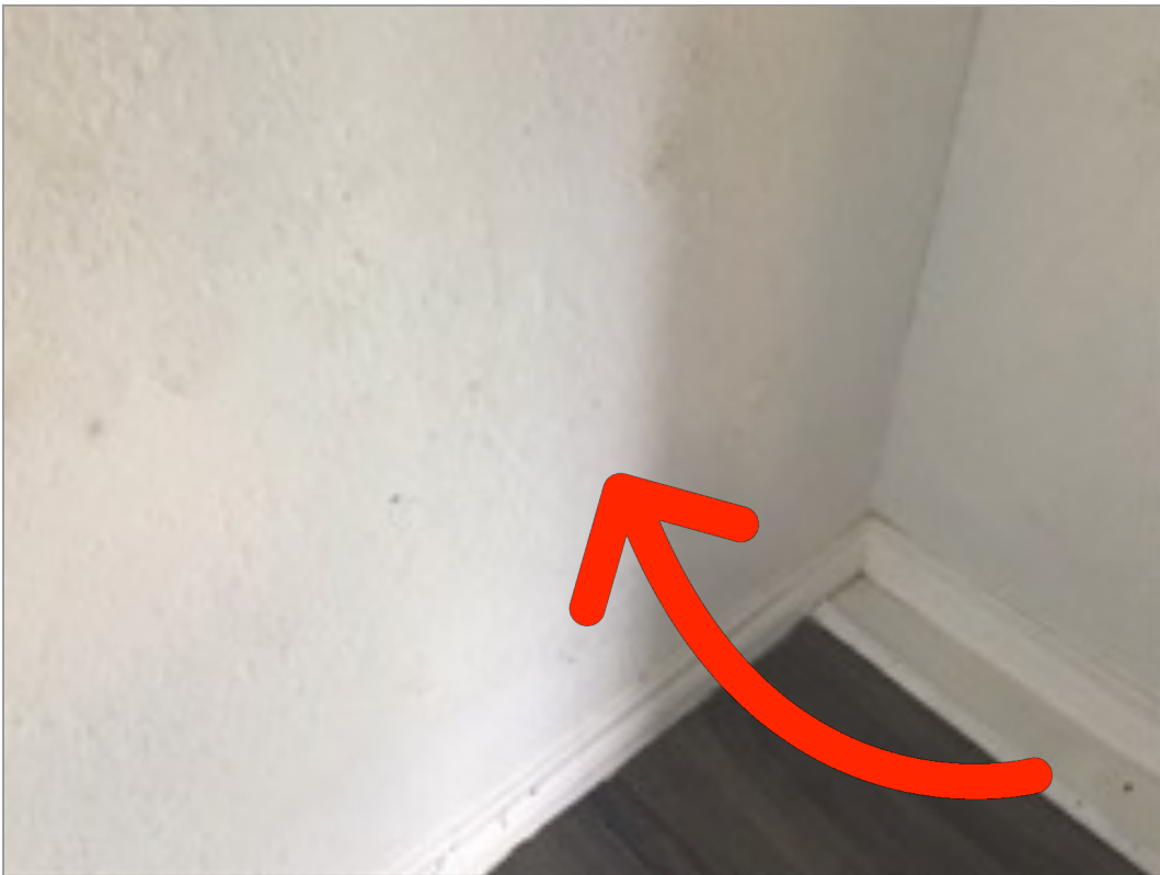
Bedroom 2 Closets Stains on the wall
