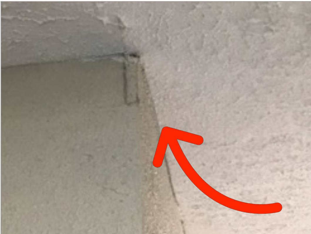
Kitchen Walls/Paint Cracks in texture
