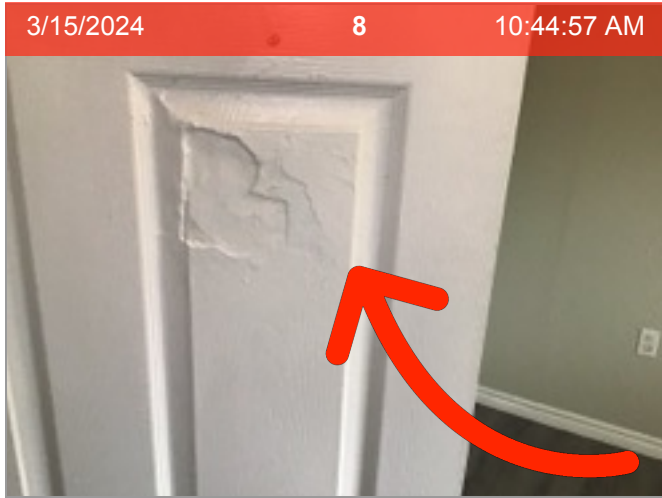
Door | Door is cracked
