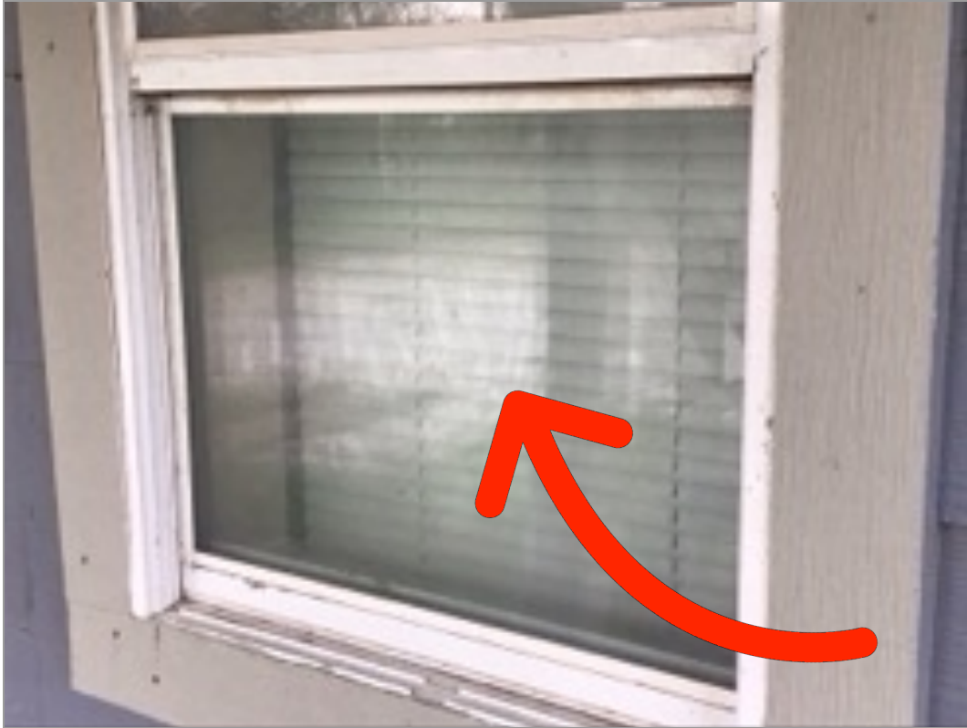
Front Exterior Window Screens Screen(s) are missing
