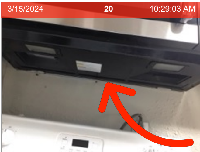
Microwave Oven | GE | No power to light
