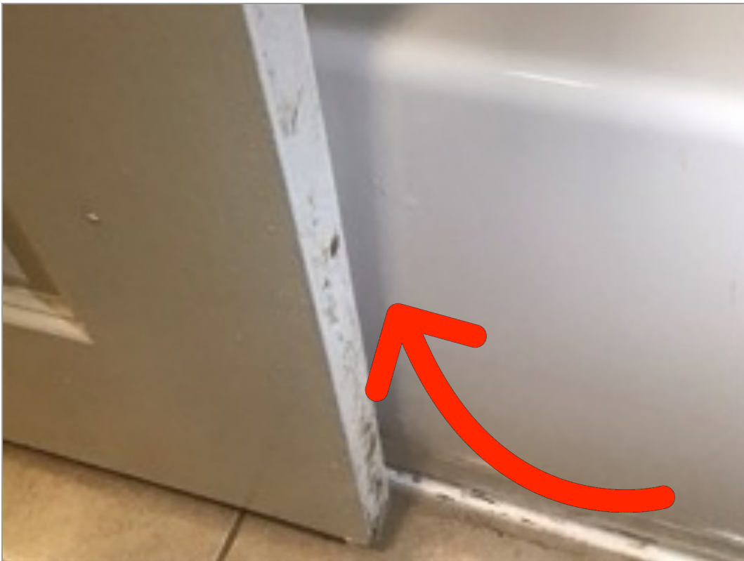
Bathroom 1 Door Stop Missing- wall damage noted.
