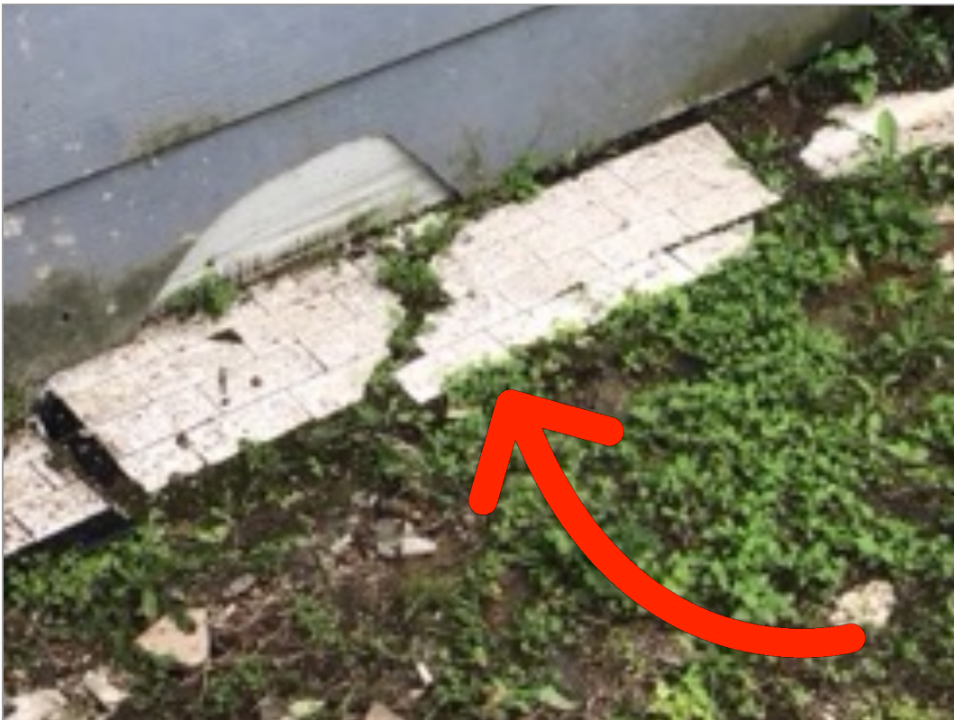
Front Exterior Walls/Siding/Trim Cracked/peeling paint
