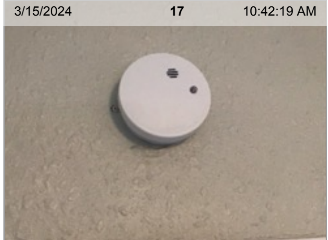
3/15/2024 17 10:42:19 AM Wireless Smoke Alarm (mfd 11/2021) | Smoke test: Failed | Alarm in place | 2.4 years old
