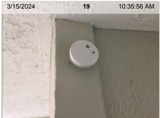
Wireless Smoke Alarm (mfd 11/2021) | Smoke test: Failed | Alarm in place
