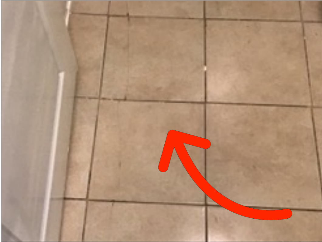
Bathroom 1 Floors Crack in flooring.
