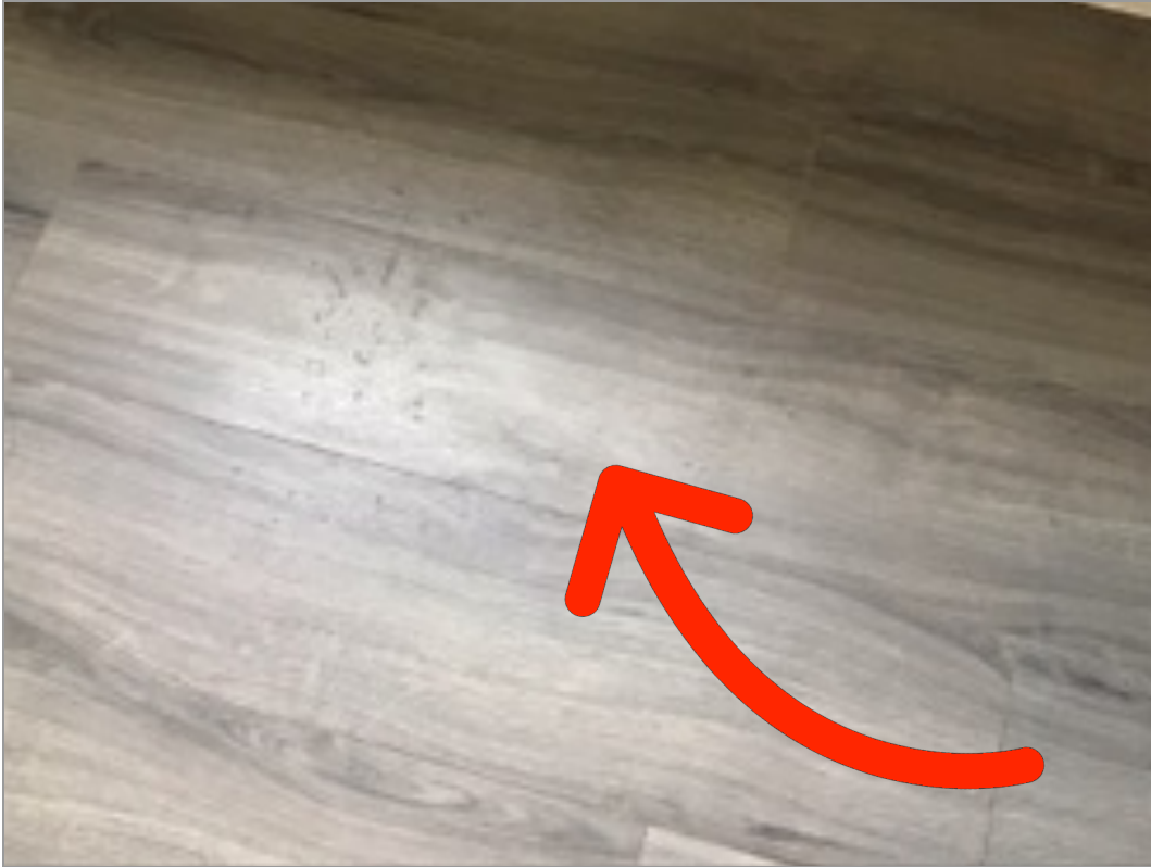
Bedroom 1 Floors Flooring is stained.
