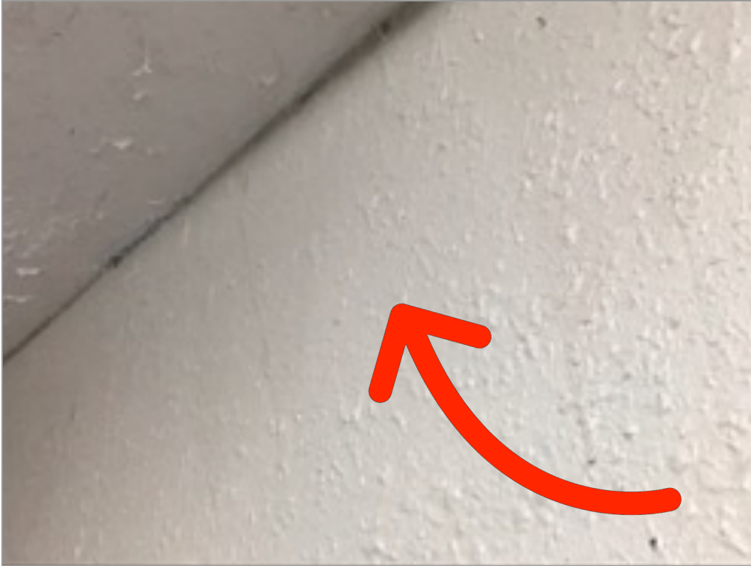
Kitchen Walls/Paint Spiderwebs
