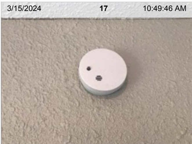
Wireless Smoke Alarm (mfd 11/2021) | Smoke test: Passed | Alarm in place
