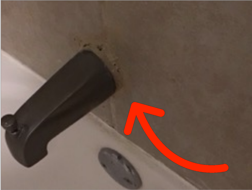
Bathroom 1 Tub/Fixture Grout is discolored/cracking
