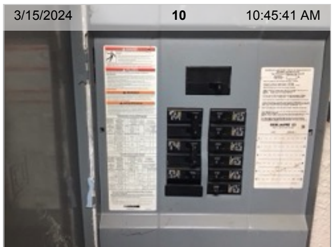
Electrical Breaker Panel
