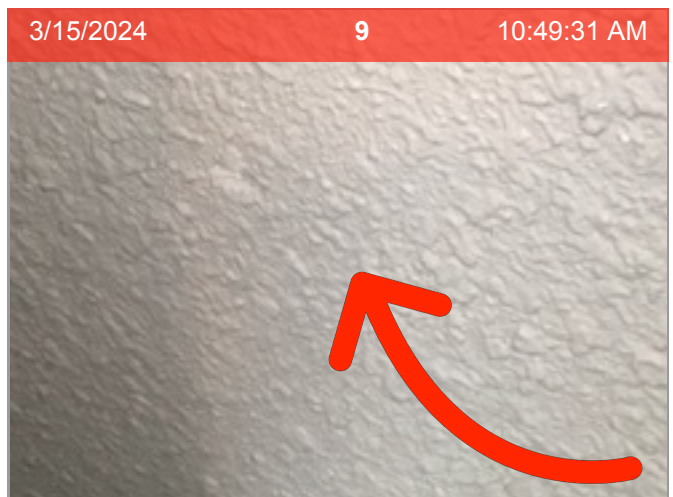
Door Stop | Missing- wall damage noted.
