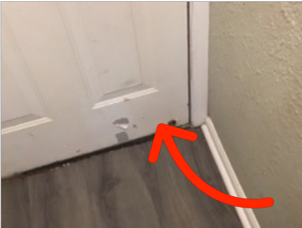
Entry Front Door Interior Scuffs on door
