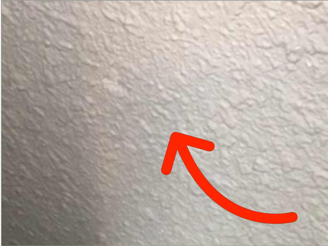
Bedroom 2 Door Stop Missing- wall damage noted.
