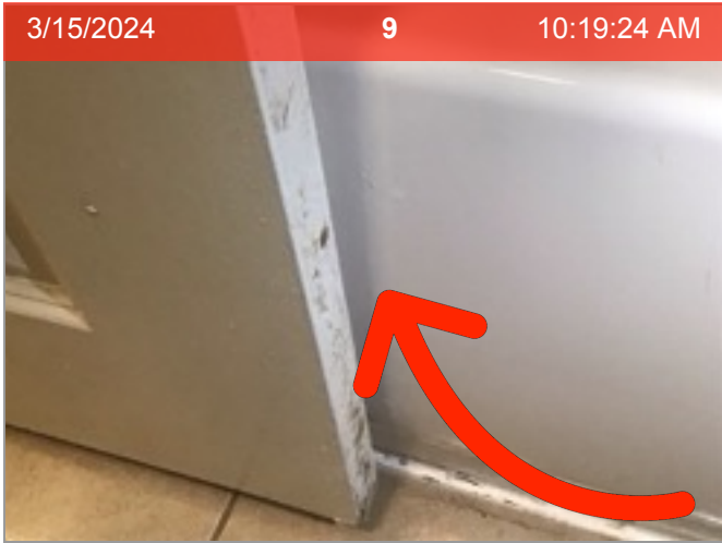
Door Stop | Missing- wall damage noted.
