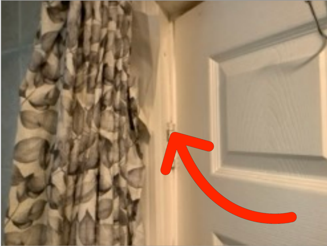
Bathroom 1 Door Stop Missing- no wall damage noted.
