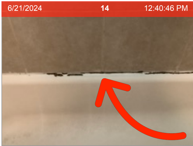
Tub/Fixture | Grout is discolored/cracking
