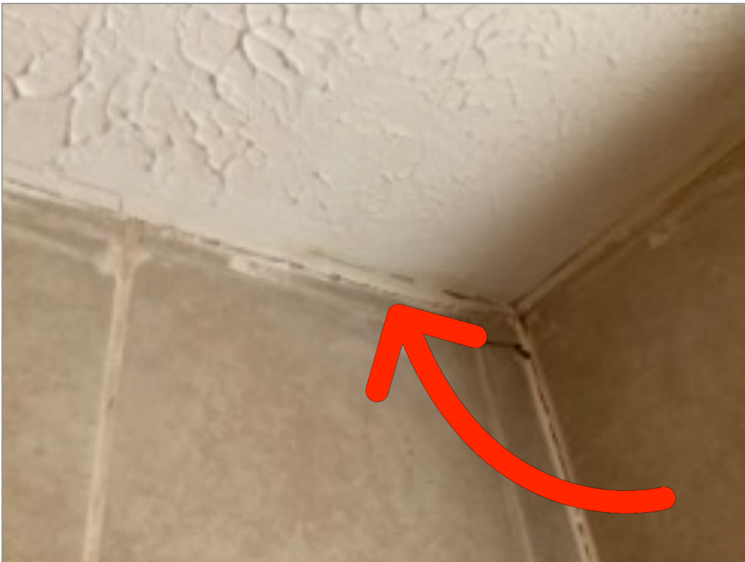
Bathroom 1 Ceiling Cracks in ceiling.
