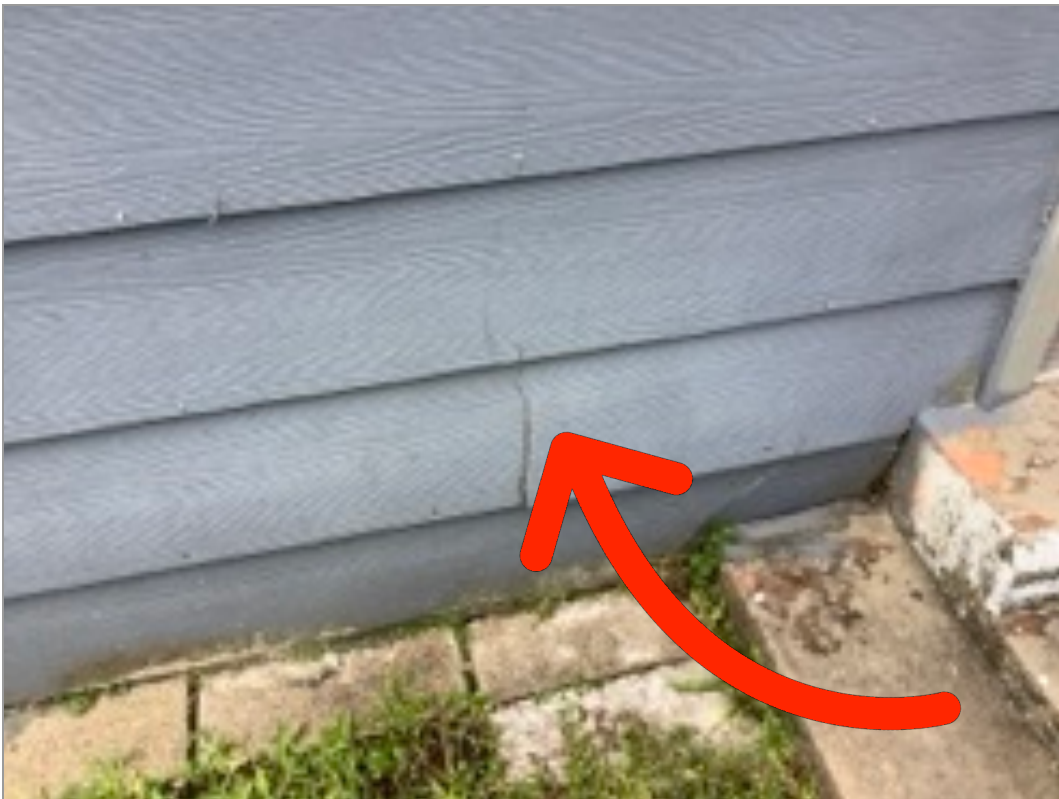
Front Exterior Walls/Siding/Trim Cracked/peeling paint
