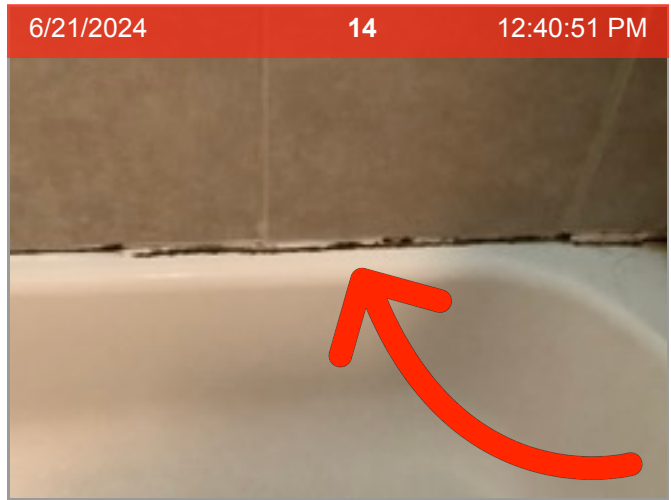
Tub/Fixture | Grout is discolored/cracking
