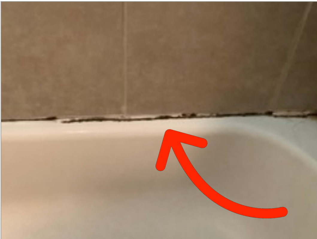
Bathroom 1 Tub/Fixture Grout is discolored/cracking
