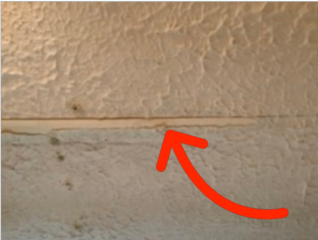
Bathroom 1 Ceiling Cracks in ceiling.
