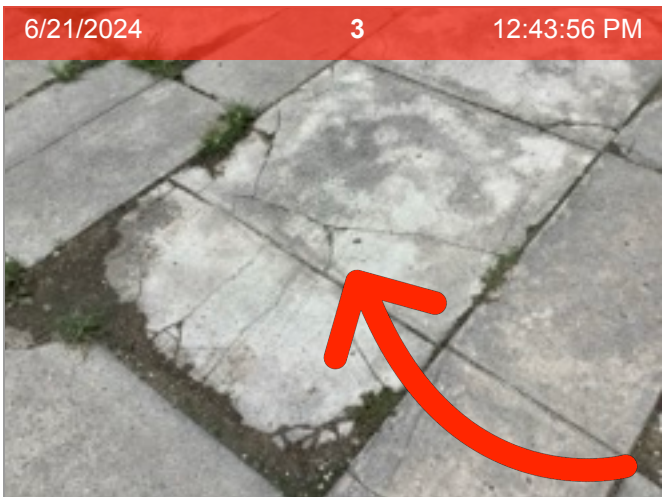
Driveway | Spider cracks in driveway.
