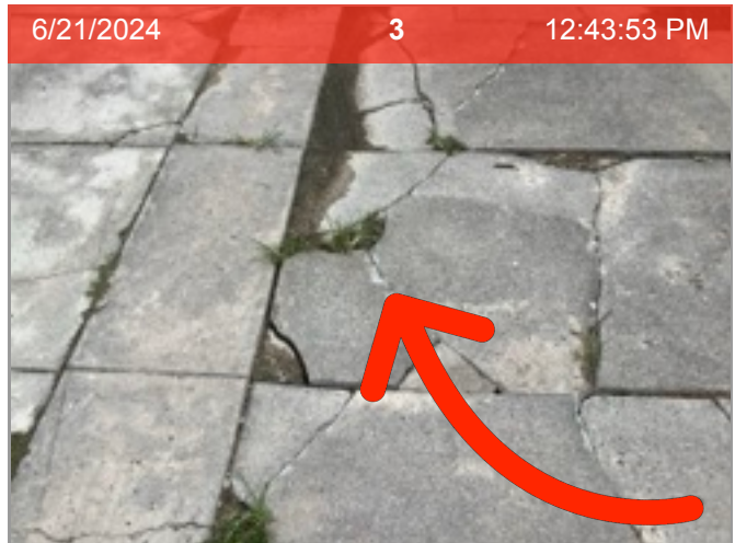
Driveway | Spider cracks in driveway.
