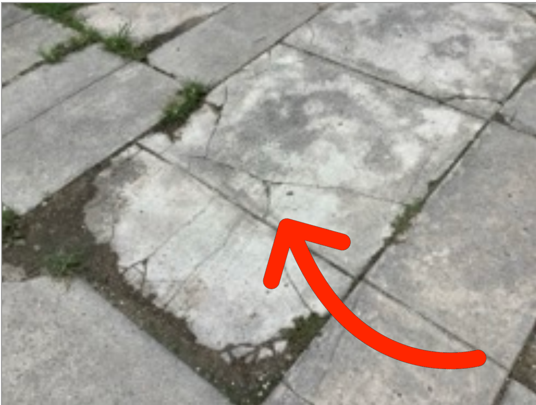
Front Exterior Driveway Spider cracks in driveway.
