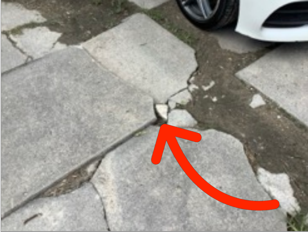
Front Exterior Driveway Driveway crack appears unlevel (see closeup).
