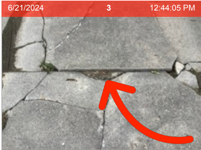
Driveway | Driveway crack appears unlevel (see closeup).
