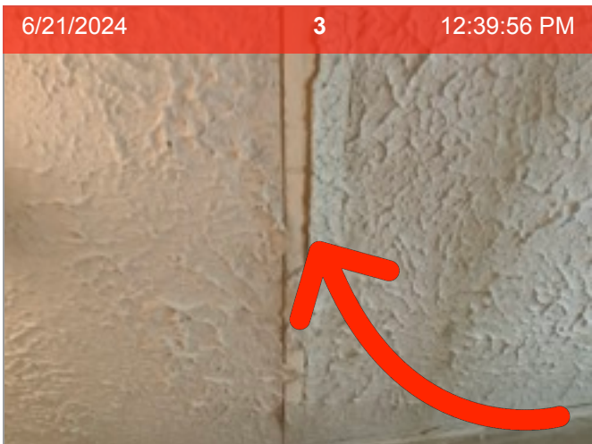
Ceiling | Cracks in ceiling.
