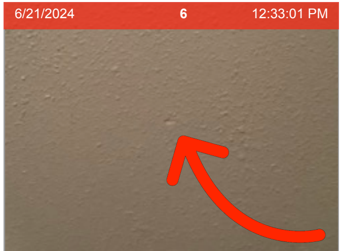
Door Stop | Missing- wall damage noted.
