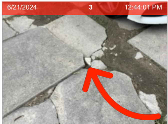
Driveway | Driveway crack appears uneven (see closeup).
