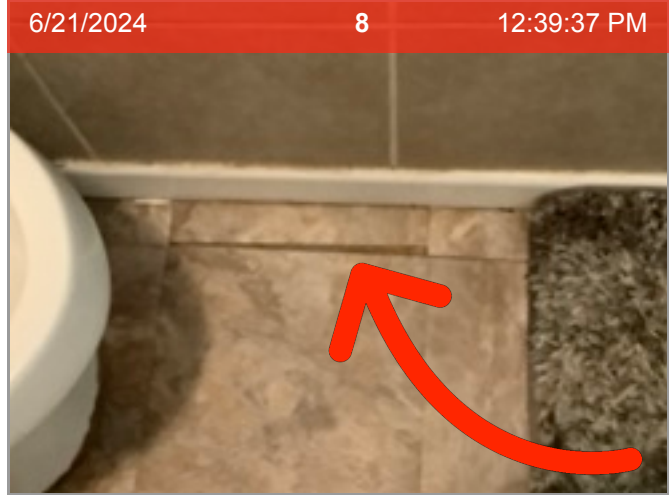
Floors | Gap in flooring.
