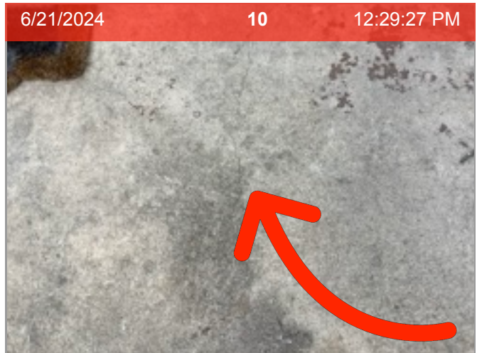
Patio/Porch | Cracks in concrete; damage ; discoloration
