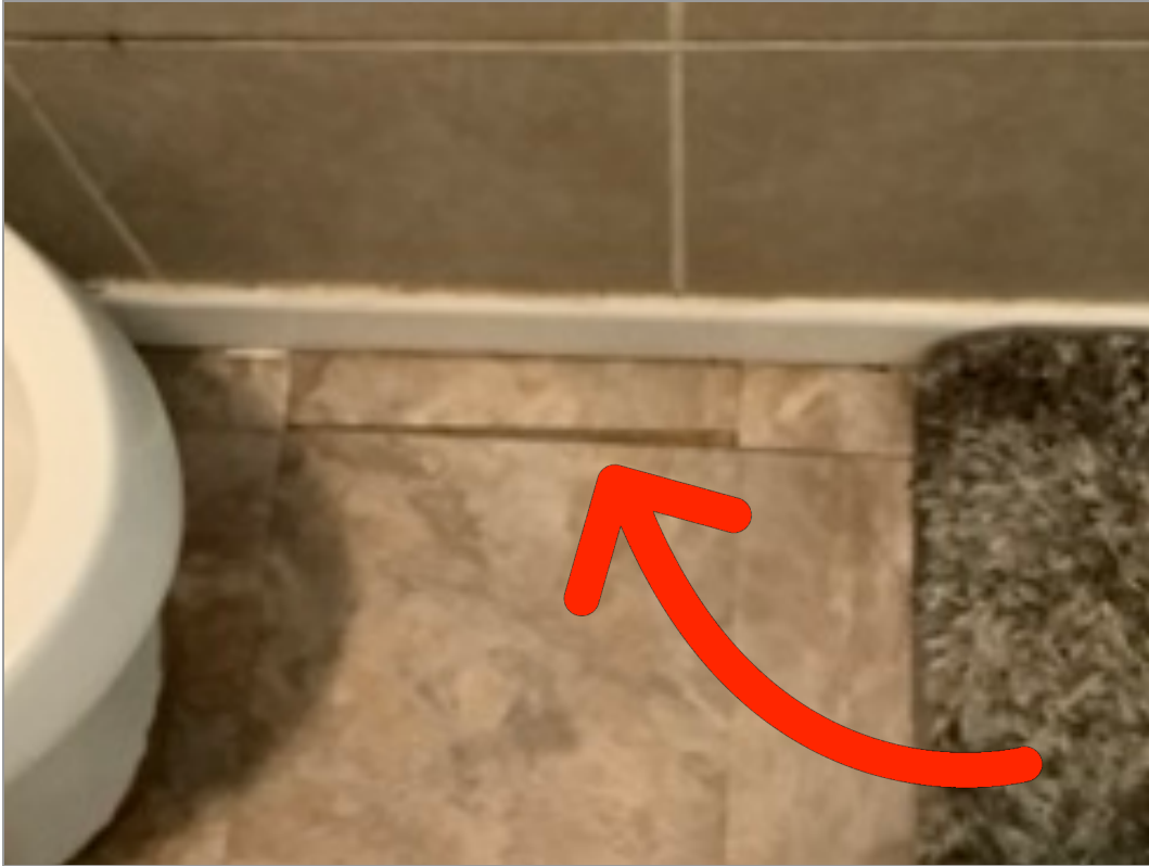
Bathroom 1 Floors Gap in flooring.
