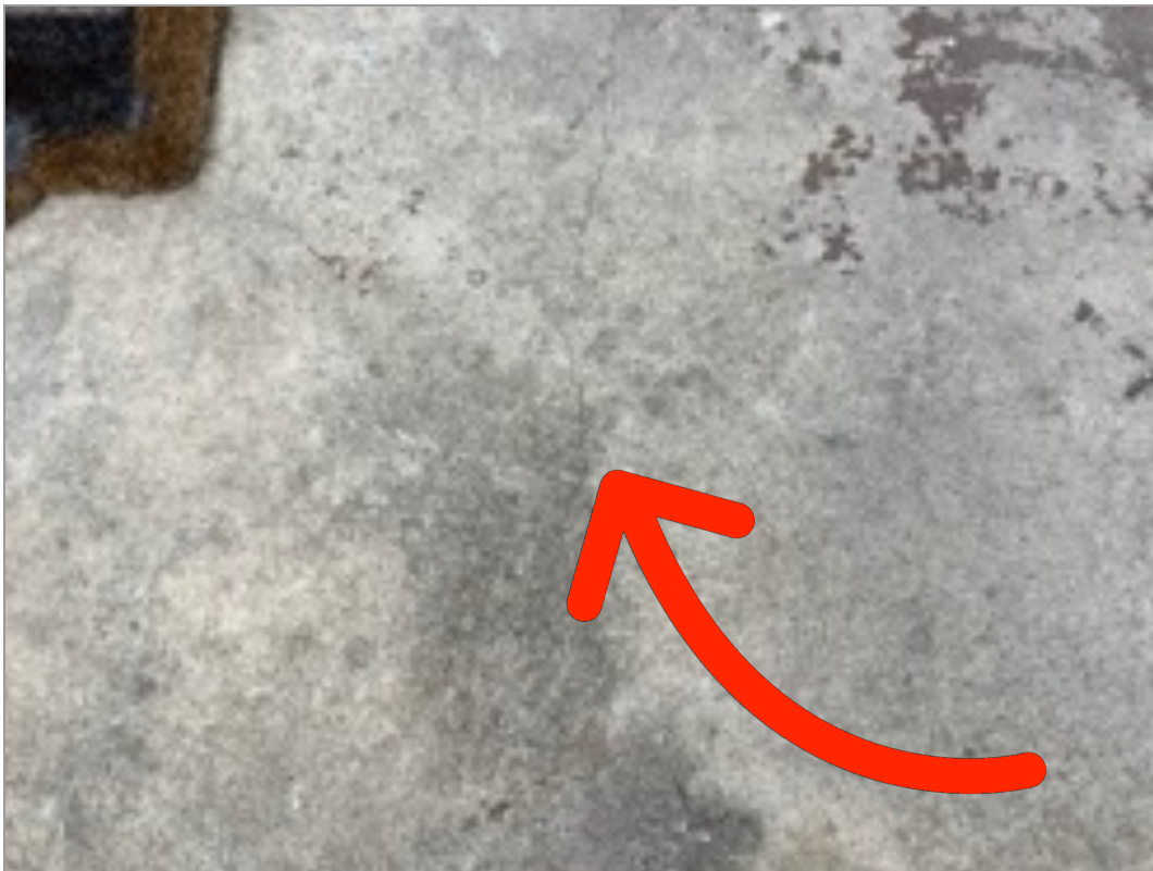
Entry Patio/Porch Cracks in concrete; damage ; discoloration
