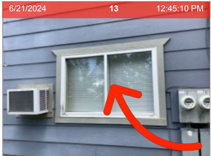
Window Screens | Screen(s) are missing
