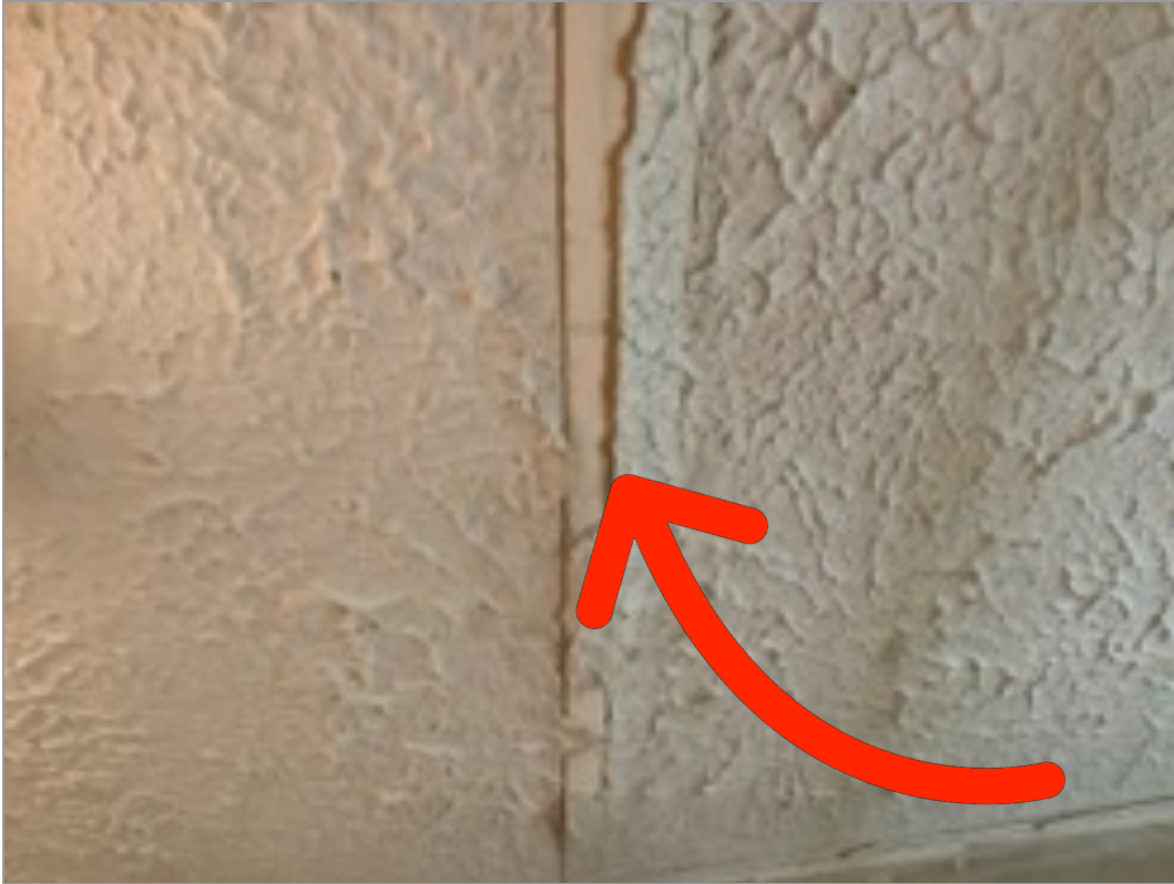
Bathroom 1 Ceiling Cracks in ceiling.
