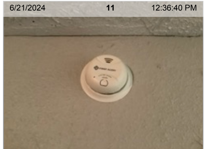
Wireless Smoke Alarm (mfd 3/2022) | Smoke test: Passed | Alarm in place
