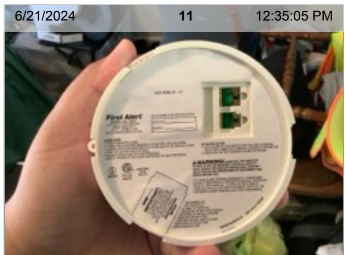
Wireless Smoke Alarm (mfd 3/2022) | Smoke test: Passed | Close-up of printed manufacture date | 2.3 years old
