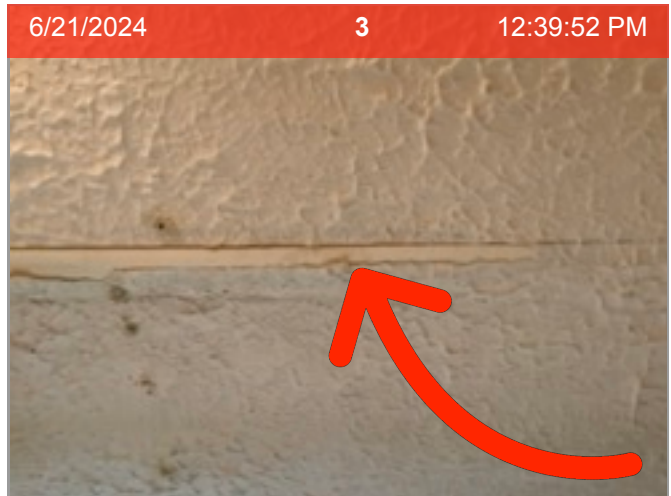
Ceiling | Cracks in ceiling.
