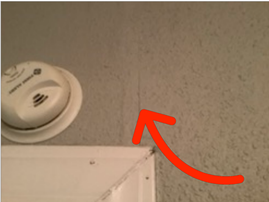
Bedroom 1 Walls/Paint Cracks in texture
