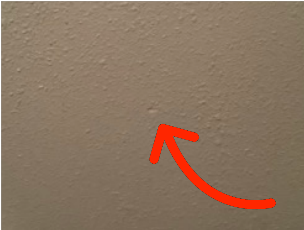
Bedroom 1 Door Stop Missing- wall damage noted.
