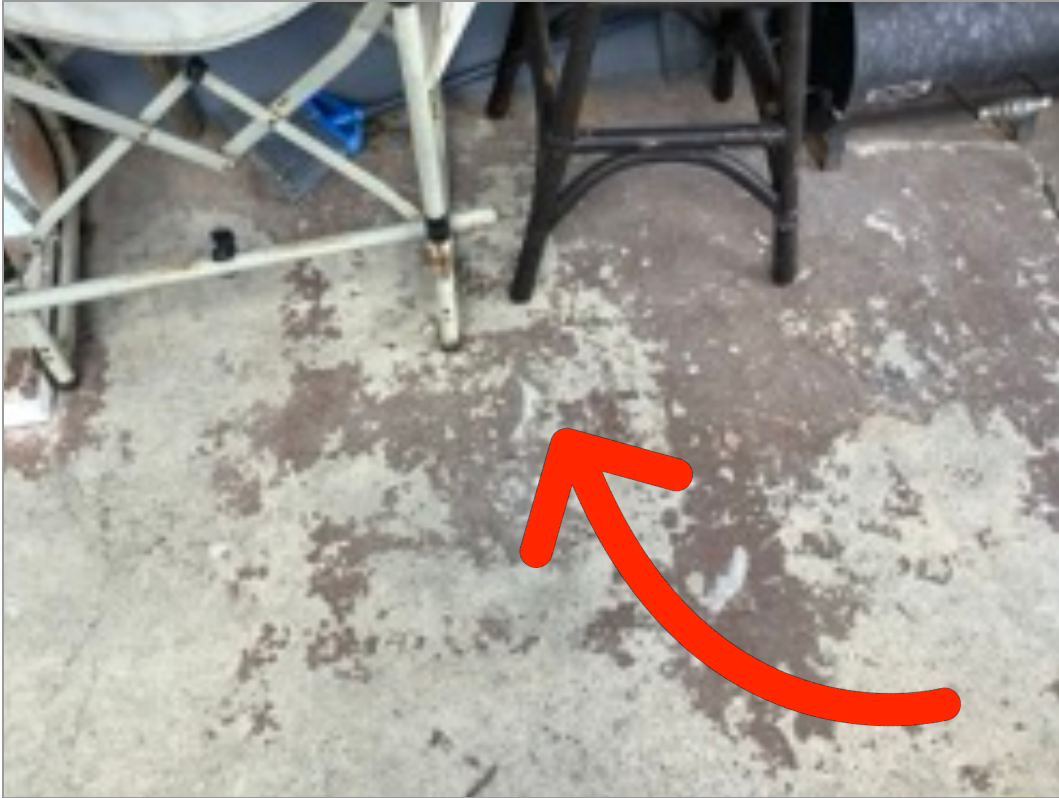
Entry Patio/Porch Cracks in concrete; damage ; discoloration
