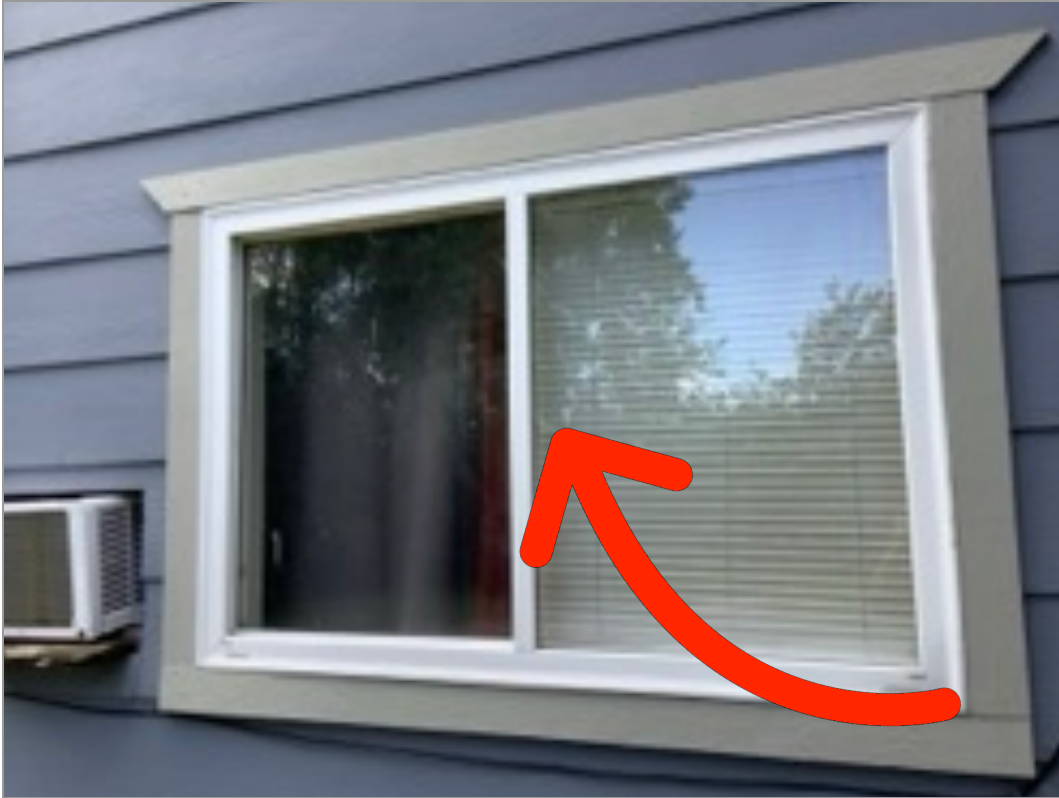
Front Exterior Window Screens Screen(s) are missing
