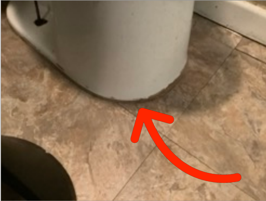
Bathroom 1 Commode Seal around bottom of commode is cracking/ discolored.
