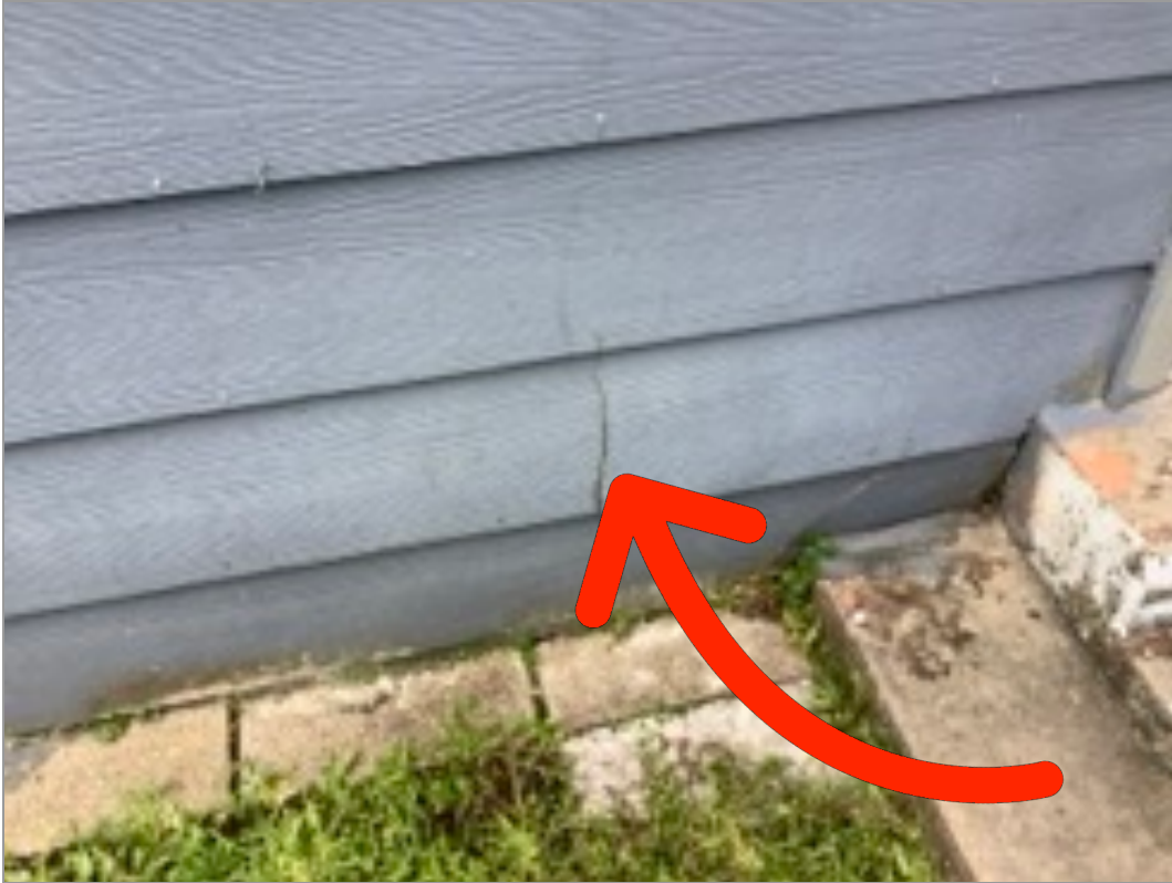
Front Exterior Walls/Siding/Trim Siding warping/pulling away
