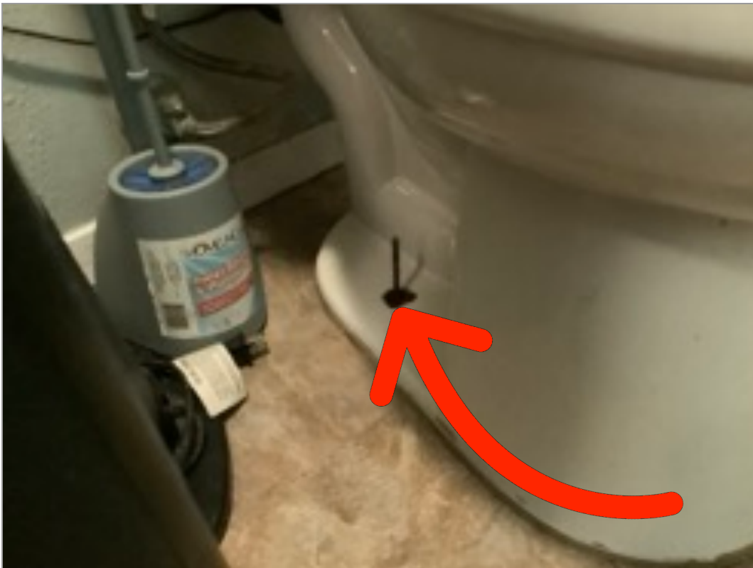
Bathroom 1 Commode Bolt caps missing
