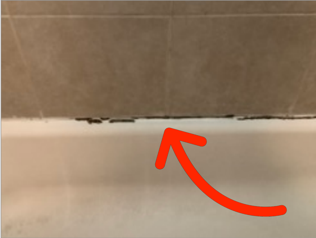
Bathroom 1 Tub/Fixture Grout is discolored/cracking
