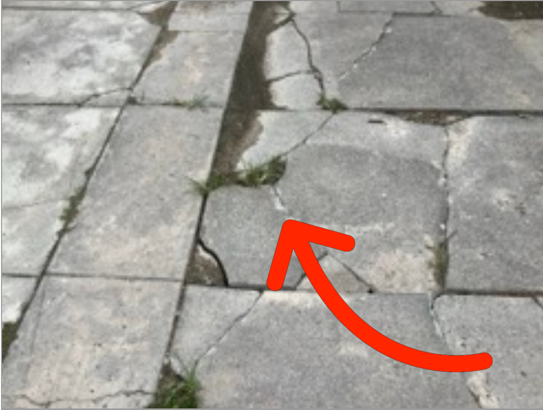
Front Exterior Driveway Spider cracks in driveway.
