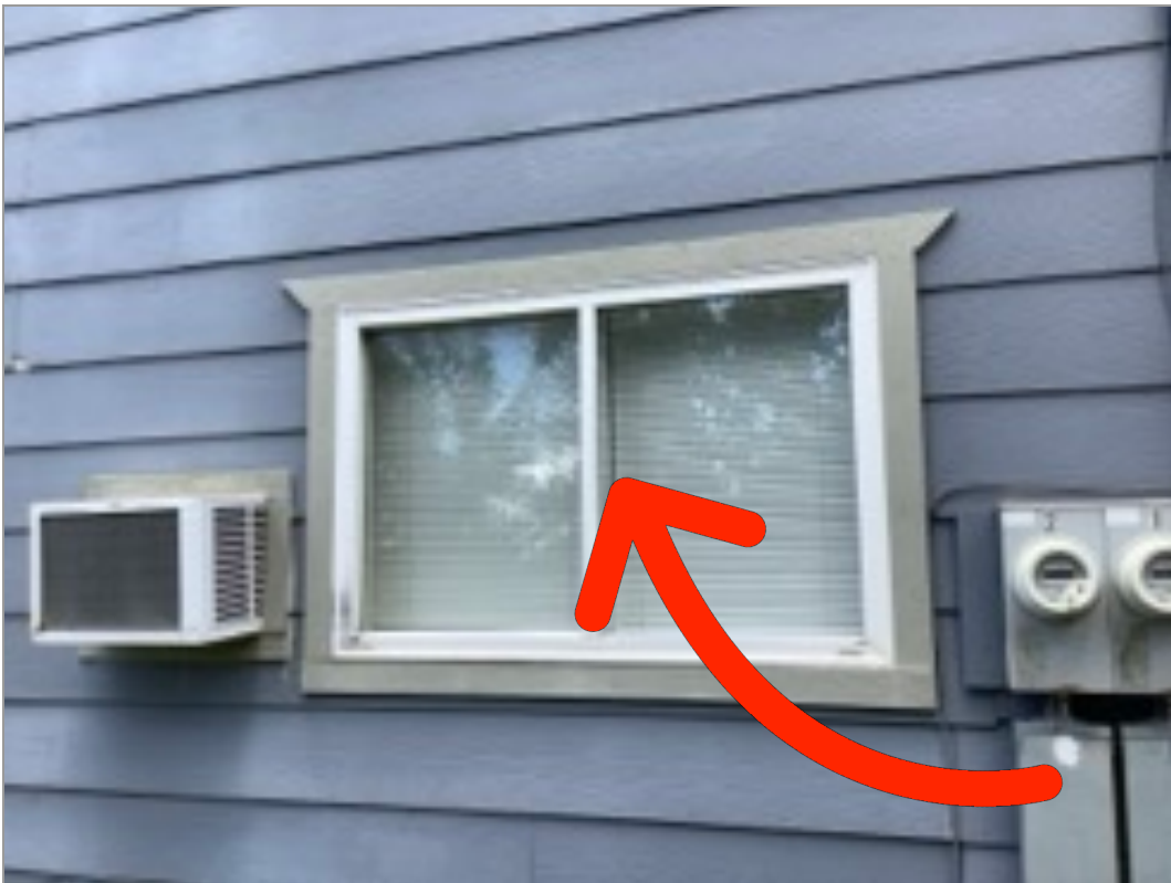
Front Exterior Window Screens Screen(s) are missing
