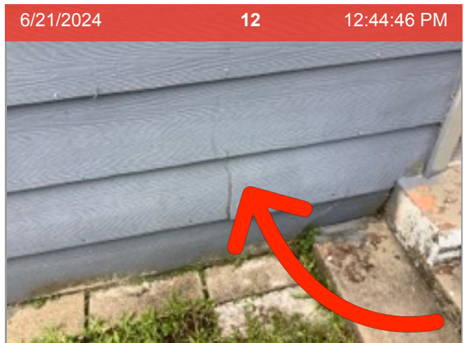
Walls/Siding/Trim | Cracked/peeling paint
