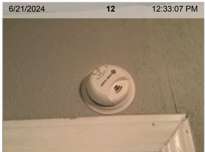
Wireless Smoke Alarm (mfd 5/2022) | Smoke test: Passed | Alarm in place
