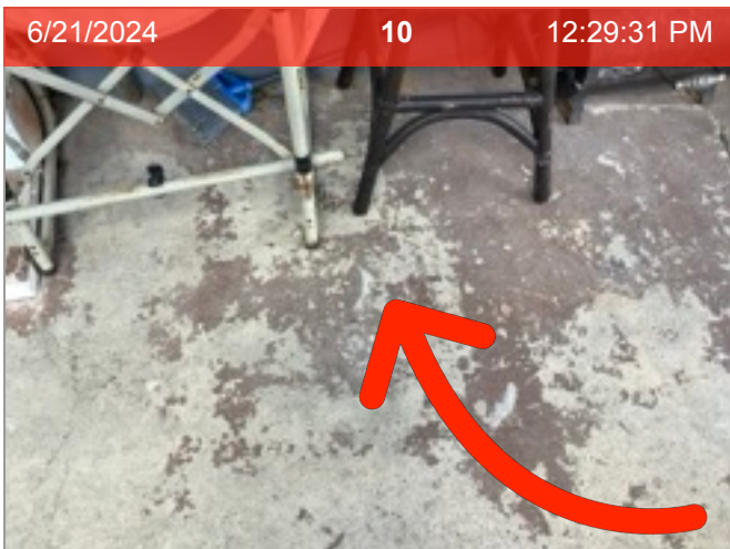
Patio/Porch | Cracks in concrete; damage ; discoloration
