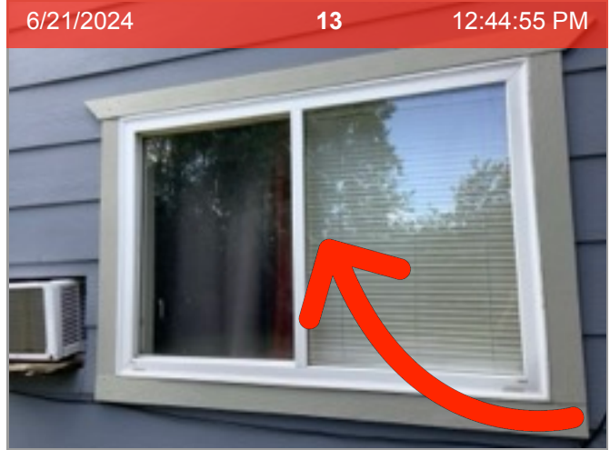
Window Screens | Screen(s) are missing
