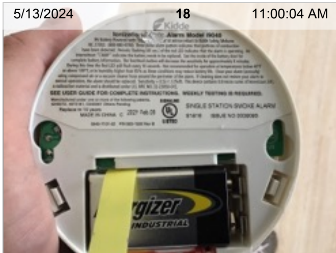
Wireless Smoke Alarm (mfd 2/2021) | Smoke test: Passed | Close-up of printed manufacture date | 3.3 years old
