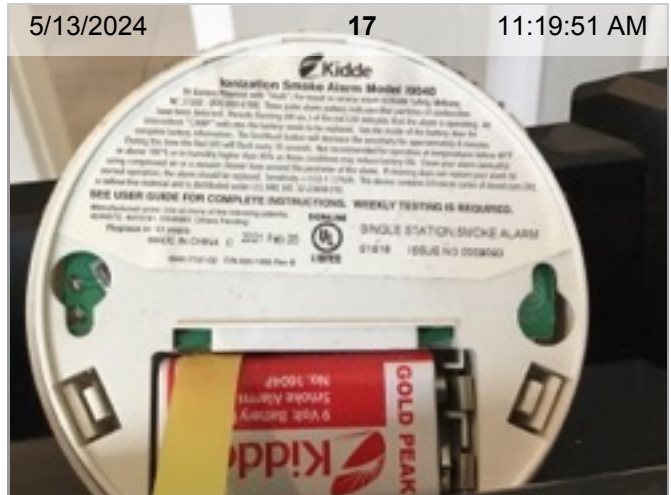
Wireless Smoke Alarm (mfd 2/2021) | Smoke test: Passed | Close-up of printed manufacture date | 3.3 years old
