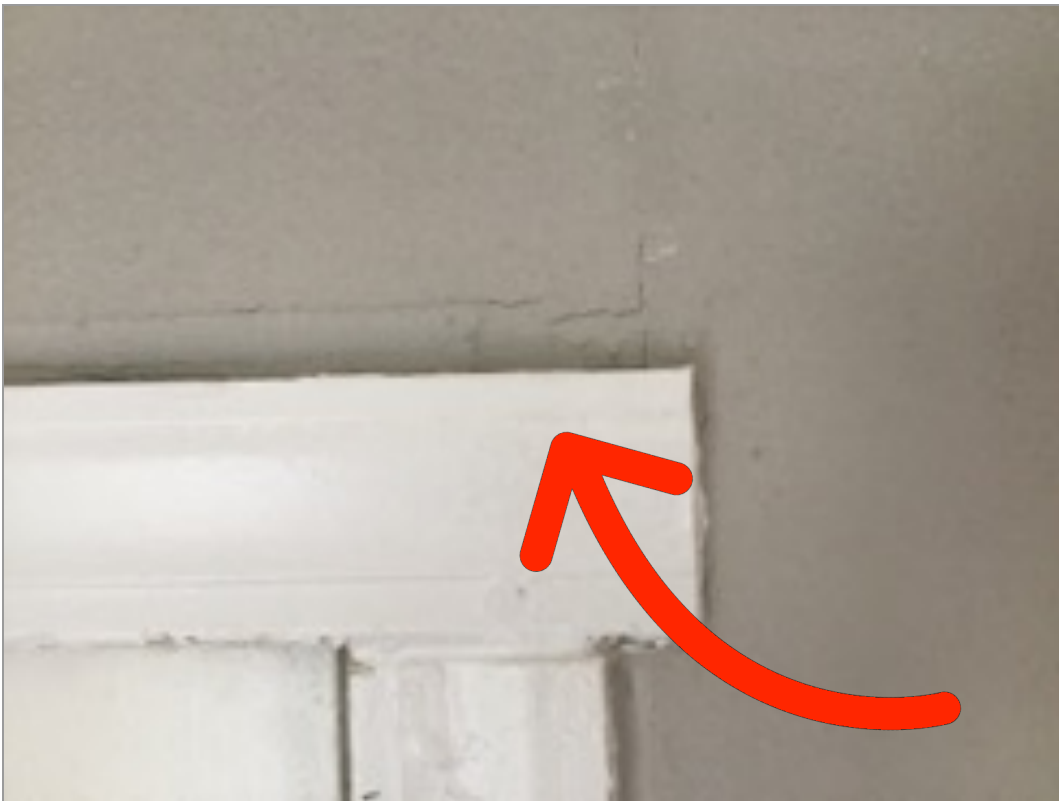
Entry Walls/Paint Cracks in texture
