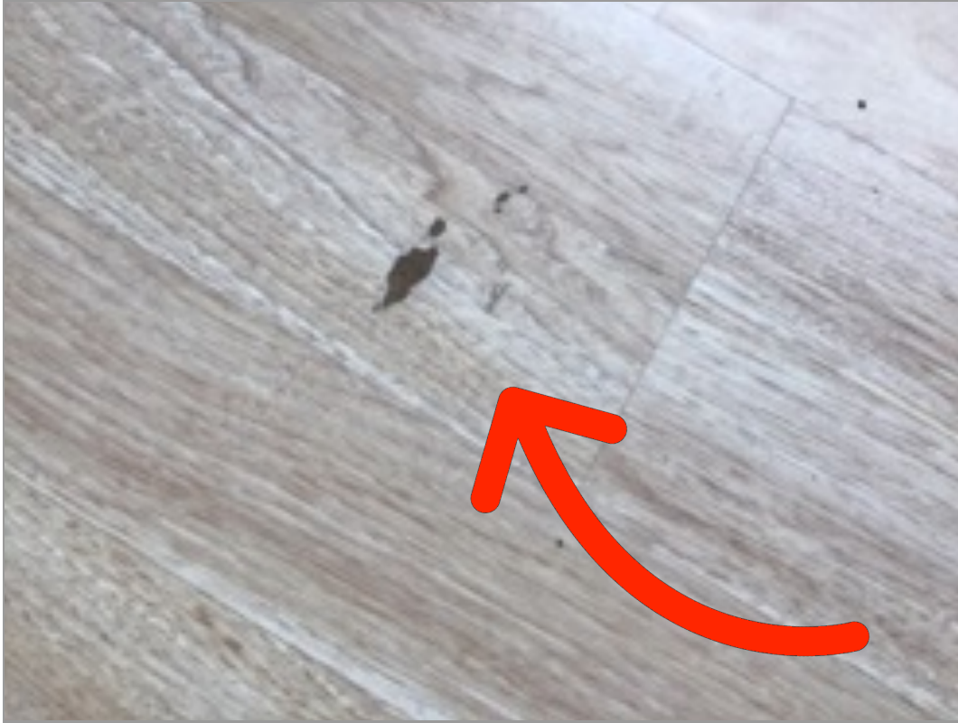
Bedroom 1 Floors Flooring is scratched.
