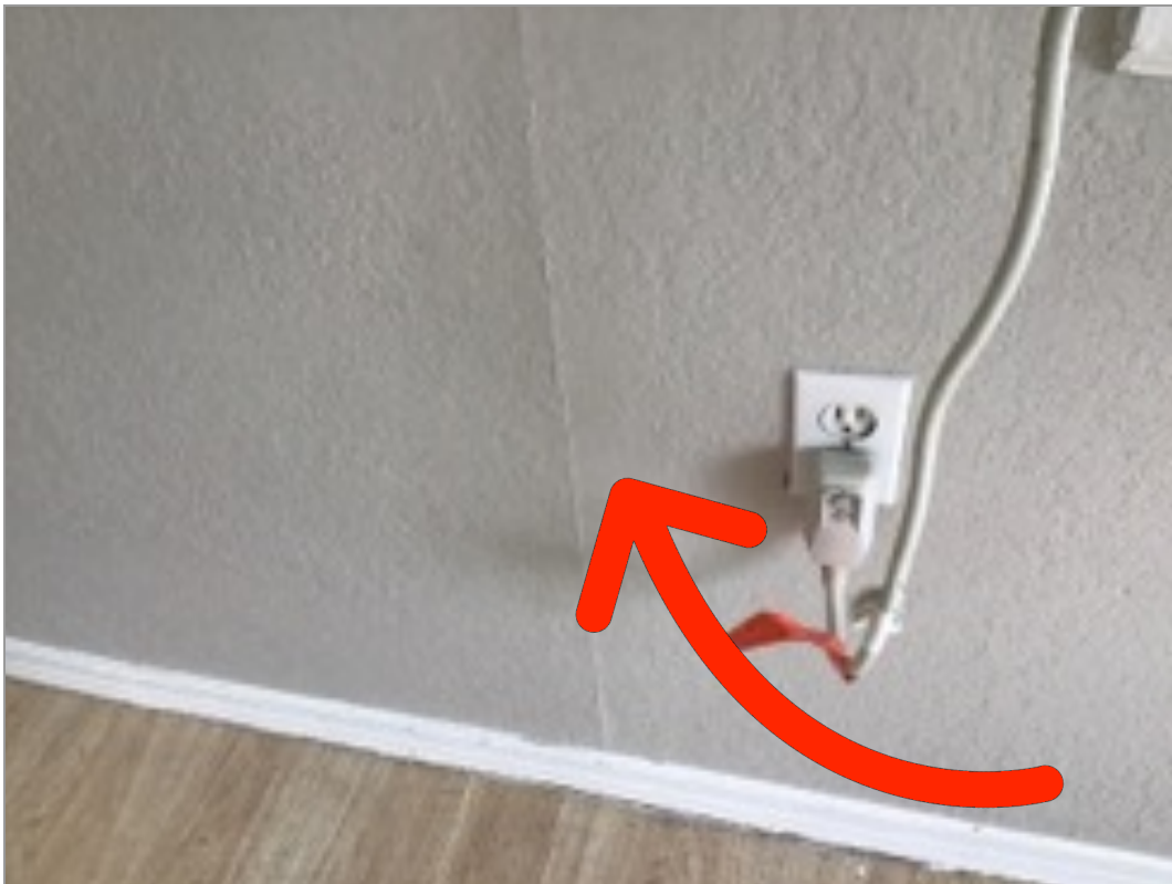
Living Room Walls/Paint Cracks in texture
