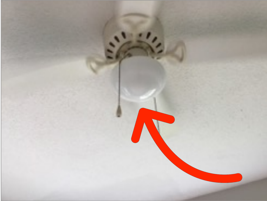
Living Room Light Fixtures Light did not turn on.
