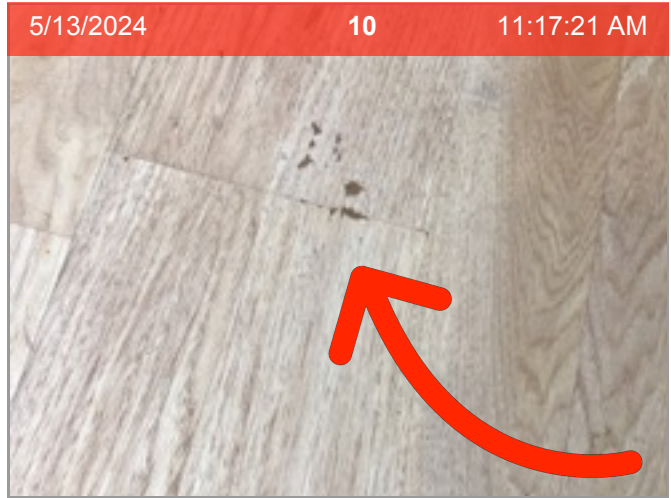
Floors | Flooring is scratched.
