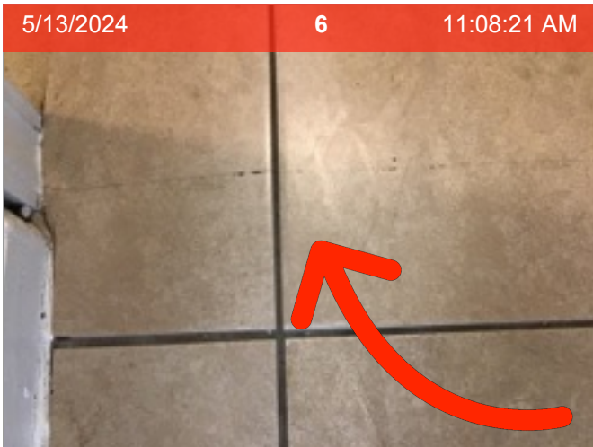
Floors | Crack in flooring.
