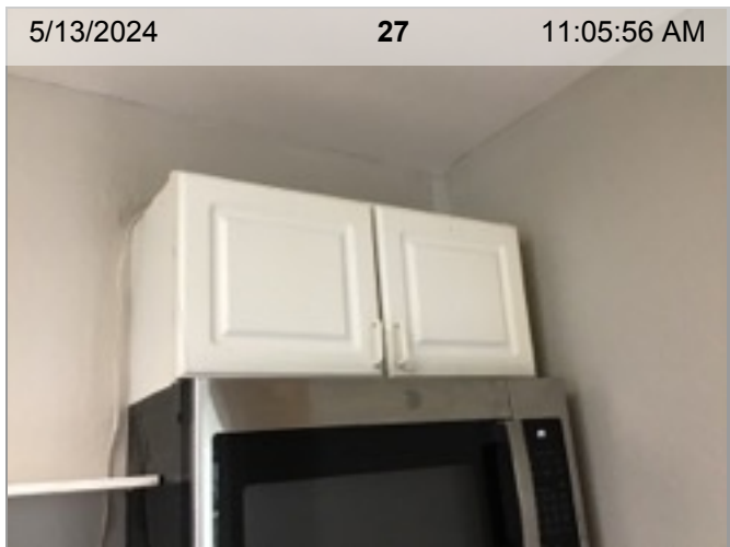
Upper Cabinets - Exterior
