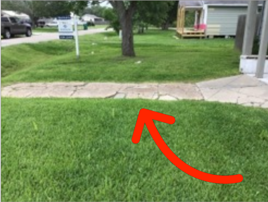
Front Exterior Walkways Cracked or uneven
