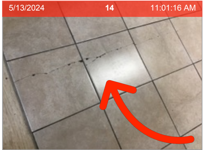
Floors | Crack in flooring.
