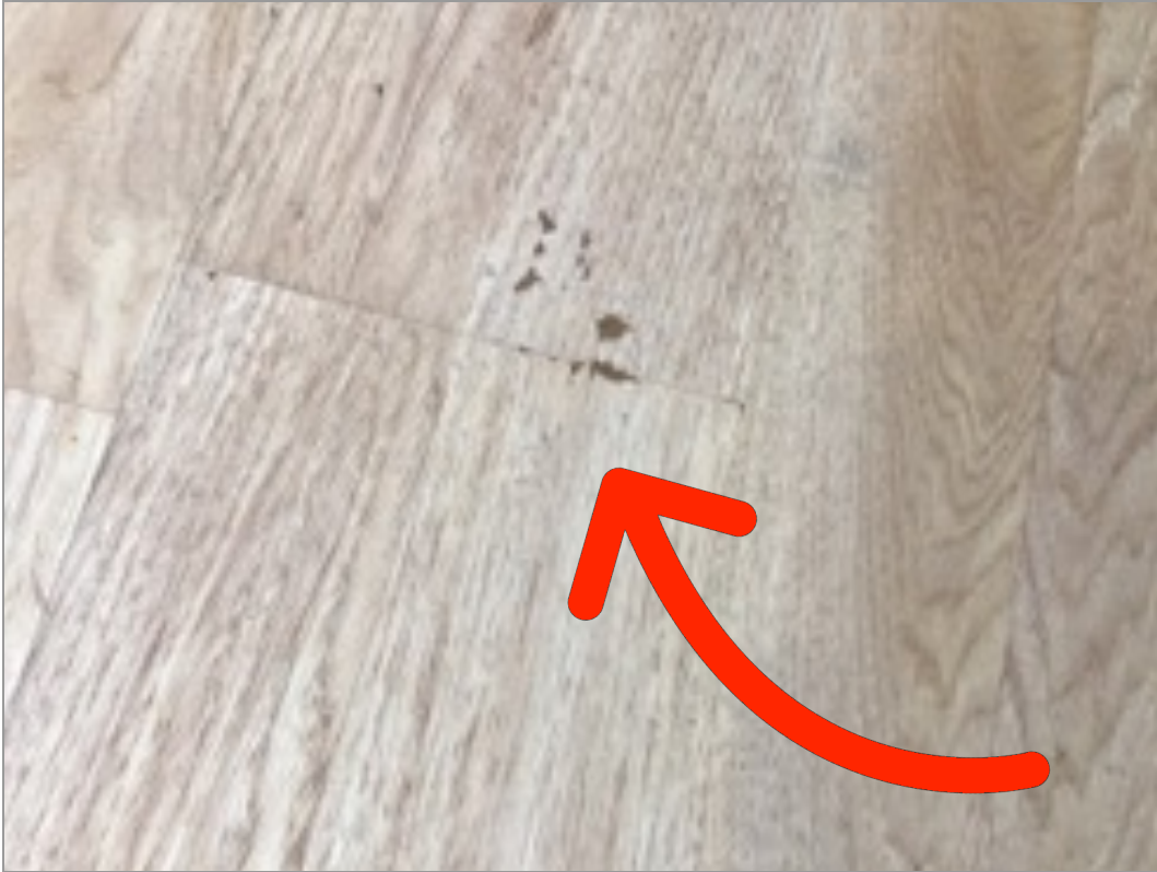
Bedroom 2 Floors Flooring is scratched.
