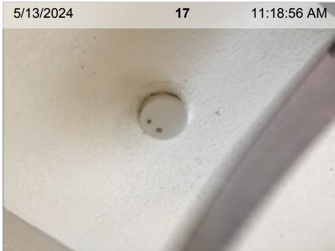
Wireless Smoke Alarm (mfd 2/2021) | Smoke test: Passed | Alarm in place
