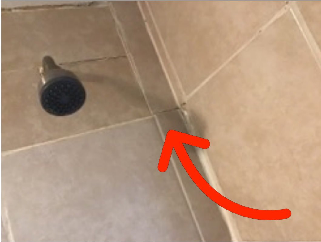
Bathroom 1 Shower/Fixture Grout is dicolored/cracking.
