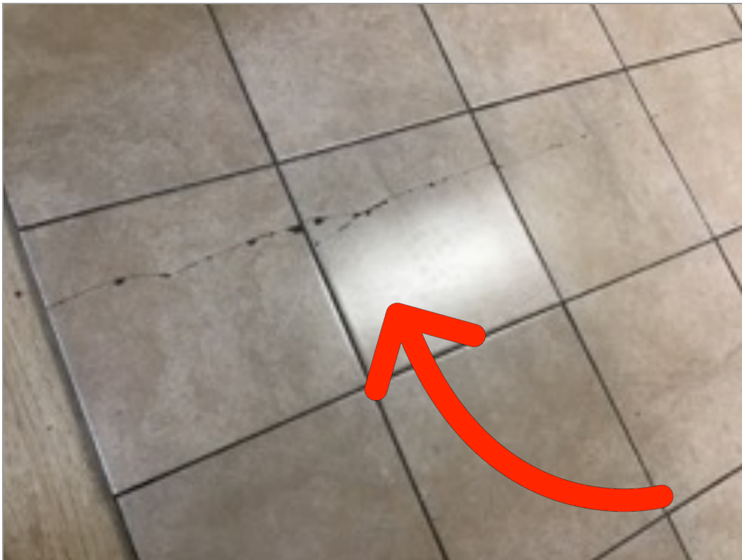
Kitchen Floors Crack in flooring.
