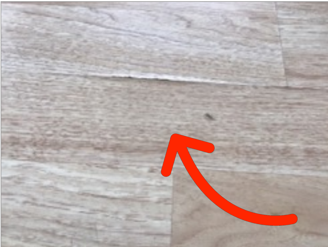
Living Room Floors Crack in flooring.
