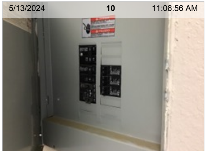
Electrical Breaker Panel
