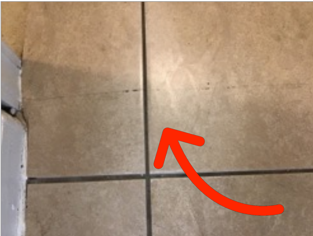
Hallway/Stairway Floors Crack in flooring.
