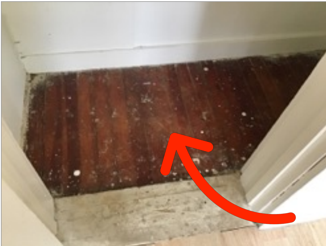
Bedroom 1 Closets Stains on flooring
