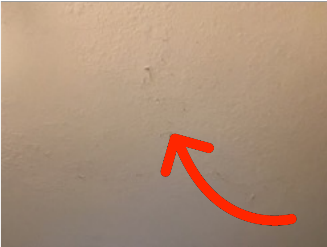
Bathroom 1 Ceiling Cracks in ceiling.
