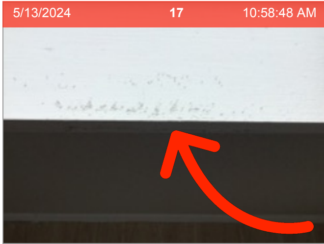
Windows | The window sill is cracking
