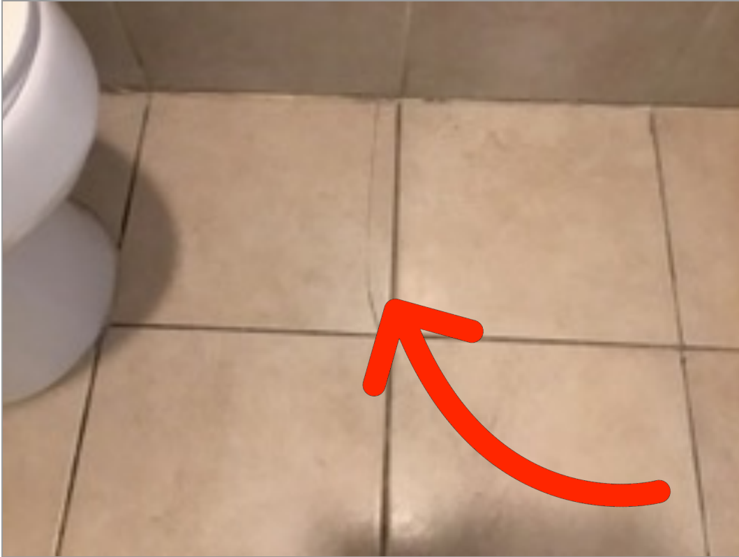
Bathroom 1 Floors Crack in flooring.
