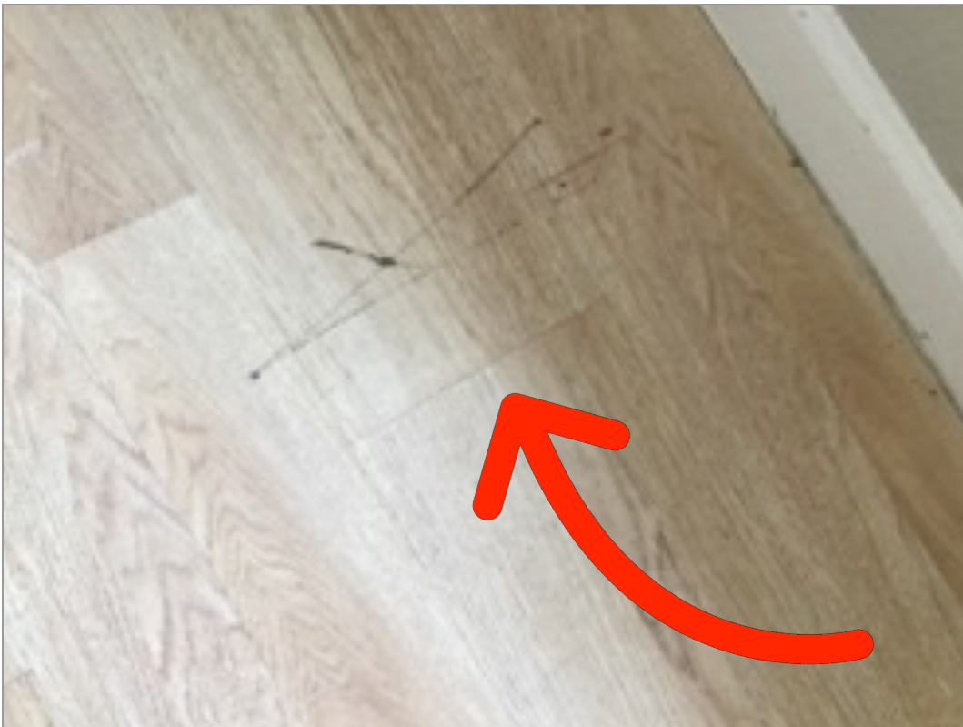
Bedroom 2 Floors Flooring is scratched.
