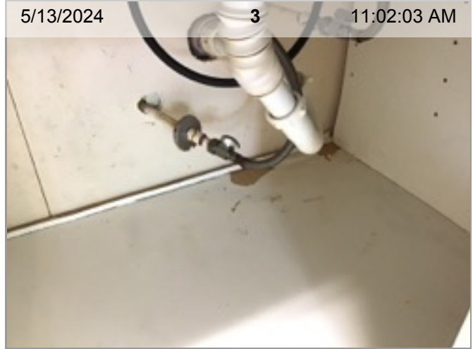
Cabinet Under Sink
