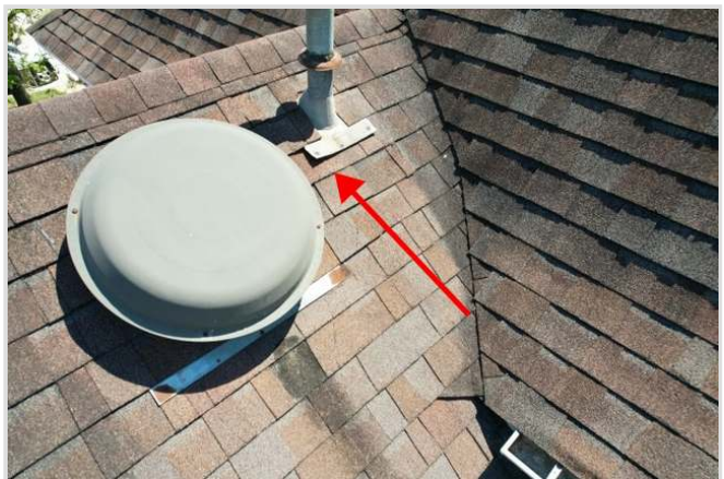
Lifted flashing - water heater flue
