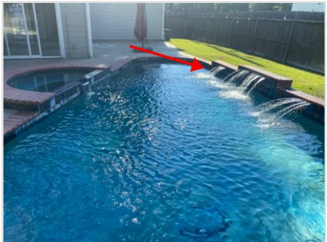
Water feature pump functioning
