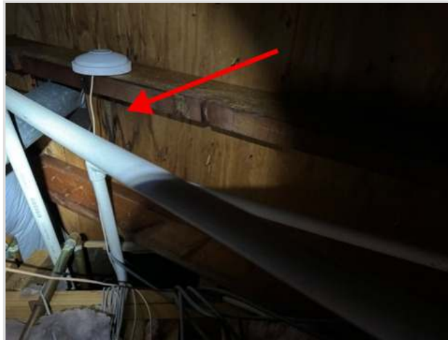
Indications of prior water penetration around the water heater flue
