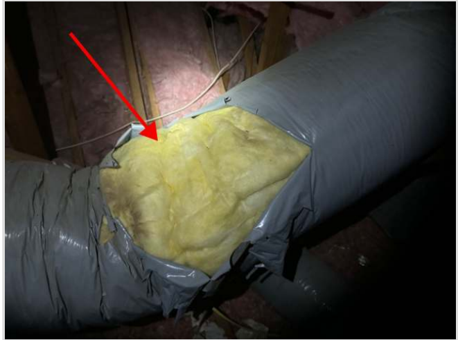
Damaged HVAC duct covering in the upper attic
