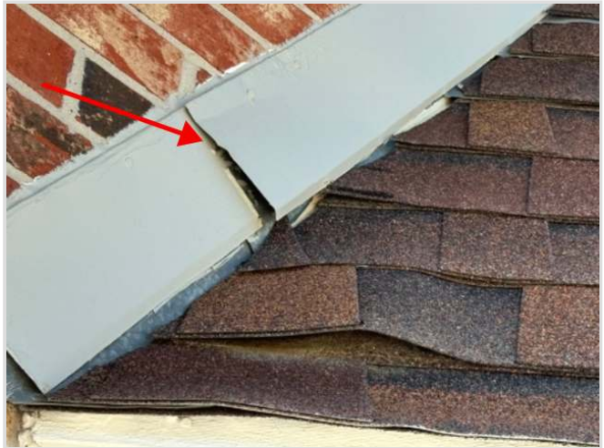
Loose counter-flashing on front wall
