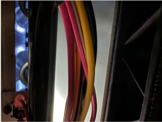
Unit #1: Furnace burners functioning
