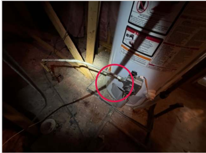
No sediment trap on the gas line to the water heater
