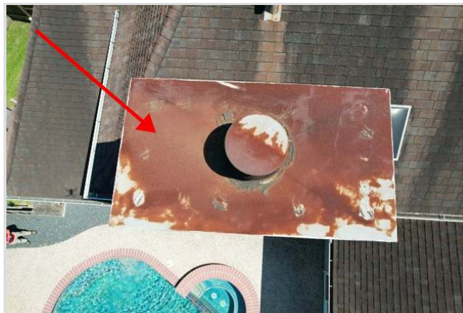
Rusted chimney top
