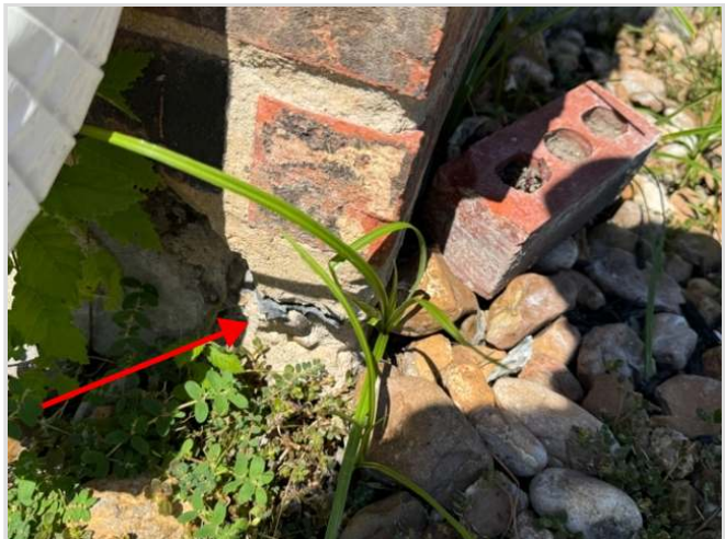
Deterioration of exterior beam - left front corner
