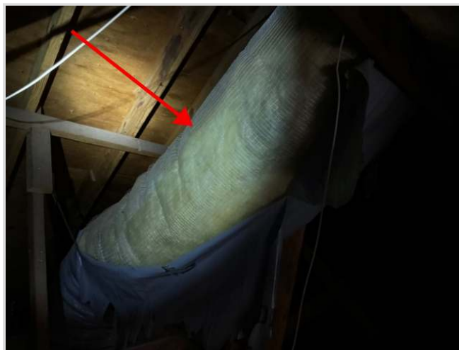
Damaged HVAC duct cover in the second floor right side attic
