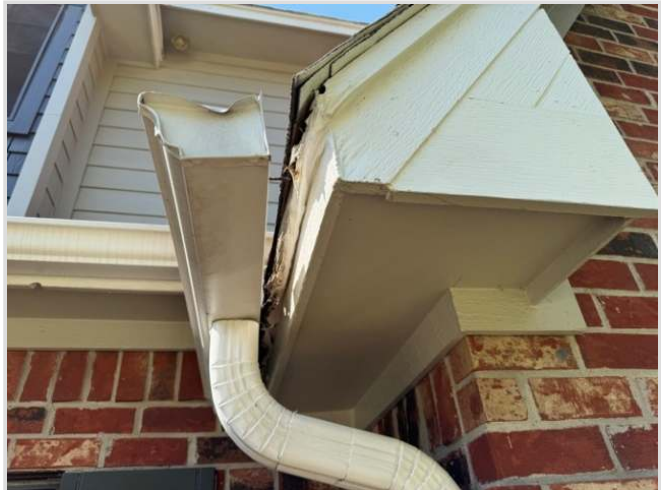
Gutter not secured to front wall
