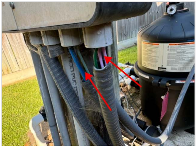
Conduit detached at ends exposing wire
