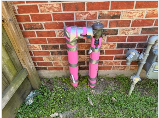
Backflow prevention valve
