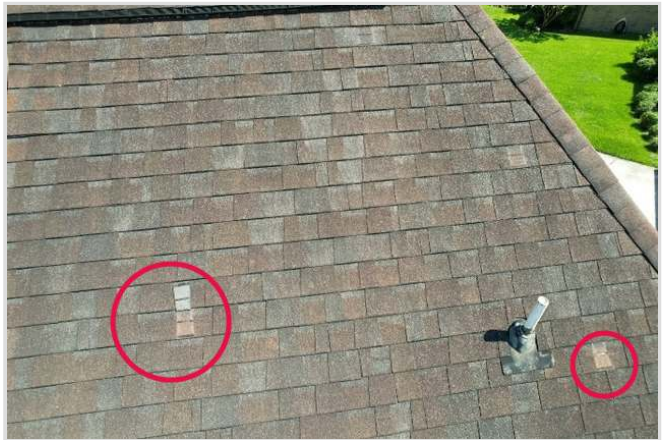
Damaged shingles on the rear left slope
