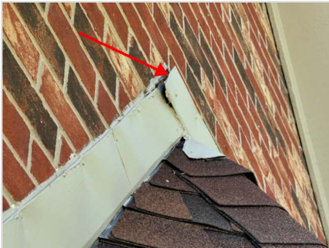
Loose counter flashing on front wall
