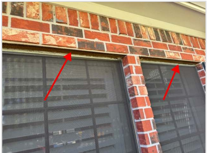
Rusted lintels - front wall
