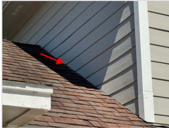
Siding in contact with adjacent shingles
