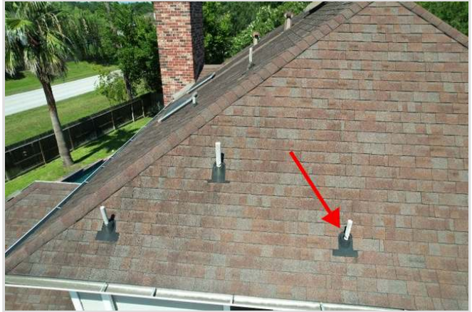
Deteriorated seal - left side
