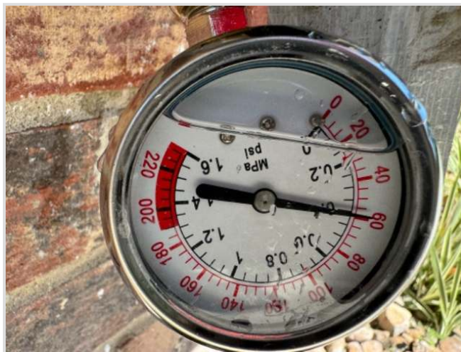
Water pressure reading
