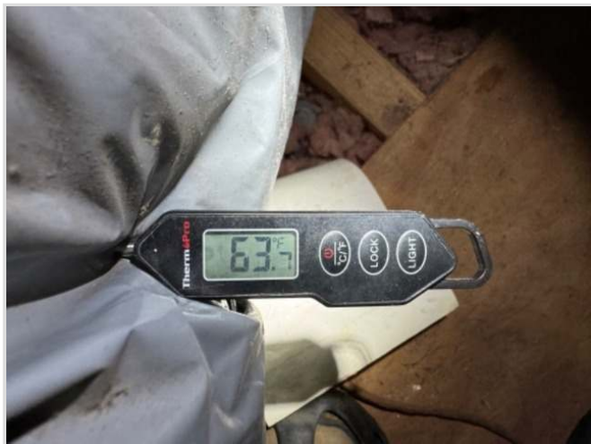
Unit #1: Supply air temperature
