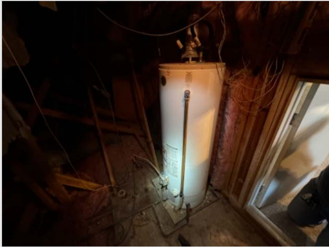
Water heater in attic
