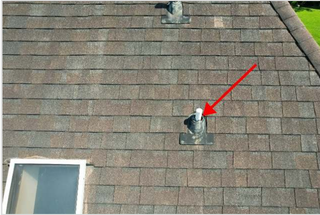
Deteriorated seal - rear slope
