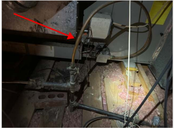
Copper gas line pipe to Unit #2
