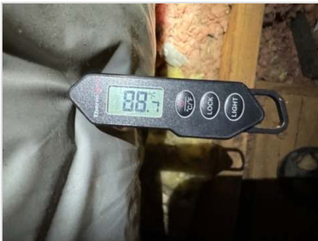
Unit #1: Return air temperature
