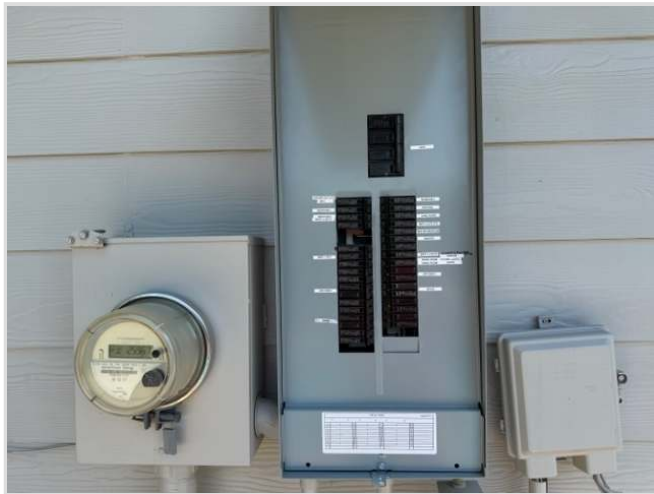
Main electric panel
