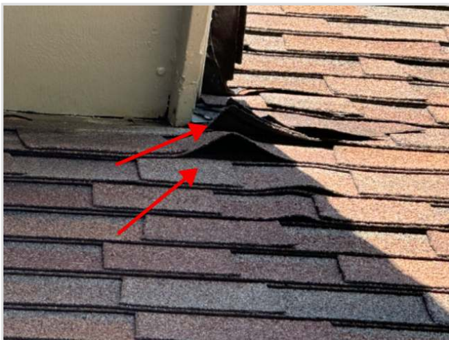
Lifted shingles - right side slope over left gable
