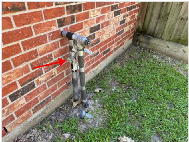
Main water valve
