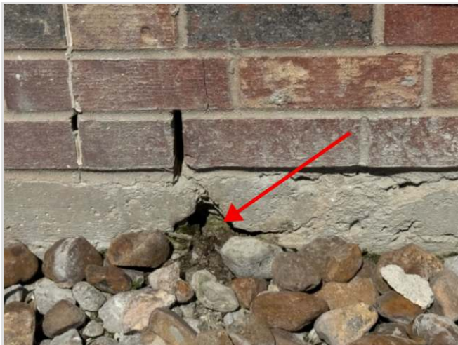
Void in left exterior beam
