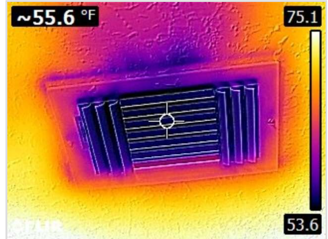
Unit #2: Supply air temperature
