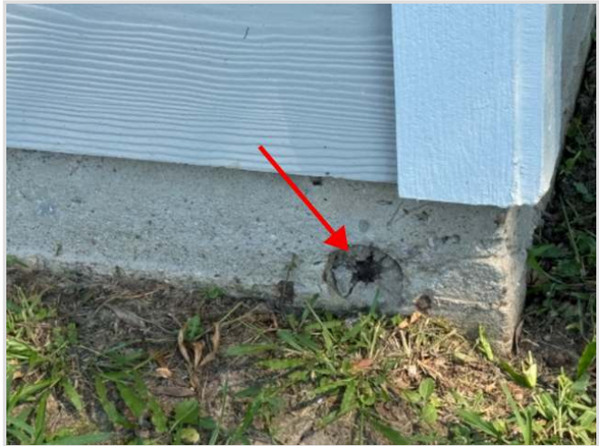
Post-tension end not protected on garage rear wall
