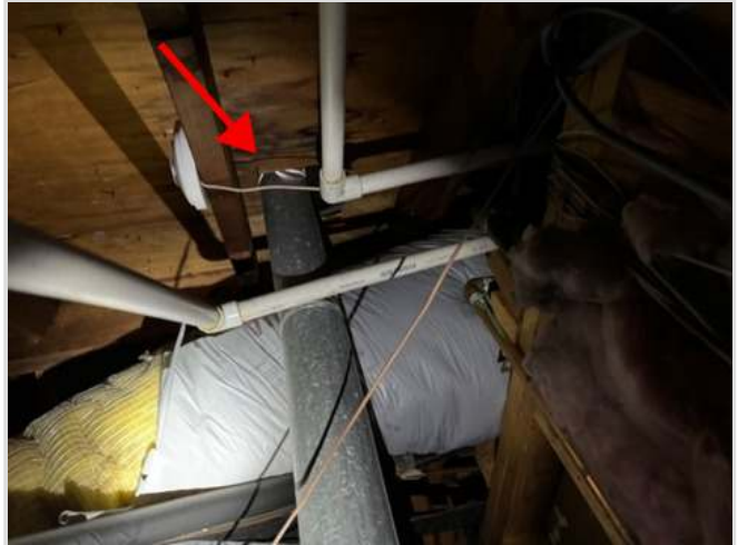
Flue pipe in contact with roof decking
