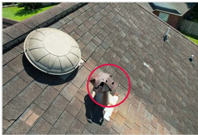
Vent cap rusted through (flue cap for one of the furnaces)
