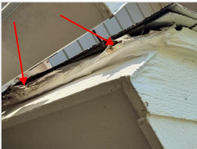
Wood damage at the right side gable on the front wall
