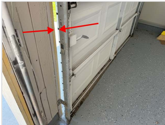
Large gap - right side of left overhead garage door
