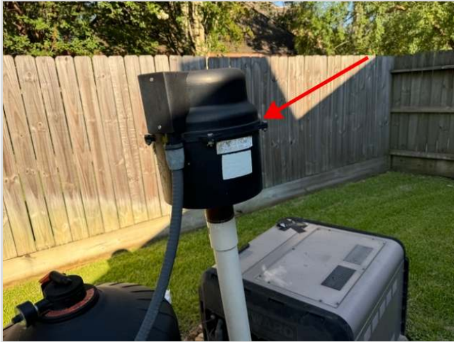
Blower motor did not appear to be functioning
