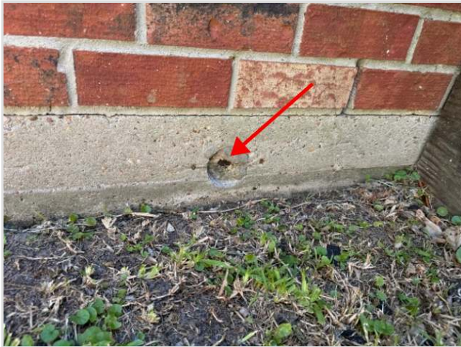
Post-tension end not protected on right side
