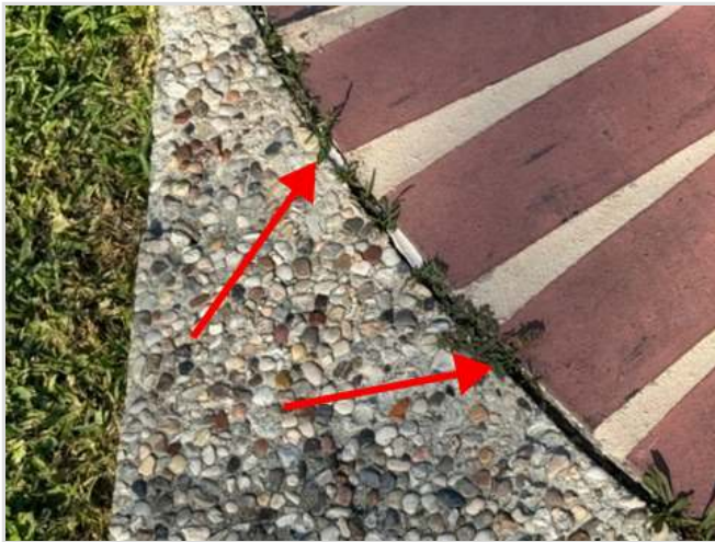
Gap in sealant between coping and deck
