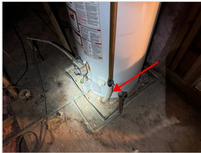
TPR discharge pipe did not terminate to the exterior
