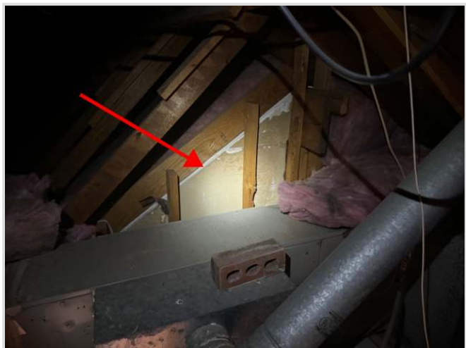
Fallen vertical insulation
