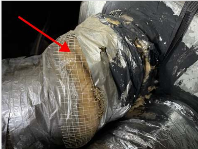
Damage HVAC duct covering above the garage
