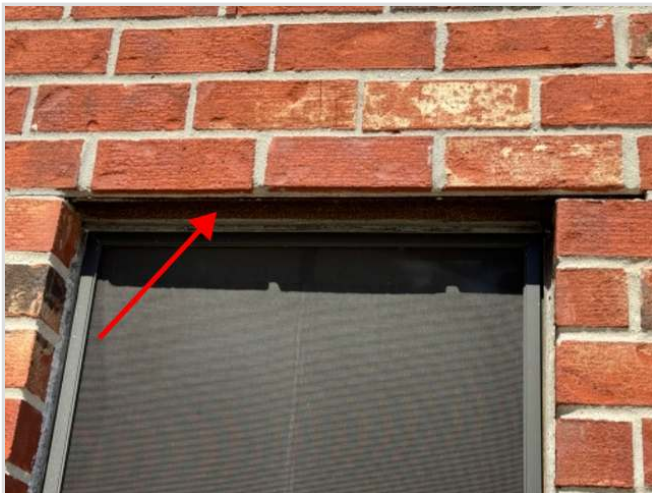
Rusted lintel - left side
