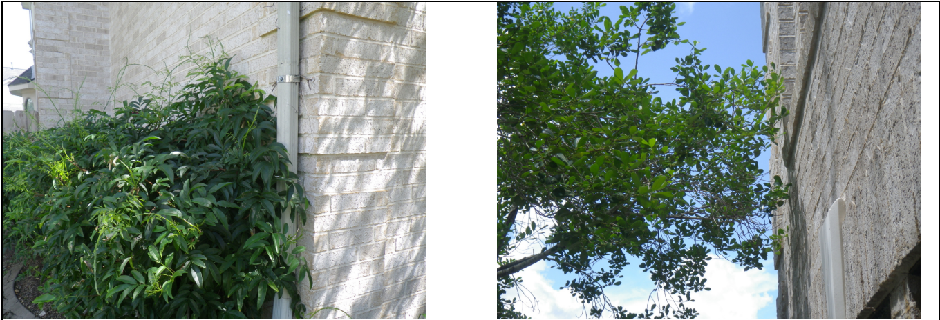
Pictures of shrub and tree limbs growing and or touching exterior walls.
