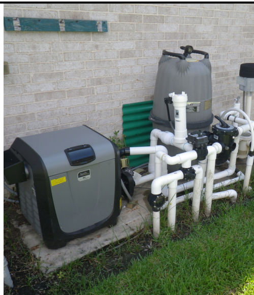
Picture of Pump Equipment
