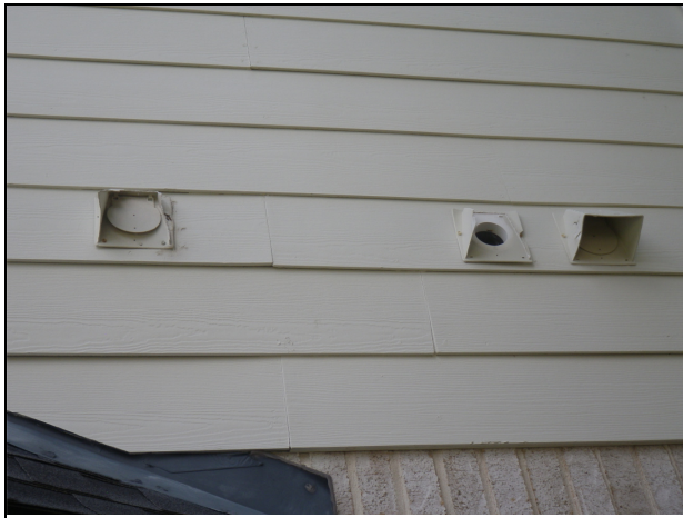
Picture of damaged exterior vent housings observed at
