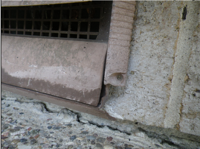
Picture of damaged louvered vent opening for
