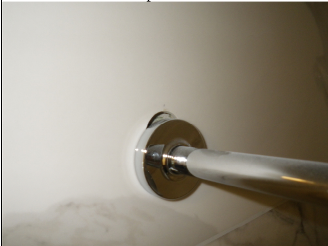
Picture of opening above shower head in tub/shower enclosure at upstairs east side guest bathroom.
