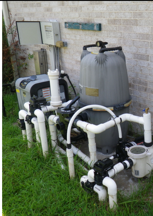
Picture of Pump Equipment
