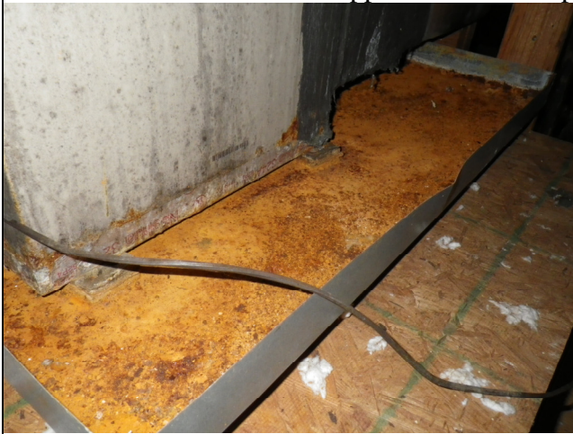
Picture of corrosion observed in safety pan under
