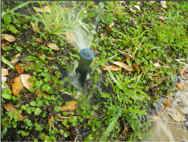
Picture of water bubbling up around base of pop up spray head in zone 2.
