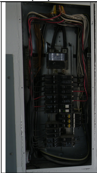
Picture of Main Breaker Box
