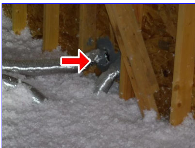
F. Item 1(Picture) Disconnected vent fan duct
