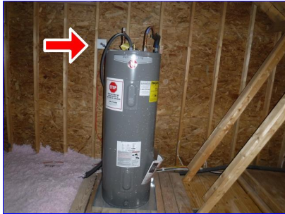
C. Item 1(Picture) Water heater located in attic
