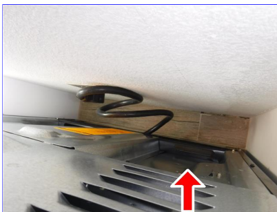
D. Item 1(Picture) Missing anti tip device
