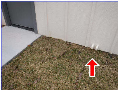
C. Item 3(Picture) Pan and T&P valve drain lines right side
