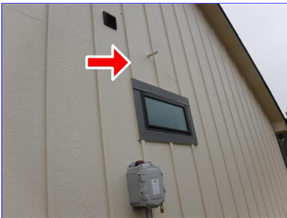
A. Item 3(Picture) Pan drain left gable
