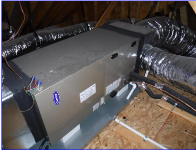
A. Item 2(Picture) Heater / air handler
