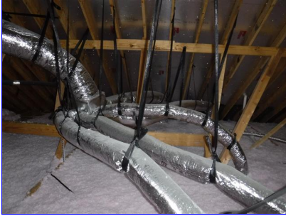
C. Item 1(Picture) Ducts supported and sealed as needed
