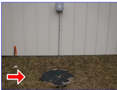
E. Item 1(Picture) Grinder lift pump left side
