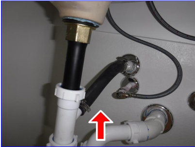
A. Item 1(Picture) Primary drain line guest bathroom sink trap
