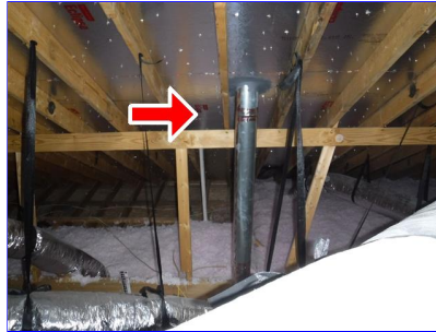
E. Item 2(Picture) Vented through roof
