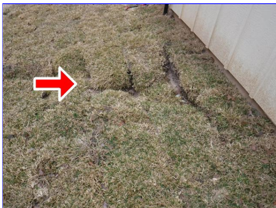
B. Item 3(Picture) Ground settlement right side at electric
