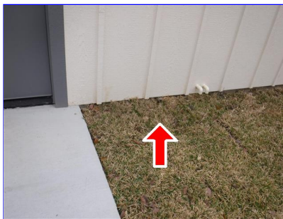
B. Item 2(Picture) High soil right side
