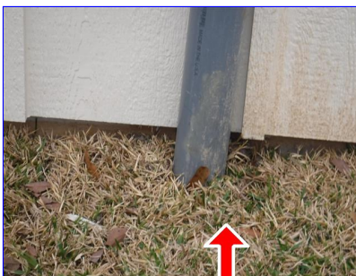
A. Item 4(Picture) Ground rod not visible
