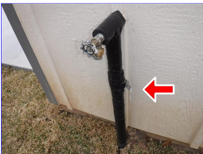
A. Item 1(Picture) Water shutoff right side
