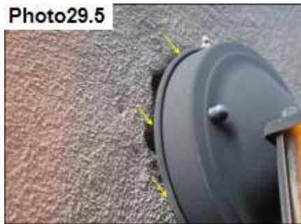
Penetration Sealants / Seal
