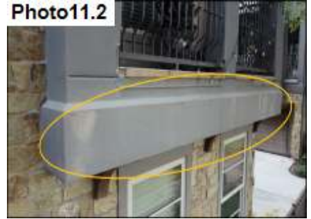
Efflorescence and Deteriorated Paint / Clean & Repaint
