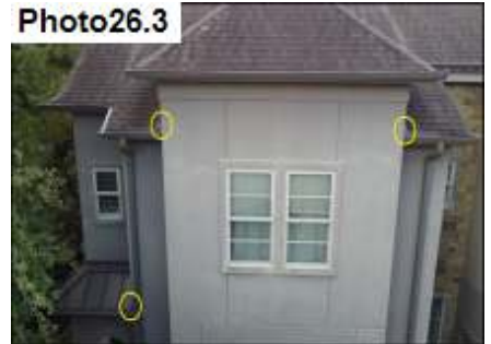
Kickout Flashing / Seal
