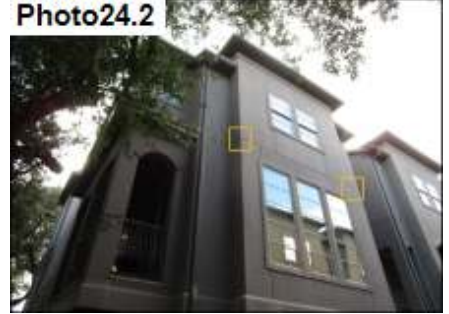
Control Joint Cracks / Repair
