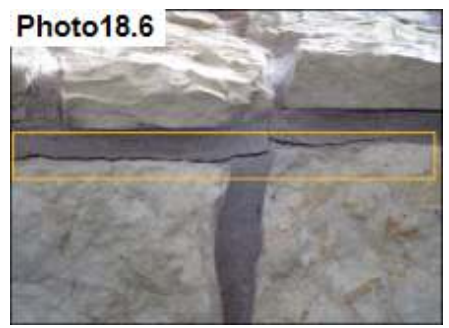
Deteriorated Mortar / Re-point
