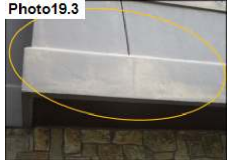
Efflorescence and Deteriorated Paint / Clean & Repaint
