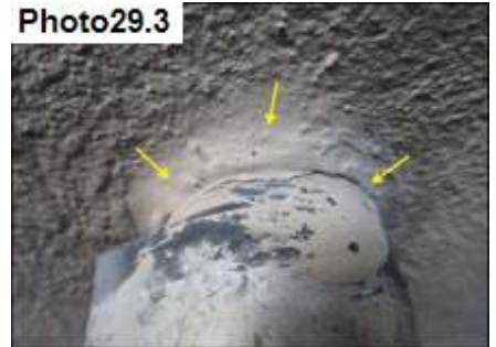
Penetration Sealants / Seal
