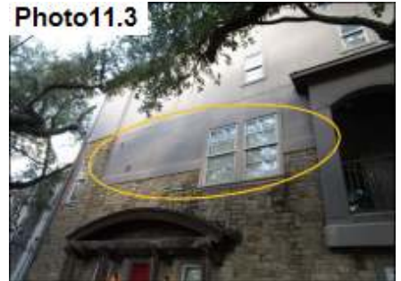
Efflorescence and Deteriorated Paint / Clean & Repaint
