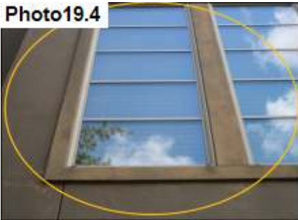
Efflorescence and Deteriorated Paint / Clean & Repaint
