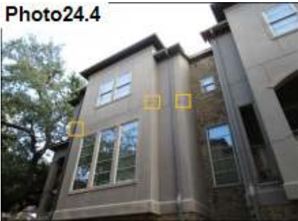
Control Joint Cracks / Repair
