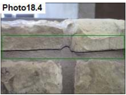
Deteriorated Mortar / Re-point
