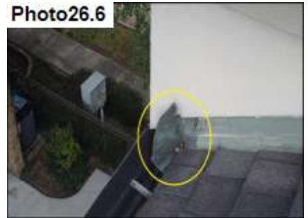
Kickout Flashing / Seal
