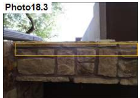
Deteriorated Mortar / Re-point
