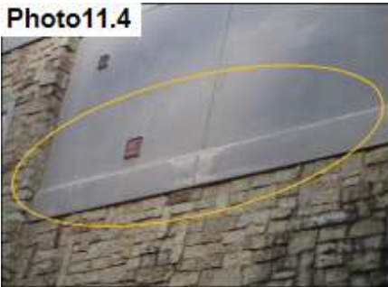
Efflorescence and Deteriorated Paint / Clean & Repaint
