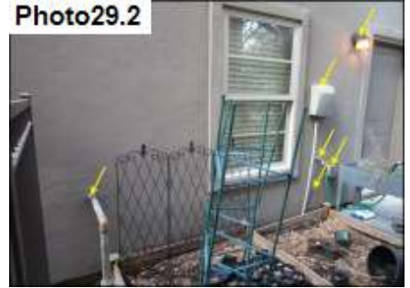
Penetration Sealants / Seal
