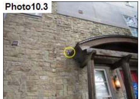
Kickout Flashing / Seal
