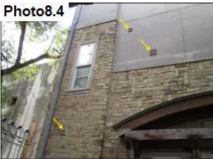
Penetration Sealants / Seal
