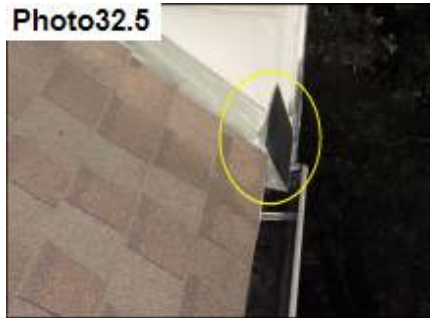
Kickout Flashing / Seal
