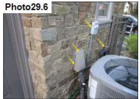
Penetration Sealants / Seal
