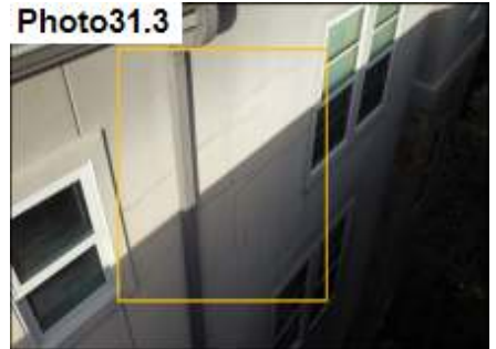
Crack Noted / Seal, Paint or Repair as Needed
