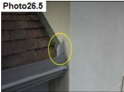
Kickout Flashing / Seal
