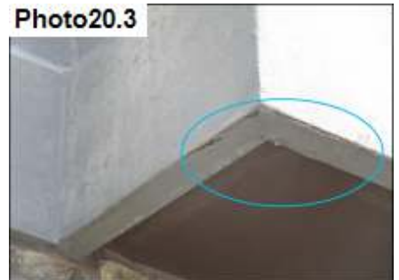
Broken & Rusted Casing Bead / Repair
