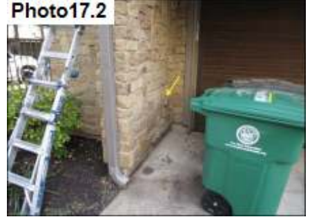
Penetration Sealants / Seal
