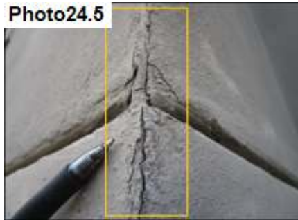
Control Joint Cracks / Repair
