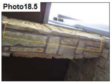
Deteriorated Mortar / Re-point
