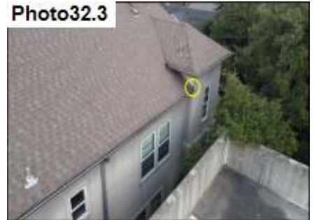
Kickout Flashing / Seal
