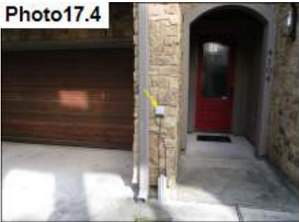
Penetration Sealants / Seal
