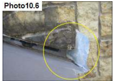
Kickout Flashing / Seal
