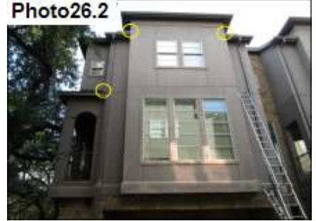
Kickout Flashing / Seal
