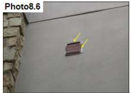
Penetration Sealants / Seal
