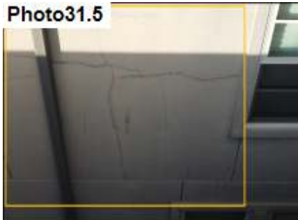
Crack Noted / Seal, Paint or Repair as Needed
