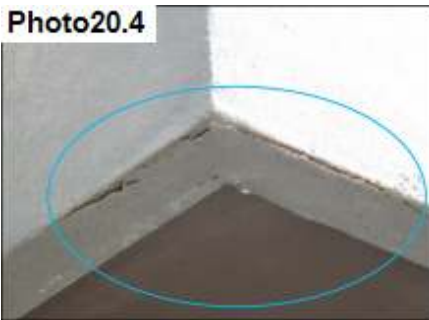
Broken & Rusted Casing Bead / Repair
