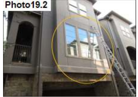
Efflorescence and Deteriorated Paint / Clean & Repaint
