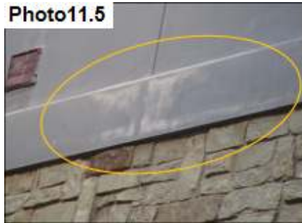
Efflorescence and Deteriorated Paint / Clean & Repaint
