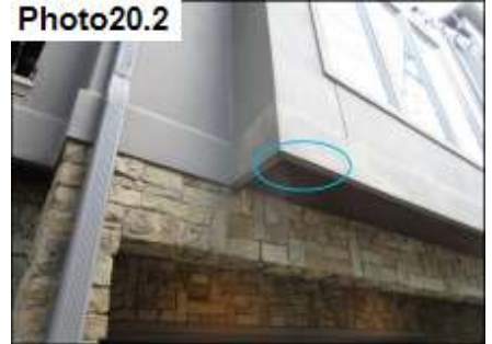
Broken & Rusted Casing Bead / Repair
