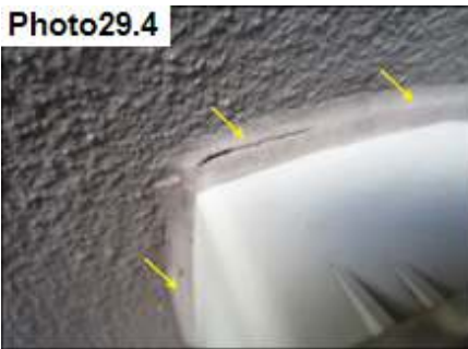
Penetration Sealants / Seal
