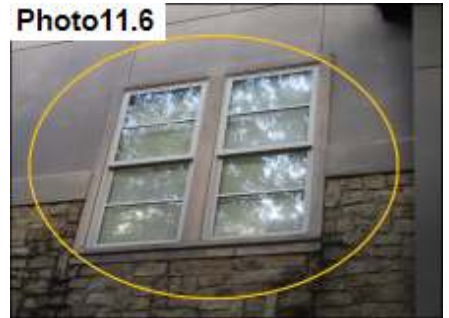
Efflorescence and Deteriorated Paint / Clean & Repaint
