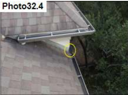
Kickout Flashing / Seal
