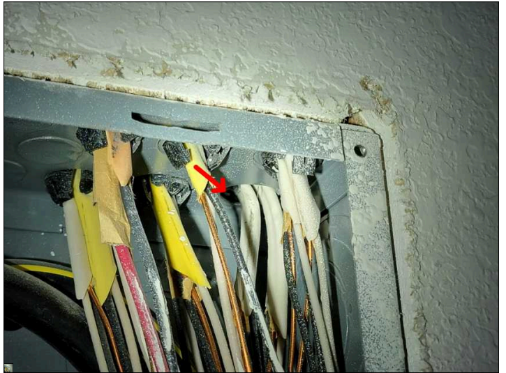
Conductors are not protected against sharp edges. Missing grommets or protective adapters.
