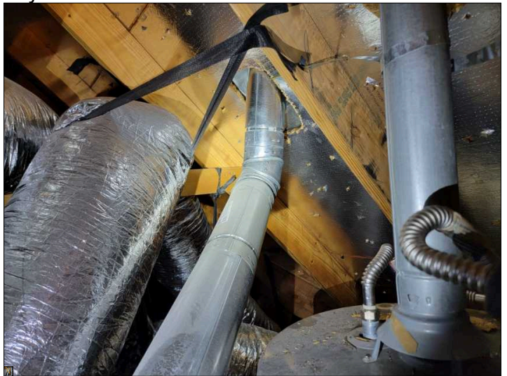
Flue missing strapping near roof. Wind can cause flue to loosen and become disconnected if not secured properly.
