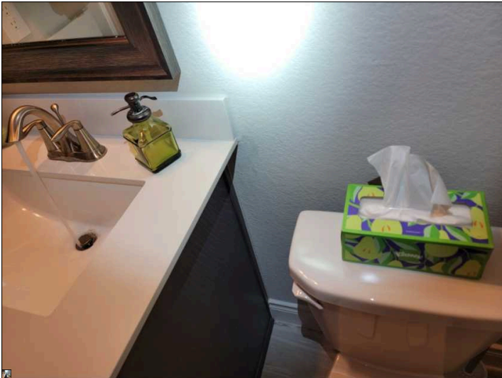
Water stain noted on wall of half bath
