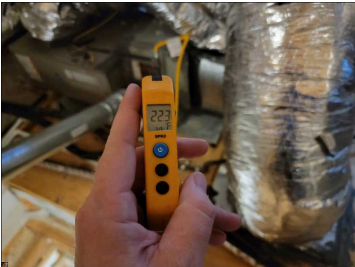
22f delta T across coil is acceptable. Downstairs
