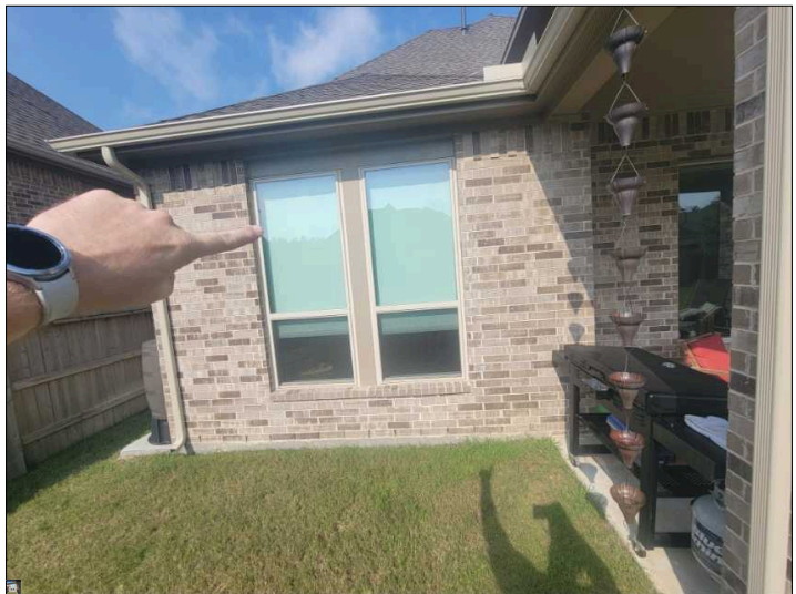
Film damage present inside double pane windows. This is a sign that the gas between panes is gone, and the windows are less energy efficient and can be difficult to see through.
