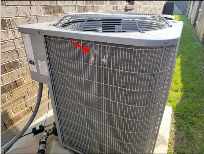
Damaged condenser fins.
