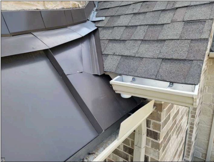
Downspout and gutter near front door are too small to adequately collected and drain. Installed gutter is loose at wall and leaks.
