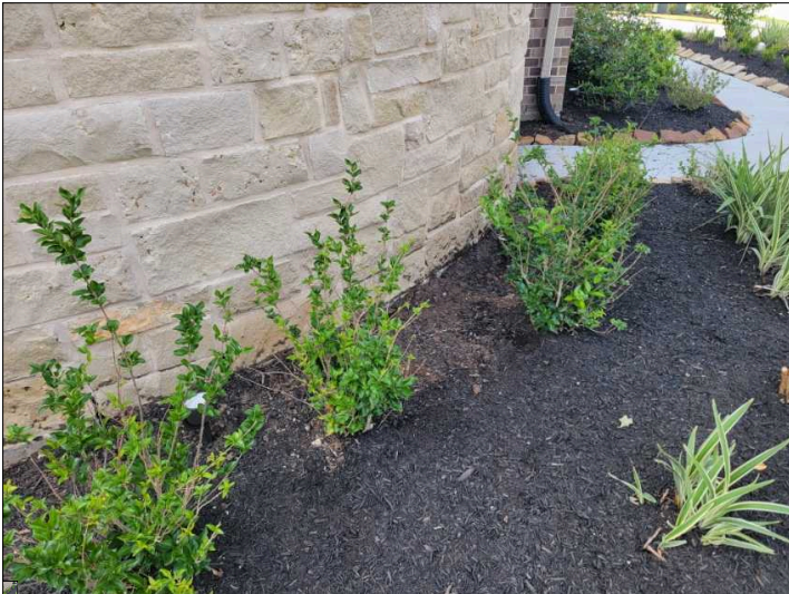
Mulch too tall and allows water to slope back towards house around the round wall. Lower much and keep minimum 4" from weep holes at bottom of stone.
