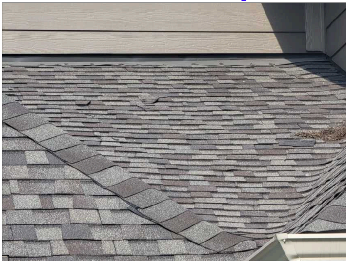
Multiple pieces of shingle debris on roof. No missing pieces found while scanning the roof. Possible construction debris.
