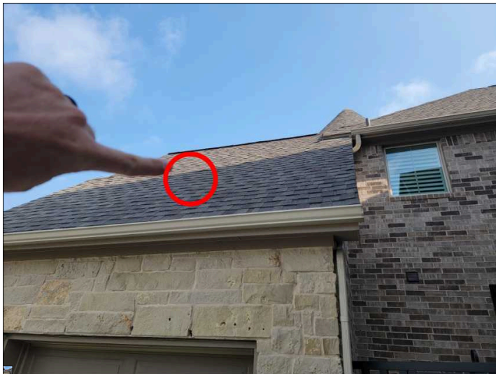
Lifted shingles noted. These are subject to wind drive rain and water entering house.
