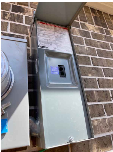
Sub Panel Location: Garage
