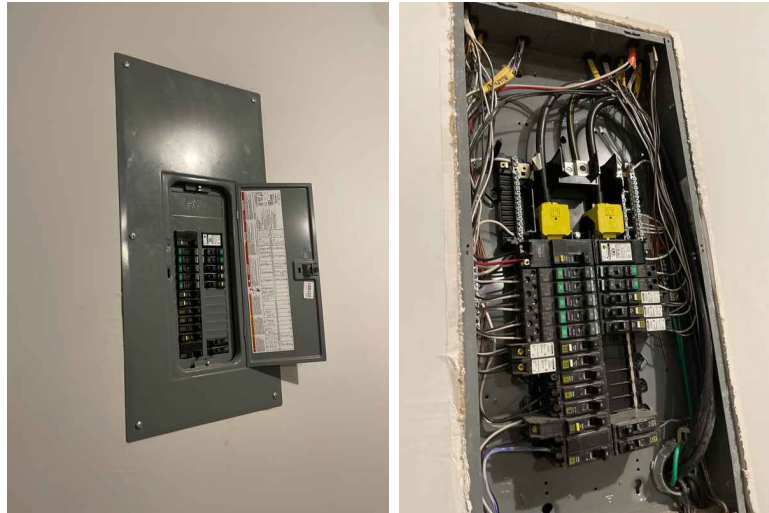
Main Service Panel Amperage: 150 Amp Main Service Panel Manufacturer: Square D
