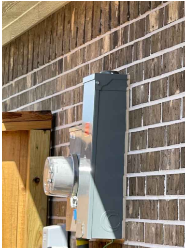
Main Service Panel Location: Rear, East Exterior Wall
