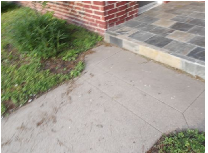
Inadequate grading - improper slope in some areas
