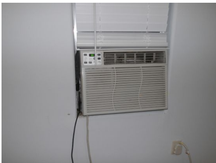
A/C window unit blocking only window in bedroom is a safety hazard - does not provide adequate exit in the case of a fire in Back Building
