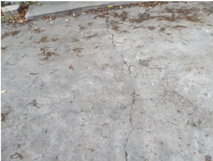
Cracks noted on driveway
