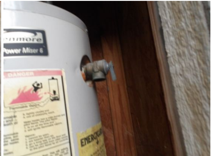
No T/P drain line
