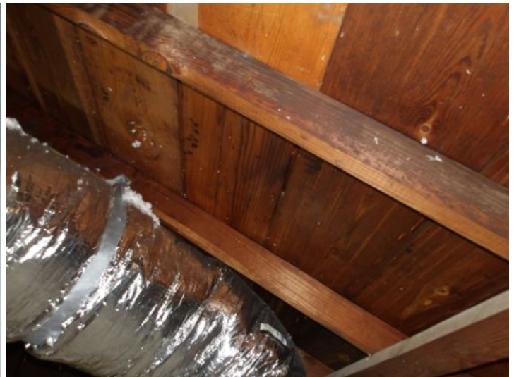
Previous water stains noted on roof sheeting in attic
