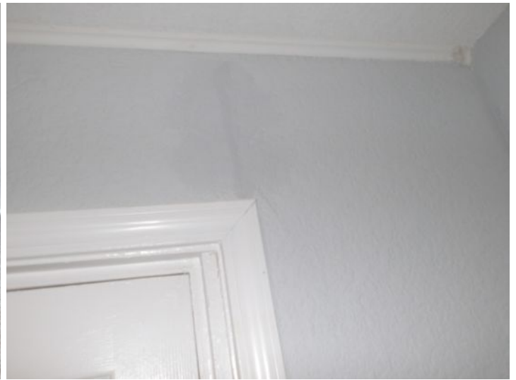
Cracks on sheetrock in different areas
