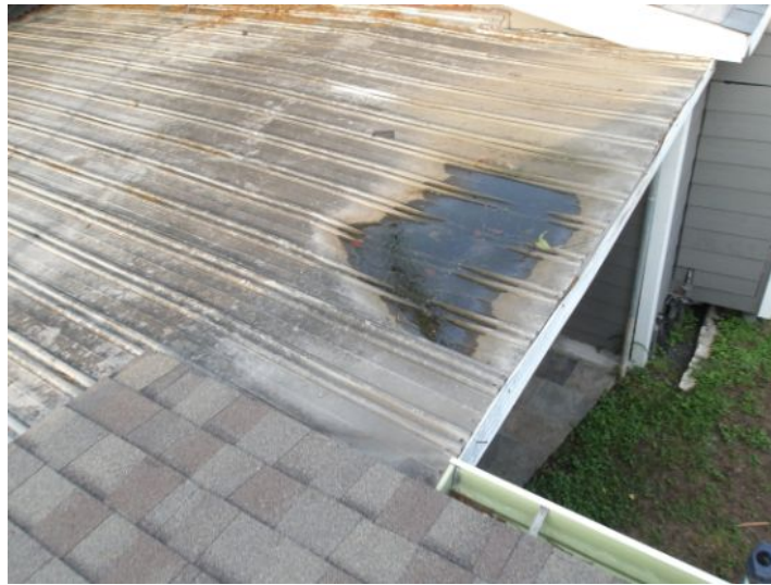
Water standing on roof of carport
