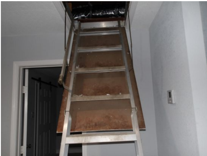
Missing weatherstripping and insulation on attic door
