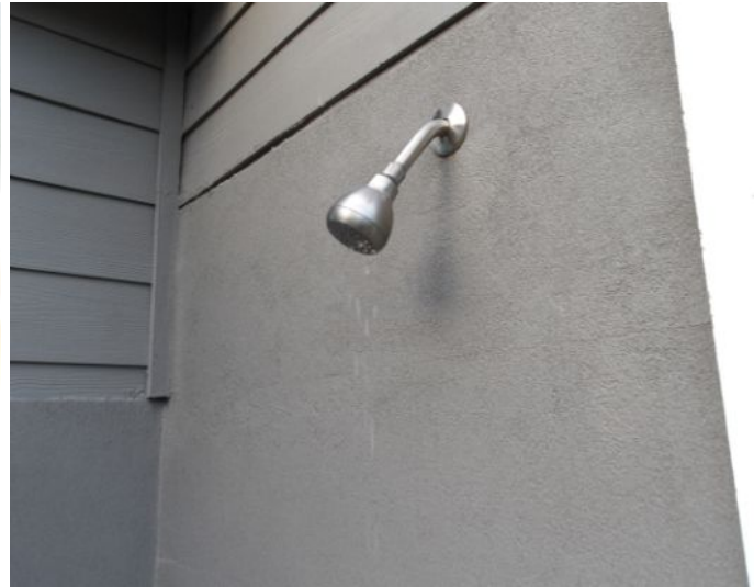
No water out of exterior shower
