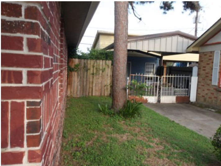
Tree too close to structure
