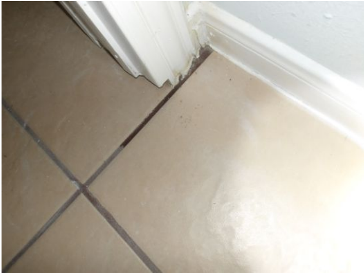
Bath in Back Building - some type of leak coming from shower - unable to determine source
