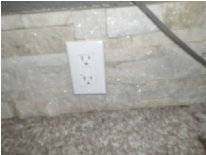
Exterior outlet not weather covered
