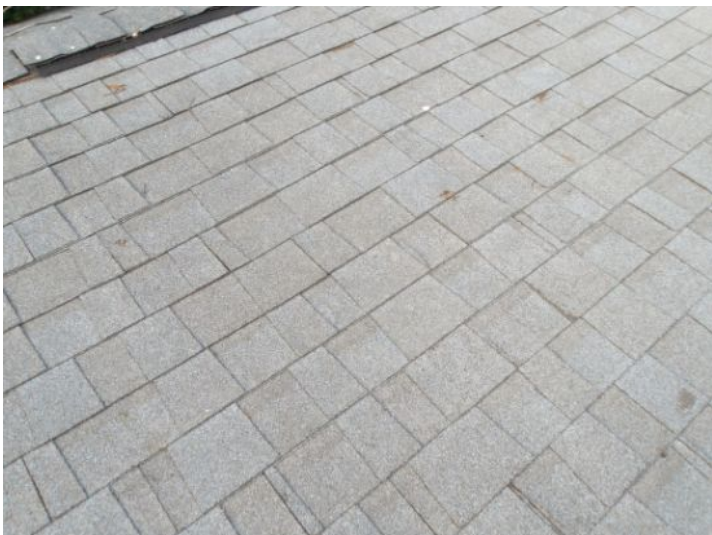
Roof covering was functioning as intended at the time of inspection on Back Building
