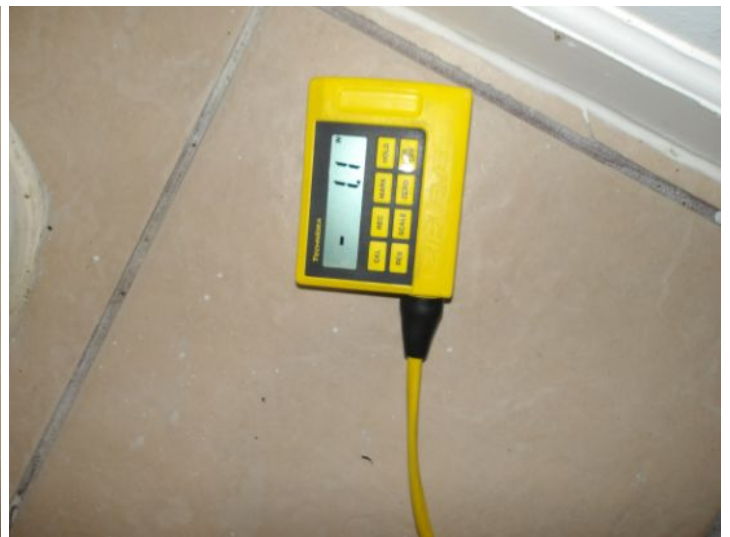
Structural movement and/or settling noted in Back Building. Suggest that a licensed professional be consulted for further evaluation.
