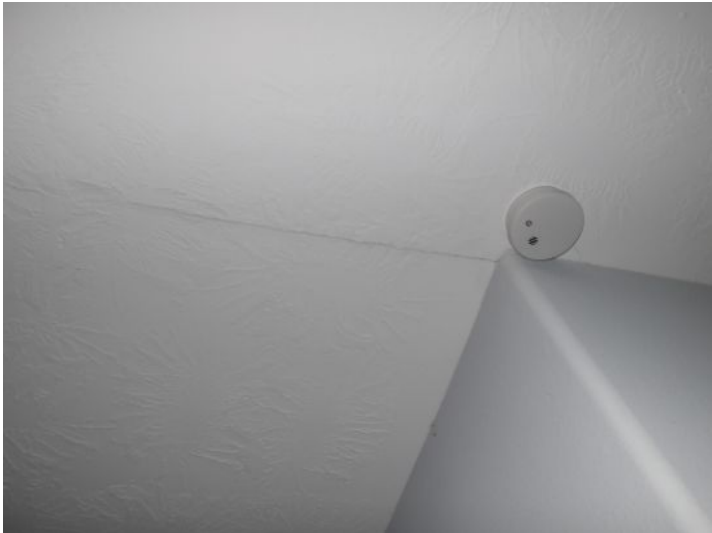
Cracks on ceiling in Back Building
