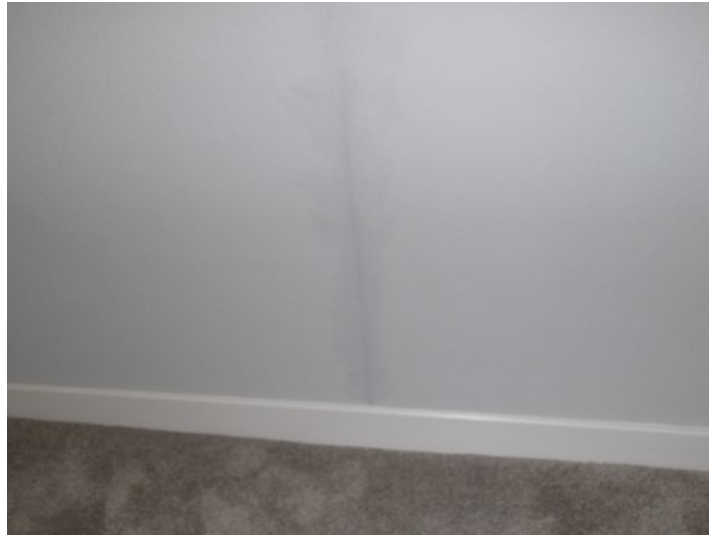
Previous patches on sheetrock in some areas
