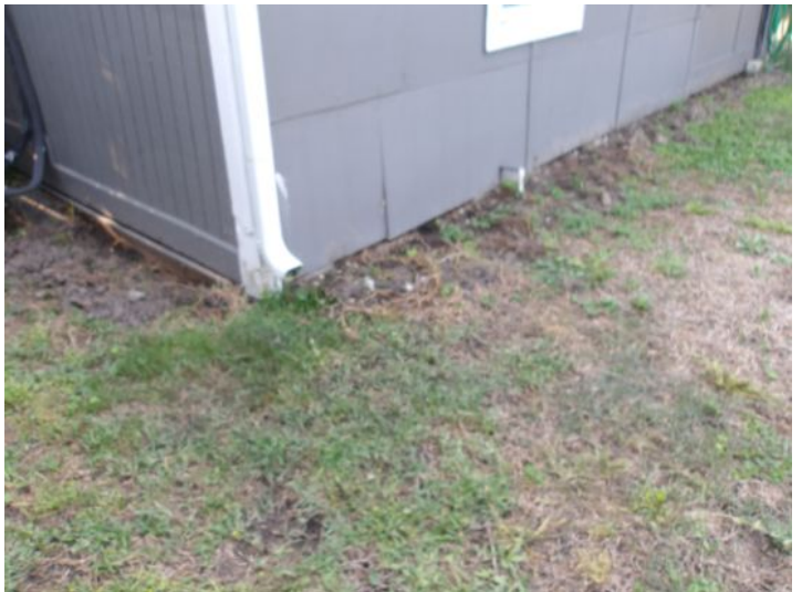
Inadequate grading - improper slope in some areas
