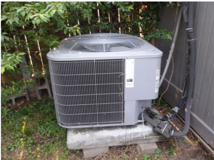
Unit did not cool sufficiently
