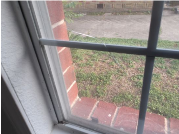
Cracked window pane in Master Bedroom and in Living Area
