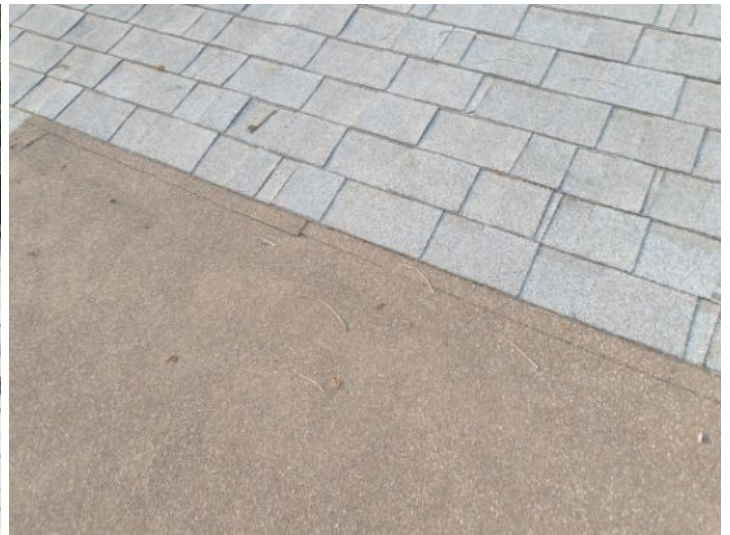
Unable to determine if some type of flashing was used on roof level of Back Building
