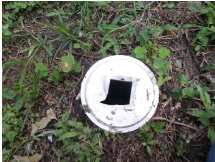
Broken cap on exterior drain - Unable to determine source of drain (no water flowing through drain at the time of inspection)
