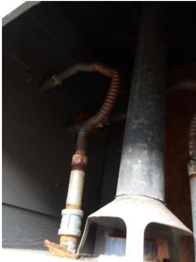
Flue vent not the proper type
