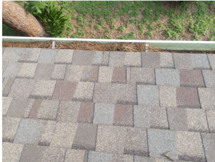
Debris in gutters
