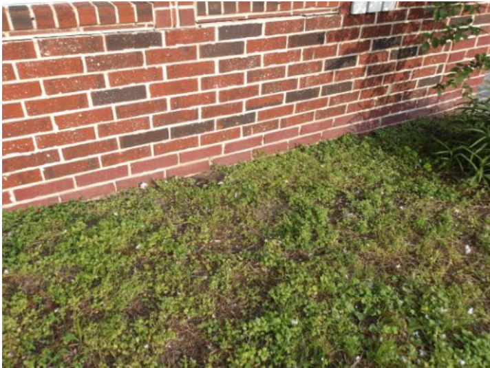
Inadequate grading - high soil
