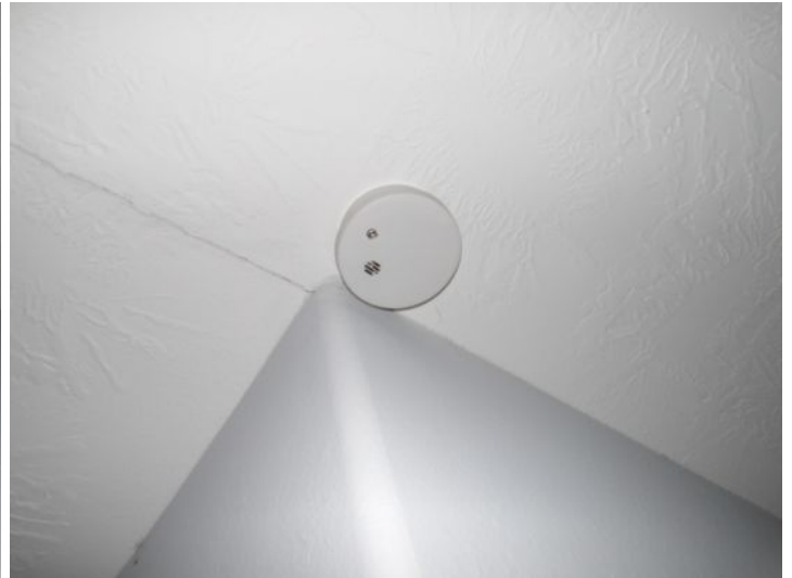
Smoke detector in Back Building functioned at the time of inspection
