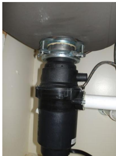
NEW - Disposal in Back Building functioned as intended
