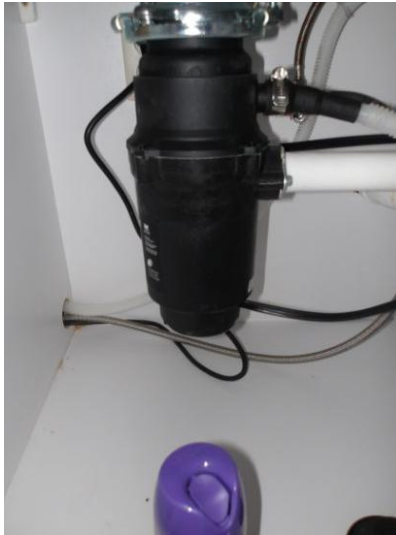
Unit functioned as intended at the time of inspection
