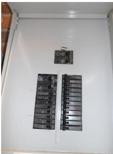
The panel was not labeled properly
