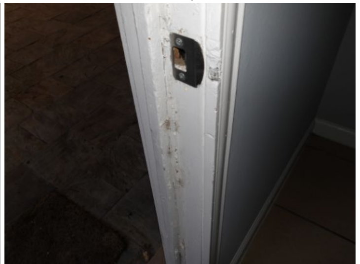
Missing weatherstripping on Front Door of Back Building
