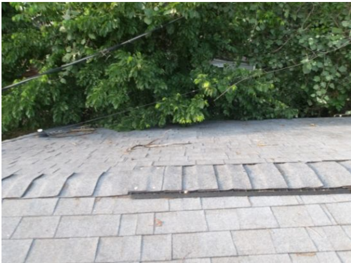
Rotted and damaged roof sheeting on Back shed
