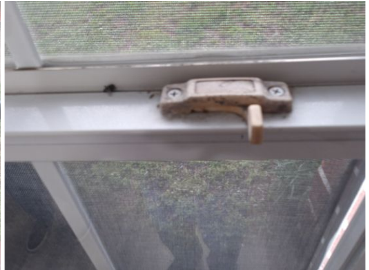
Some windows do not lock
