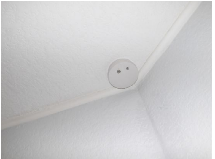
Smoke detectors functioned at the time of inspection
