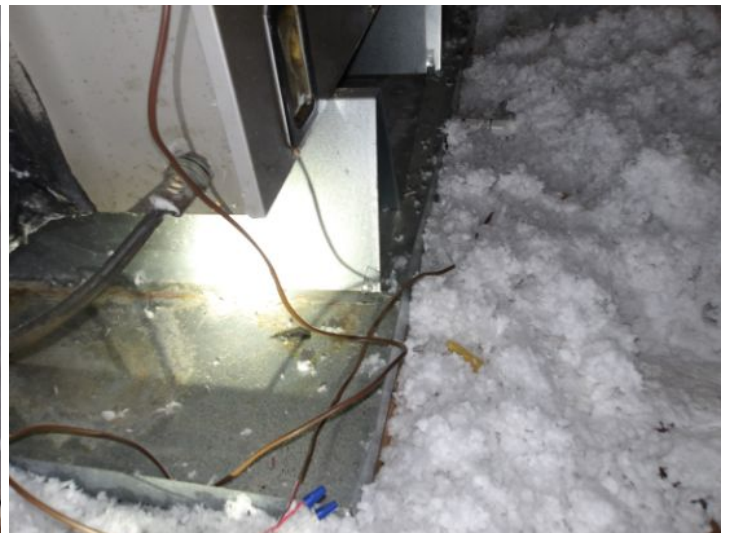
No cut off switch on secondary drain pan
