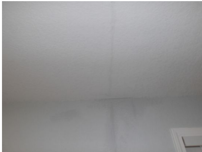
Crack on ceiling in Living Area
