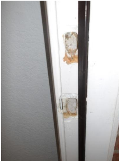
Missing striker plates on back doors
