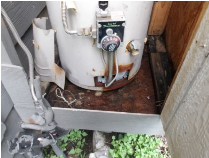
Rust damage on unit
