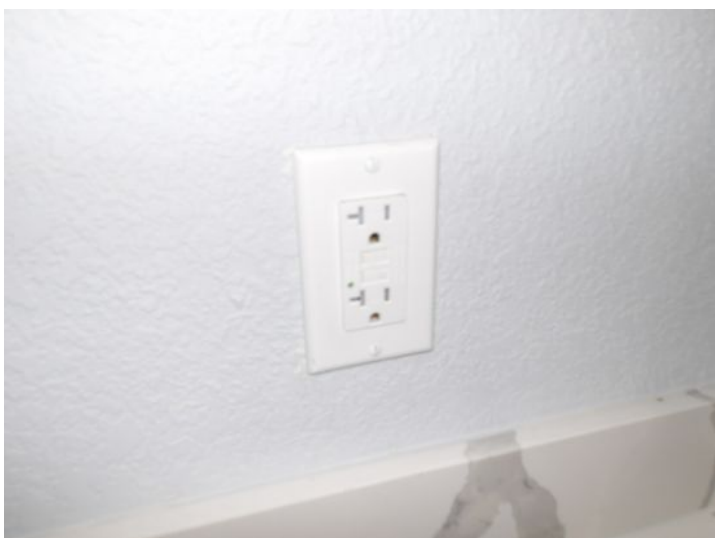
GFCI outlet in Hall Bath did not function at the time of inspection
