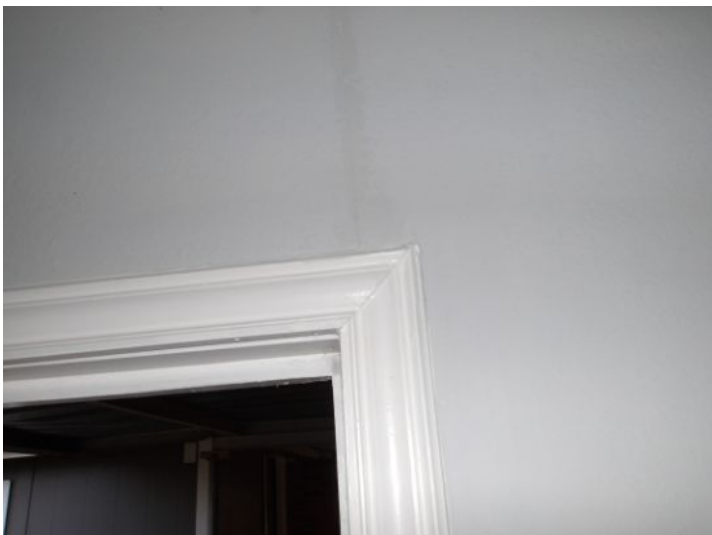
Cracks on sheetrock in Back Building
