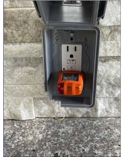
B. Item 8(Picture) Outdoor cooking area
