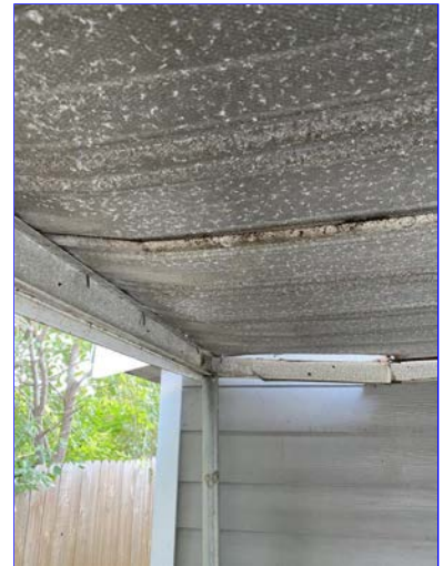
K. Item 6(Picture) Sag not corrected
