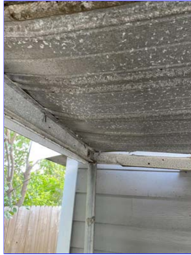
K. Item 2(Picture) Sag not corrected
