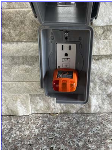
B. Item 12(Picture) Outdoor cooking area
