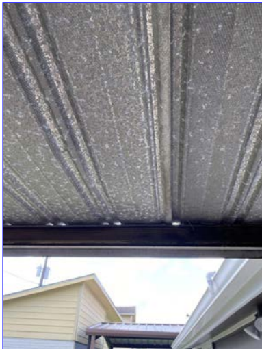
K. Item 4(Picture) Leak corrected
