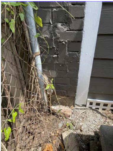
E. Item 21(Picture) Corrected
