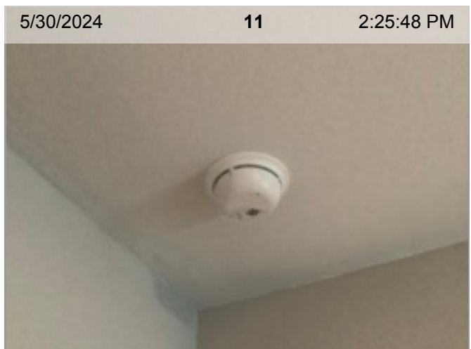
Wired Smoke Alarm (mfd 9/2022) | Smoke test: Passed | Alarm in place
