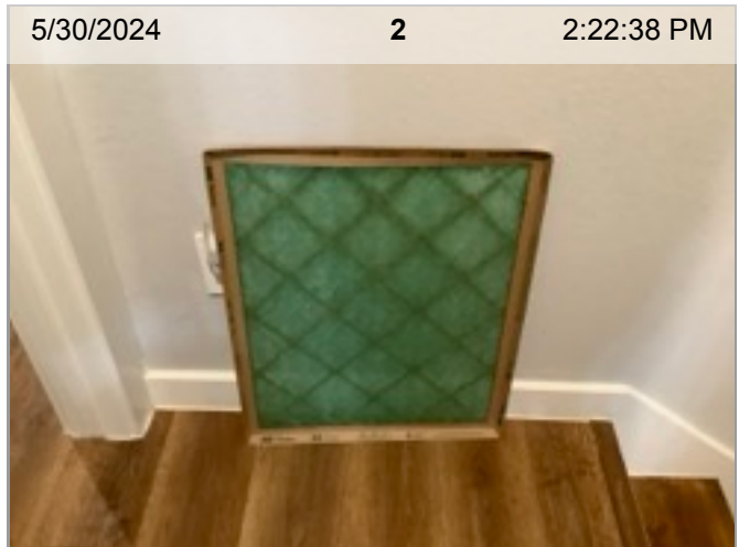
20 x 25 x 1 Air Filter Installed | Front
