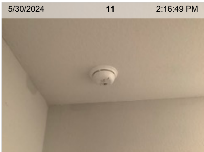
Wired Smoke/CO Combo Smoke Alarm | Smoke test: Not tested | Alarm in place | Alarms with no date are over 10 years old.
