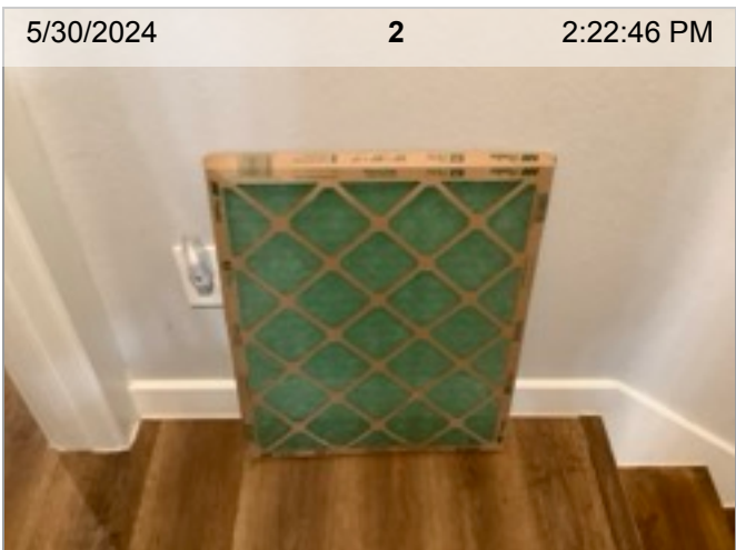
20 x 25 x 1 Air Filter Installed | Back
