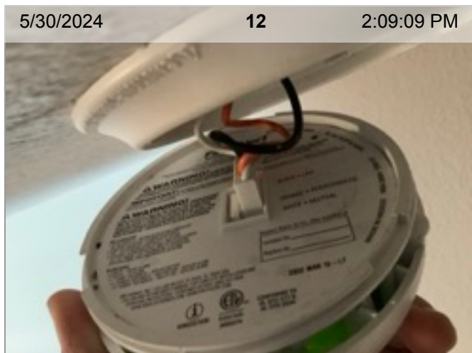
Wired Smoke/CO Combo Smoke Alarm (mfd 3/2022) | Smoke test: Passed | Close-up of printed manufacture date | 2.2 years old
