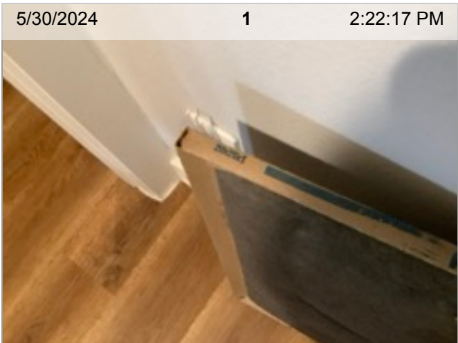
20 x 25 x 1 Air Filter Removed | Close-up of size/initials/date
