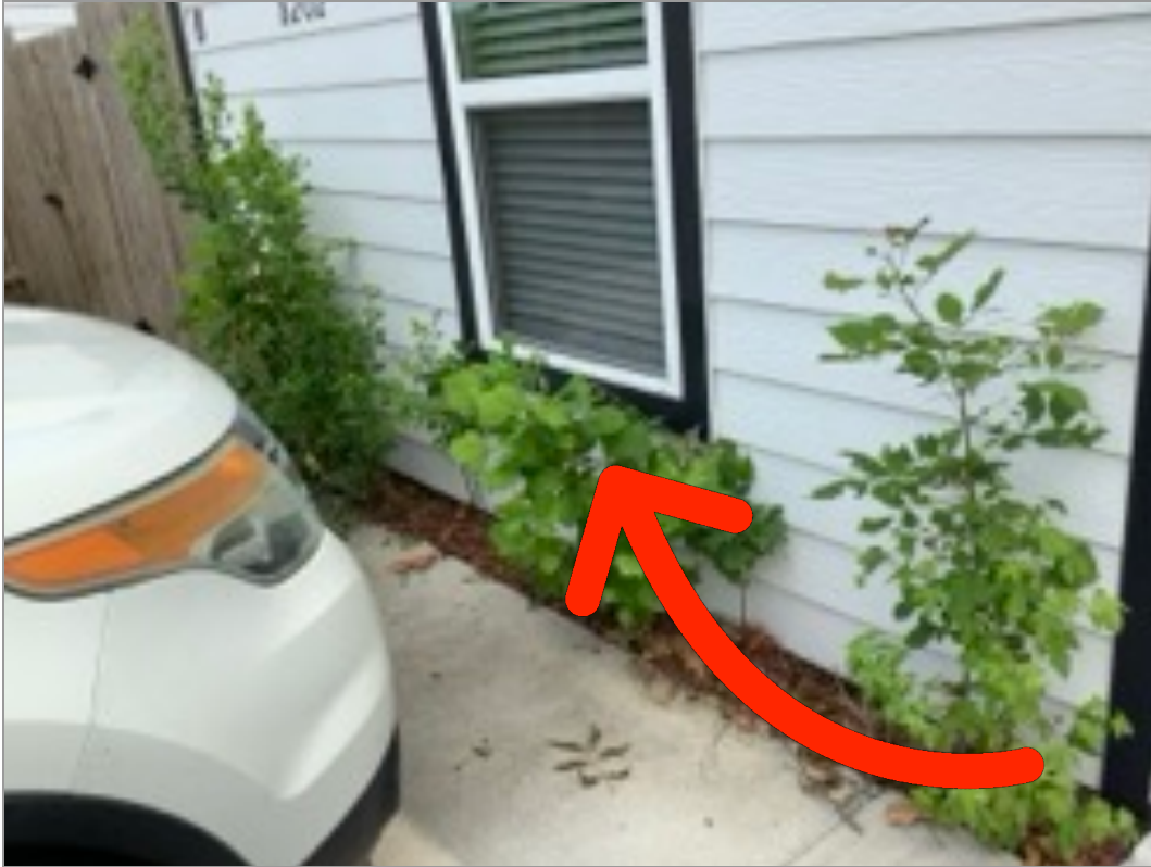
Front Exterior Trees/Shrubs/Landscaping Overgrown landscaping
