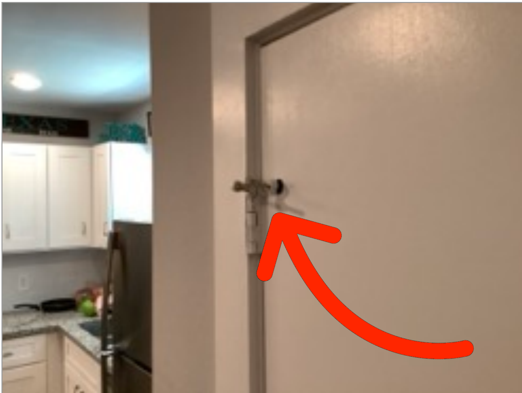
Laundry Room Door Stop Broken- no wall damage noted.
