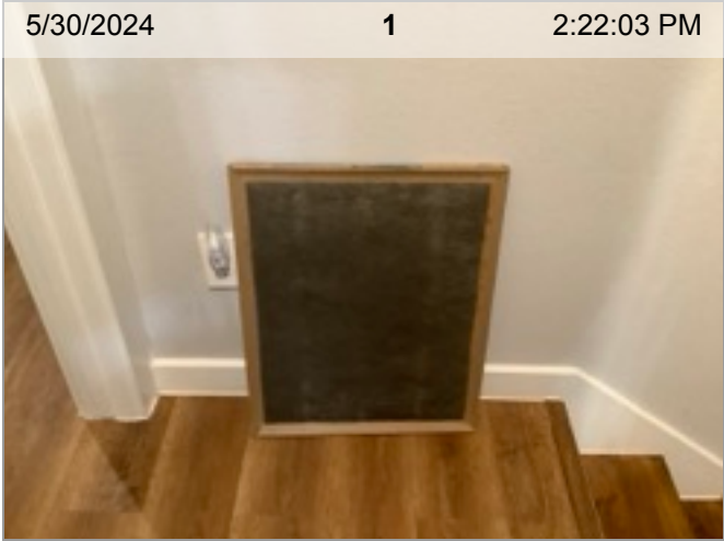
20 x 25 x 1 Air Filter Removed | Front
