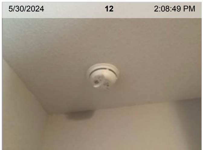
Wired Smoke/CO Combo Smoke Alarm (mfd 3/2022) | Smoke test: Passed | Alarm in place
