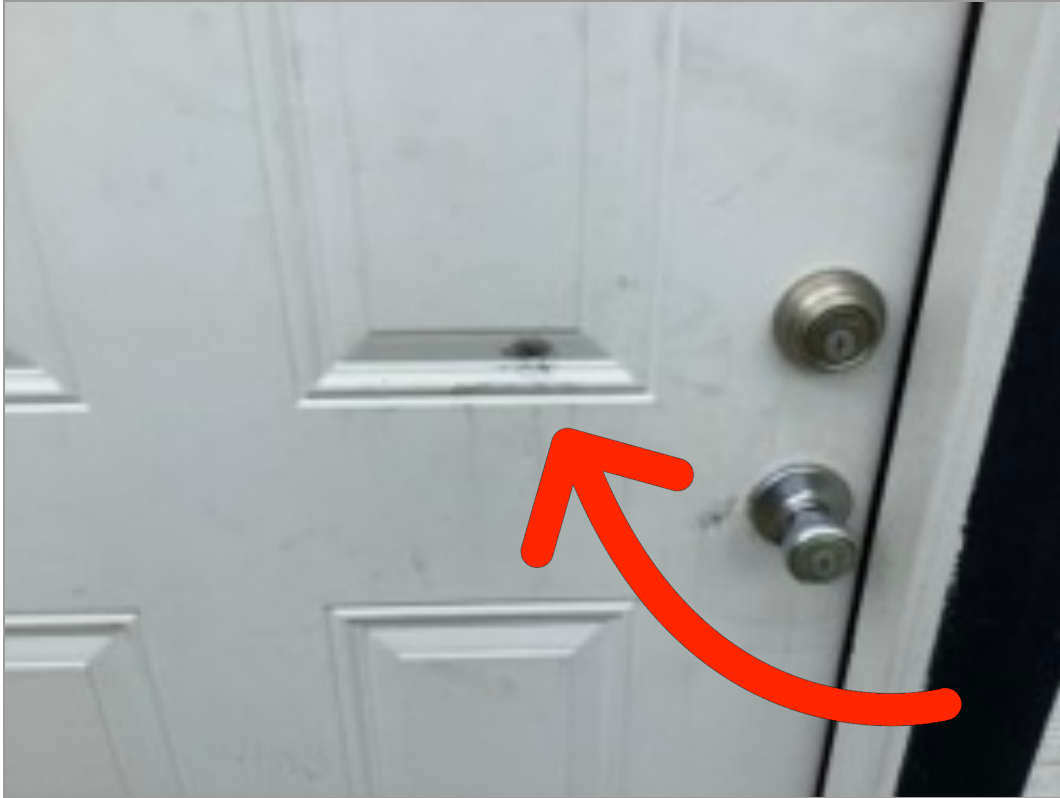
Entry Front Door Exterior Scratches; stains; discoloration or chipping of door casing
