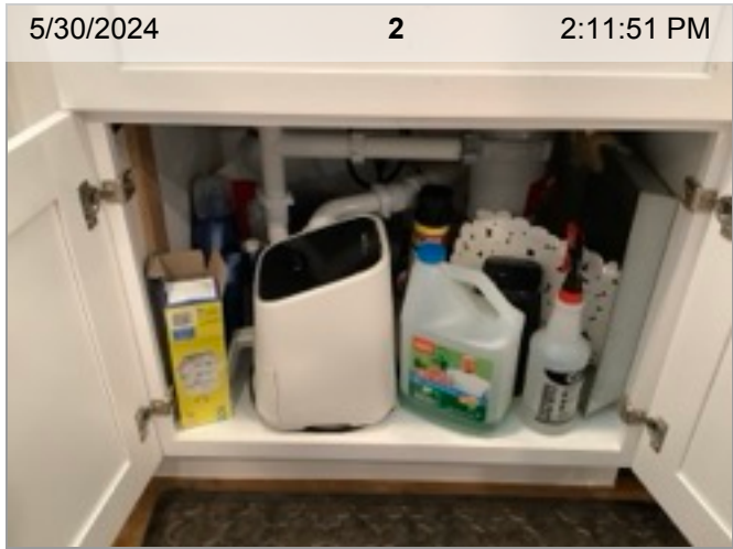
Cabinet Under Sink
