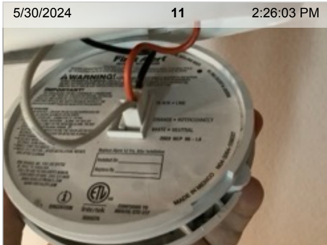
Wired Smoke Alarm (mfd 9/2022) | Smoke test: Passed | Close-up of printed manufacture date | 1.7 years old
