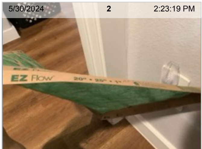
20 x 25 x 1 Air Filter Installed | Close-up of size/initials/date
