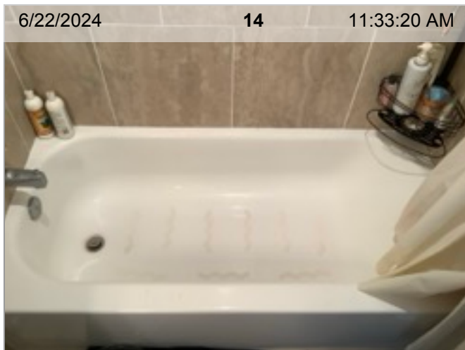
Tub/Fixture | Base of Tub
