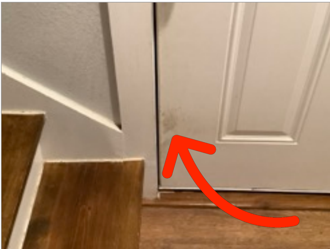
Entry Front Door Interior Scuffs on door
