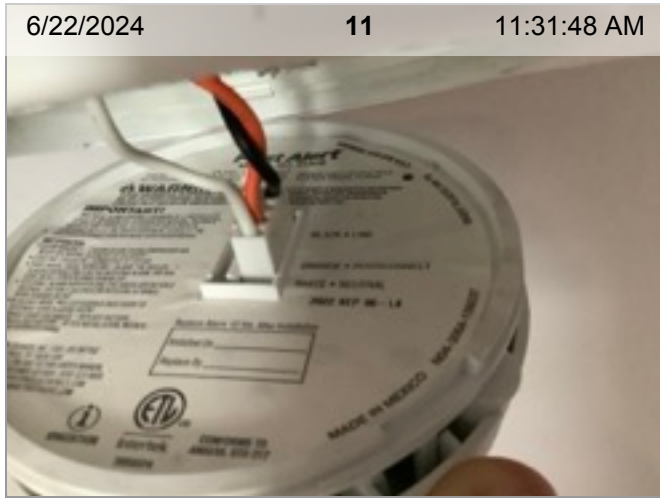
Wired Smoke Alarm (mfd 9/2022) | Smoke test: Passed | Close-up of printed manufacture date | 1.8 years old
