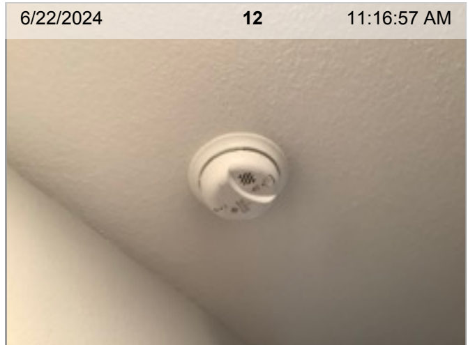
Wired Smoke/CO Combo Smoke Alarm (mfd 5/2022) | Smoke test: Passed | Alarm in place
