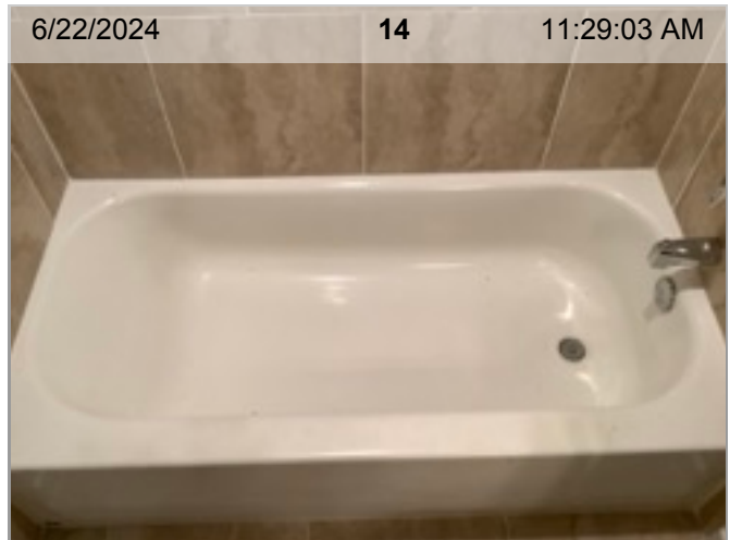
Tub/Fixture | Base of Tub
