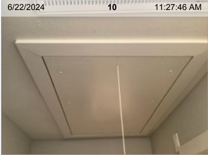
Inaccessible Water Heater | NA | Water heater (with expansion tank if present) | Water heater is in the attic
