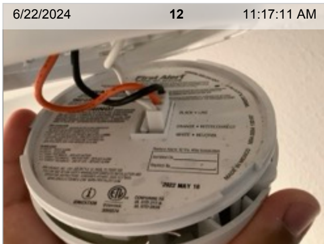
Wired Smoke/CO Combo Smoke Alarm (mfd 5/2022) | Smoke test: Passed | Close-up of printed manufacture date | 2.1 years old
