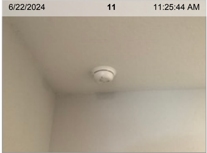
Wired Smoke/CO Combo Smoke Alarm | Smoke test: Not tested | Alarm in place | Alarms with no date are over 10 years old.
