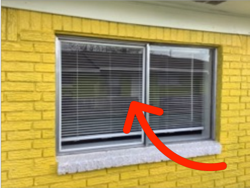
Front Exterior Window Screens Screen(s) are missing
