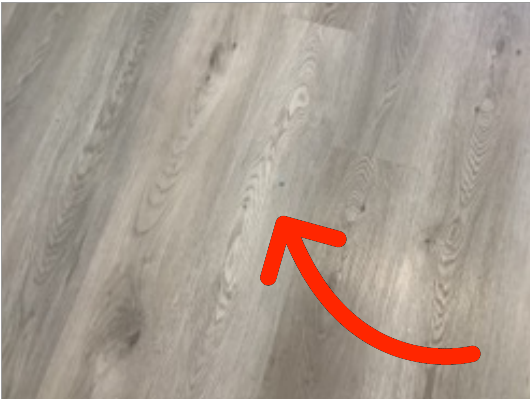
Entry Floors Flooring is stained.
