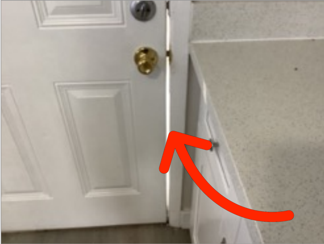
Kitchen Exterior Door Gaps in weather stripping
