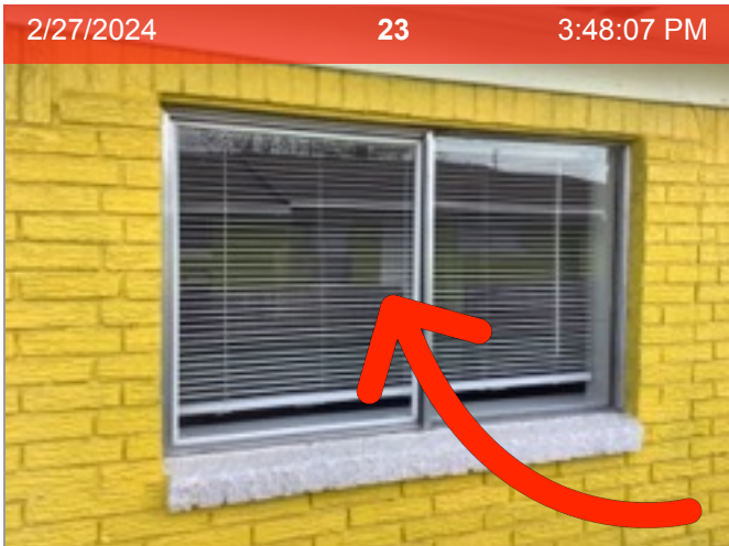
Window Screens | Screen(s) are missing
