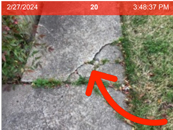
Walkways | Cracked or uneven
