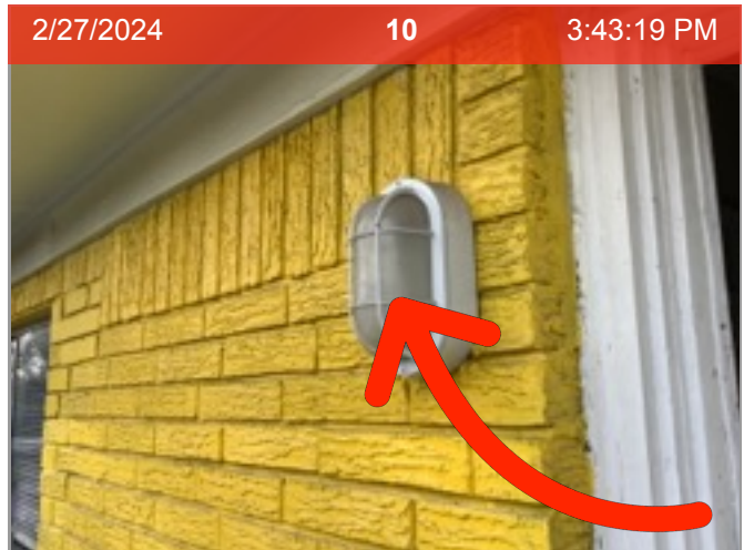
Light Fixtures | Light did not turn on. |
