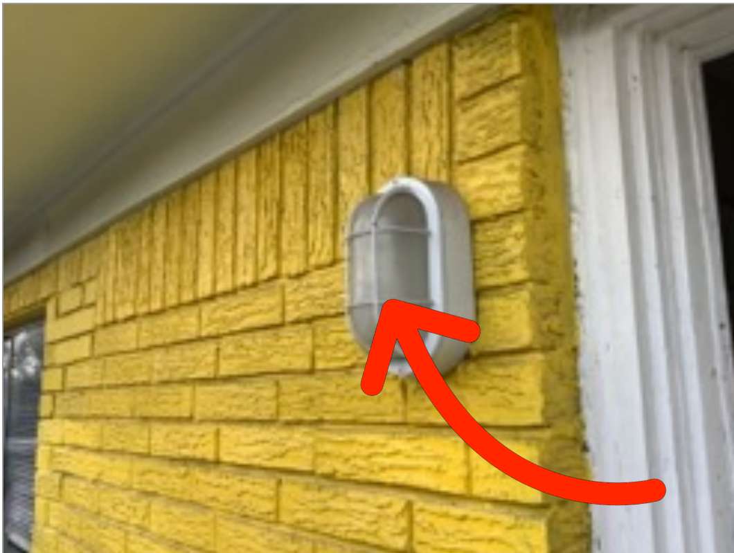
Rear Exterior Light Fixtures Light did not turn on.
