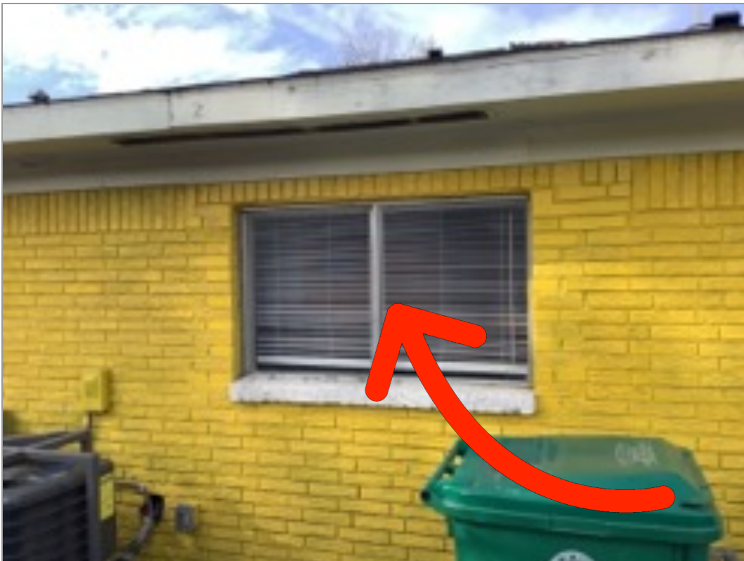
Rear Exterior Window Screens Screen(s) are missing
