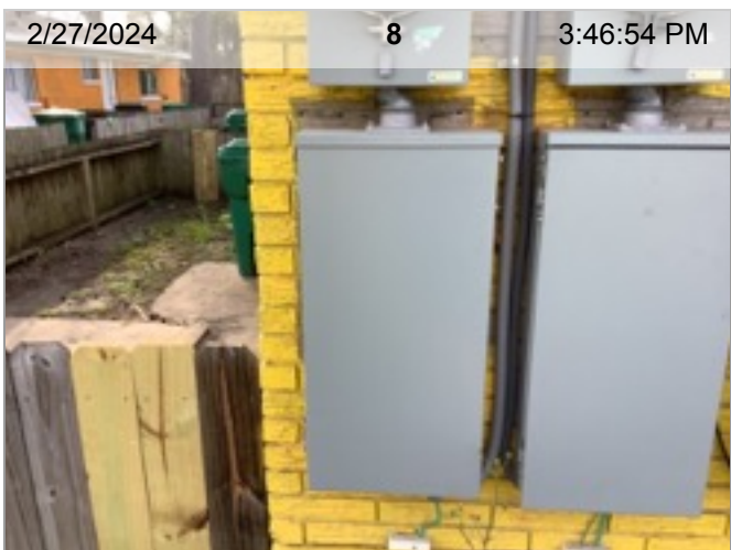
Electrical Breaker Panel
