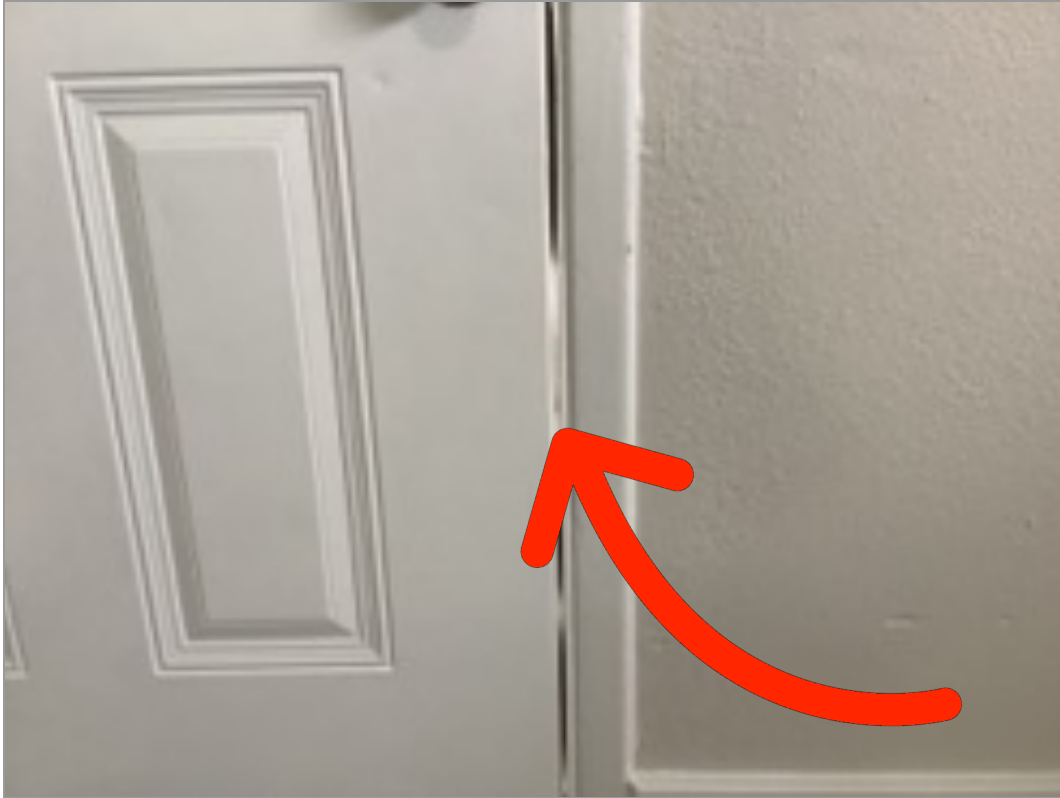
Entry Front Door Interior Gaps in weather stripping
