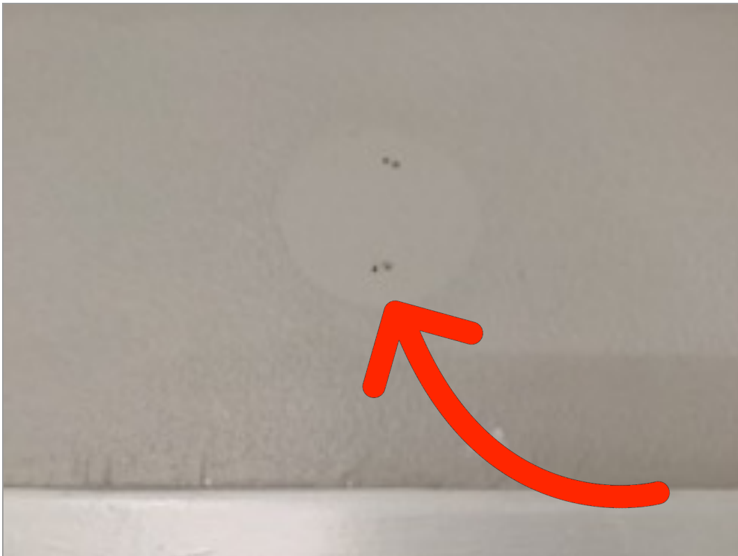
Bedroom 1 Walls/Paint Holes in wall.
