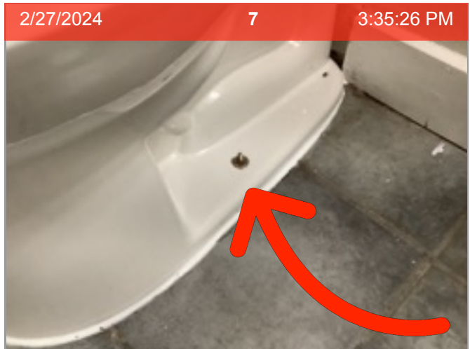
Commode | Bolt caps missing
