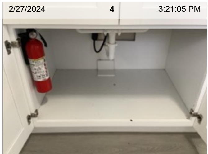
Cabinet Under Sink
