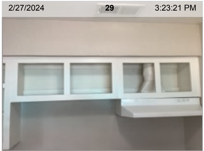
Upper Cabinets - Exterior
