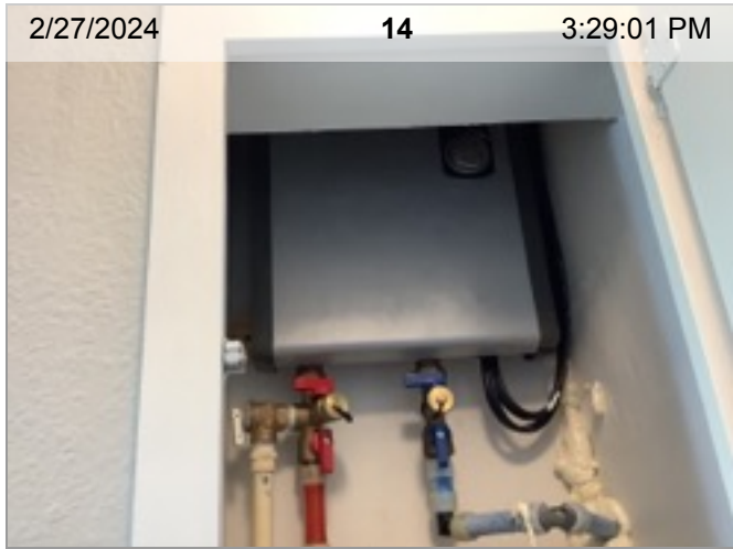
Electric Water Heater | Rheem | Water heater (with expansion tank if present)
