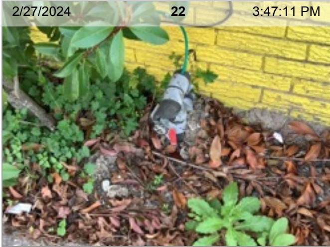
Water Shut Off
