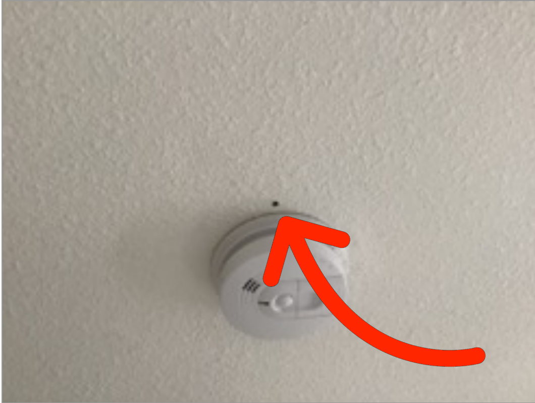
Bedroom 1 Ceiling Holes
