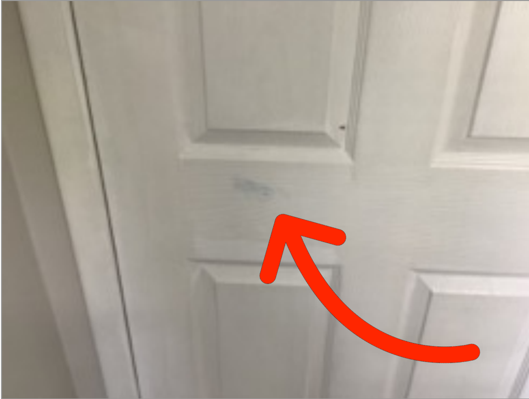
Bedroom 2 Door Discolored
