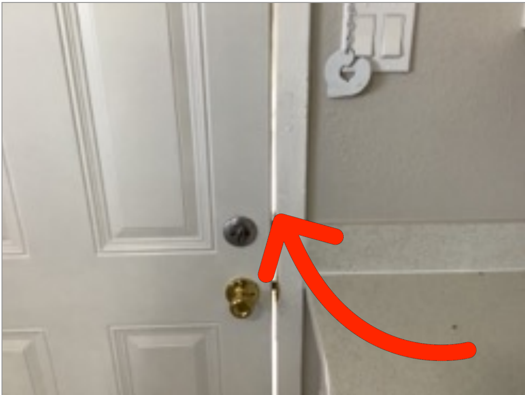
Kitchen Exterior Door Gaps in weather stripping
