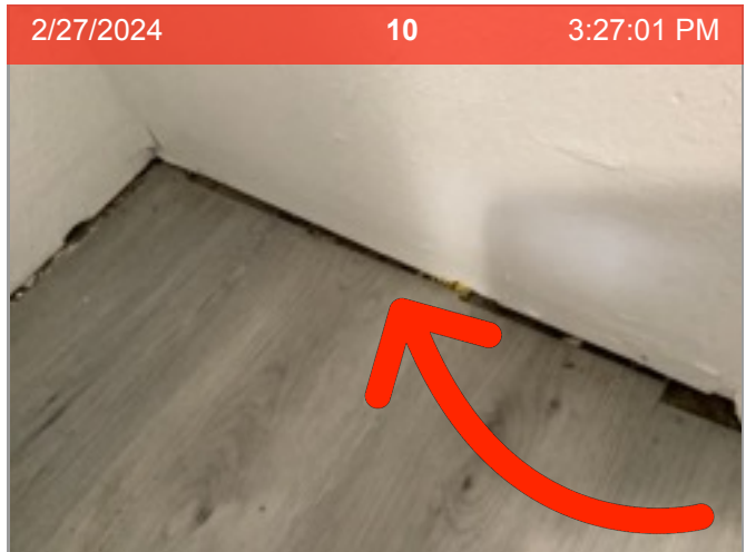
Floors | Gap in flooring.
