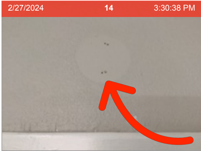
Walls/Paint | Holes in wall.
