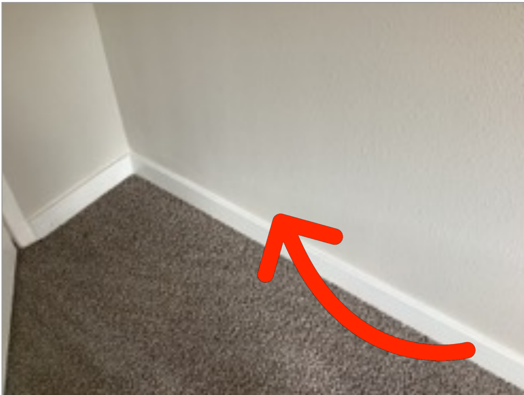
Bedroom 1 Door Stop Missing- no wall damage noted.
