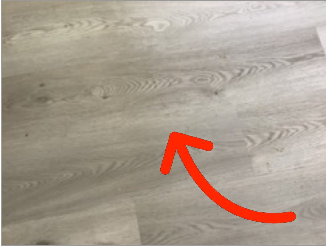
Entry Floors Flooring is scratched.
