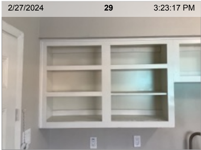
Upper Cabinets - Exterior
