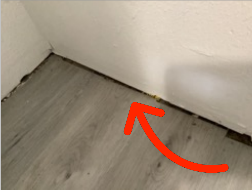
Laundry Room Floors Gap in flooring.
