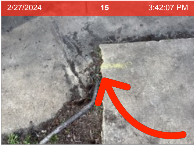
Porch/Patio/Deck | Cracked concrete
