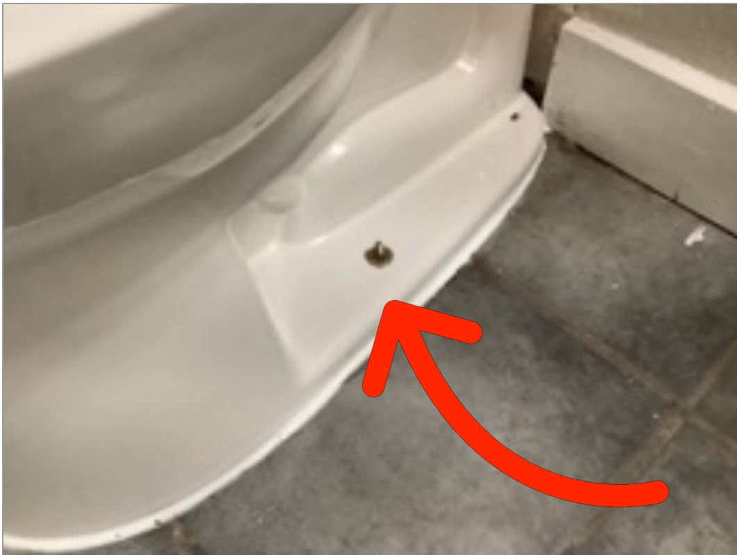
Bathroom 1 Commode Bolt caps missing
