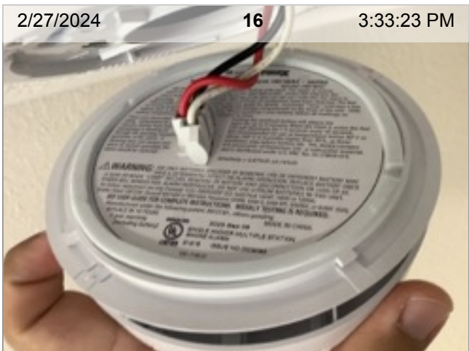
Wired Smoke Alarm (mfd 9/2023) | Smoke test: Passed | Close-up of printed manufacture date | .5 years old
