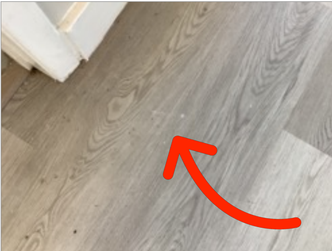
Hallway/Stairway Floors Flooring is scratched.
