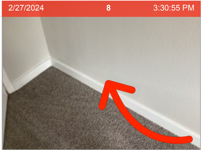
Door Stop | Missing- no wall damage noted.
