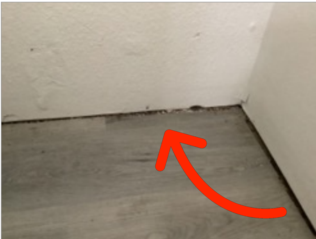
Laundry Room Floors Gap in flooring.
