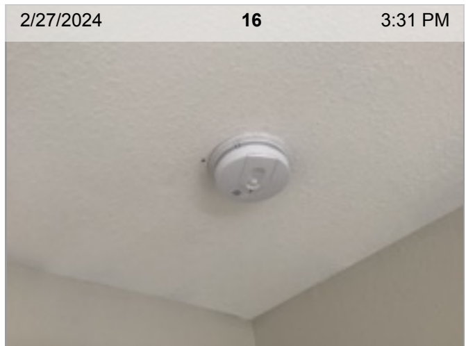
Wired Smoke Alarm (mfd 8/2023) | Smoke test: Passed | Alarm in place
