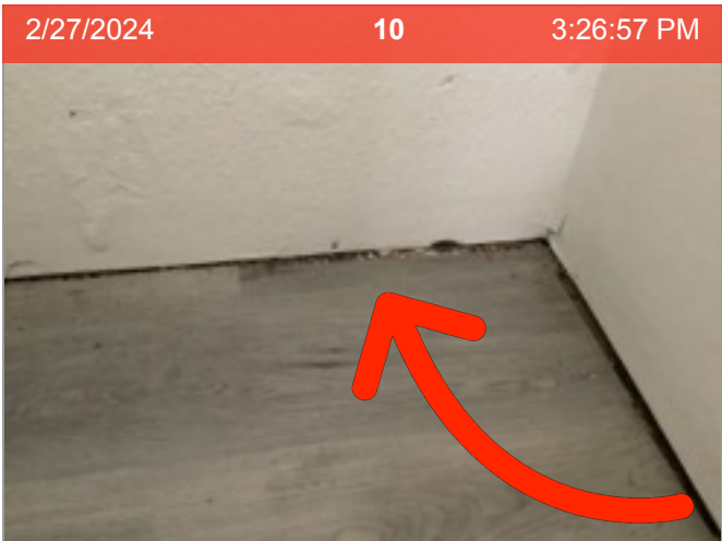
Floors | Gap in flooring.
