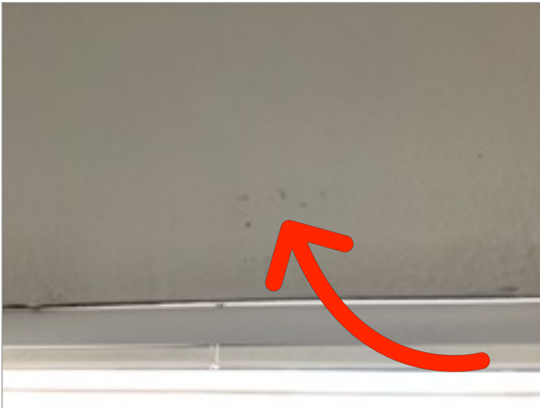
Entry Walls/Paint Scratches on the wall
