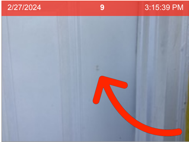
Front Door Exterior | Scratches; stains; discoloration or chipping of door casing
