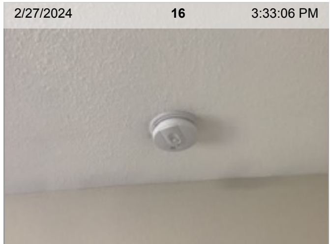
Wired Smoke Alarm (mfd 9/2023) | Smoke test: Passed | Alarm in place
