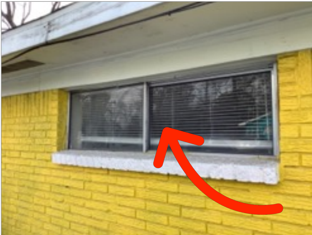
Front Exterior Window Screens Screen(s) are missing
