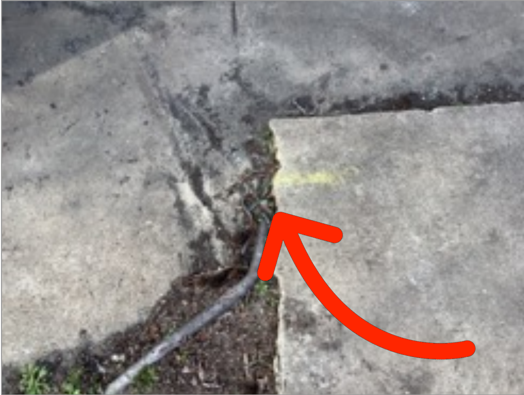
Rear Exterior Porch/Patio/Deck Cracked concrete
