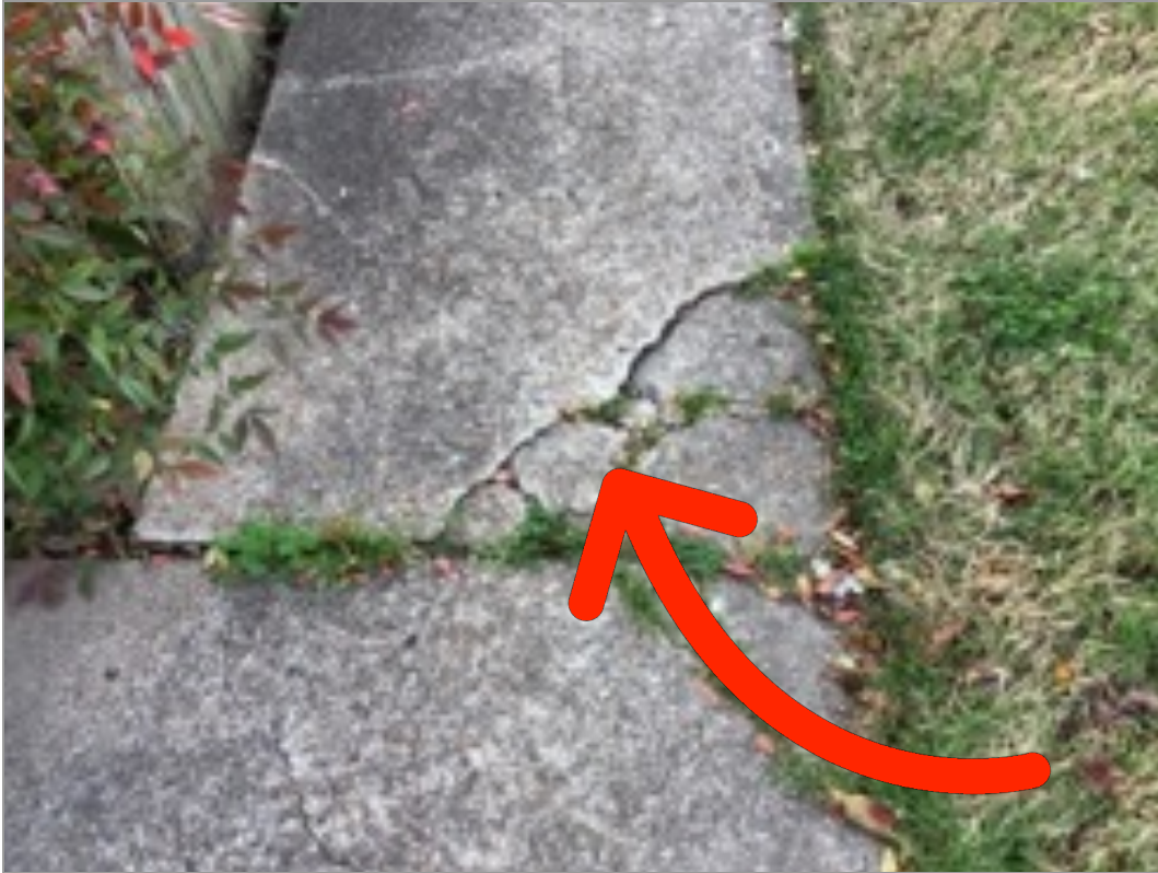
Front Exterior Walkways Cracked or uneven
