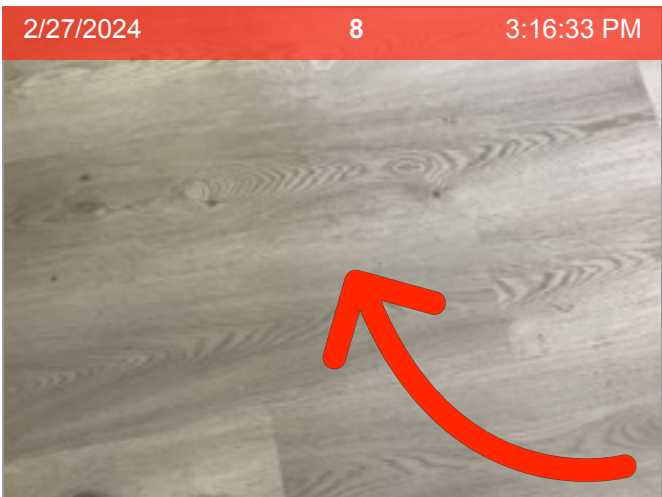
Floors | Flooring is scratched.
