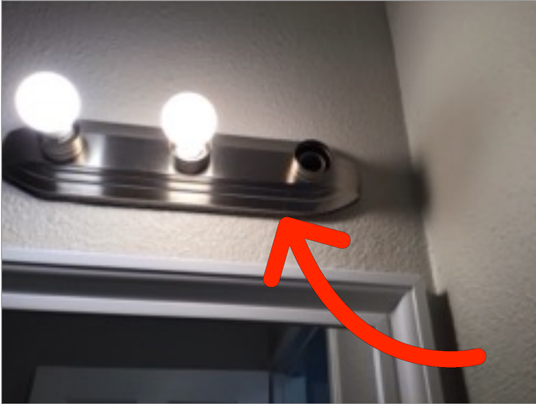
Bathroom 1 Light Fixtures Bulb is missing
