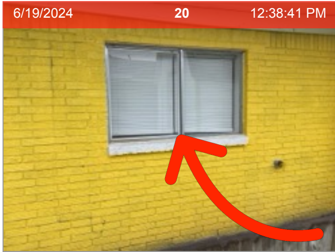
Window Screens | Screen(s) are missing
