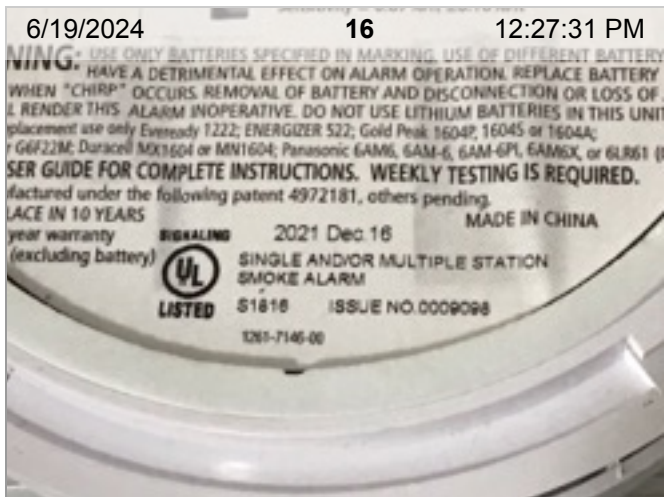
Wired Smoke Alarm (mfd 12/2021) | Smoke test: Passed | Close-up of printed manufacture date | 2.6 years old
