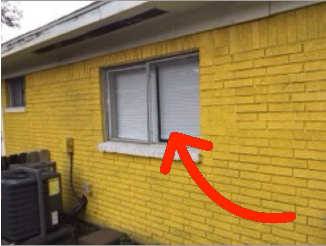
Rear Exterior Window Screens Screen(s) are missing
