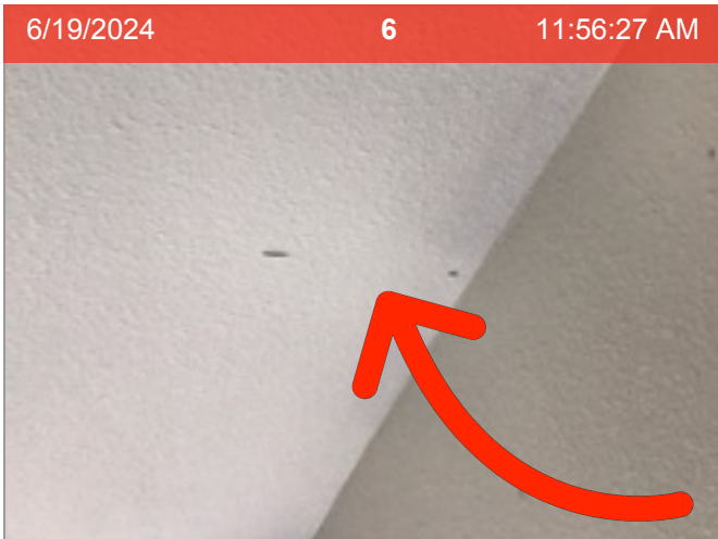
Ceiling | Cracks in ceiling.
