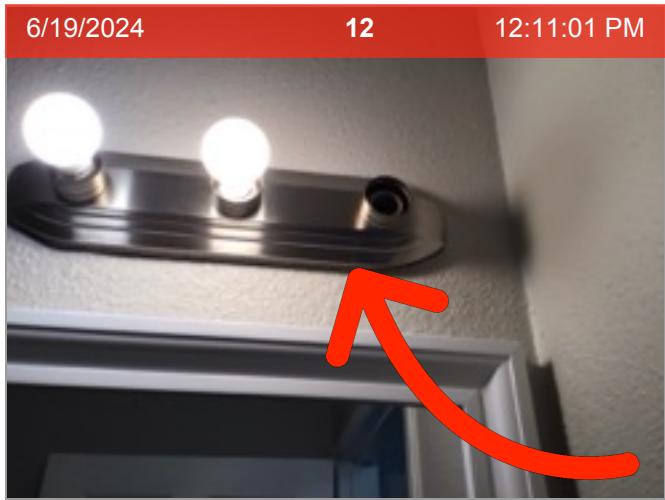
Light Fixtures | Bulb is missing
