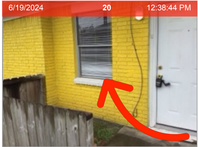
Window Screens | Screen(s) are missing
