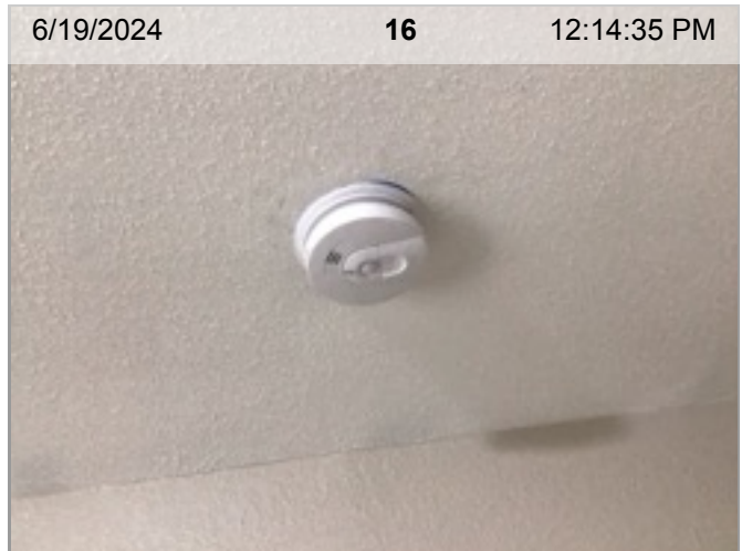
Wired Smoke Alarm (mfd 12/2021) | Smoke test: Passed | Alarm in place
