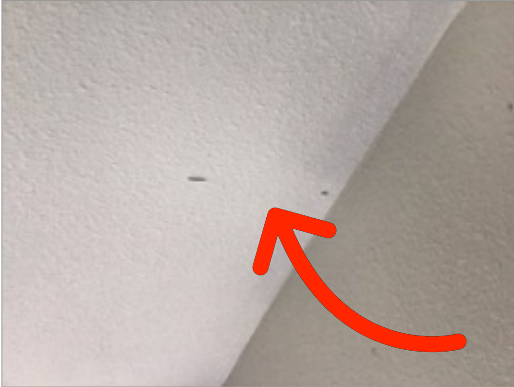
Living Room Ceiling Cracks in ceiling.
