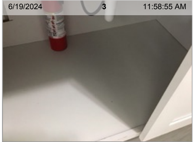
Cabinet Under Sink
