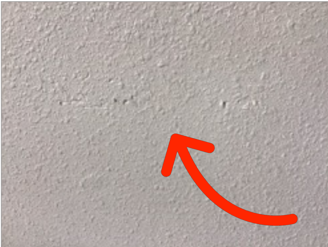
Bedroom 2 Walls/Paint Scratches on the wall
