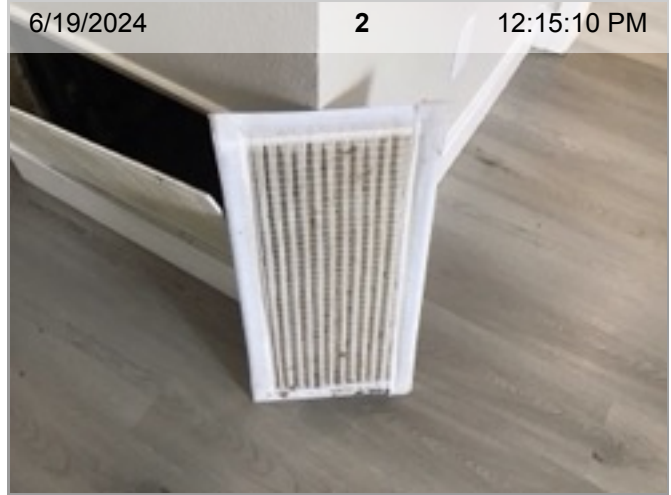
12 x 24 x 1 Air Filter Removed | Front
