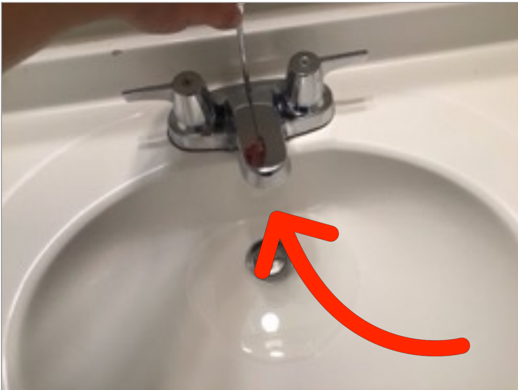
Bathroom 1 Sink/Faucet Drain switch not functioning
