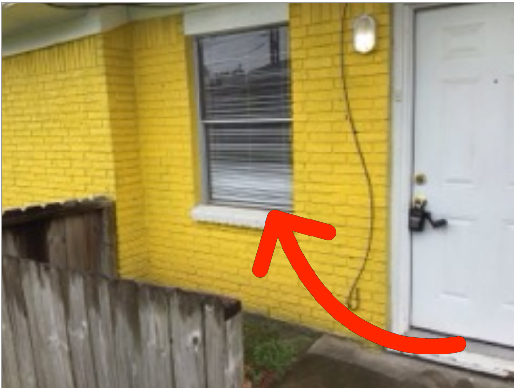
Front Exterior Window Screens Screen(s) are missing
