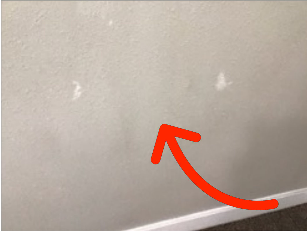
Bedroom 1 Walls/Paint The wall is discolored
