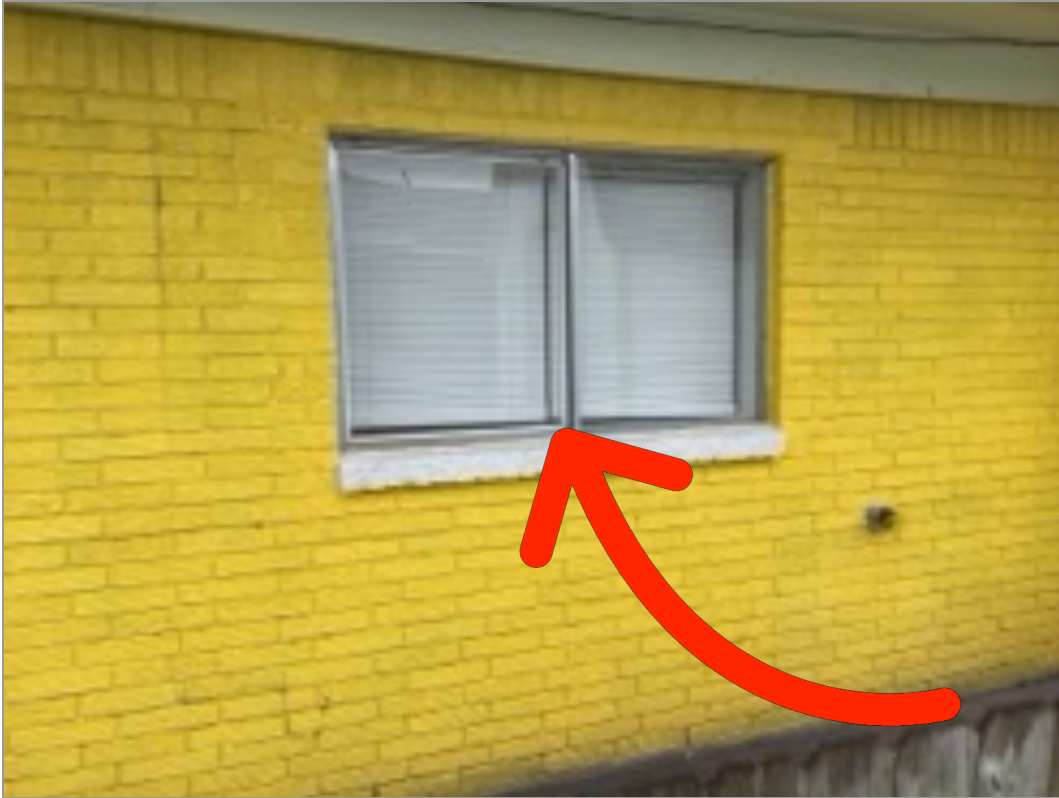
Front Exterior Window Screens Screen(s) are missing
