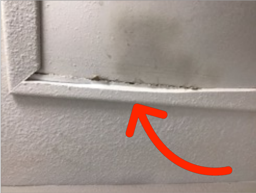
Hallway/Stairway Ceiling Cracks in ceiling.
