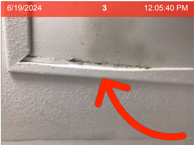
Ceiling | Cracks in ceiling.
