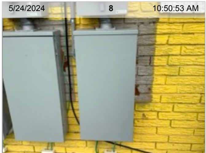
Electrical Breaker Panel
