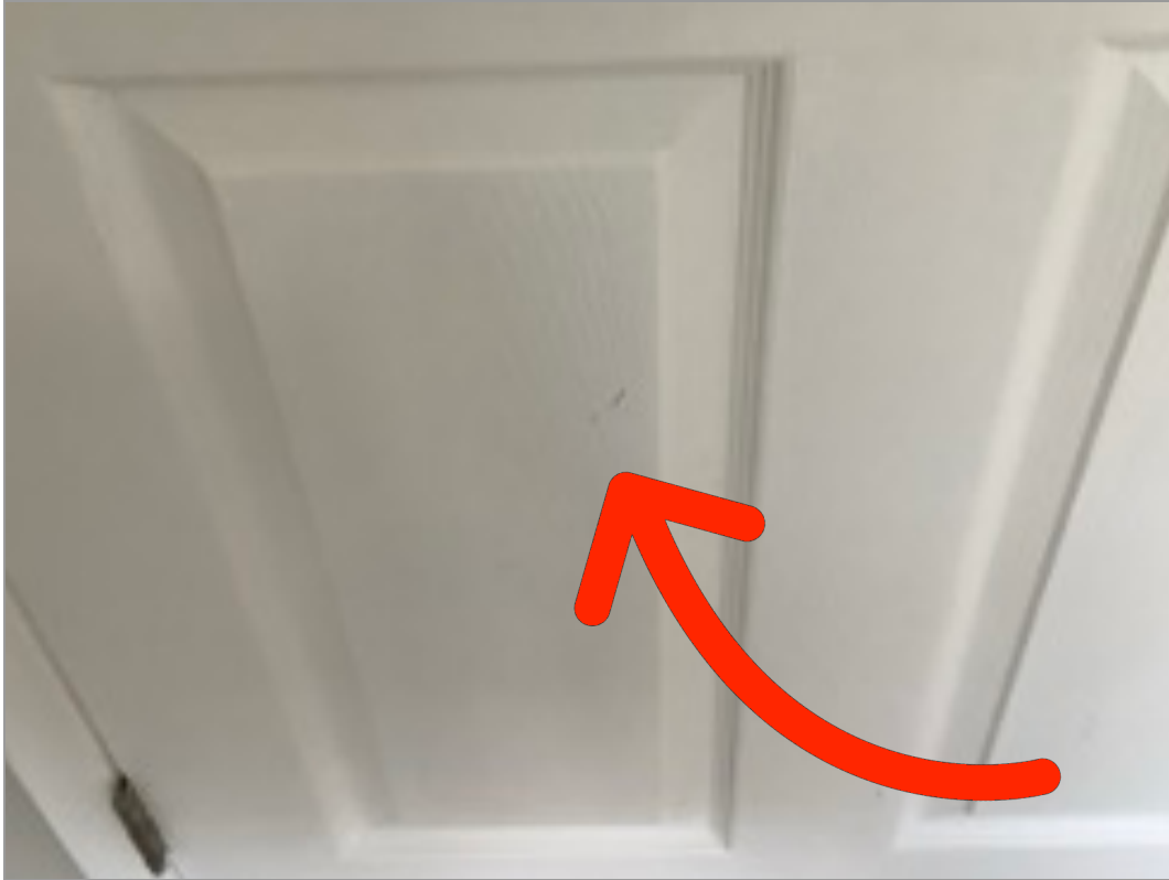
Bedroom 2 Door Scuffs on door.
