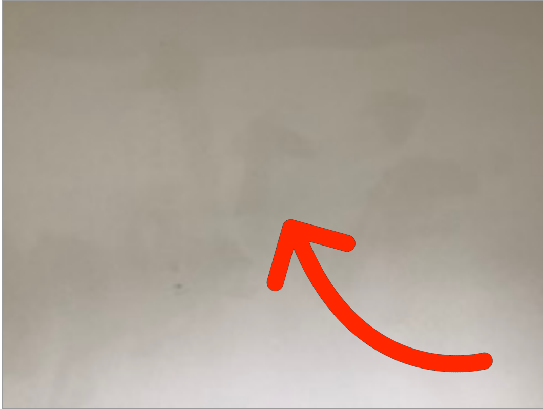
Entry Walls/Paint The wall is discolored
