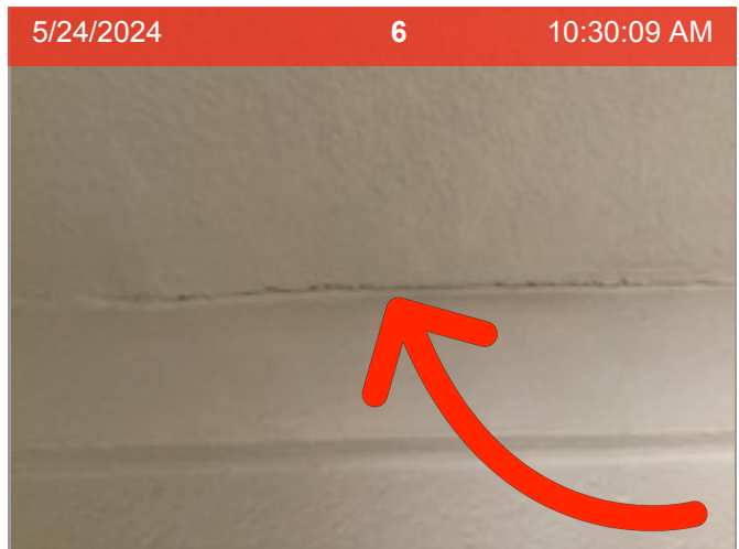
Closets | Cracks in ceiling
