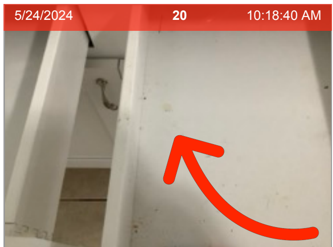
Lower Cabinets - Interior | Base of the cabinet is discolored
