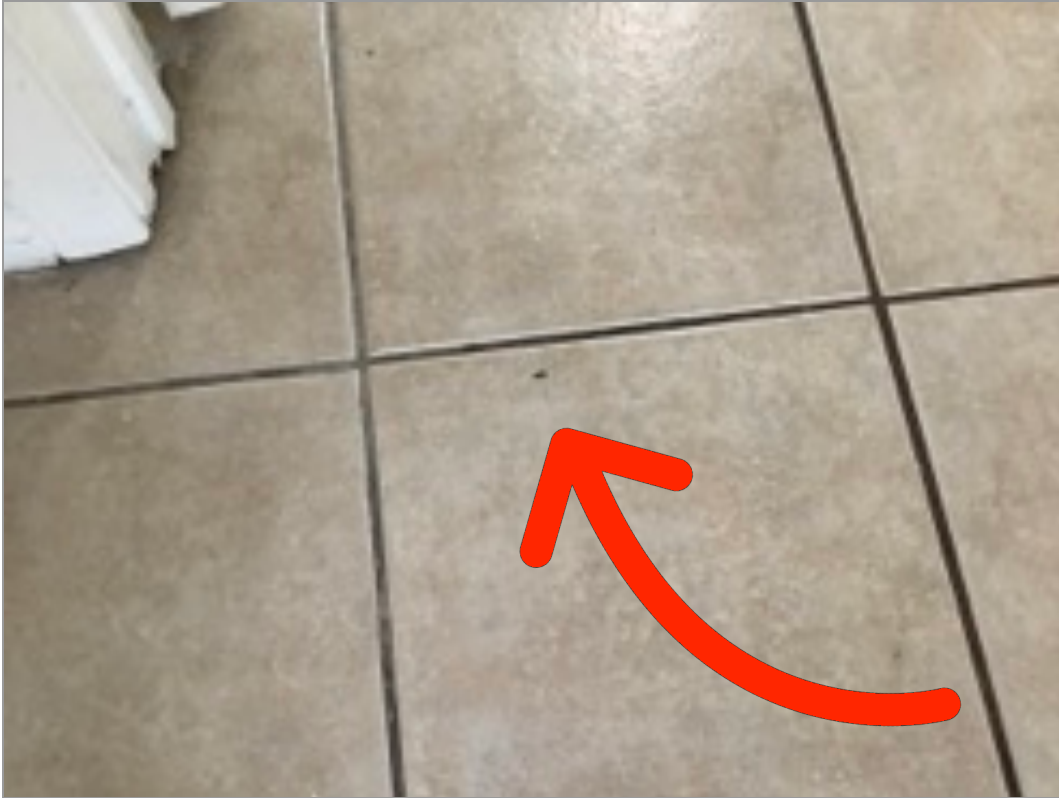
Hallway/Stairway Floors Gap in flooring.
