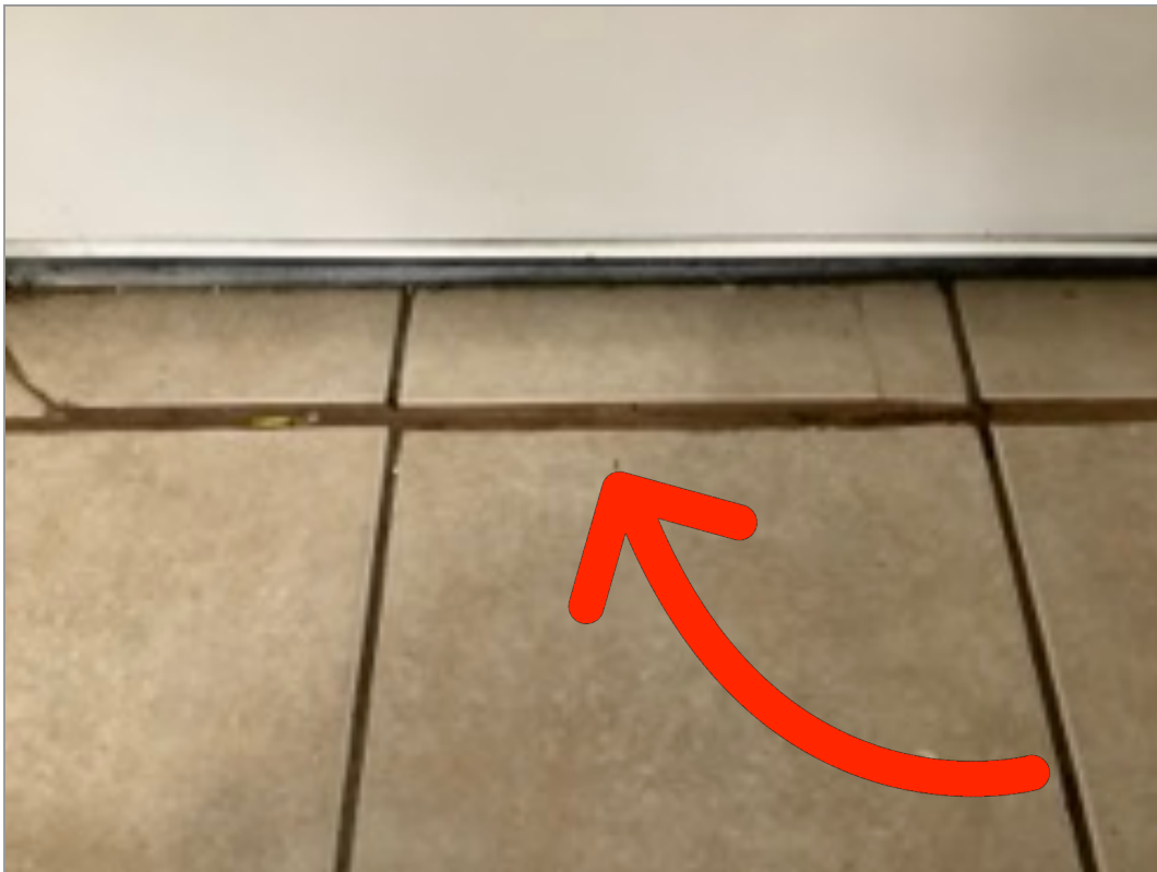
Kitchen Floors Gap in flooring.
