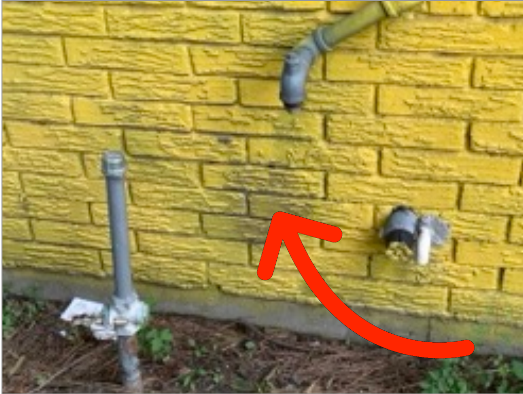
Rear Exterior Walls/Siding/Trim Siding is discolored
