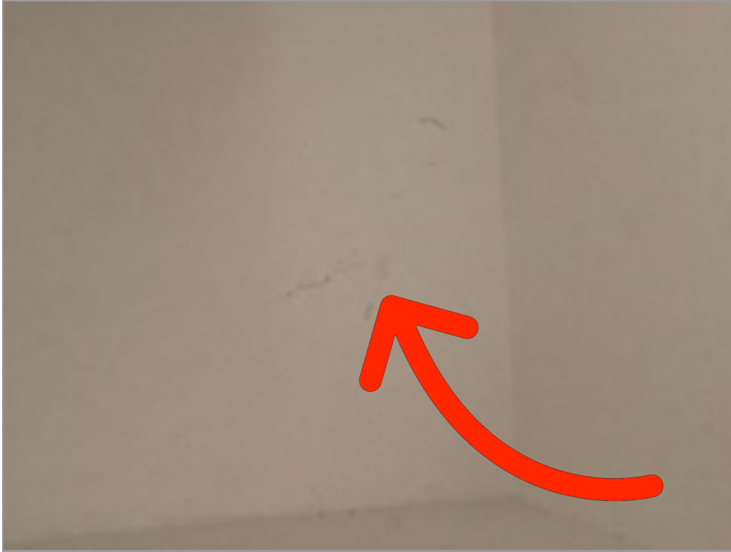
Kitchen Pantry The walls are marked up.
