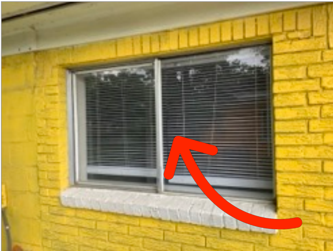
Rear Exterior Window Screens Screen(s) are missing
