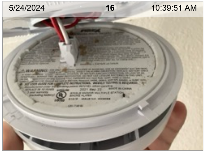
Wired Smoke Alarm (mfd 9/2021) | Smoke test: Passed | Close-up of printed manufacture date | 2.7 years old
