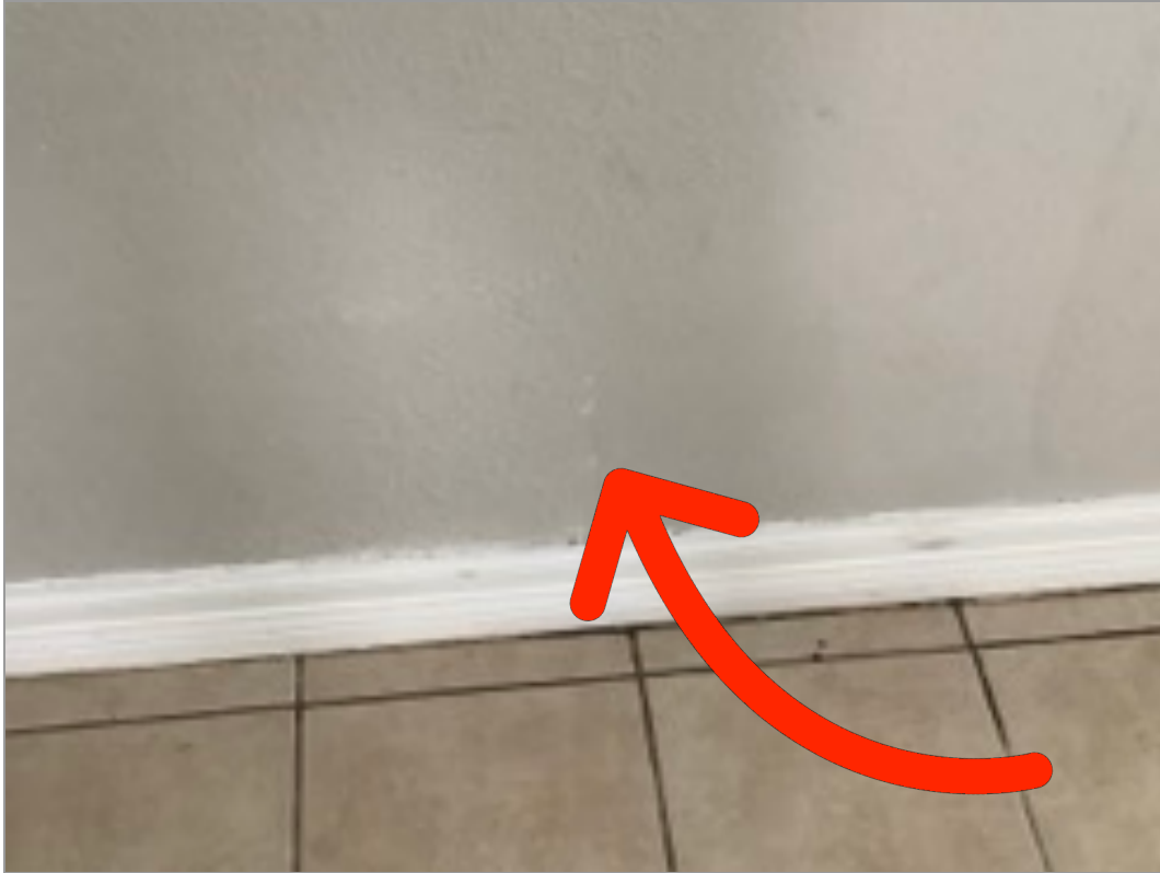
Bedroom 1 Walls/Paint Scratches on the wall
