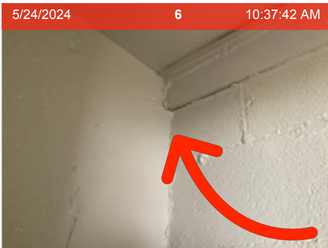
Closets | Cracks in texture
