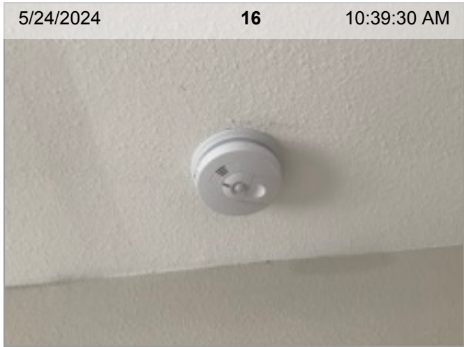
Wired Smoke Alarm (mfd 9/2021) | Smoke test: Passed | Alarm in place
