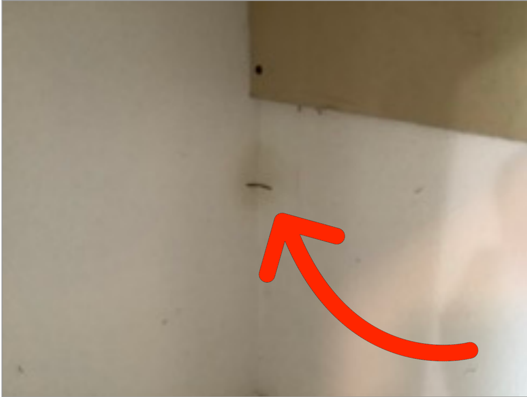
Hallway/Stairway Closets The walls are marked up.
