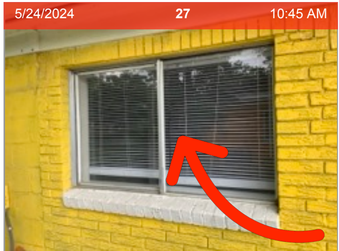
Window Screens | Screen(s) are missing
