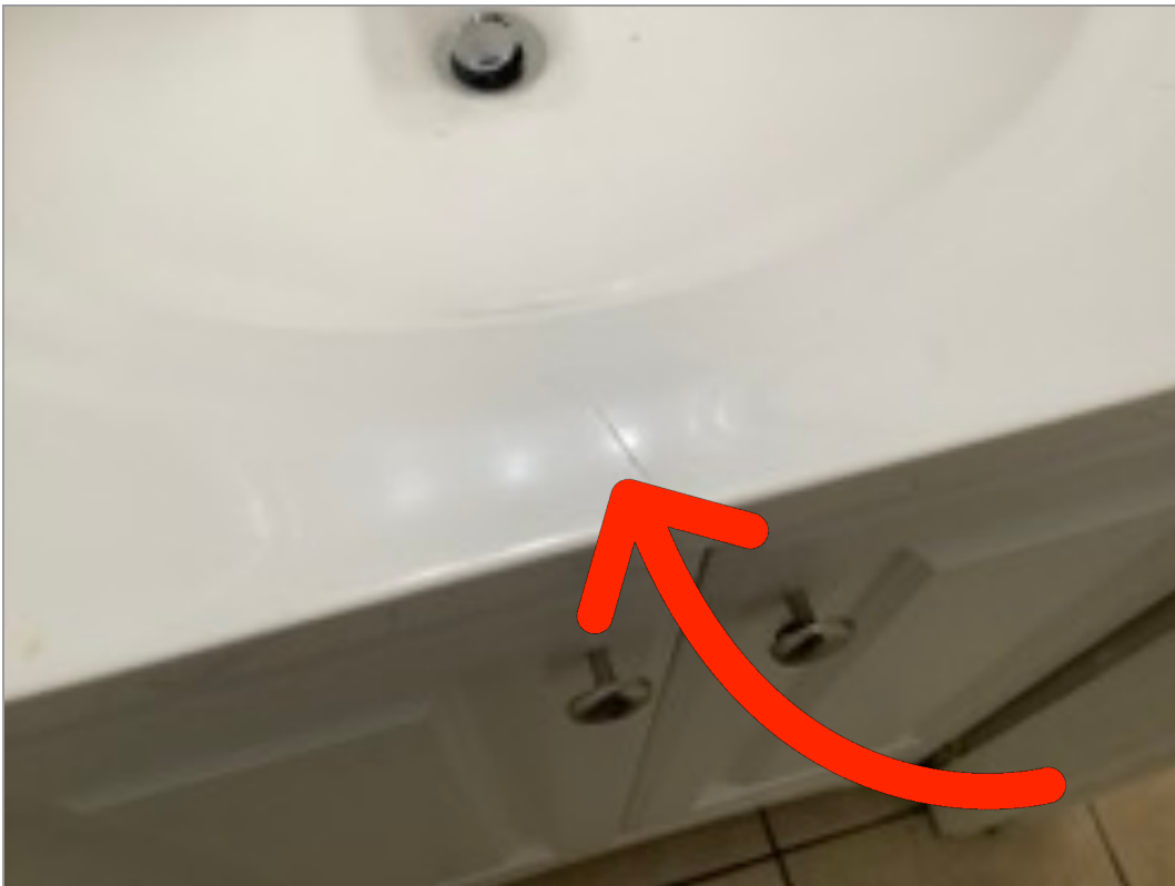
Bathroom 1 Sink/Faucet Cracking front part of sink
