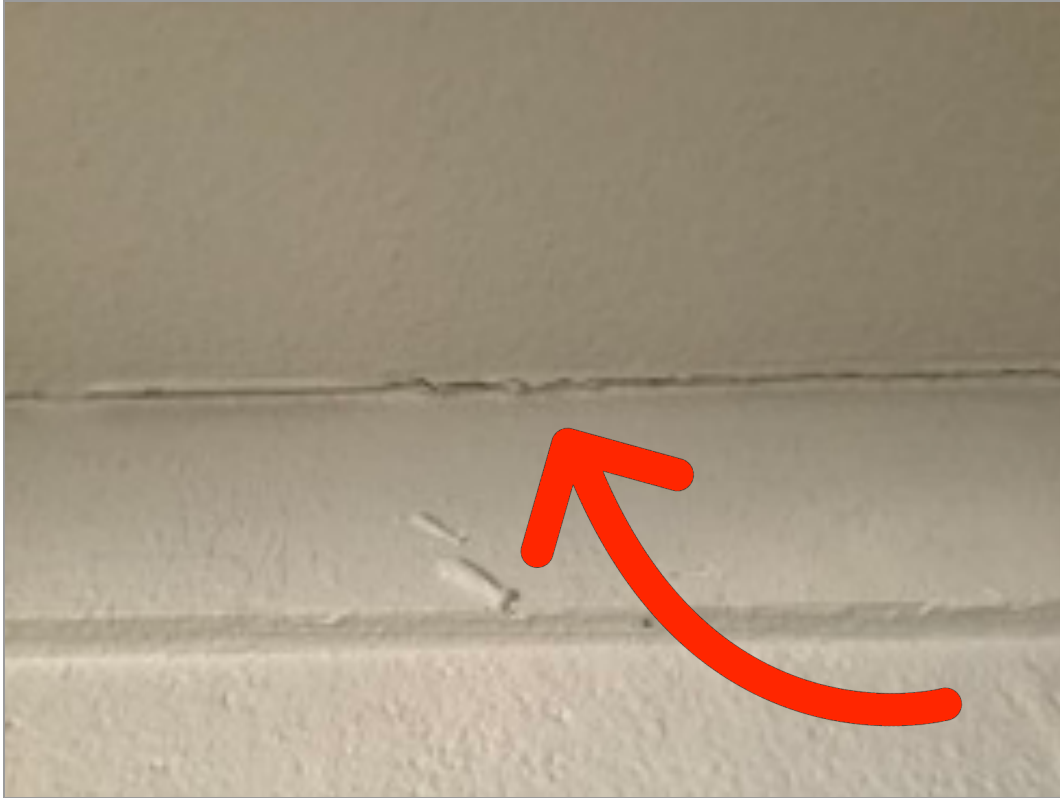
Bedroom 1 Closets Cracks in ceiling
