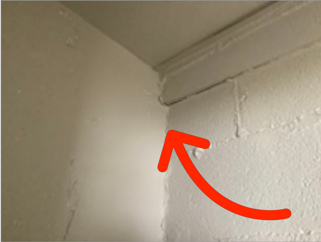
Bedroom 2 Closets Cracks in texture
