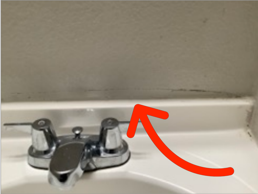
Bathroom 1 Walls/Paint Scratches on the wall
