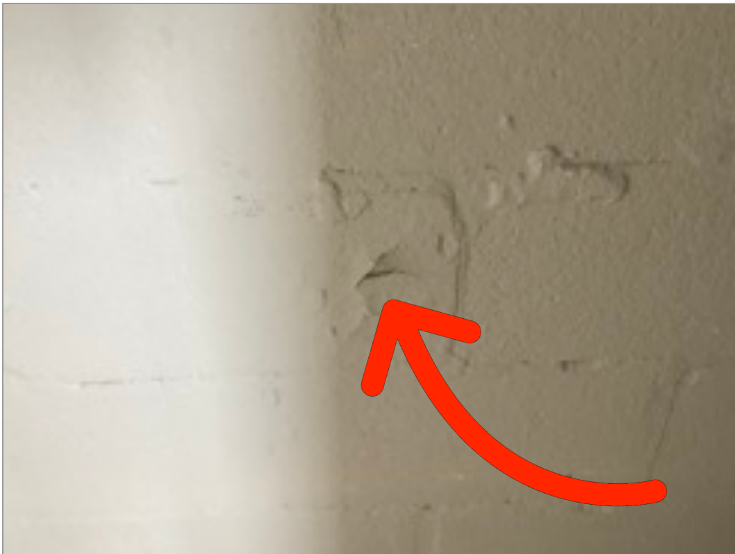
Bedroom 2 Closets Cracks in texture
