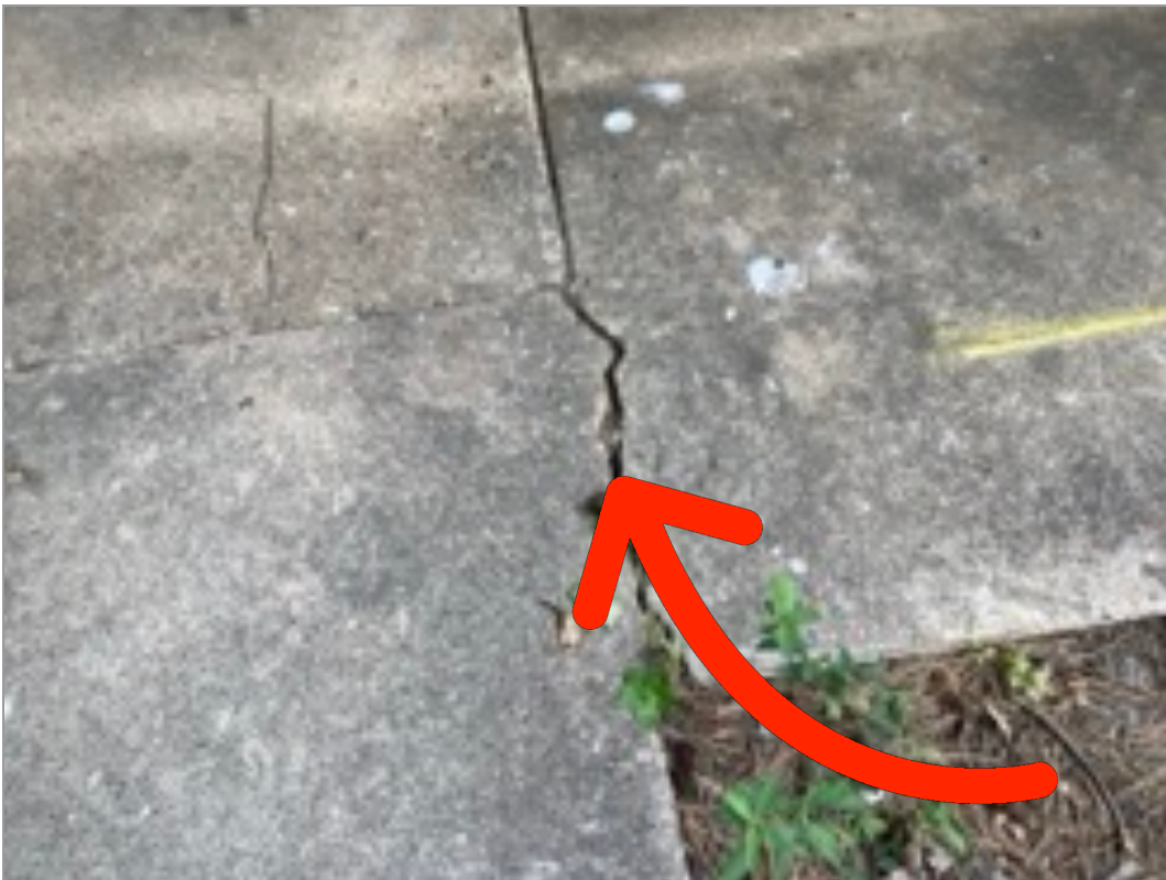
Rear Exterior Porch/Patio/Deck Cracked concrete
