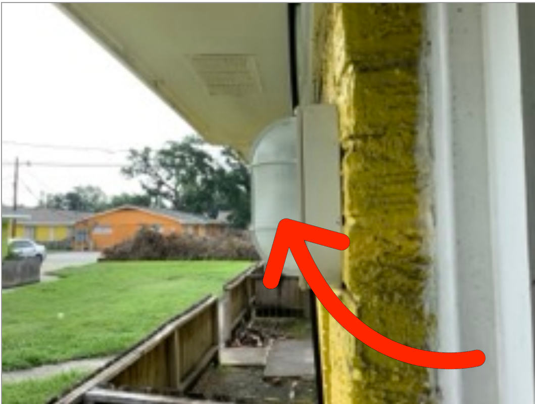
Front Exterior Light Fixtures Bulb is out
