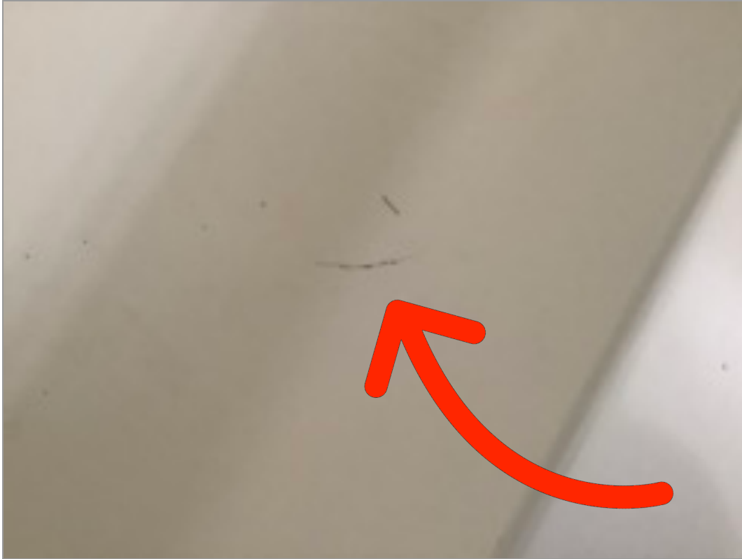
Bathroom 1 Tub/Fixture The floor is discolored around the base of the tub.
