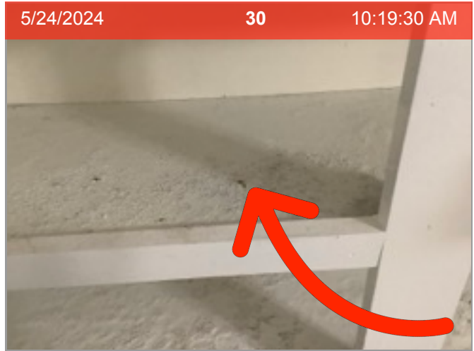
Upper Cabinets - Interior | Base of the cabinet is discolored
