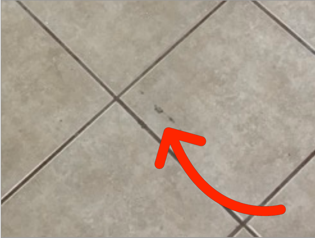
Bedroom 1 Floors Flooring is scratched.
