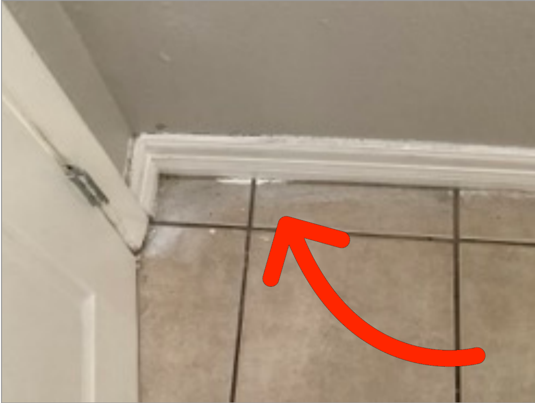
Bathroom 1 Floors Flooring is stained.
