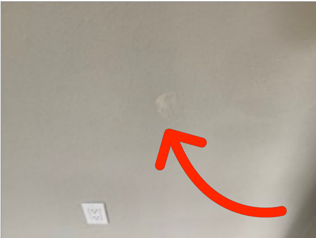
Entry Walls/Paint The wall is discolored
