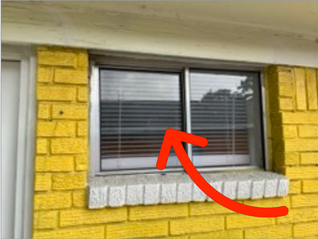
Rear Exterior Window Screens Screen(s) are missing
