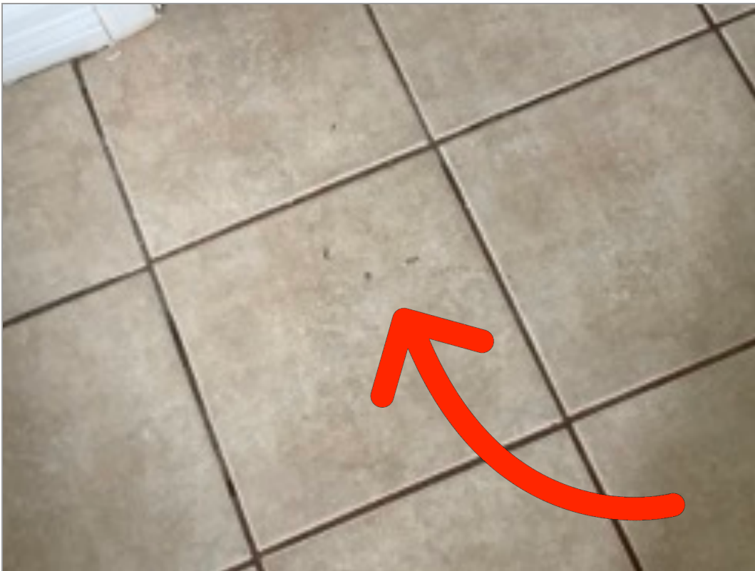
Bedroom 1 Floors Flooring is scratched.
