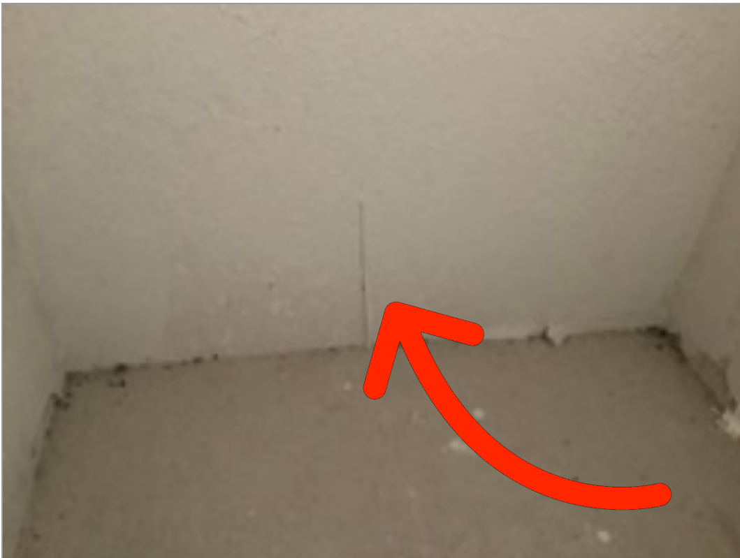
Laundry Room Walls/Paint Scratches on the wall
