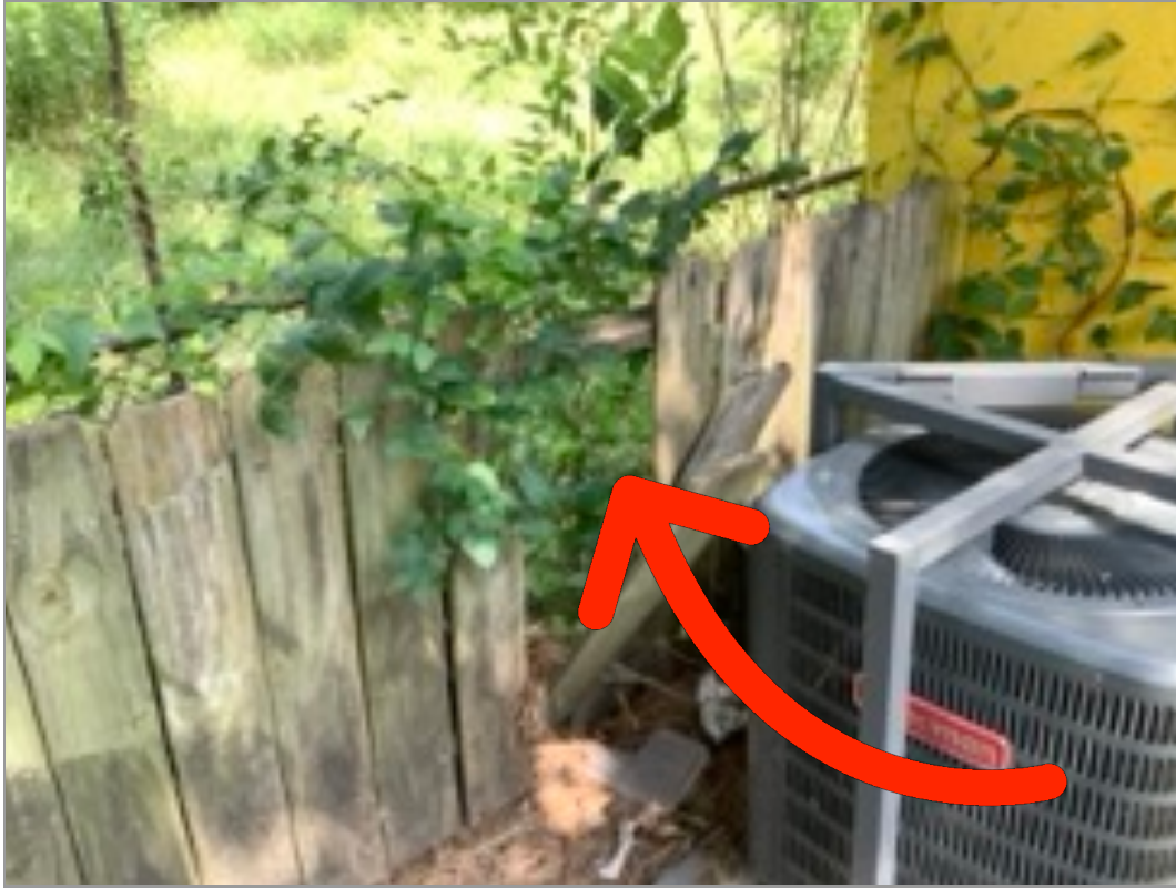
Rear Exterior Fence Damaged, rotten, or chipping fence materials; holes/gaps in fence; damaged clasps; gates that don't close securely
