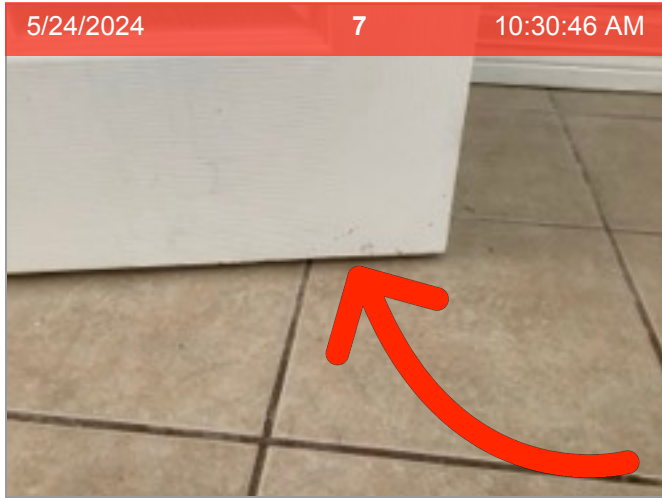
Door | Scuffs on door.
