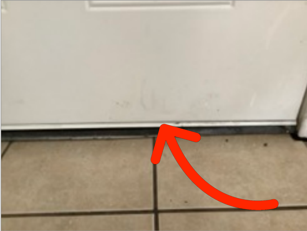
Entry Front Door Interior Scuffs on door
