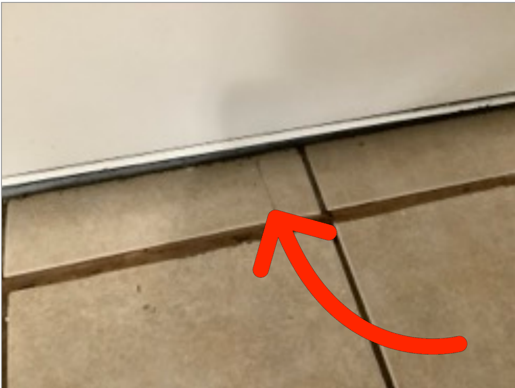
Kitchen Floors Crack in flooring.
