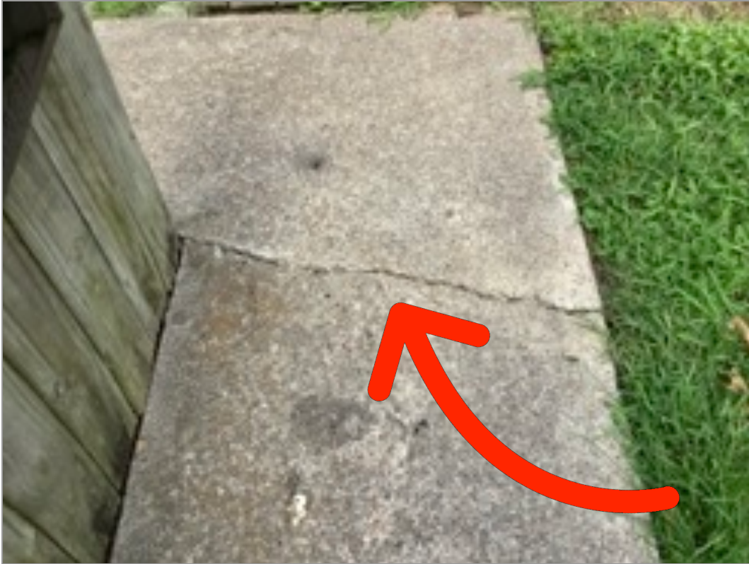
Front Exterior Walkways Cracked or uneven
