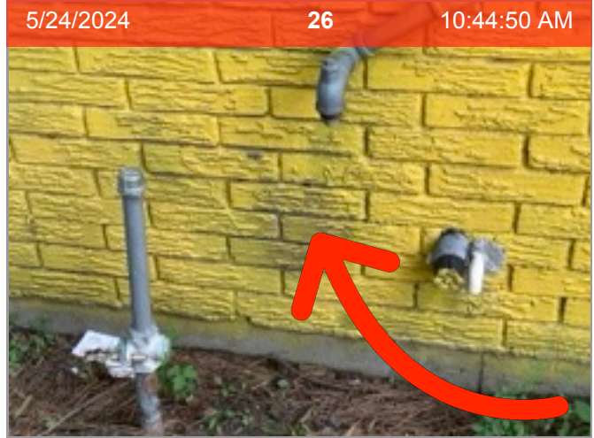
Walls/Siding/Trim | Siding is discolored
