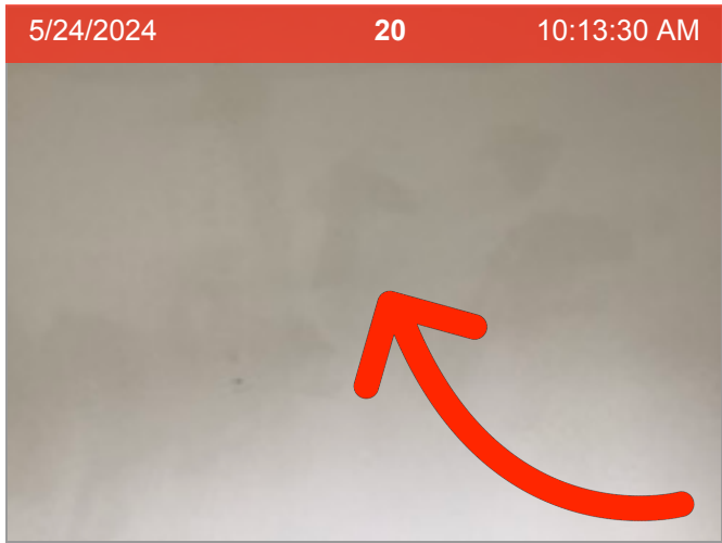
Walls/Paint | The wall is discolored
