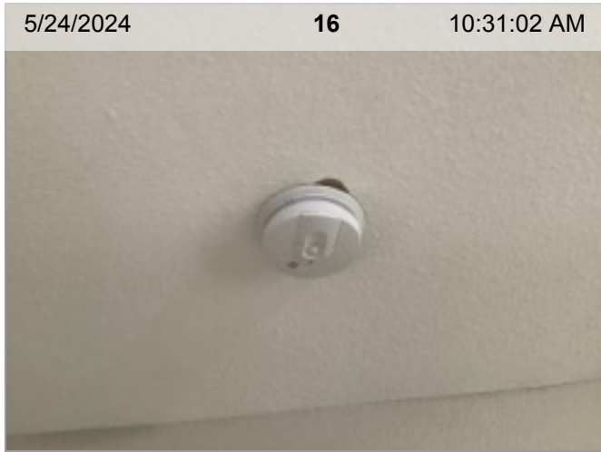
Wired Smoke Alarm (mfd 4/2021) | Smoke test: Passed | Alarm in place
