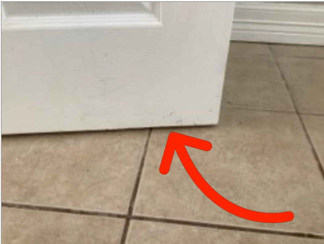
Bedroom 1 Door Scuffs on door.
