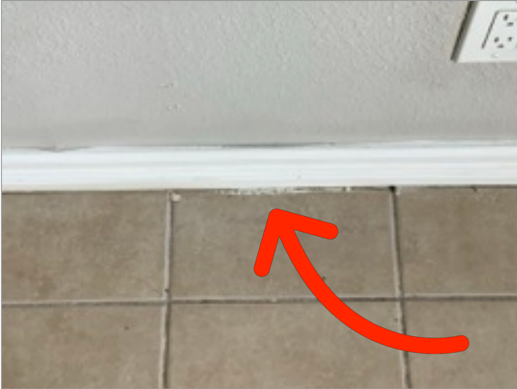
Entry Floors Flooring is stained.
