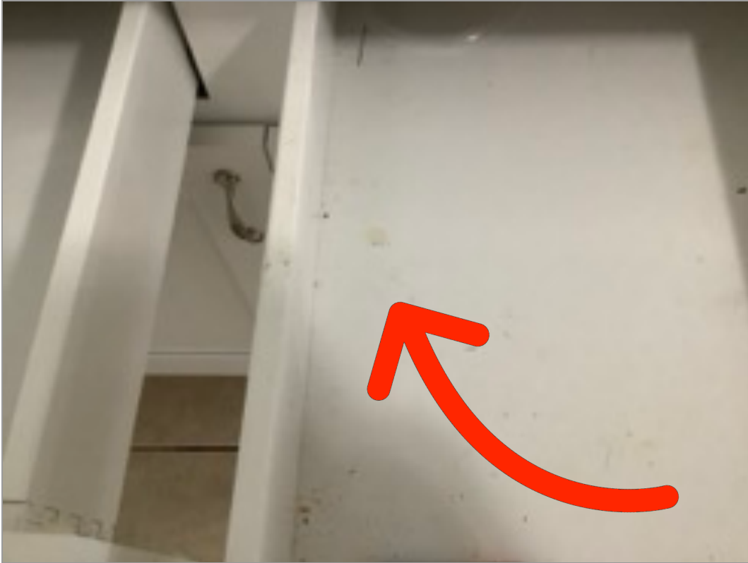
Kitchen Lower Cabinets - Interior Base of the cabinet is discolored
