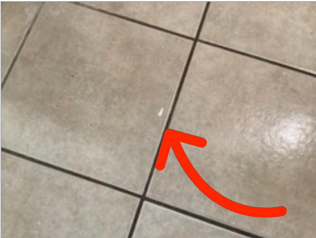
Hallway/Stairway Floors Flooring is stained.
