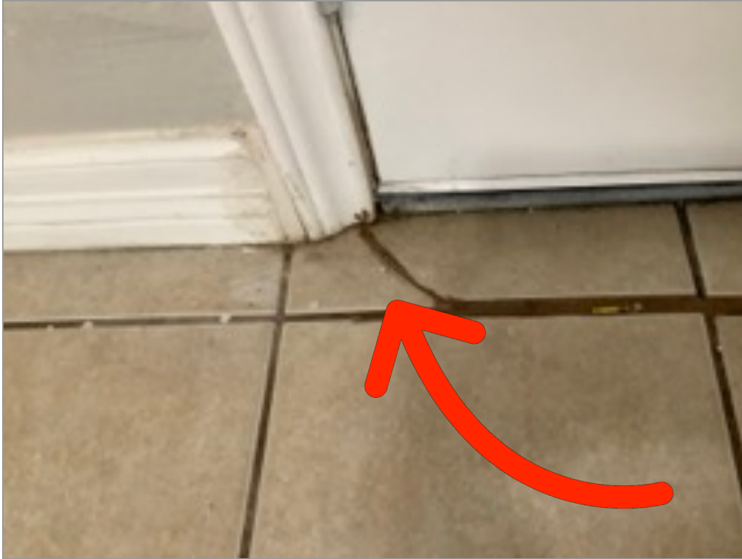
Kitchen Floors Crack in flooring.
