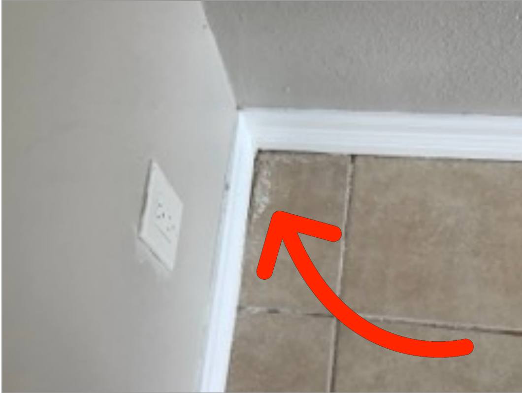
Bedroom 2 Floors Flooring is stained.
