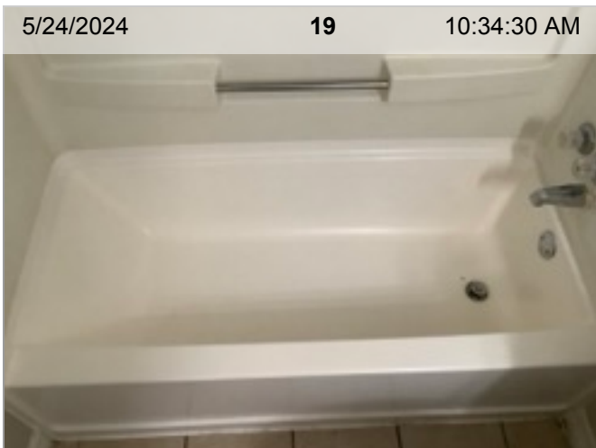
Tub/Fixture | Base of Tub
