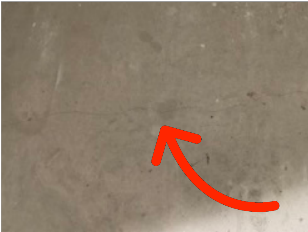
Laundry Room Floors Crack in flooring.
