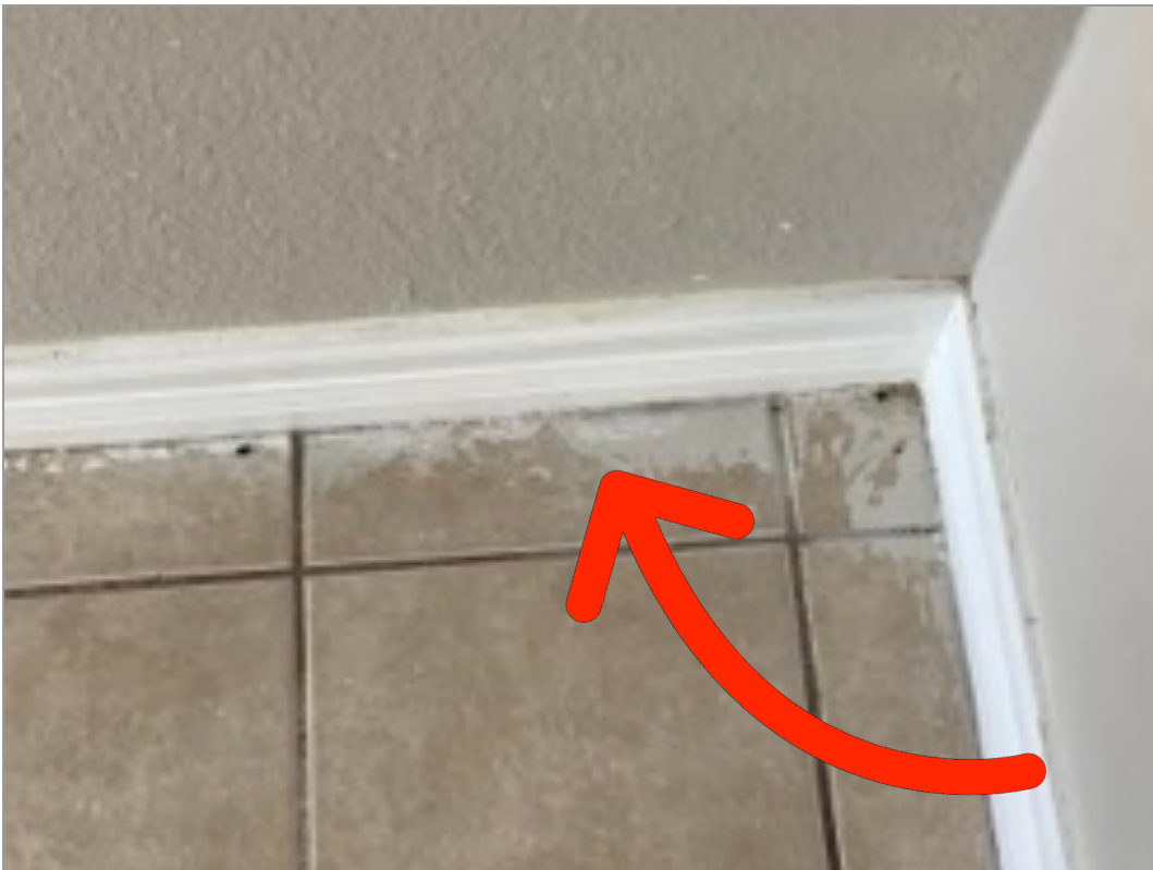
Entry Floors Flooring is stained.
