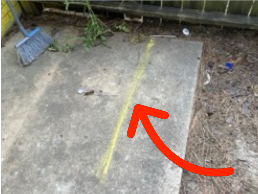
Rear Exterior Porch/Patio/Deck Discoloration
