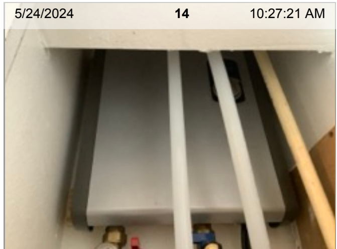
Inaccessible Water Heater | NA | Water heater (with expansion tank if present) | Cannot access full water heater
