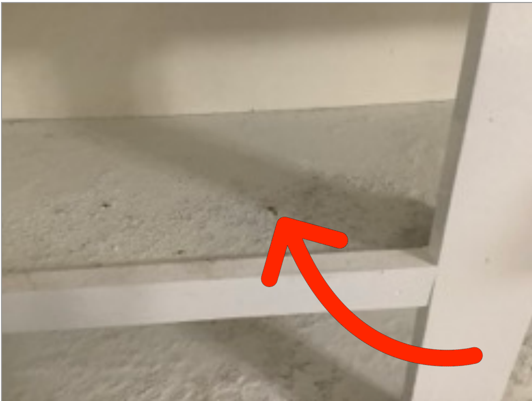
Kitchen Upper Cabinets - Interior Base of the cabinet is discolored
