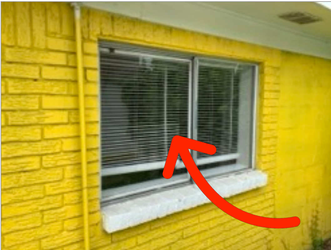
Front Exterior Window Screens Screen(s) are missing
