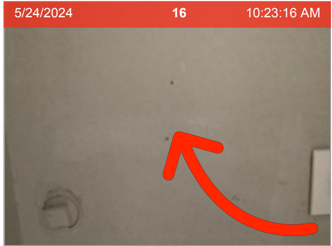
5/24/2024 16 10:23:16 AM Walls/Paint | Holes in wall.
