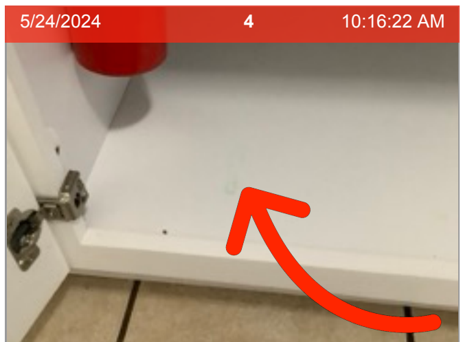
Cabinet Under Sink | The base of the cabinet is discolored. |
