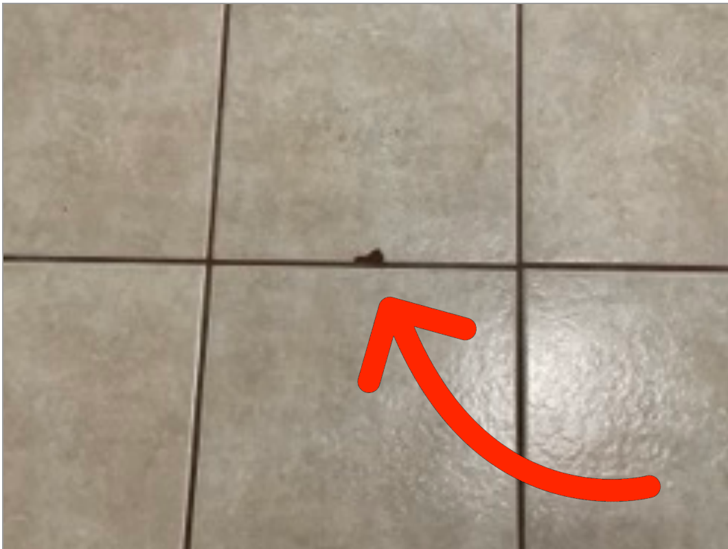
Bedroom 1 Floors Gap in flooring.
