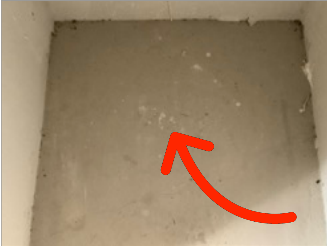
Laundry Room Floors Flooring is stained.
