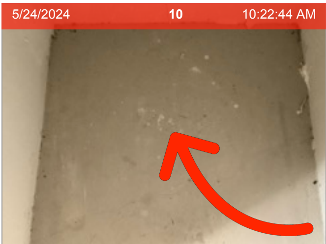
Floors | Flooring is stained.
