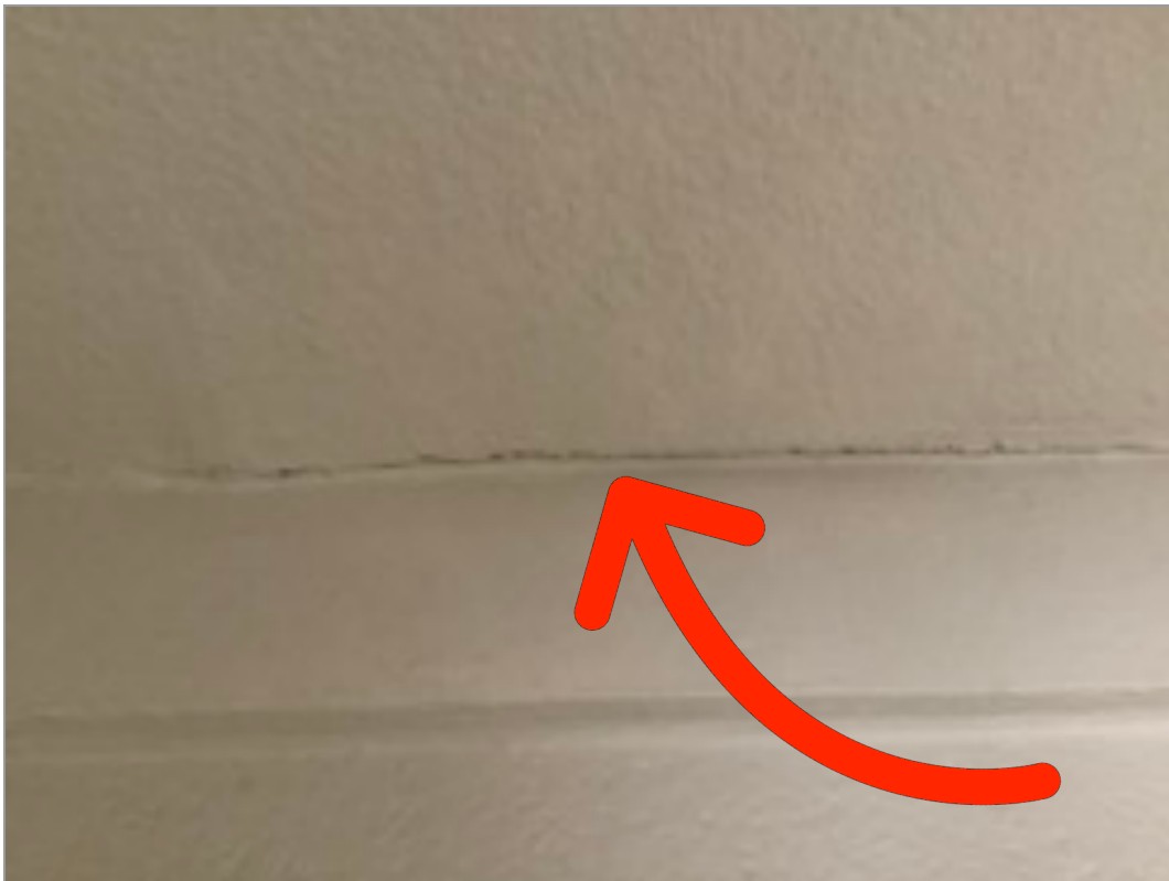
Bedroom 1 Closets Cracks in ceiling
