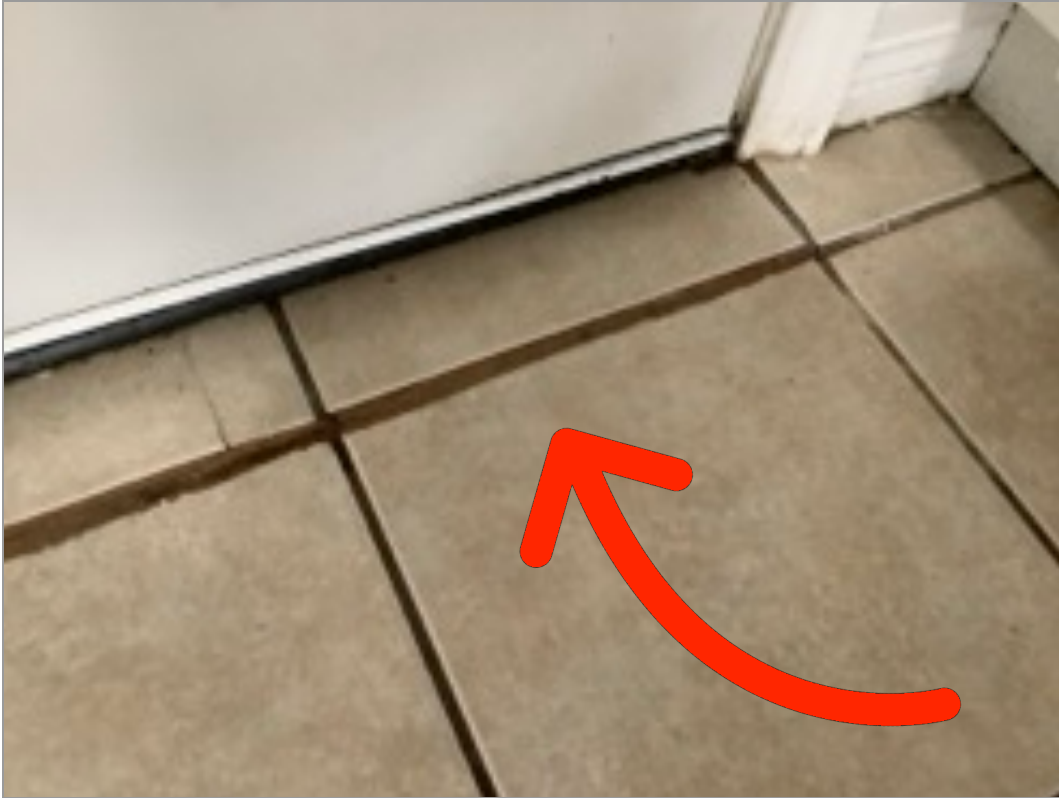
Kitchen Floors Gap in flooring.
