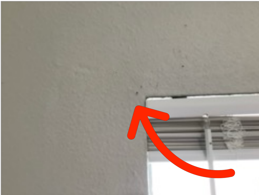
Bedroom 2 Walls/Paint Holes in wall.
