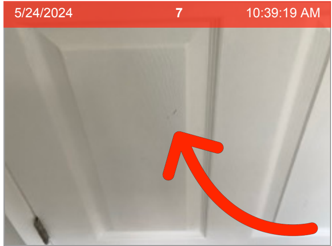
Door | Scuffs on door.
