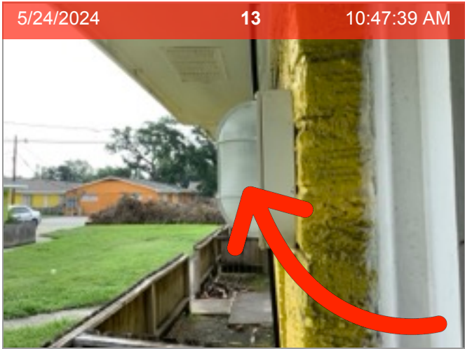
Light Fixtures | Bulb is out
