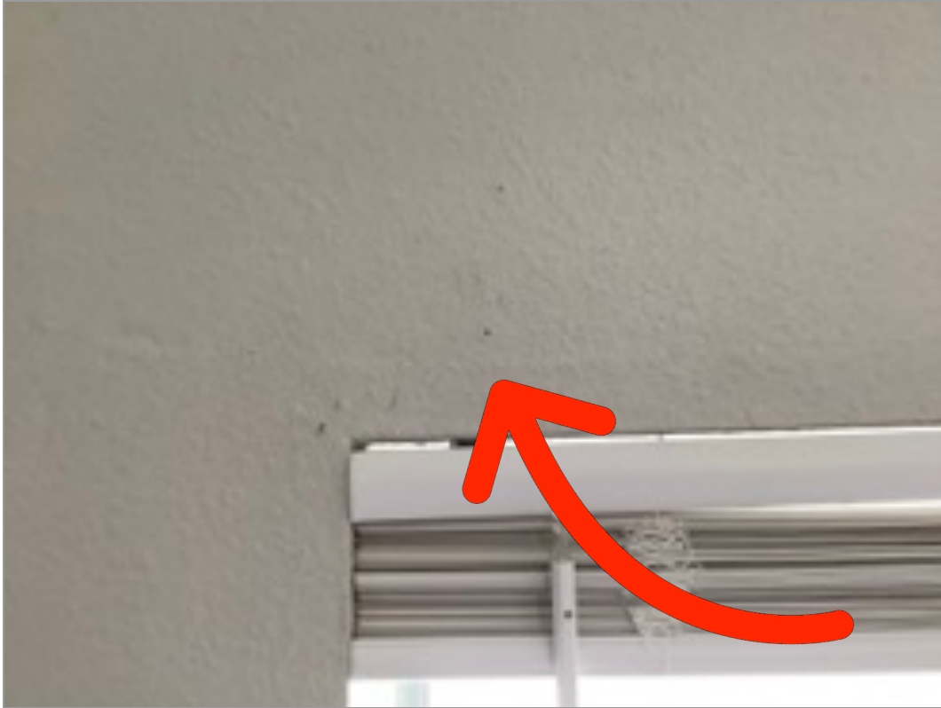
Bedroom 2 Walls/Paint Holes in wall.
