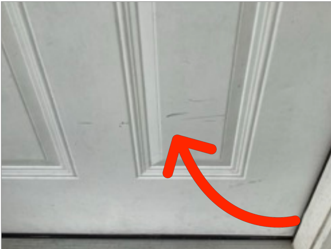
Entry Front Door Exterior Scratches; stains; discoloration or chipping of door casing
