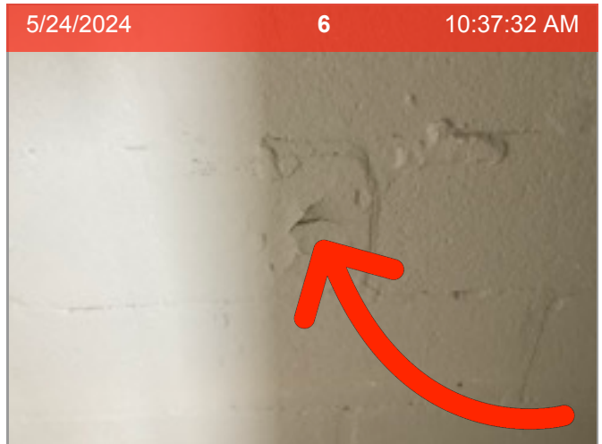
Closets | Cracks in texture
