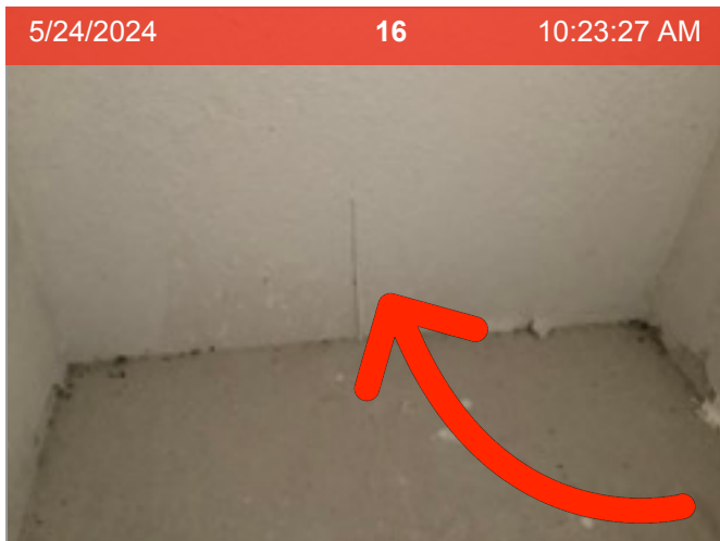
5/24/2024 16 10:23:27 AM Walls/Paint | Scratches on the wall
