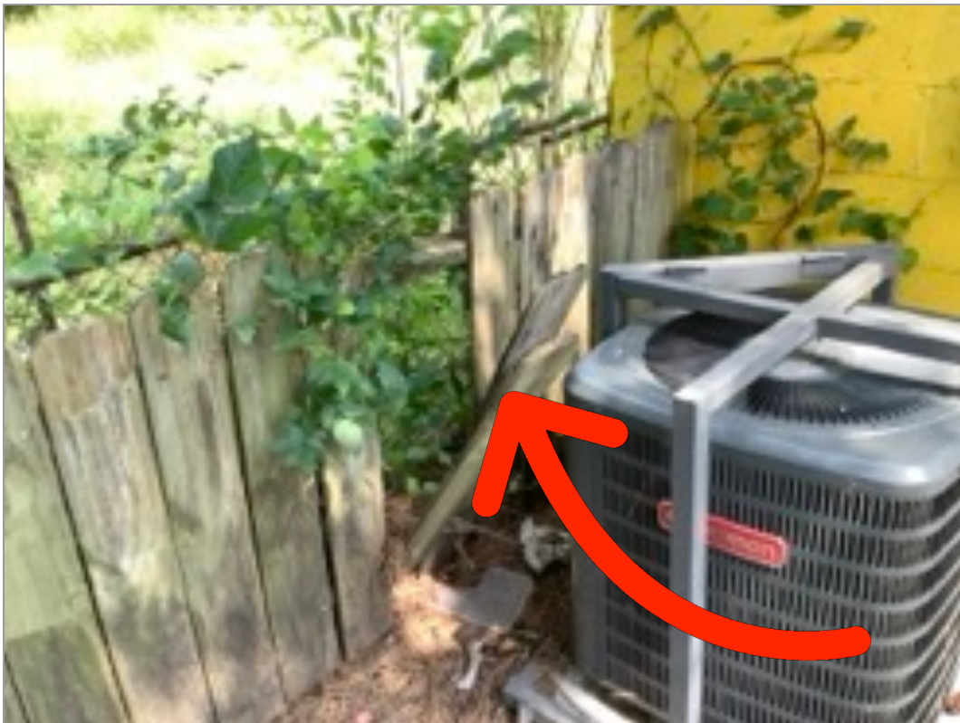
Rear Exterior Fence Fence is leaning and needs attention.
