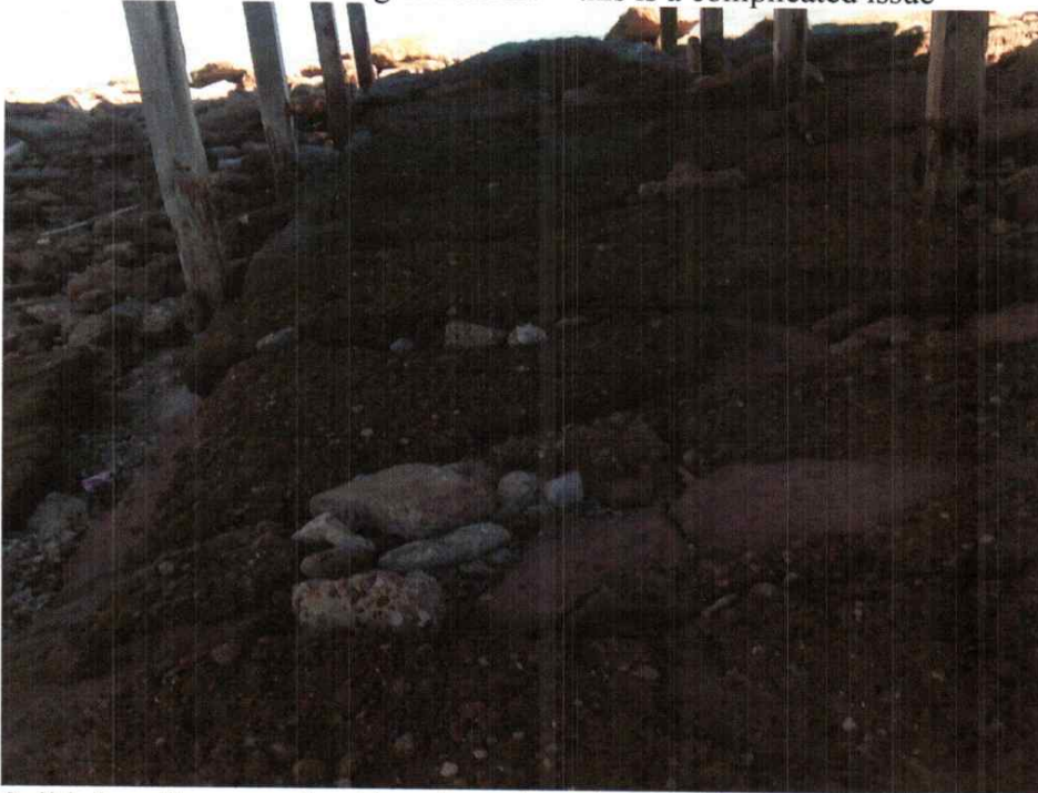
Soil is heavily scoured – this reduces lateral support capacity
