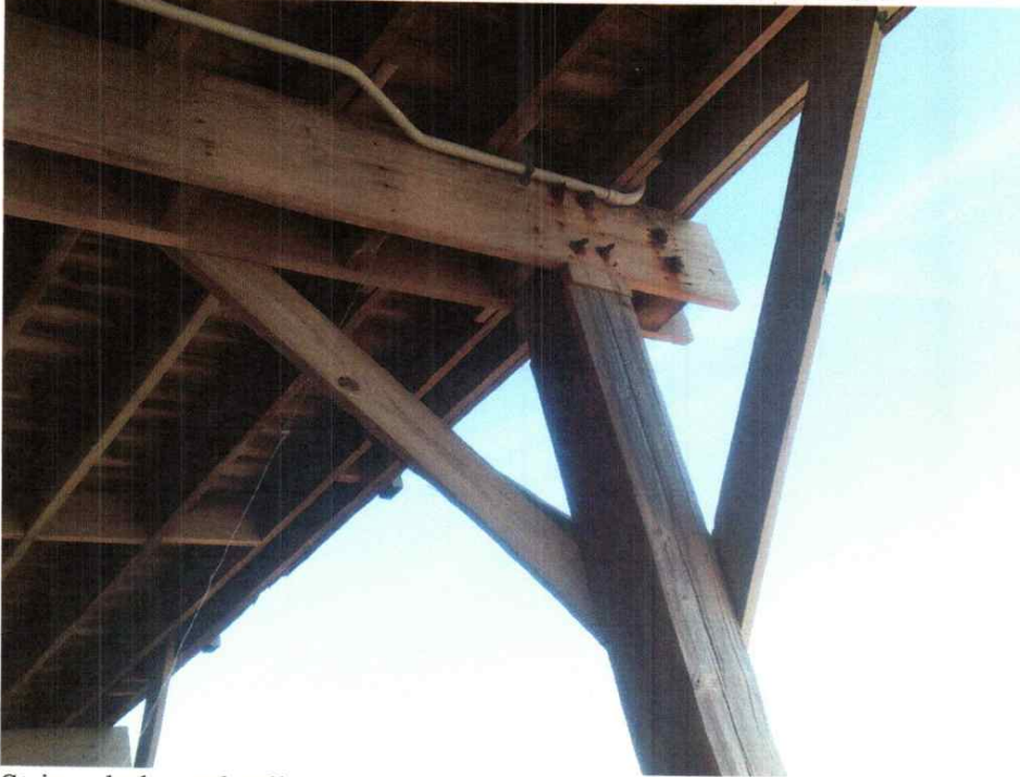
Stringer bolts and nails are severely rusted
