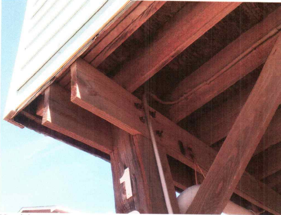
Note joists are not connected to stringer with metal fittings
