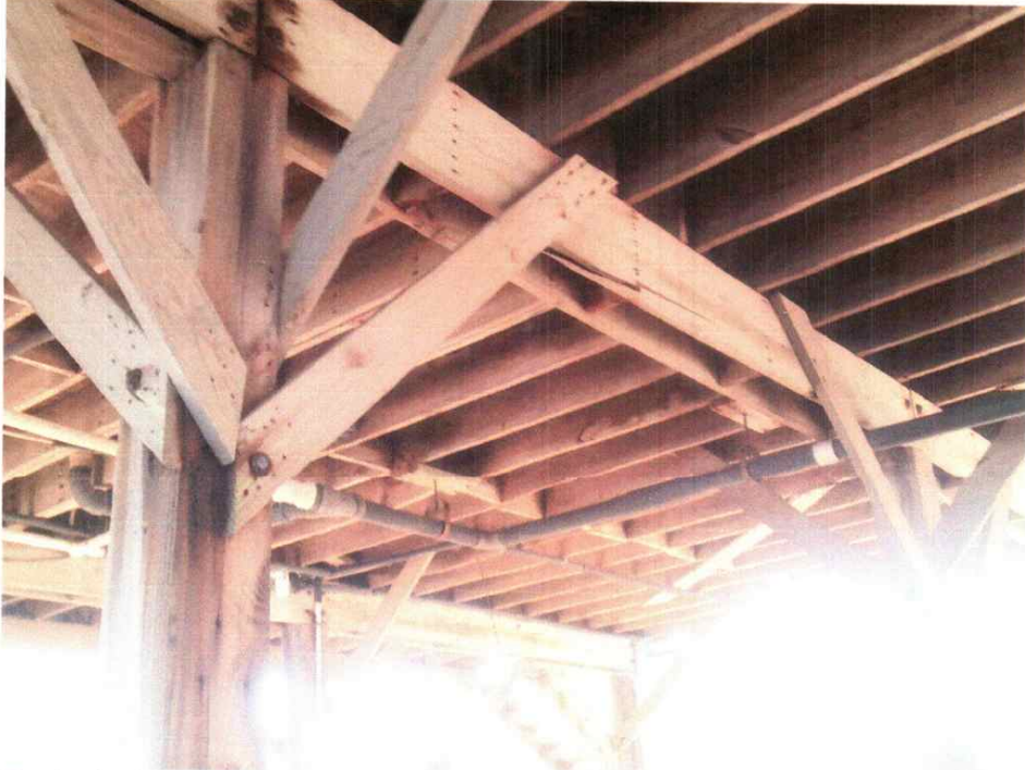
Typical ad hoc bracing scheme – note sistered joists with inadequate overlap
