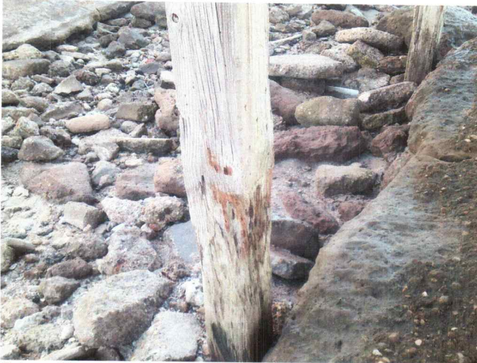
Column thinned by scouring, note deteriorated wood – all columns are severely Deteriorated due to aging in the salt water environment
