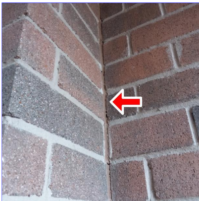
E. Item 12 (Picture) Next to front door
