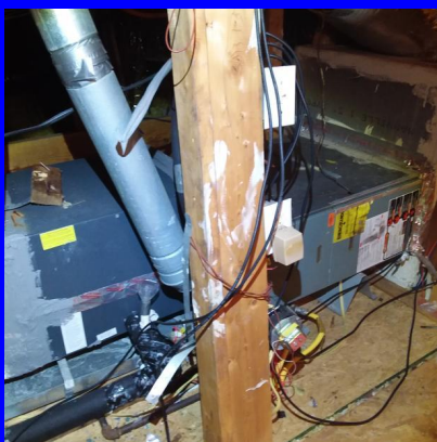
Gas furnace/air handler located in attic
