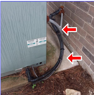
B. Item 6 (Picture) Suction line at condenser
