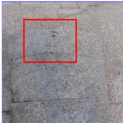
C. Item 12 (Picture) Multiple areas throughout roof
