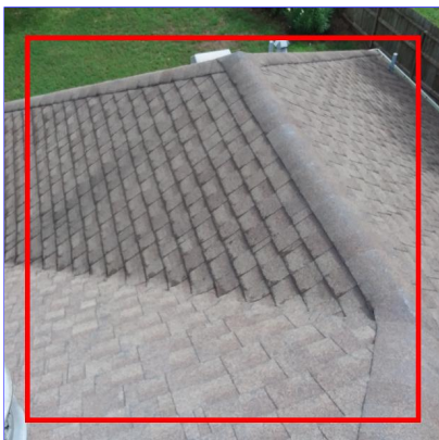
C. Item 7 (Picture) All throughout roof
