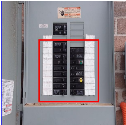
A. Item 5 (Picture) Main panel
