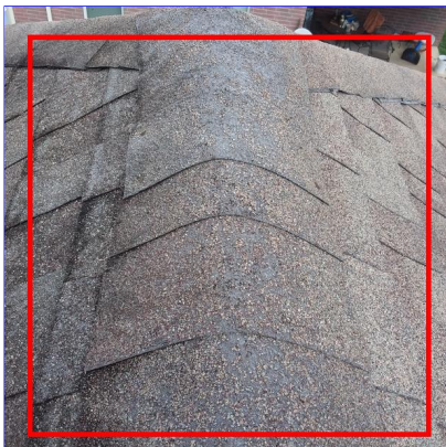
C. Item 5 (Picture) Throughout roof
