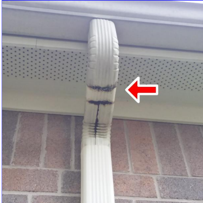
B. Item 1 (Picture) Multiple gutters
