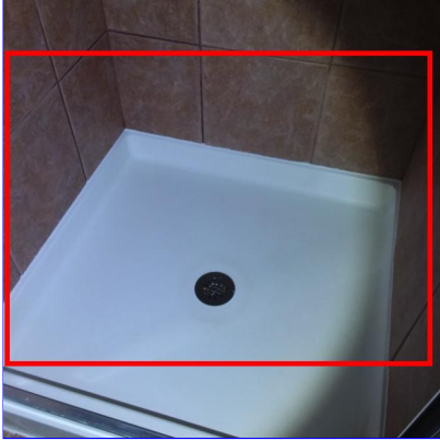
E. Item 20 (Picture) Master shower
