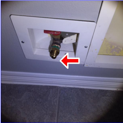
E. Item 1 (Picture) Dryer line in laundry room
