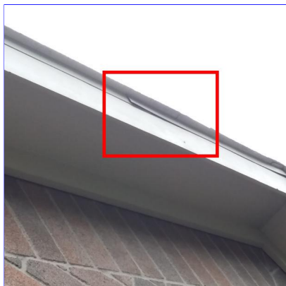
C. Item 1 (Picture) Drip edge flashing in the front
