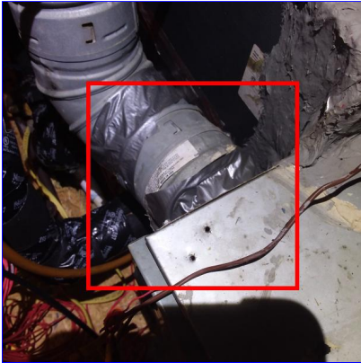
A. Item 1 (Picture) Furnace flue in attic
