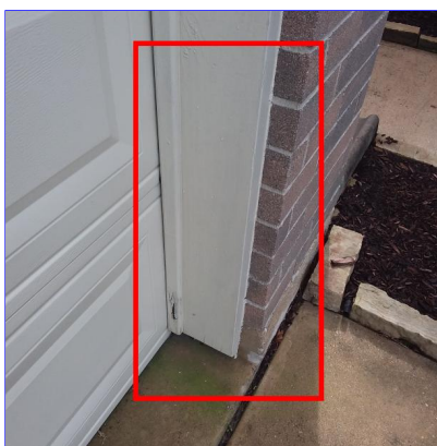
E. Item 18 (Picture) Around garage door
