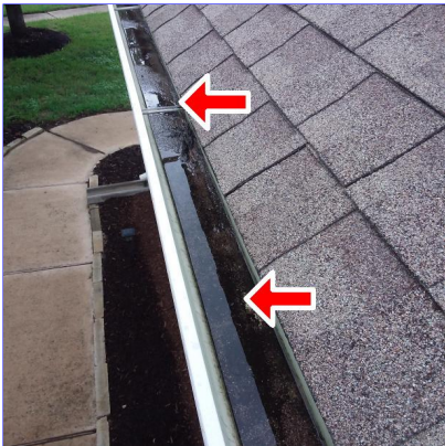
B. Item 15 (Picture) Multiple areas
