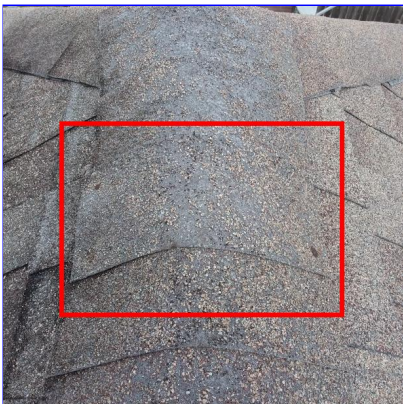
C. Item 11 (Picture) Multiple areas throughout roof
