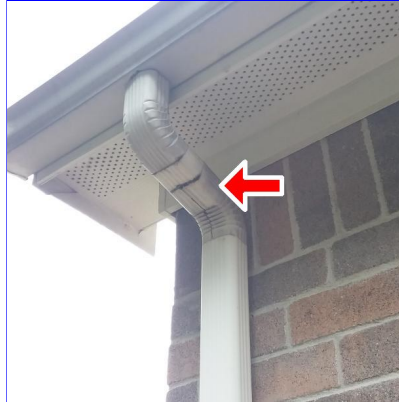
B. Item 2 (Picture) Multiple gutters around home
