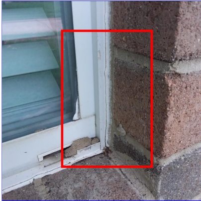
E. Item 1 (Picture) Multiple areas in window frames around home perimeter
