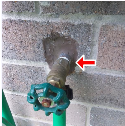
A. Item 2 (Picture) Exterior faucets
