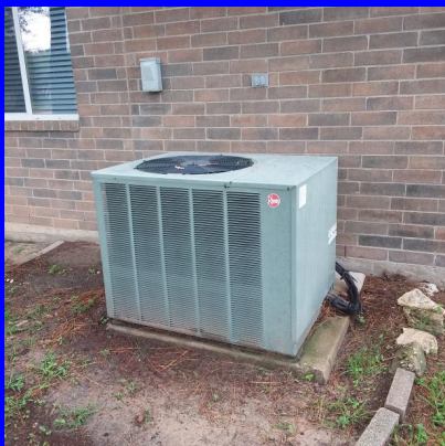
Exterior HVAC condenser located on the right side of the home
