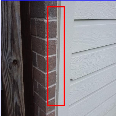
E. Item 5 (Picture) Multiple areas around home perimeter
