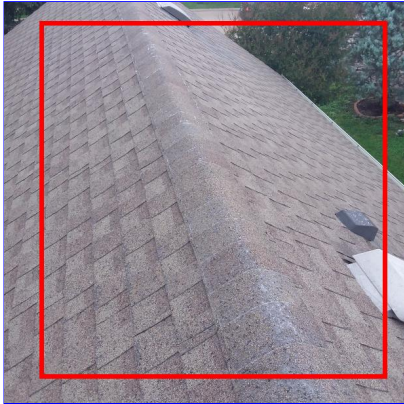
C. Item 3 (Picture) Throughout roof
