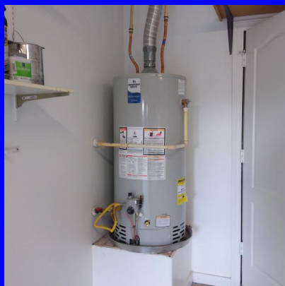
Gas water heater located in the garage
