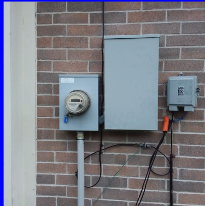
Below ground service and main panel located on the left side of the home
