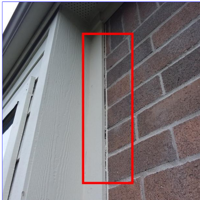
E. Item 4 (Picture) Multiple areas around home perimeter
