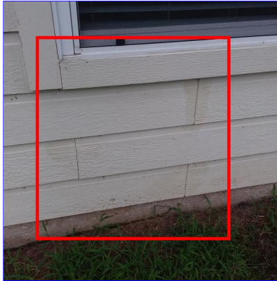
E. Item 6 (Picture) Gaps between siding boards and exterior window frames
