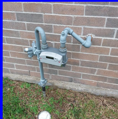
Gas meter is located on the left side of the home
