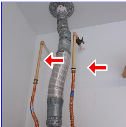
A. Item 3 (Picture) Water heater
