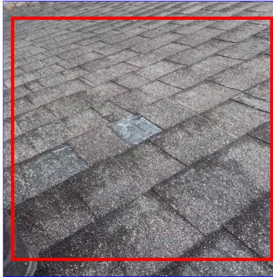
C. Item 4 (Picture) Throughout roof
