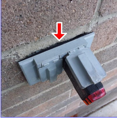
B. Item 6 (Picture) Exterior next to condenser
