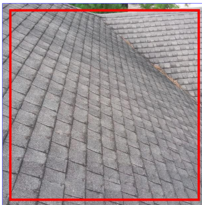
C. Item 8 (Picture) All throughout roof
