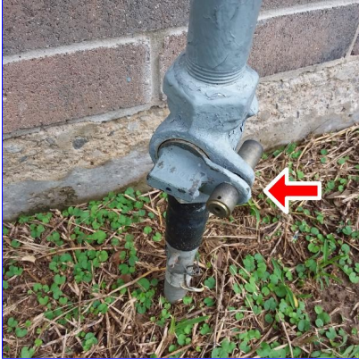
E. Item 4 (Picture) Gas meter
