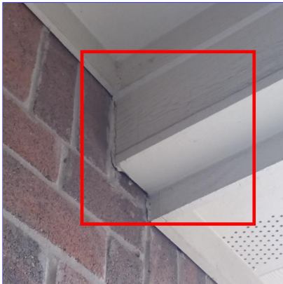
E. Item 3 (Picture) Multiple areas around home perimeter
