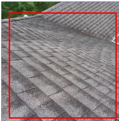
C. Item 6 (Picture) Throughout roof
