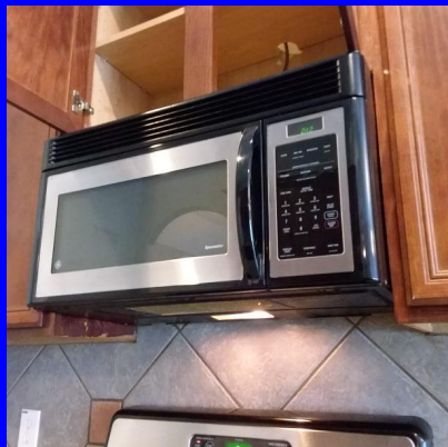
Vent hood and microwave
