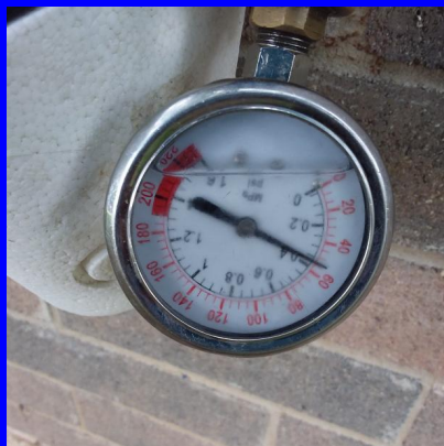
Water pressure is 55 psi
