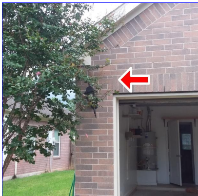
B. Item 9 (Picture) Garage light
