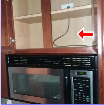
C. Item 1 (Picture) Range hood
