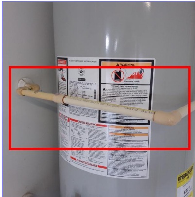
C. Item 3 (Picture) Water heater
