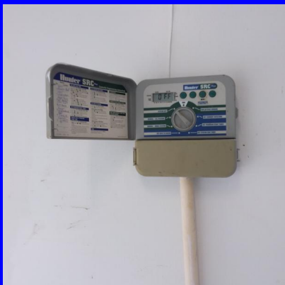
Sprinkler system control panel is located in the garage
