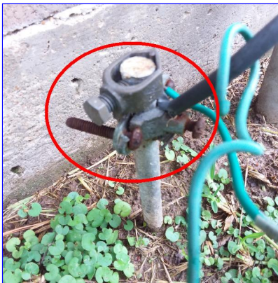
A. Item 3 (Picture) Grounding rod
