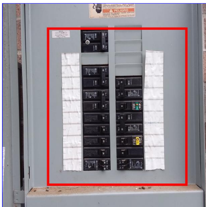
A. Item 1 (Picture) Main panel
