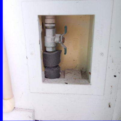
Main water shut off is located in the garage
