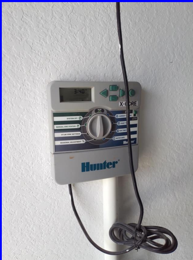
irrigation controls 7 zones
