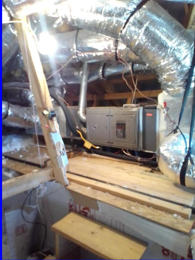
central air handler
