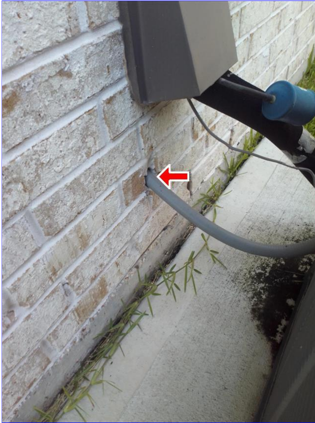
E. Item 3 (Picture) air condenser wall
