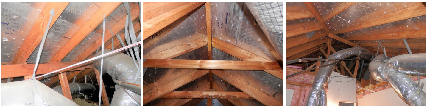
general view of the attic framing and support as seen from the limited walkway
