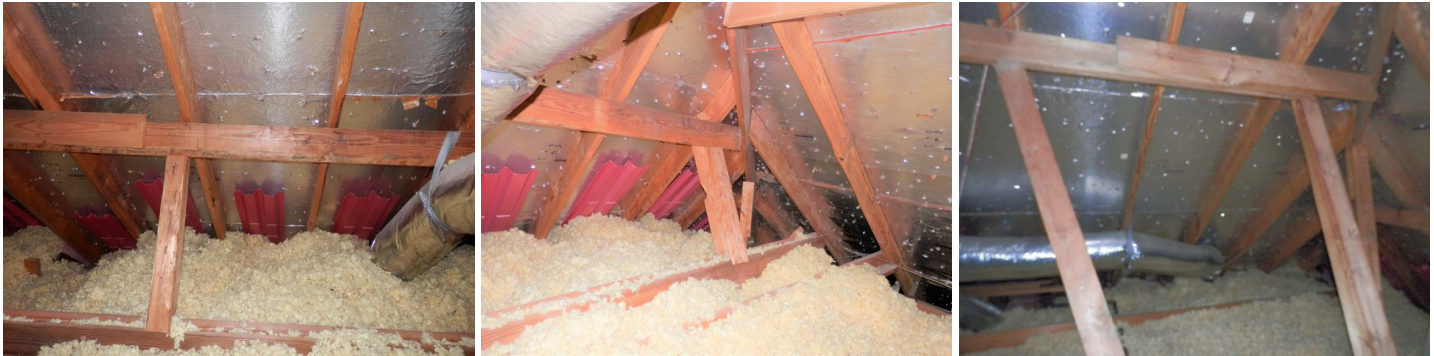
general view of the attic framing and support as seen from the limited walkway
