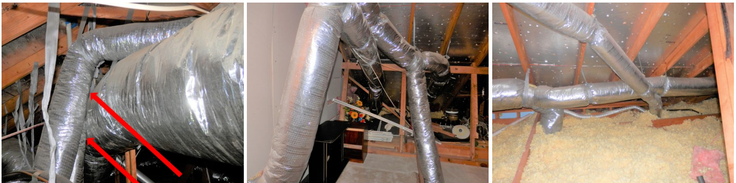
sample of ducts touching other duct lines - general view of the duct line system in the attic
