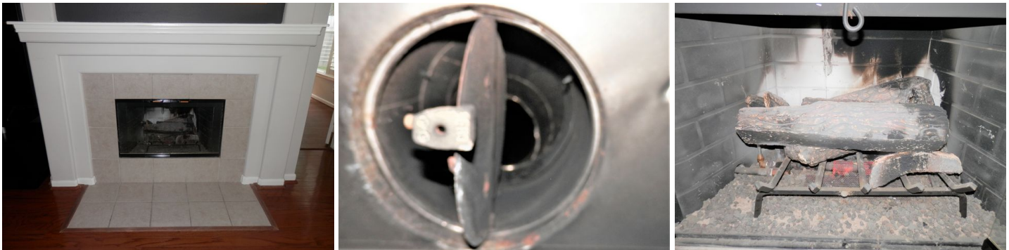
general view of the fireplace, vent / damper / flue, and the firebox
