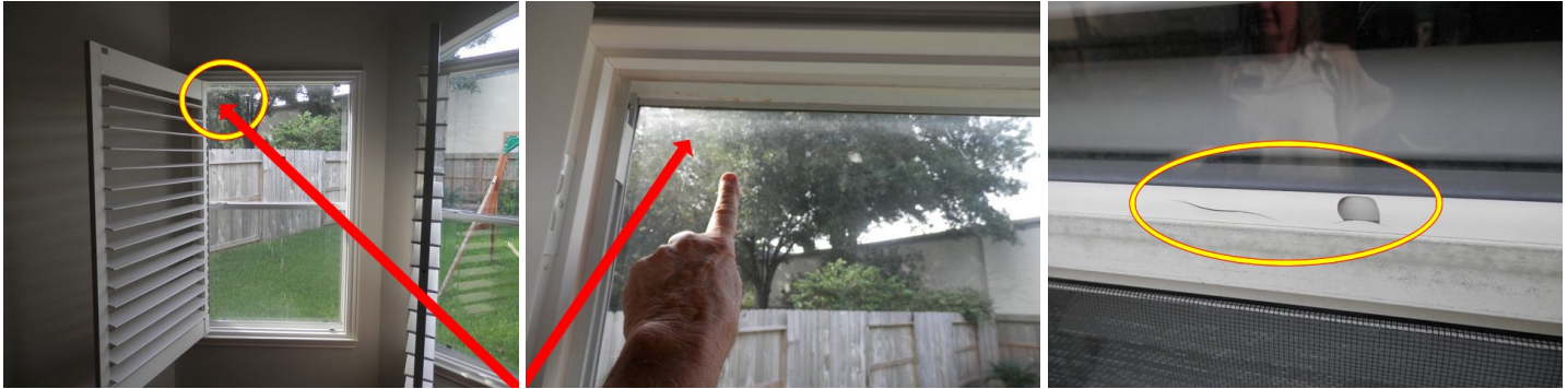
sample of broken glass at the master bedroom - sample of damaged window glaze material
