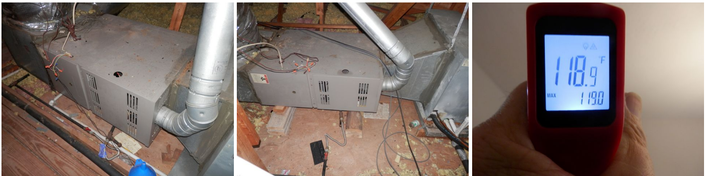
two HVAC units in the attic - checking heat output temperature in the test cycle (typical of both units)
