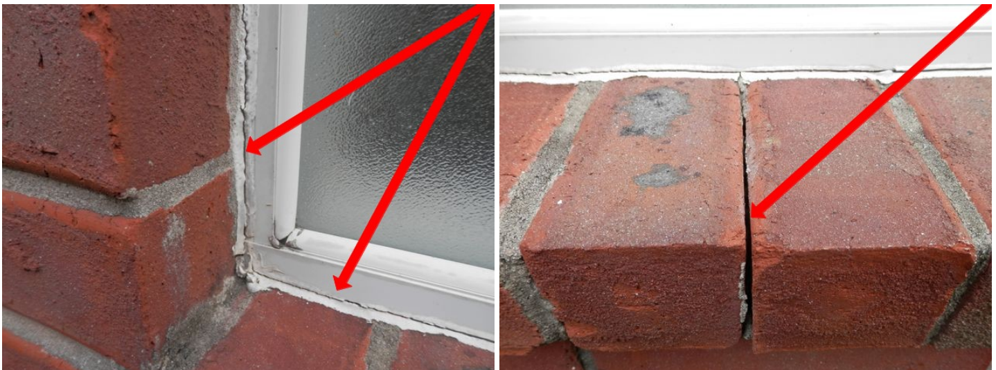
sample of caulking / sealing needed at one or more window (master bath window shown)
