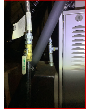
Gas shut off valve and sediment trap
