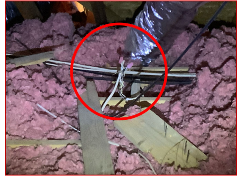
Improperly spliced and terminated wires
