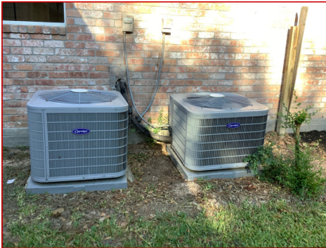
A/C condenser units
