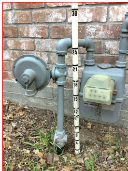
Main gas shut off valve and regulator
