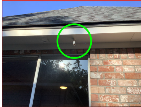
Secondary / catch pan drain termination location
