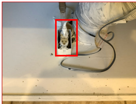
Missing cover plates
