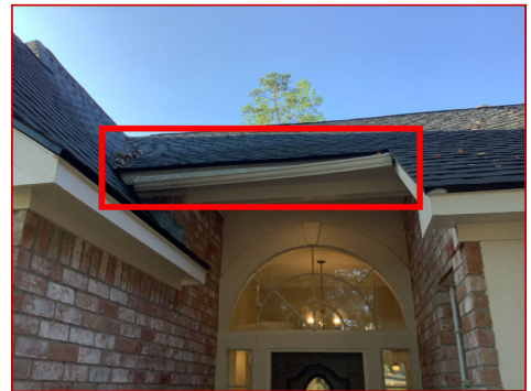
Gutter in disrepair
