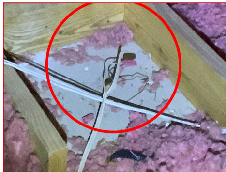
Improperly spliced and terminated wires
