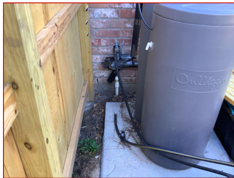
Main water shut off valve location
