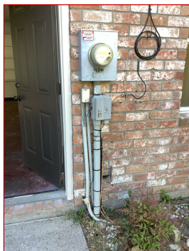
Main electrical service entrance
