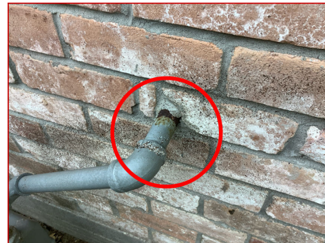
No pipe protection
