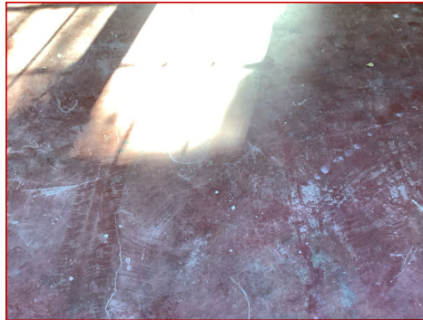
Shrinkage / random cracks
