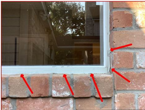
Sealant maintenance needed around windows
