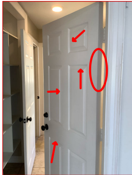
No self closing apparatus present / not a proper fire rated door
