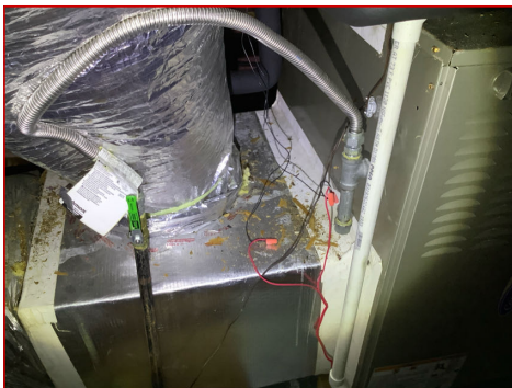
Gas shut off valve and sediment trap
