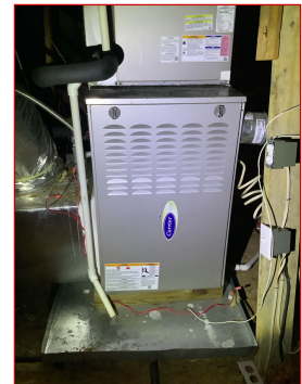
Air handler / furnace unit
