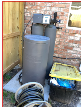
Water treatment system
