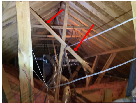
Loose collar tie
