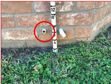
T&P relief valve and catch pan drain termination
