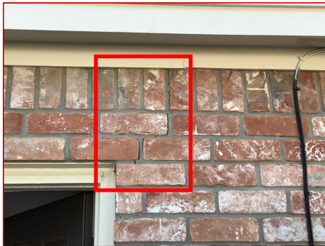
Mortar Step cracks
