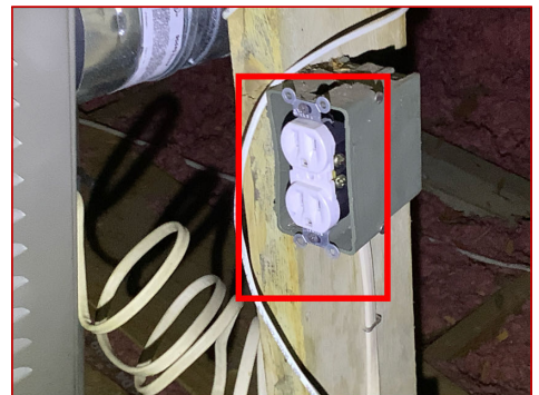
Missing cover plates
