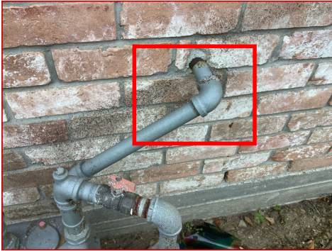
No visible bonding on gas pipe
