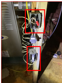
Missing cover plates
