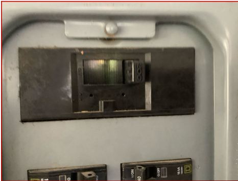
Main disconnect breaker
