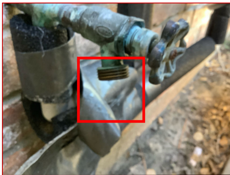
Anti siphon devices absent
