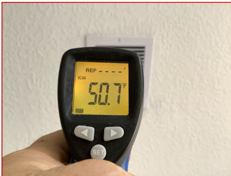
Bedroom supply temperature
