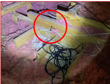
Improperly spliced and terminated wires
