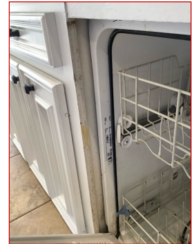
Not fastened properly
