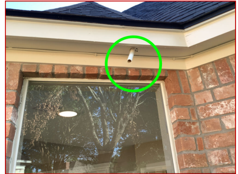
Secondary / catch pan drain termination location
