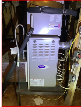
Air handler / furnace unit
