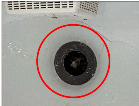
Missing drain plug
