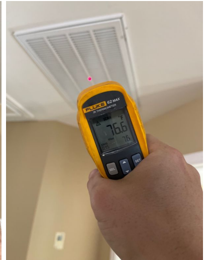
Approximately 77 degree return air upstairs.
