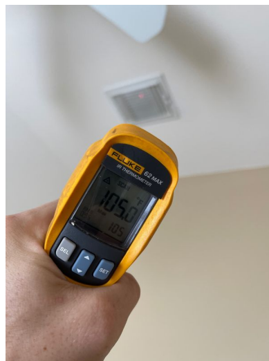
Hot supply air upstairs.
