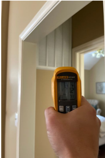
Approximately 71 degree return air downstairs.
