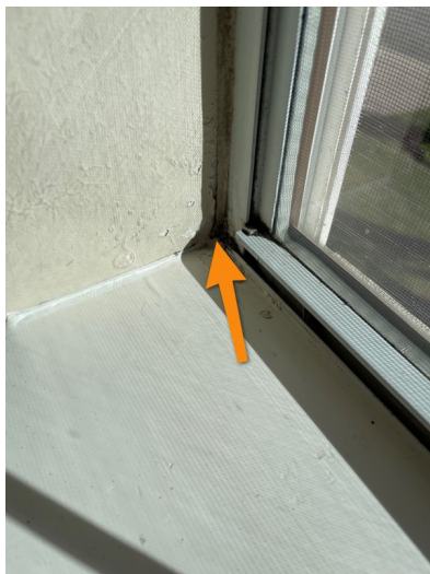
Possible slight moisture intrusion in front upstairs bedroom window corner.
