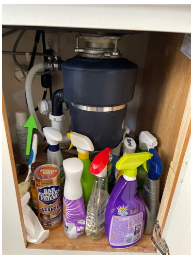
This hose should be elevated
