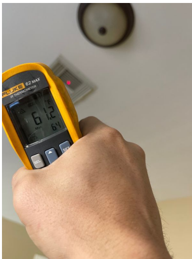
Approximately 61 degree supply air upstairs.
