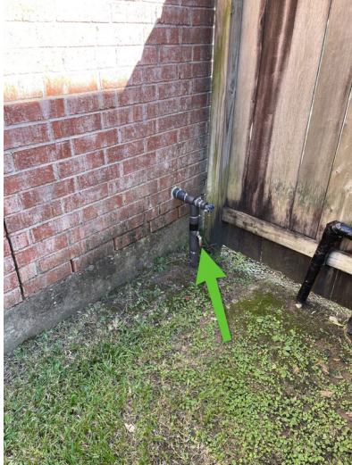
Main water shutoff valve.
