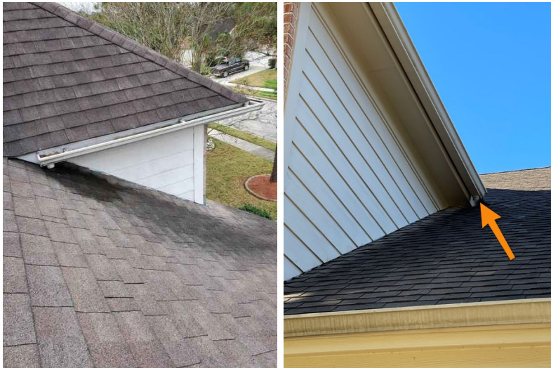
This is not your roof, but it is a good example of what you can expect to see over time.
