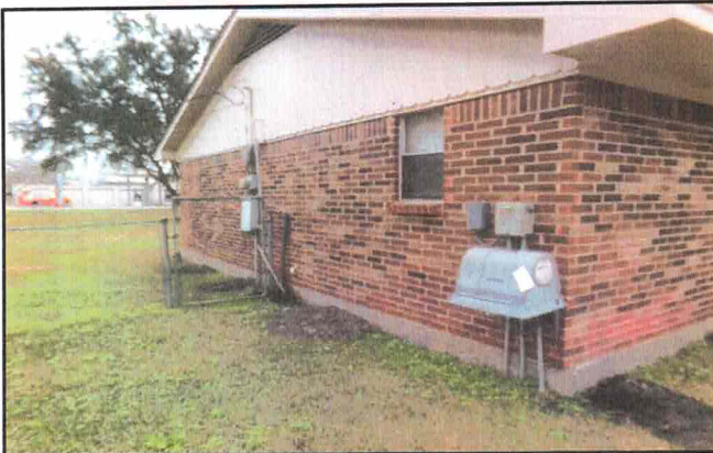
17602 Pearland Sites Rd RIGHT SIDE OF SUBJECT W/FOUNDATION REPAIR
