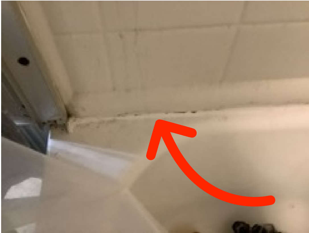
Bathroom 1 Tub/Fixture Grout is discolored/cracking
