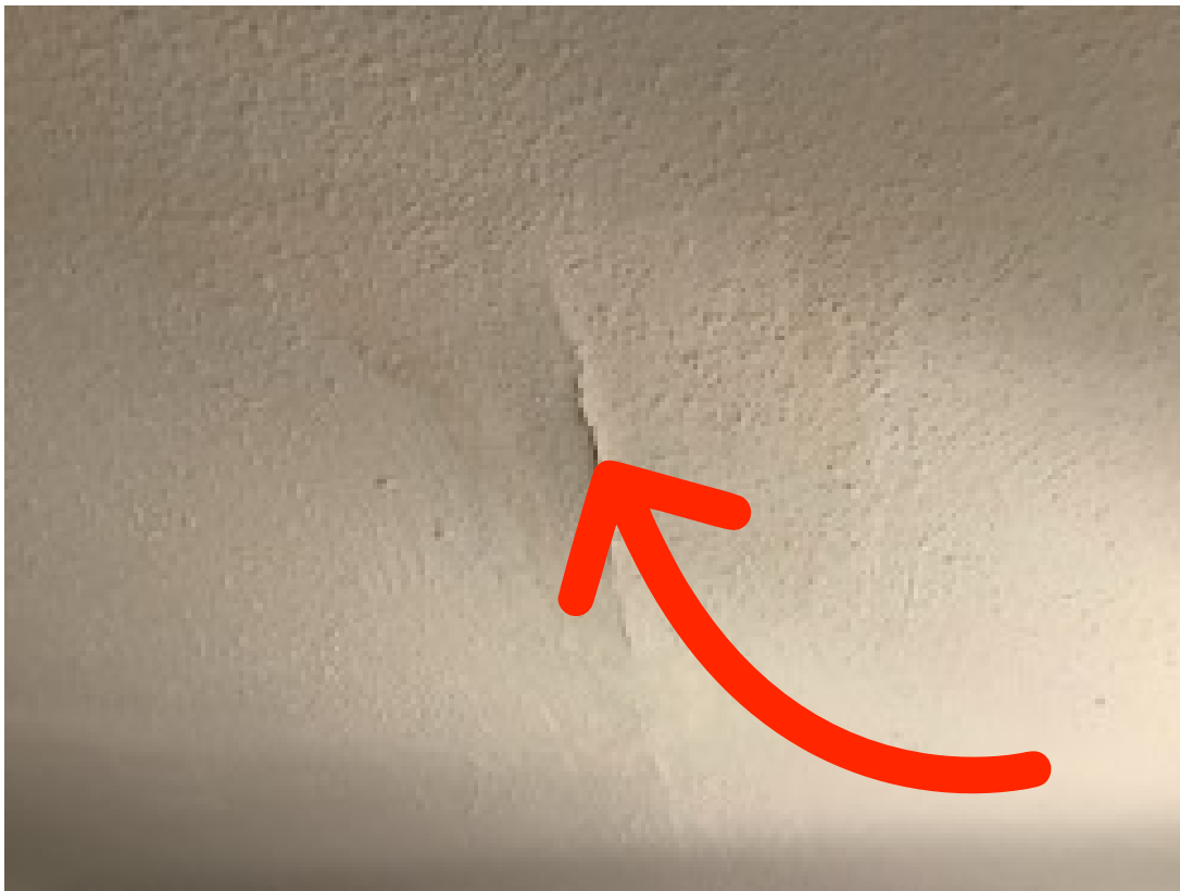
Bedroom 1 Ceiling Cracks in ceiling.
