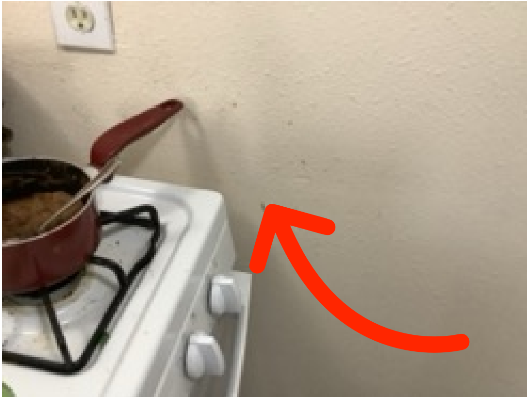
Kitchen Walls/Paint The wall is discolored
