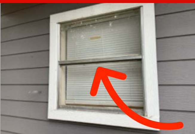
Window Screens | Screen(s) are missing
