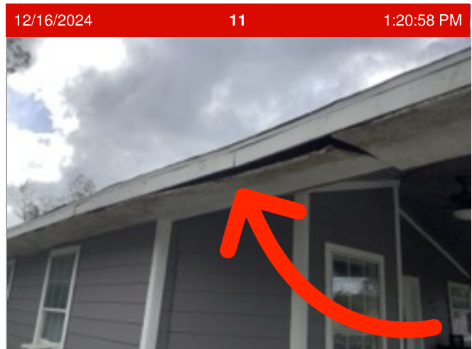
Walls/Siding/Trim | Siding warping/pulling away
