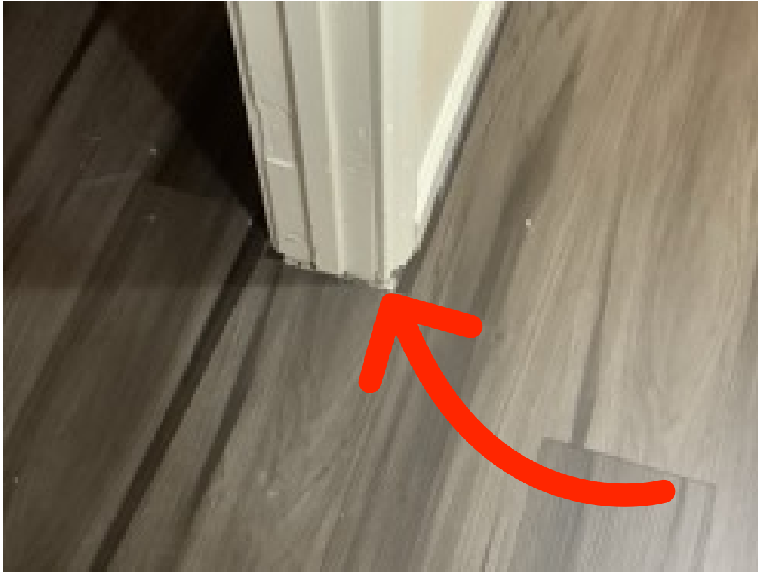
Hallway/Stairway Floors Gap in flooring.
