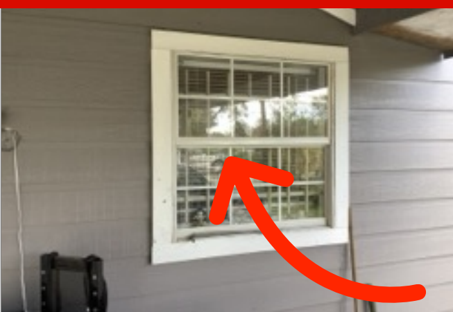
Window Screens | Screen(s) are missing
