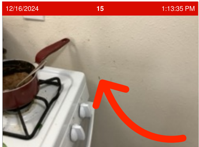
Walls/Paint | The wall is discolored
