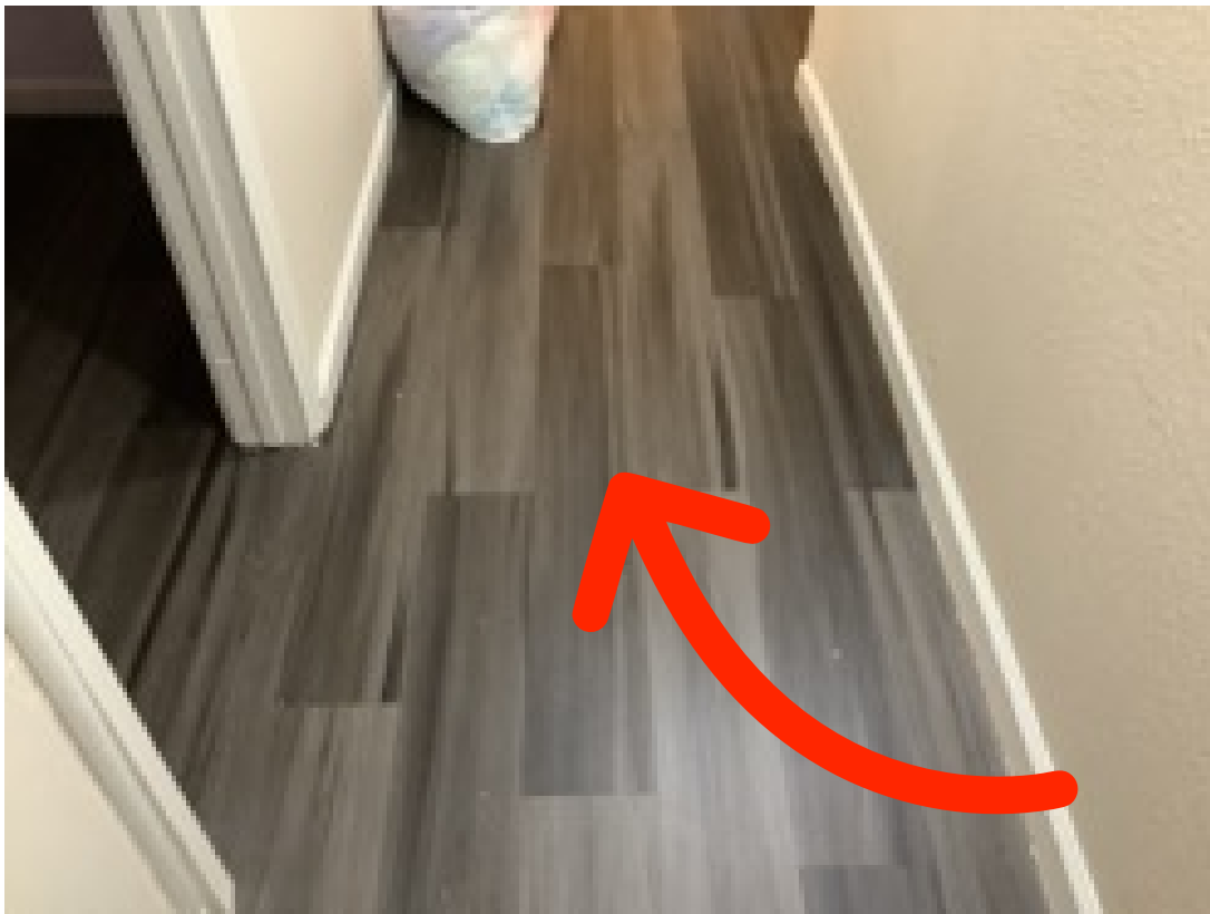
Hallway/Stairway Floors Flooring feels uneven
