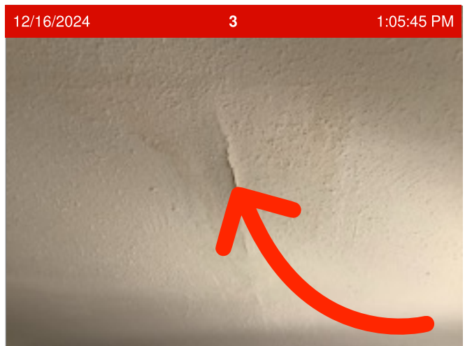
Ceiling | Cracks in ceiling.
