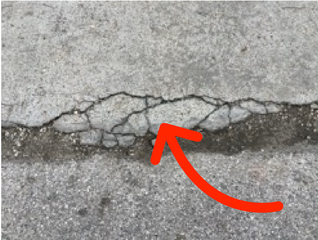
Front Exterior Driveway Spider cracks in driveway.
