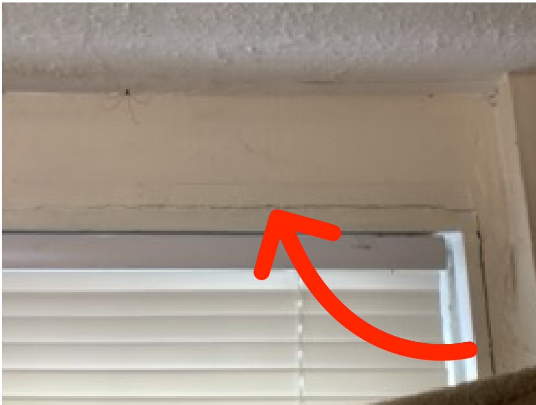
Bathroom 1 Walls/Paint Cracks in texture
