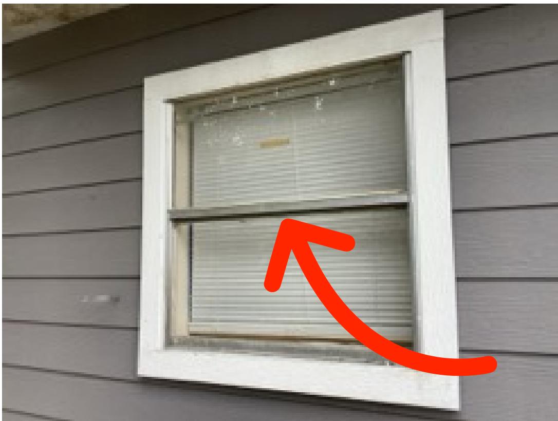
Front Exterior Window Screens Screen(s) are missing
