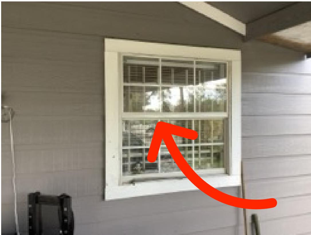
Front Exterior Window Screens Screen(s) are missing
