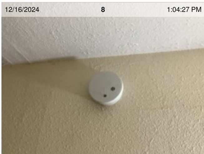
Wireless Smoke Alarm (mfd 4/2023) | Smoke test: Passed | Alarm in place
