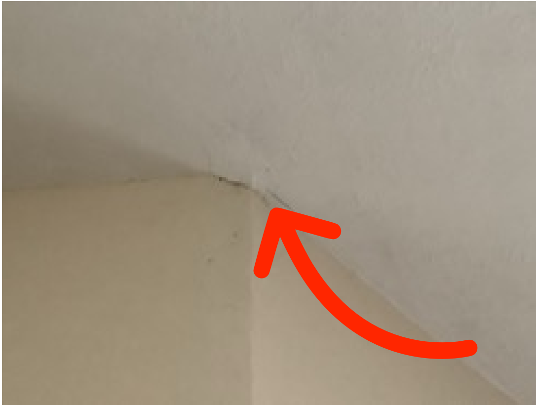
Entry Ceiling Cracks in ceiling.
