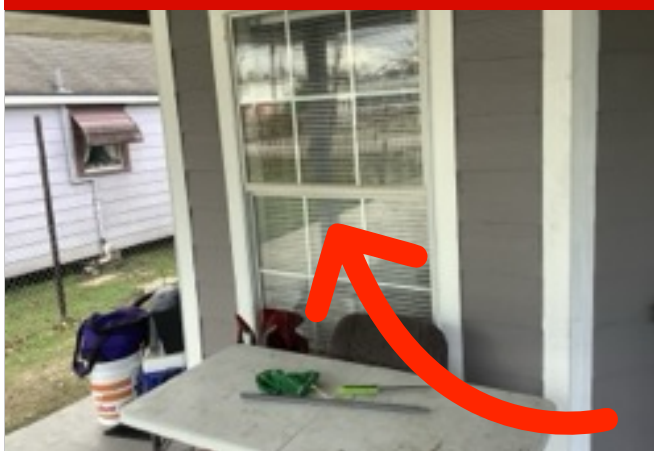
Window Screens | Screen(s) are missing
