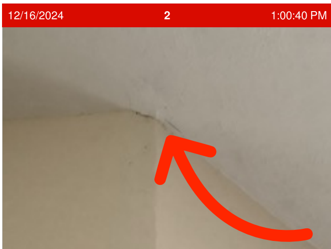
Ceiling | Cracks in ceiling.
