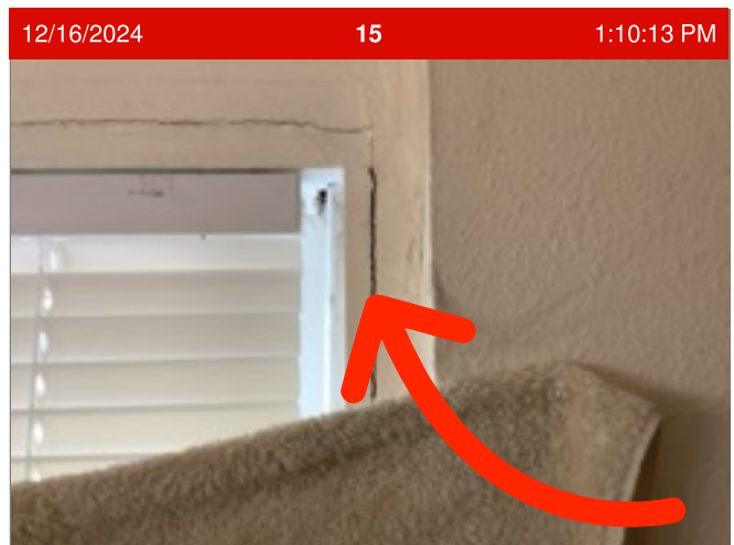
Walls/Paint | Cracks in texture
