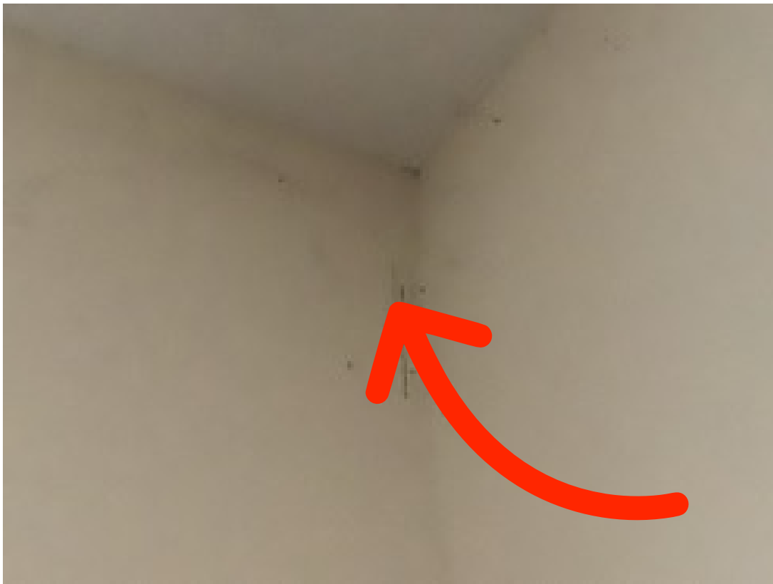
Entry Walls/Paint The wall is discolored
