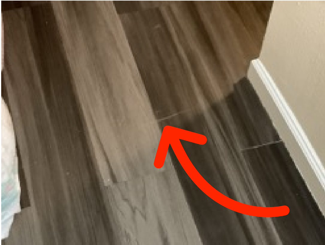
Hallway/Stairway Floors Crack in flooring.
