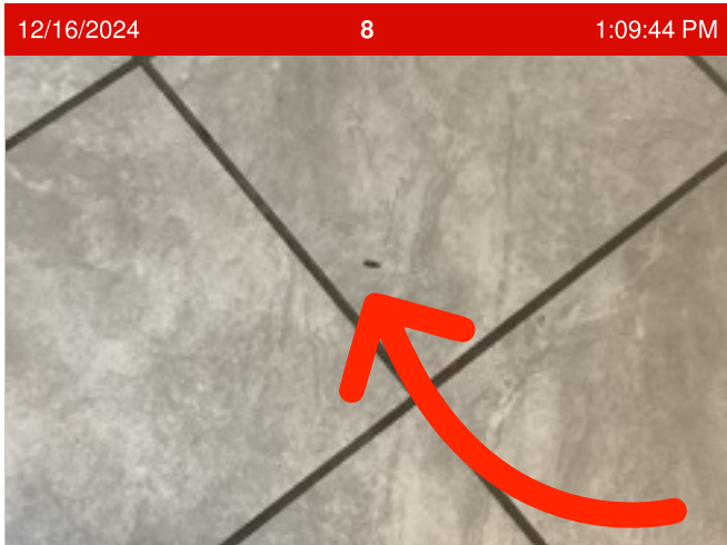
Floors | Gap in flooring.
