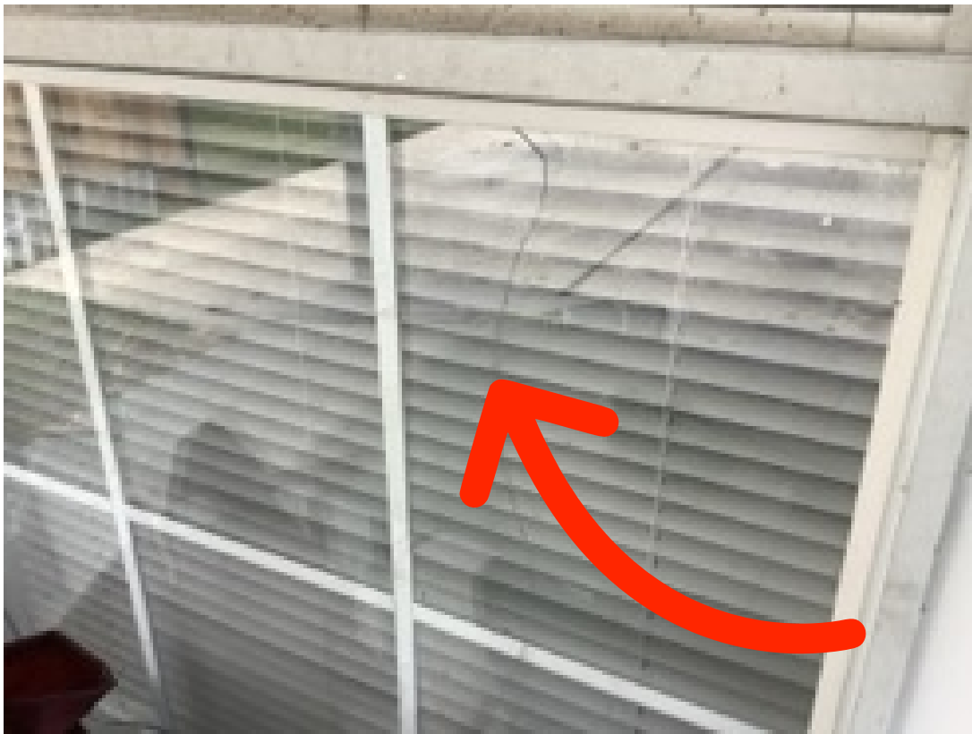
Living Room Windows Broken/cracked/damage missing/damaged locking hardware; evidence of moisture
