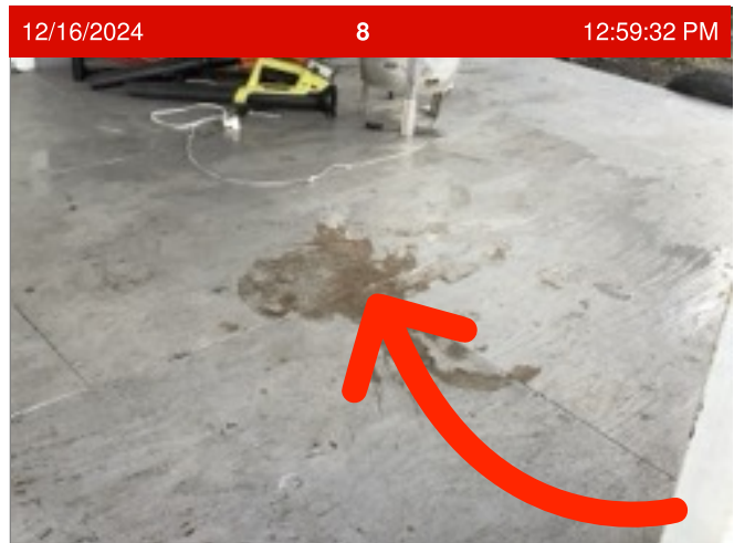
Patio/Porch | Cracks in concrete; damage ; discoloration
