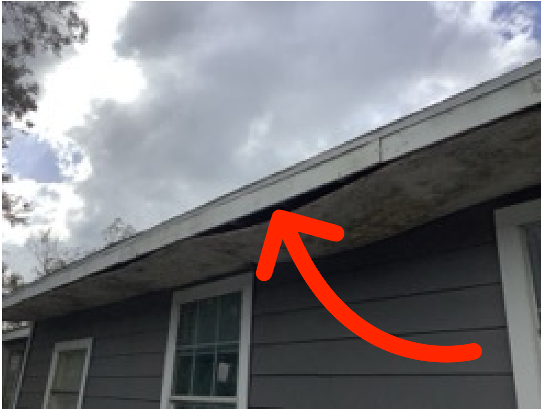
Front Exterior Walls/Siding/Trim Siding warping/pulling away
