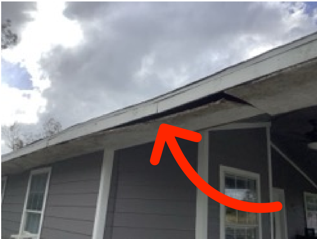
Front Exterior Walls/Siding/Trim Siding warping/pulling away
