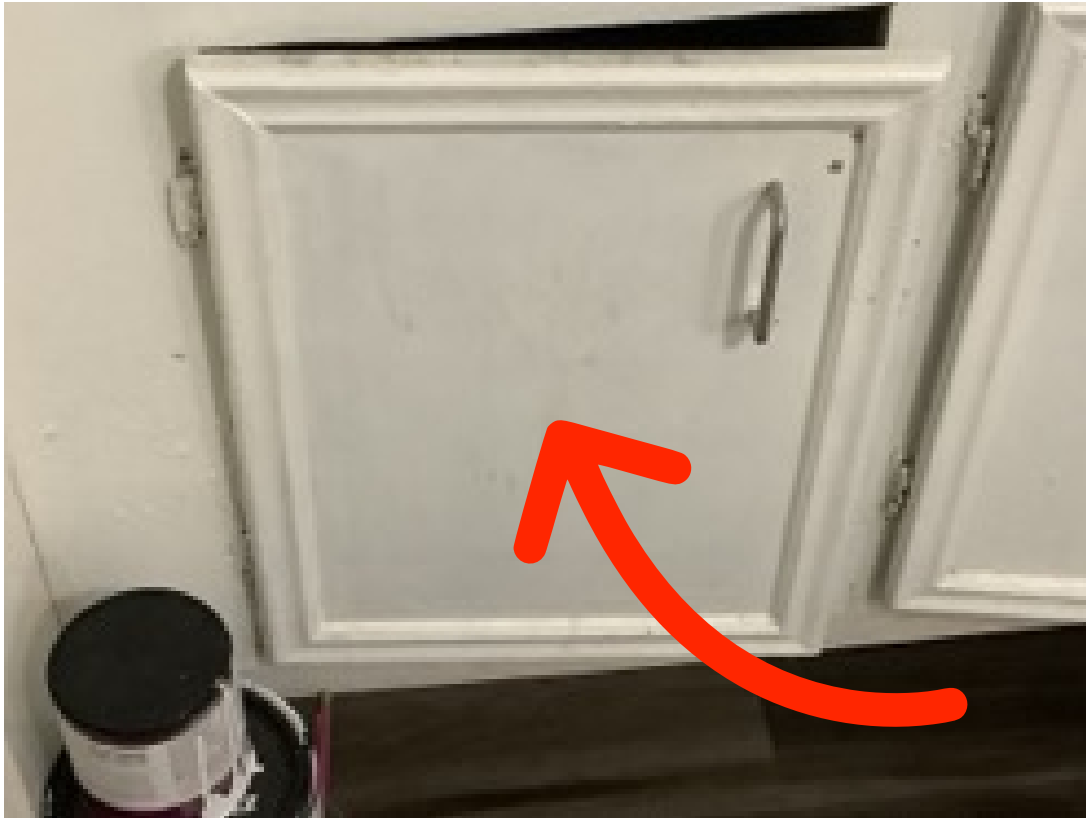
Kitchen Lower Cabinets - Exterior The cabinet doors are discolored.
