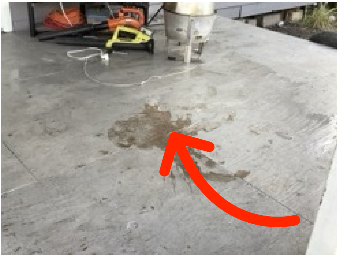
Entry Patio/Porch Cracks in concrete; damage ; discoloration
