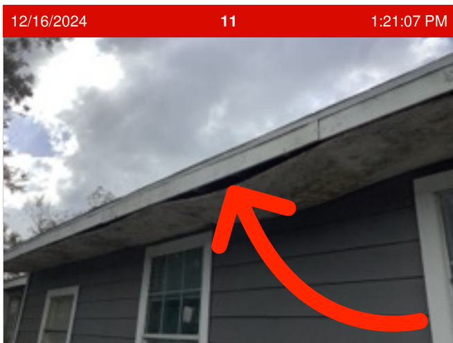
Walls/Siding/Trim | Siding warping/pulling away
