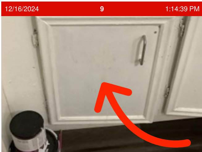
Lower Cabinets - Exterior | The cabinet doors are discolored.
