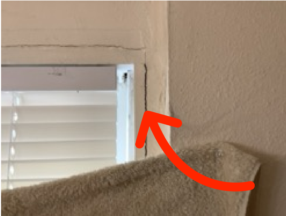
Bathroom 1 Walls/Paint Cracks in texture
