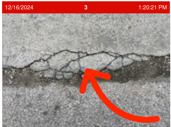
Driveway | Spider cracks in driveway.
