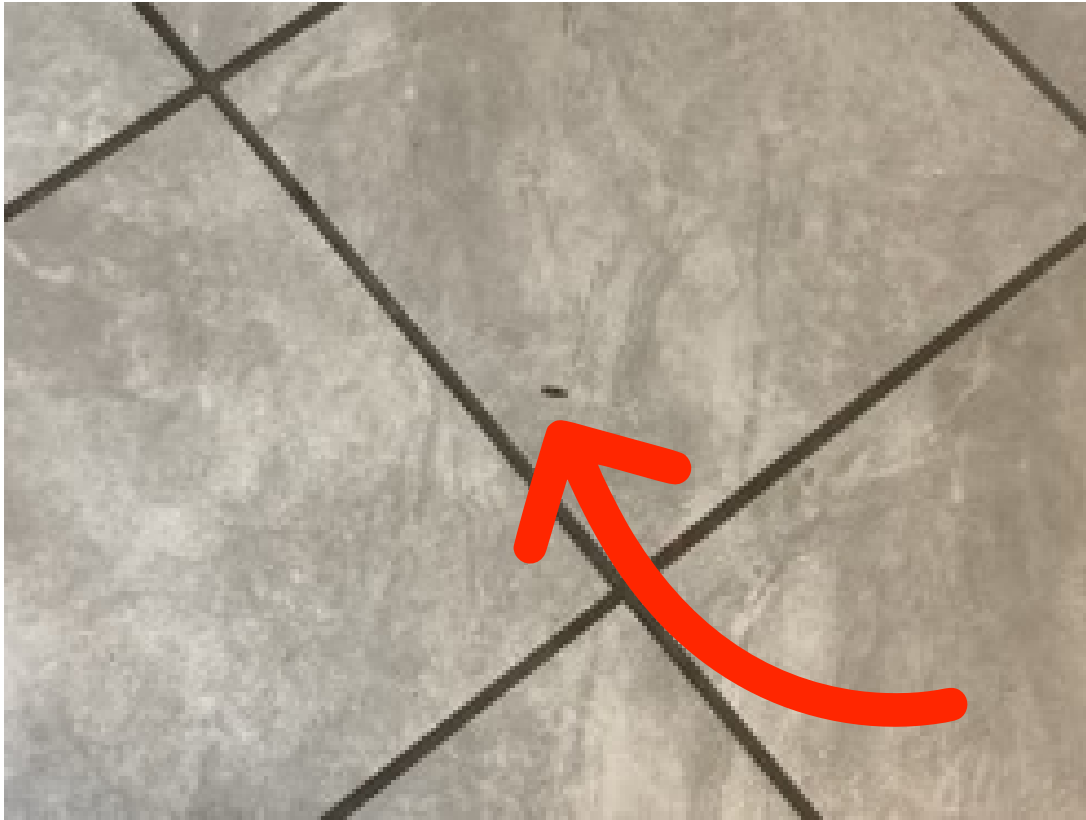
Bathroom 1 Floors Gap in flooring.
