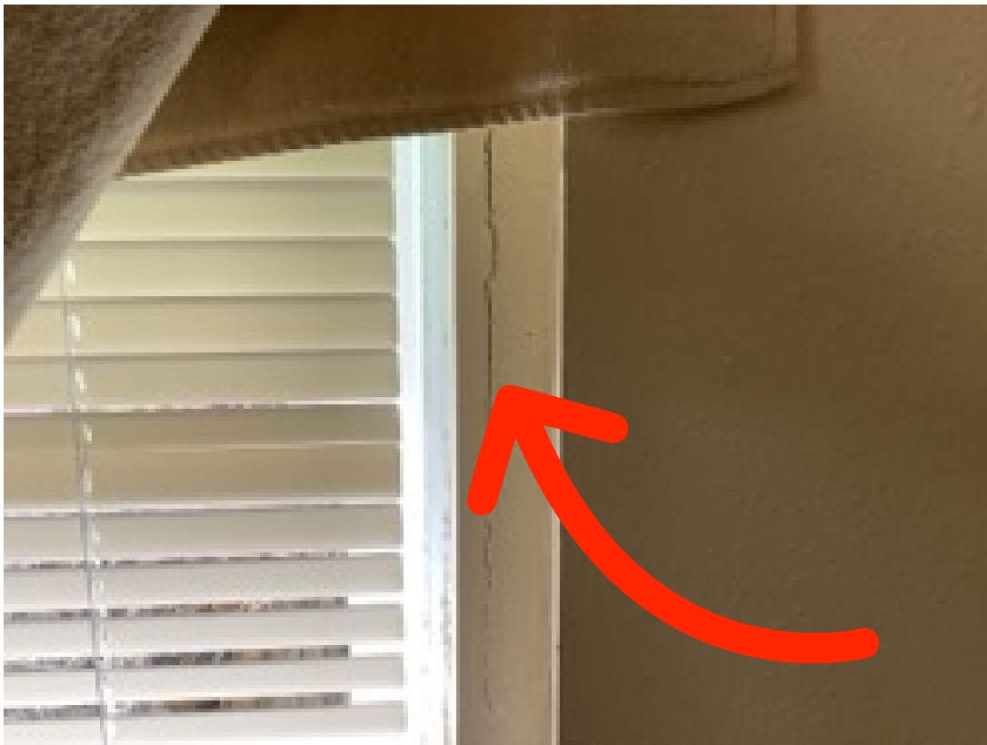
Bathroom 1 Walls/Paint Cracks in texture
