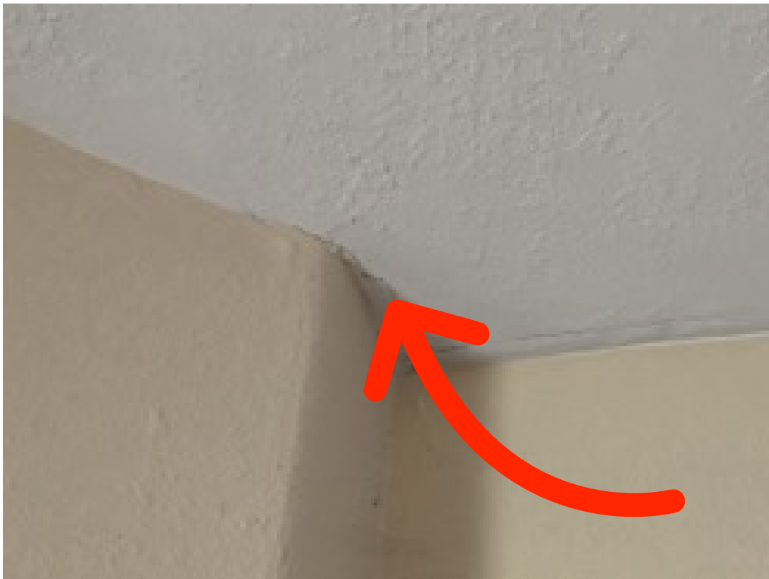
Living Room Ceiling Cracks in ceiling.
