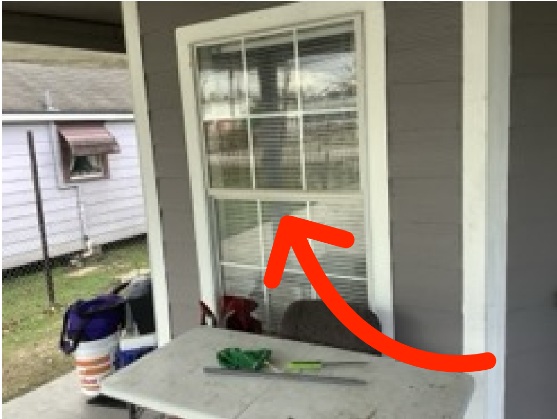
Front Exterior Window Screens Screen(s) are missing
