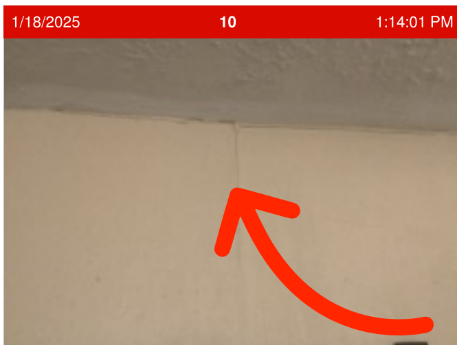
Walls/Paint | Cracks in texture
