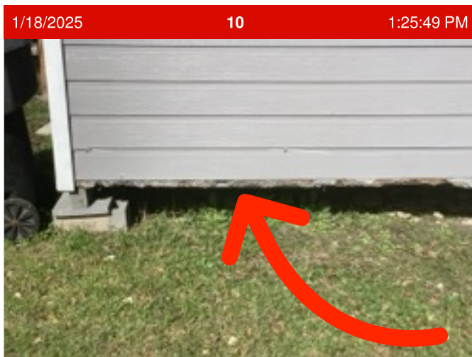
Walls/Siding/Trim | Siding is deteriorating
