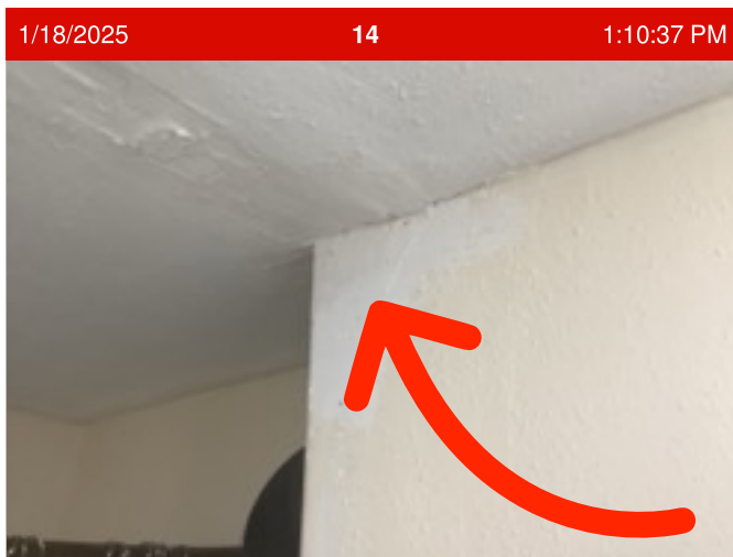
Walls/Paint | The wall is discolored
