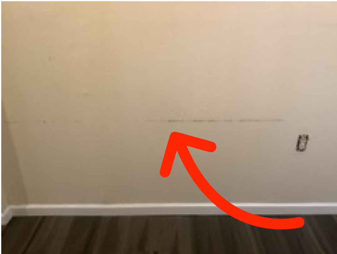
Kitchen Walls/Paint Scratches on the wall
