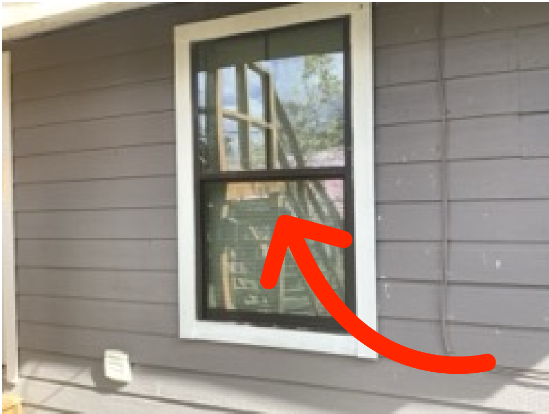
Front Exterior Window Screens Screen(s) are missing
