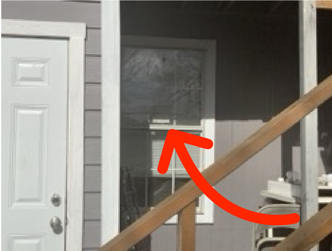
Front Exterior Window Screens Screen(s) are missing
