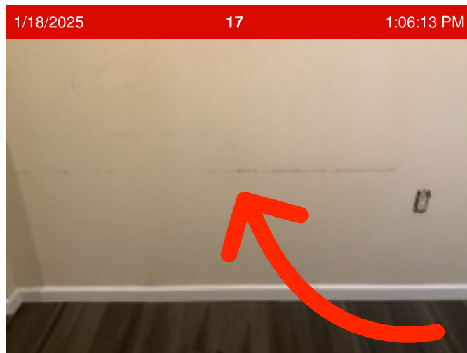
Walls/Paint | Scratches on the wall
