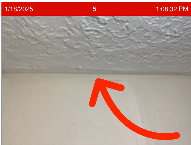
Walls/Paint | Cracks in texture
