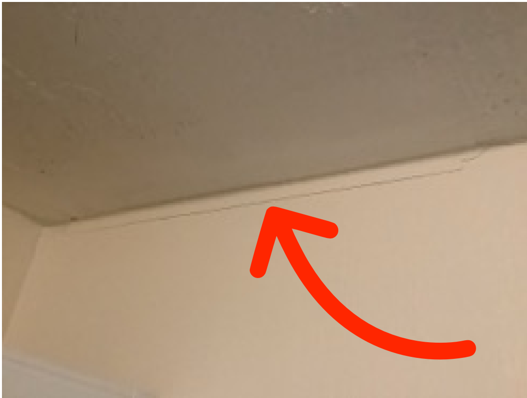
Kitchen Walls/Paint Cracks in texture
