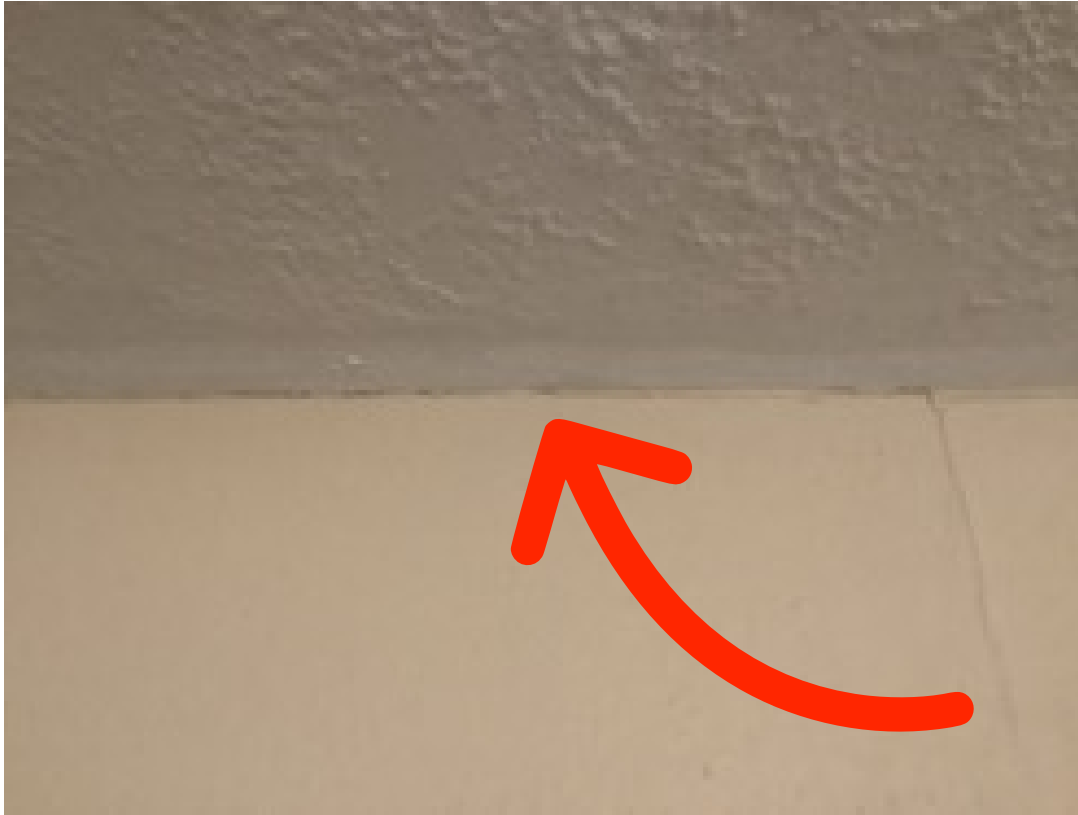
Bedroom 2 Walls/Paint Cracks in texture
