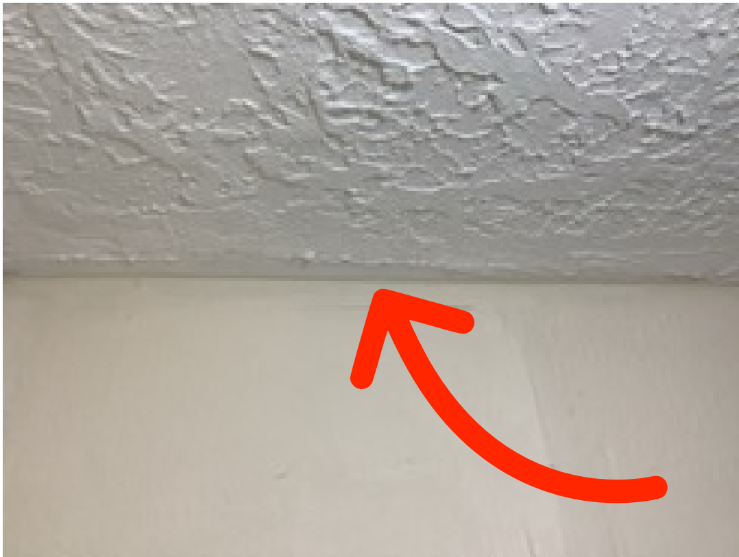
Hallway/Stairway Walls/Paint Cracks in texture
