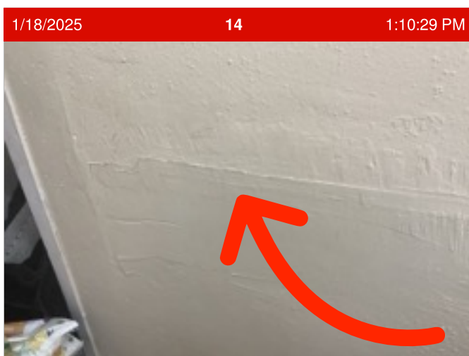
Walls/Paint | Cracks in texture
