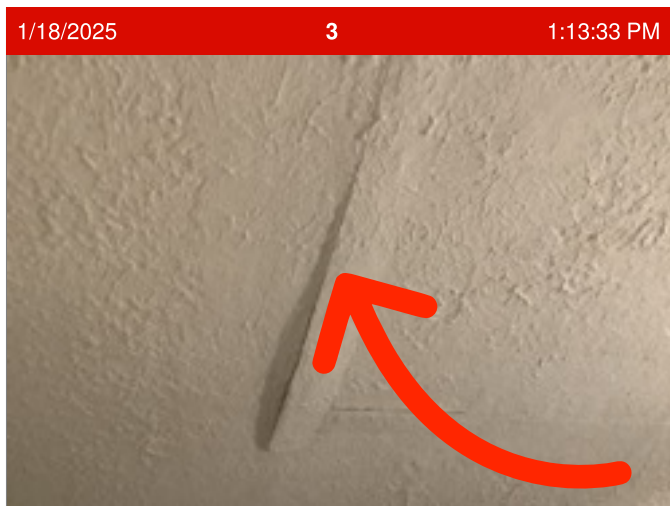
Ceiling | Cracks in ceiling.
