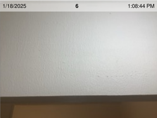
Tamper-Proof Smoke Alarm (mfd 4/2024) | Smoke test: Passed | Alarm in place
