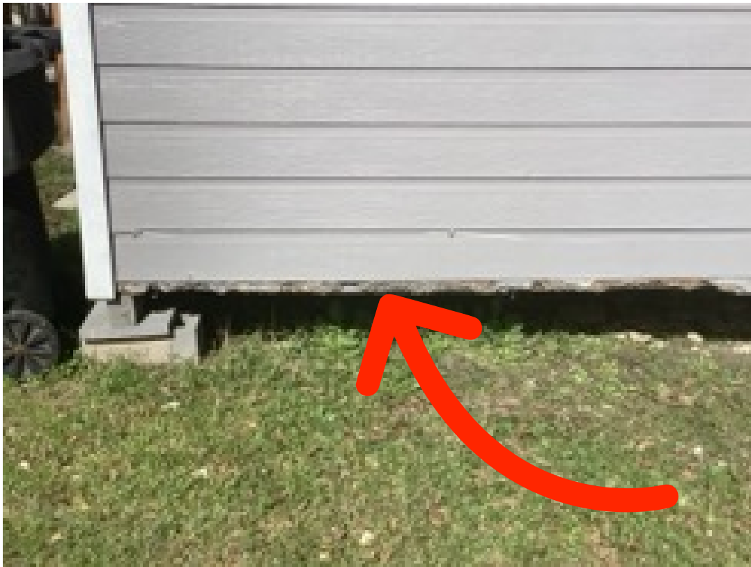
Front Exterior Walls/Siding/Trim Siding is deteriorating
