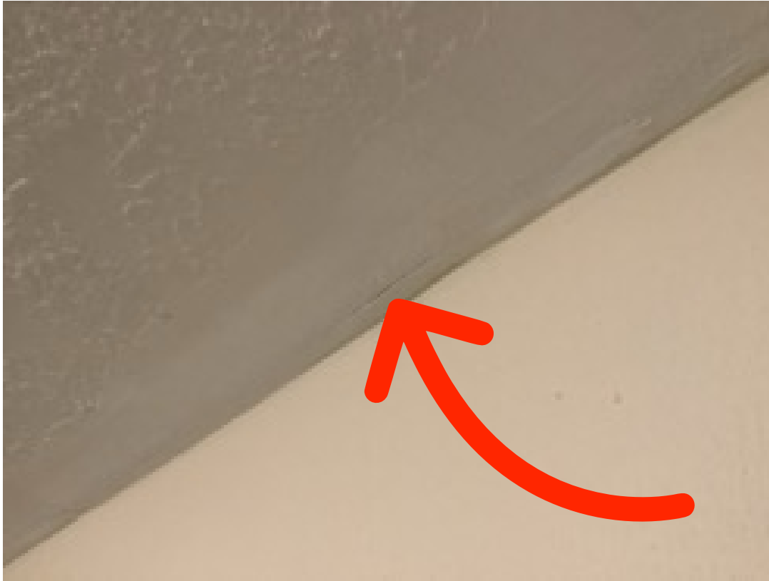
Kitchen Ceiling Cracks in ceiling.
