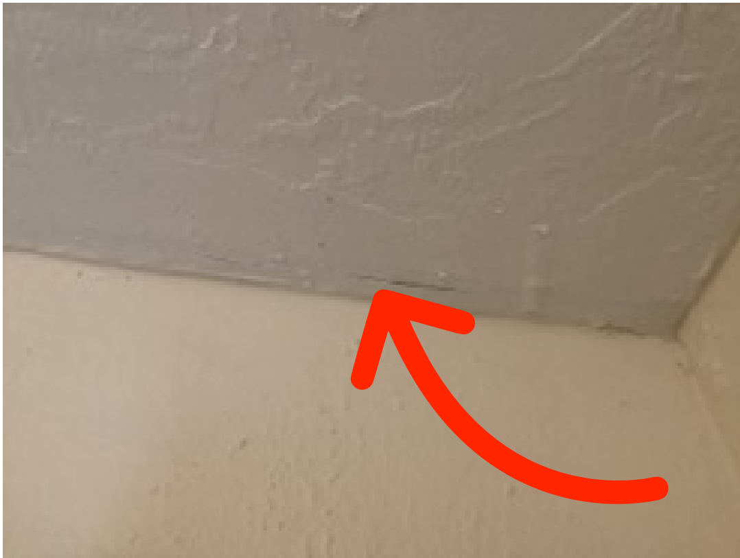
Entry Ceiling Cracks in ceiling.
