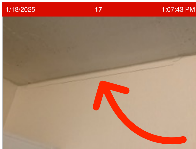
Walls/Paint | Cracks in texture
