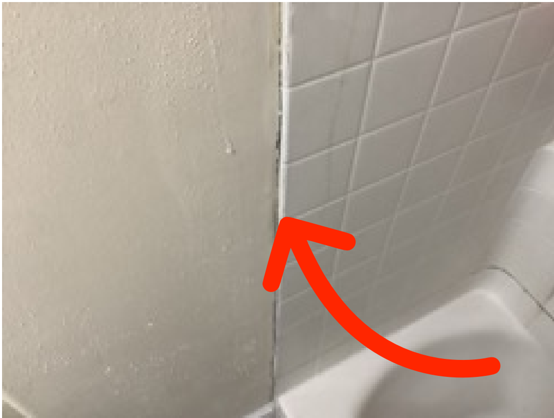
Bathroom 1 Walls/Paint Cracks in texture
