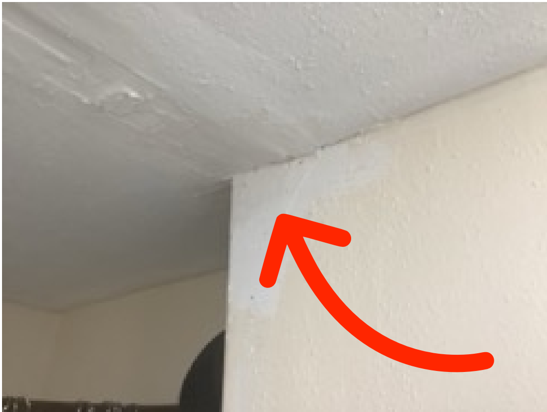
Bathroom 1 Walls/Paint The wall is discolored
