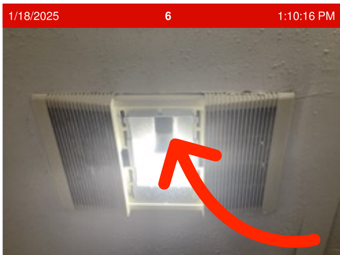
Exhaust Fan | Exhaust fan does not turn on.
