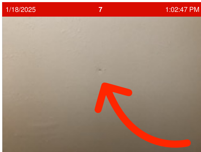
Door Stop | Broken- wall damage noted.
