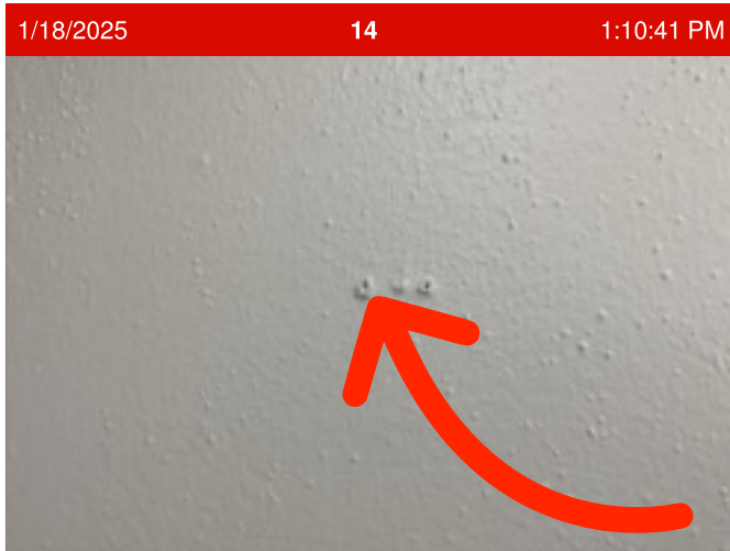
Walls/Paint | Holes in wall.
