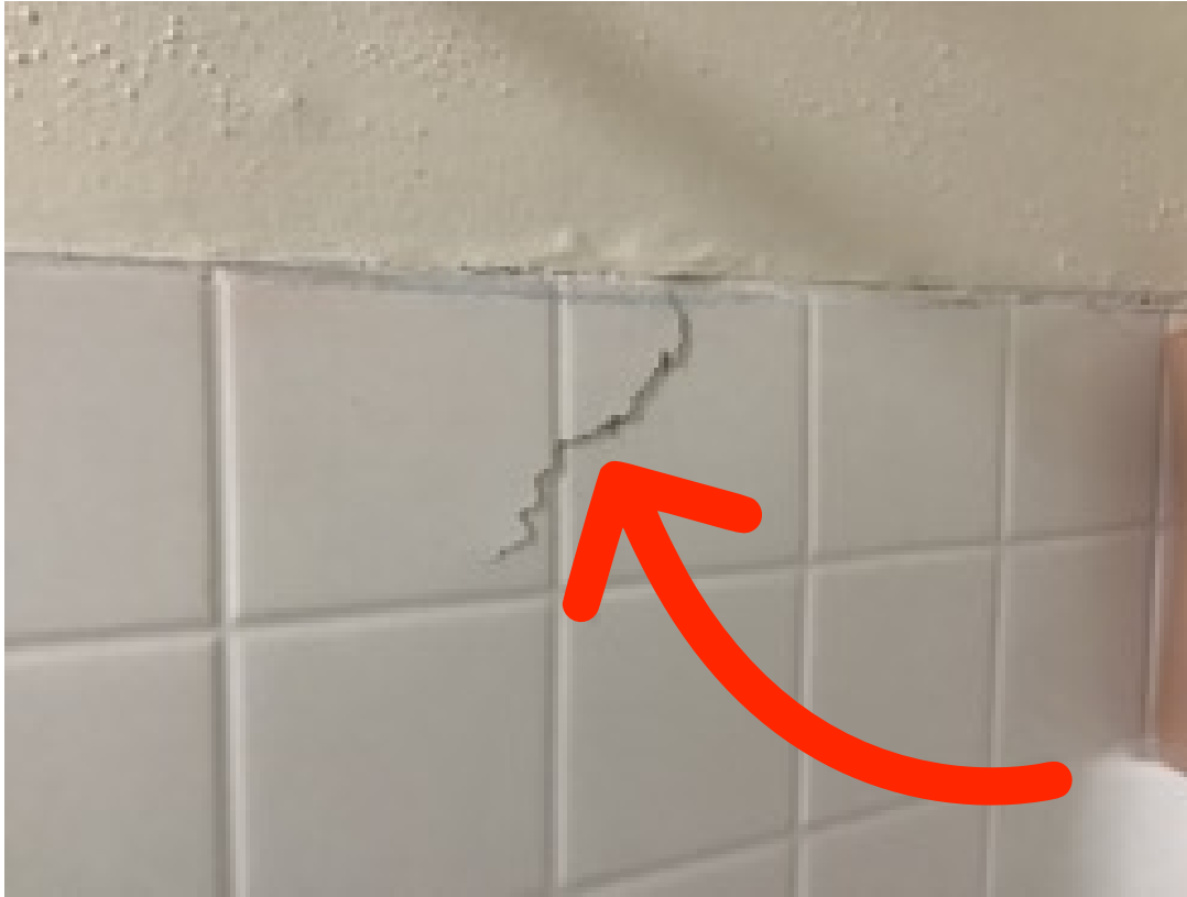
Bathroom 1 Tub/Fixture Cracked tile
