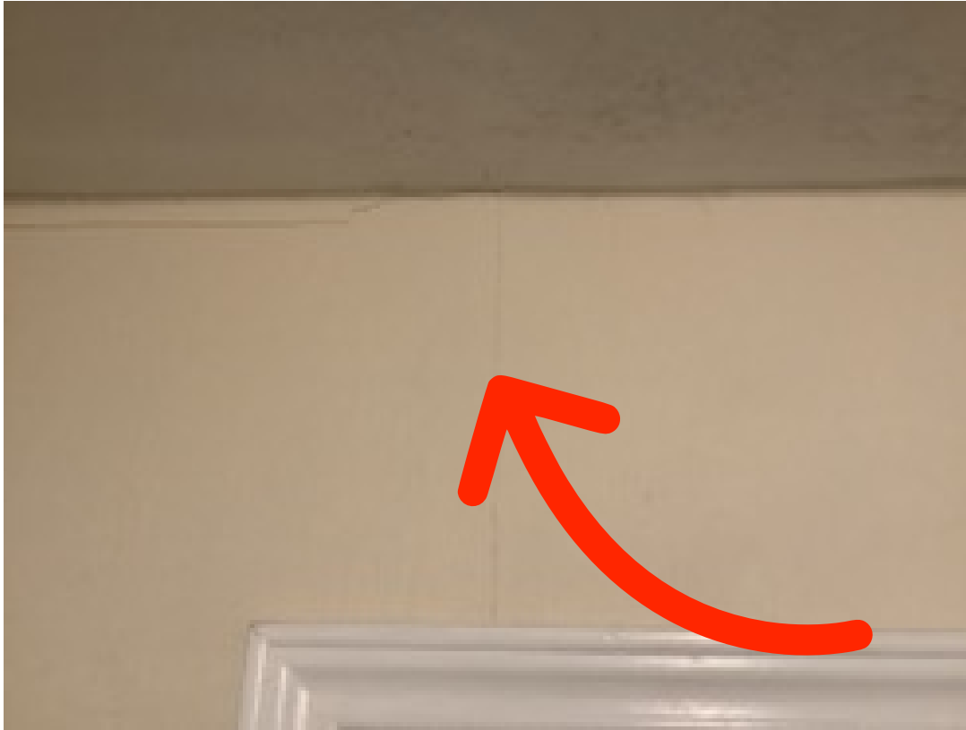
Kitchen Walls/Paint Cracks in texture
