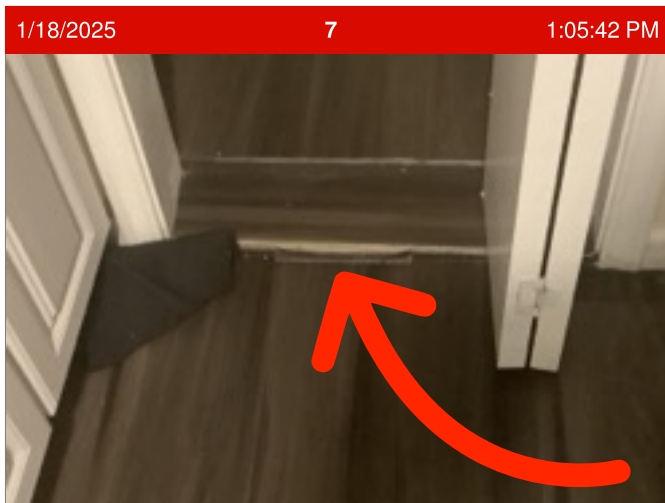
Floors | Gap in flooring.
