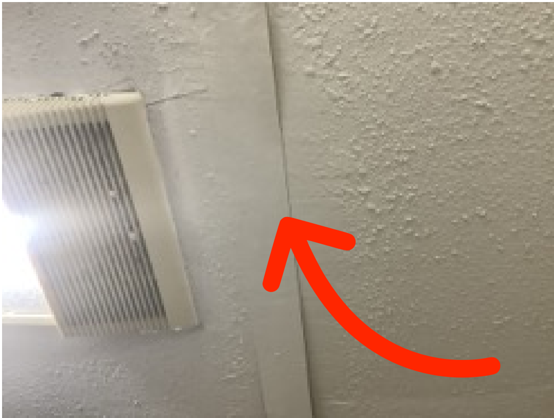
Bathroom 1 Ceiling Cracks in ceiling.
