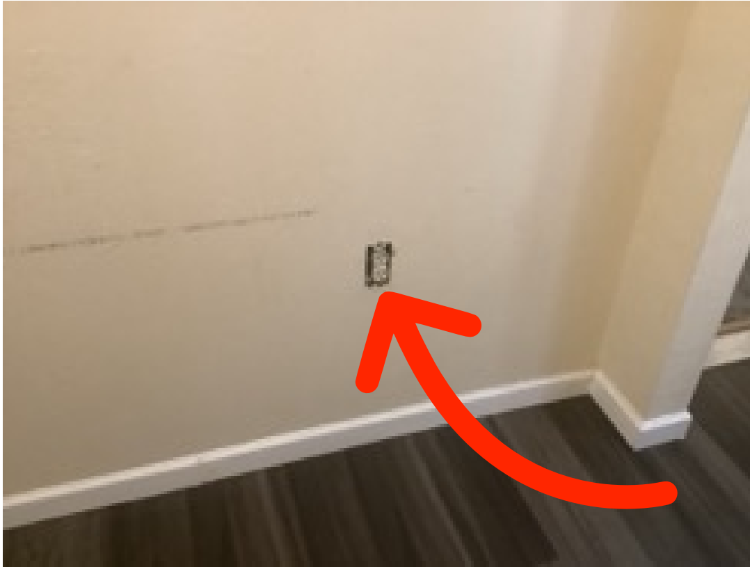
Kitchen Outlet/Switch Covers Cover is missing.
