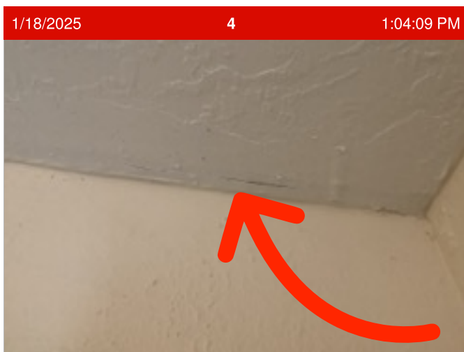
Ceiling | Cracks in ceiling.
