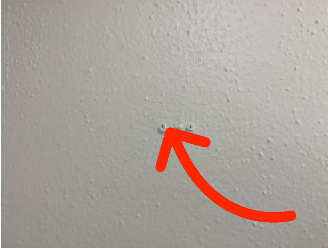
Bathroom 1 Walls/Paint Holes in wall.
