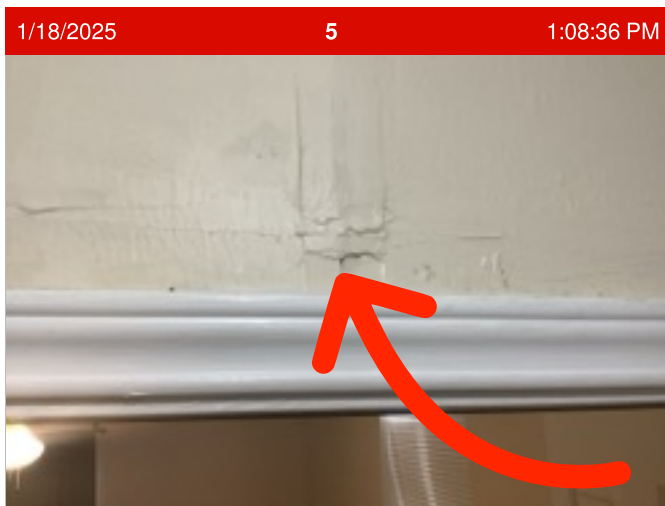
Walls/Paint | Cracks in texture
