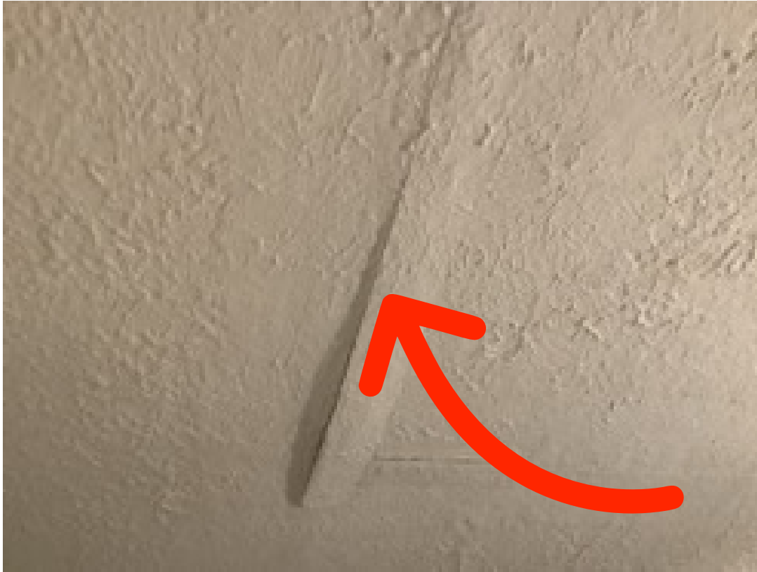
Bedroom 2 Ceiling Cracks in ceiling.
