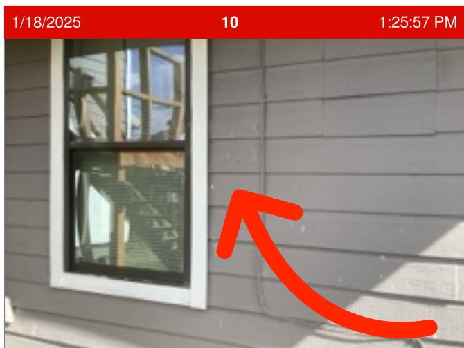
Walls/Siding/Trim | Siding is discolored
