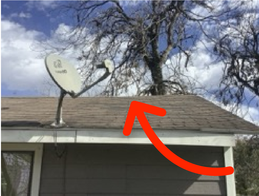
Front Exterior Roof/Trim/Gutter Missing shingles.
