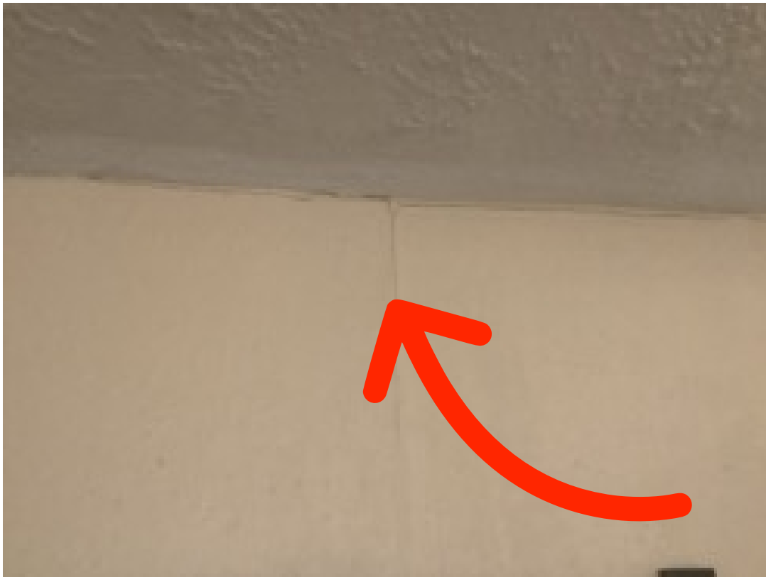
Bedroom 2 Walls/Paint Cracks in texture
