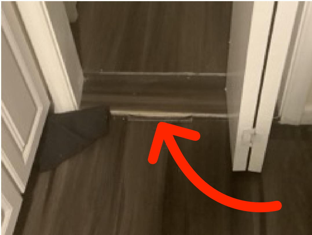
Kitchen Floors Gap in flooring.
