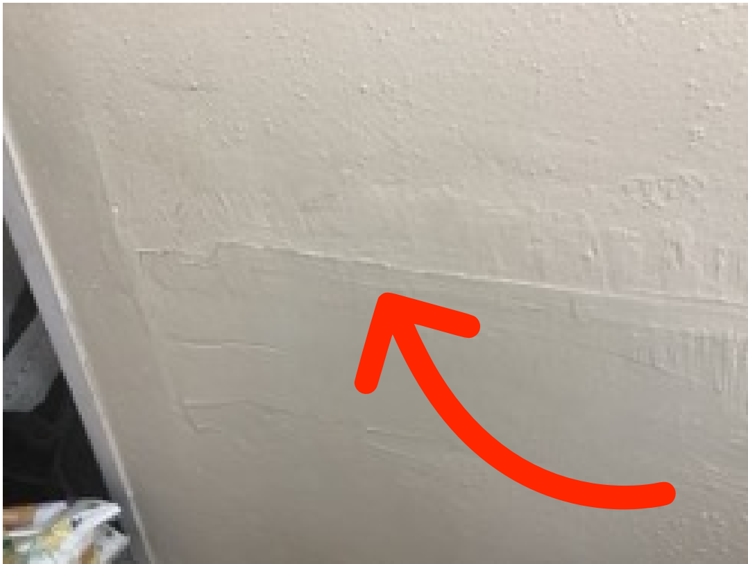
Bathroom 1 Walls/Paint Cracks in texture
