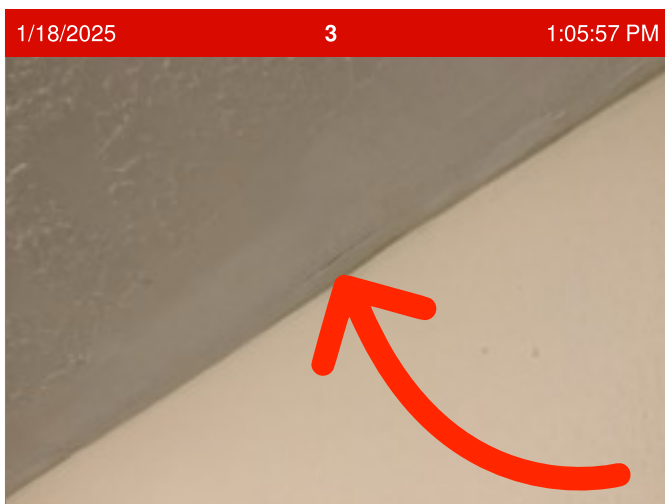
Ceiling | Cracks in ceiling.
