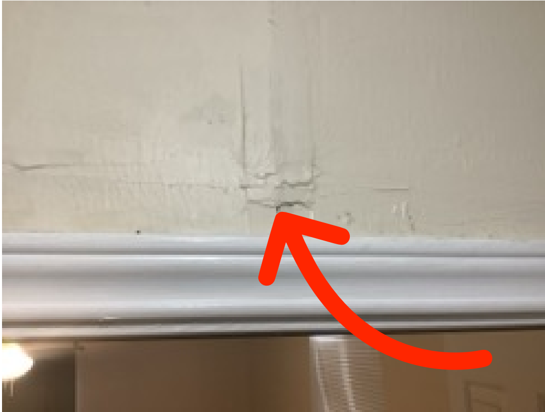
Hallway/Stairway Walls/Paint Cracks in texture
