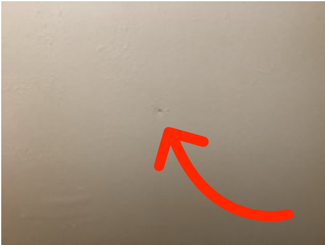
Entry Door Stop Broken- wall damage noted.
