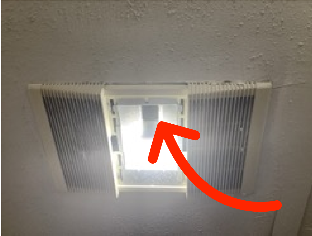
Bathroom 1 Exhaust Fan Exhaust fan does not turn on.
