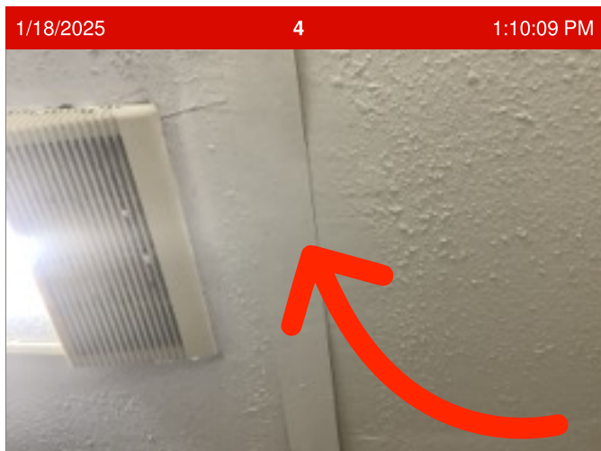
Ceiling | Cracks in ceiling.
