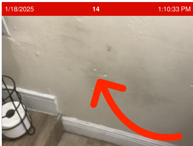
Walls/Paint | The wall is discolored
