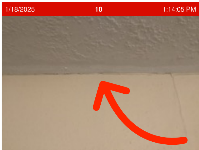
Walls/Paint | Cracks in texture
