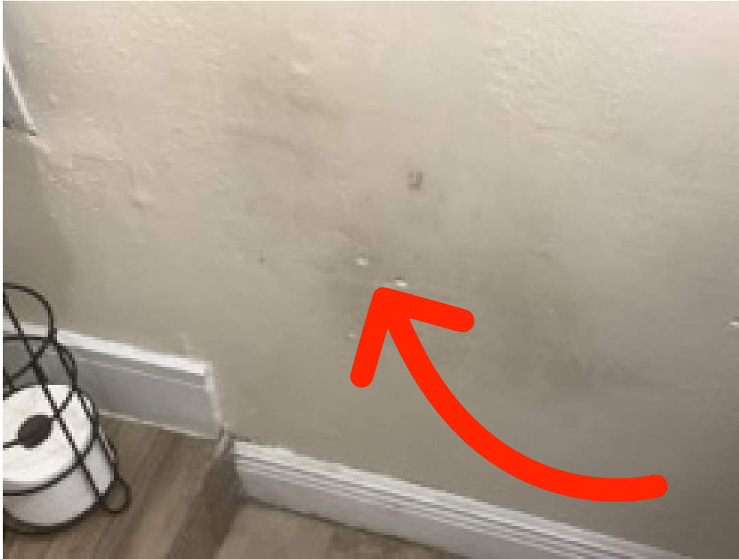
Bathroom 1 Walls/Paint The wall is discolored
