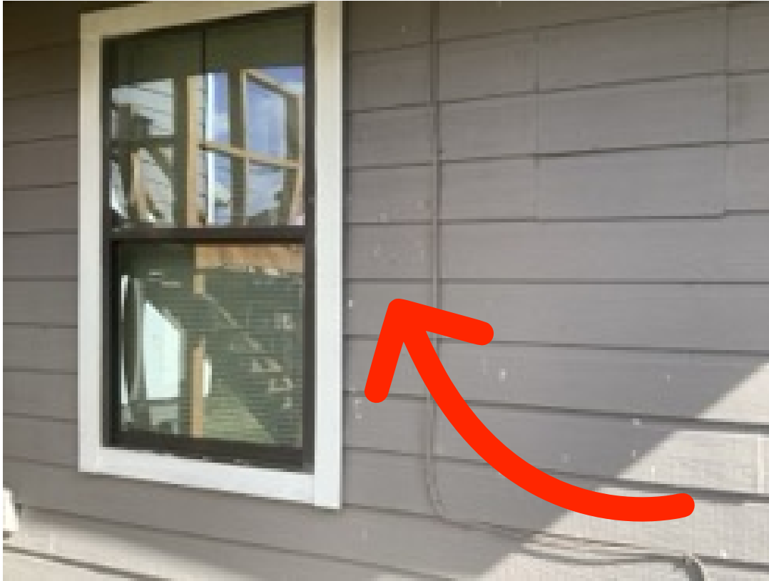
Front Exterior Walls/Siding/Trim Siding is discolored
