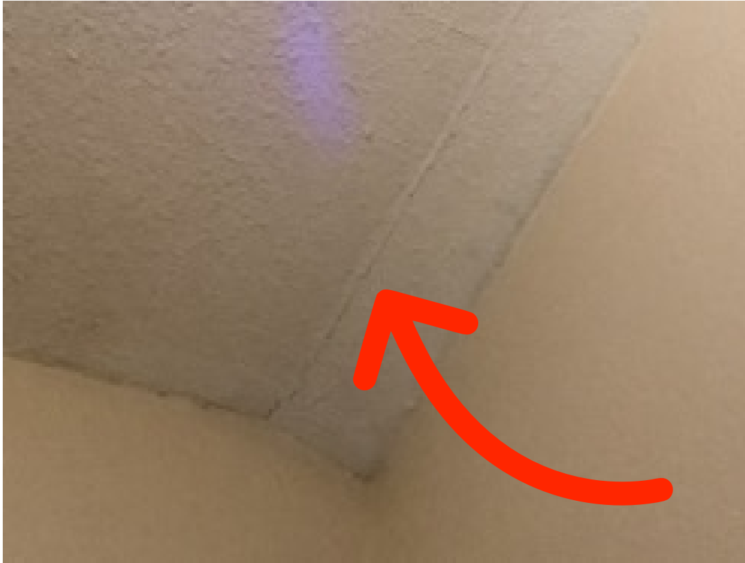
Bedroom 1 Ceiling Cracks in ceiling.
