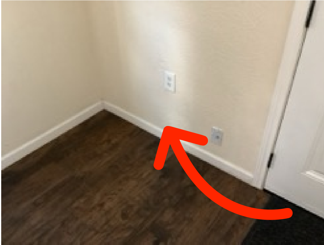
Entry Door Stop Missing- no wall damage noted.
