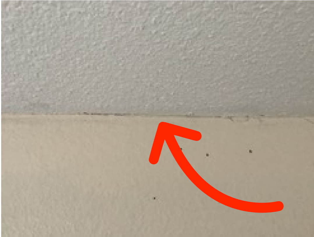
Entry Ceiling Slight separation of wall and ceiling (see closeup).
