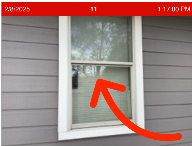
Window Screens | Screen(s) are missing
