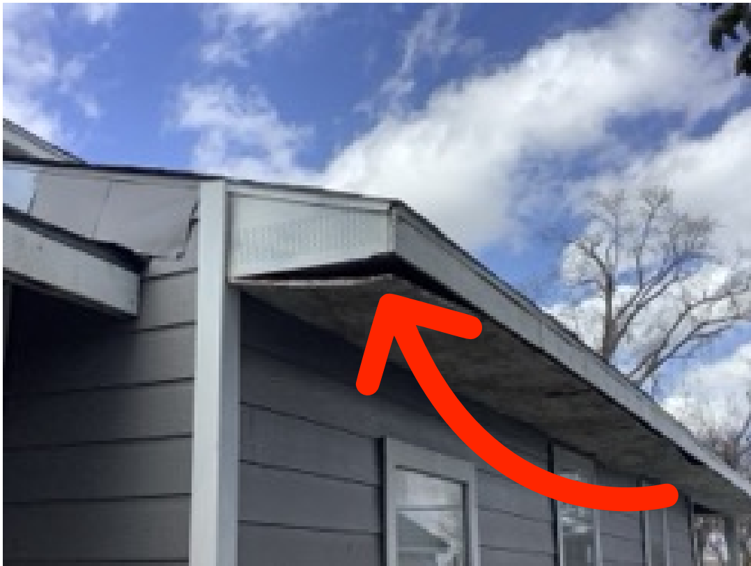
Front Exterior Walls/Siding/Trim Siding warping/pulling away
