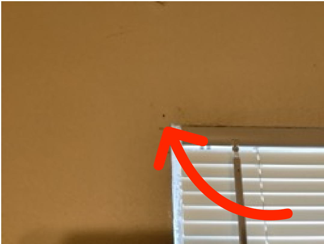
Dining Room Walls/Paint Holes in wall.
