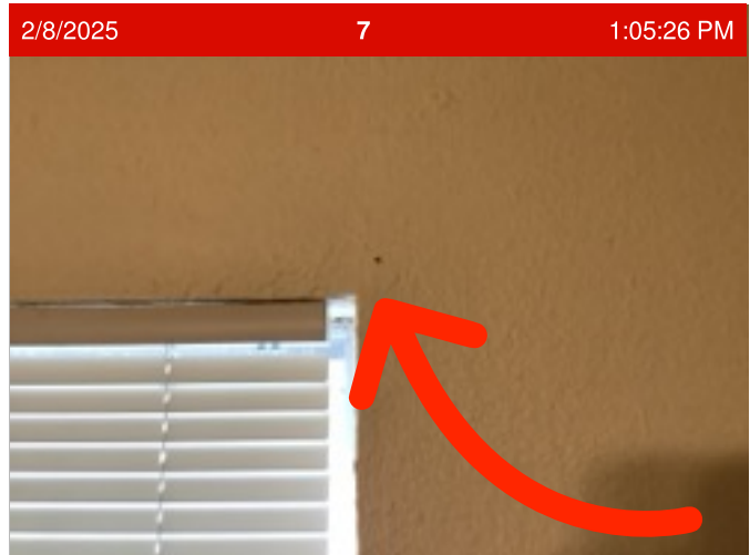
Walls/Paint | Holes in wall.
