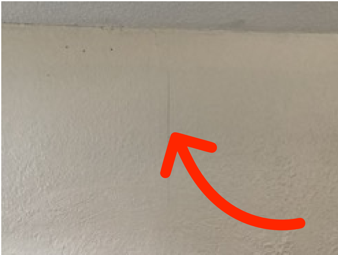
Entry Walls/Paint Cracks in texture
