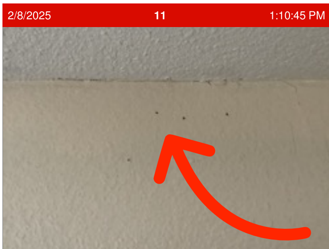
Walls/Paint | Holes in wall.
