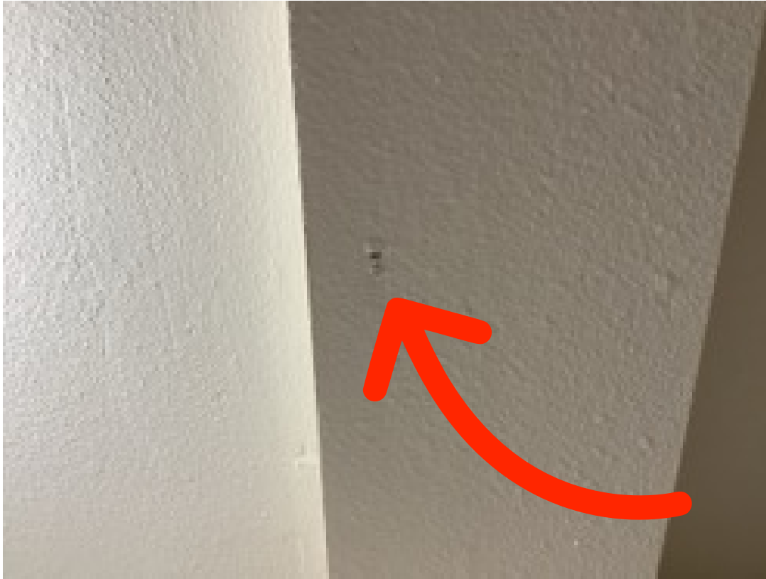
Bathroom 1 Ceiling Holes in ceiling
