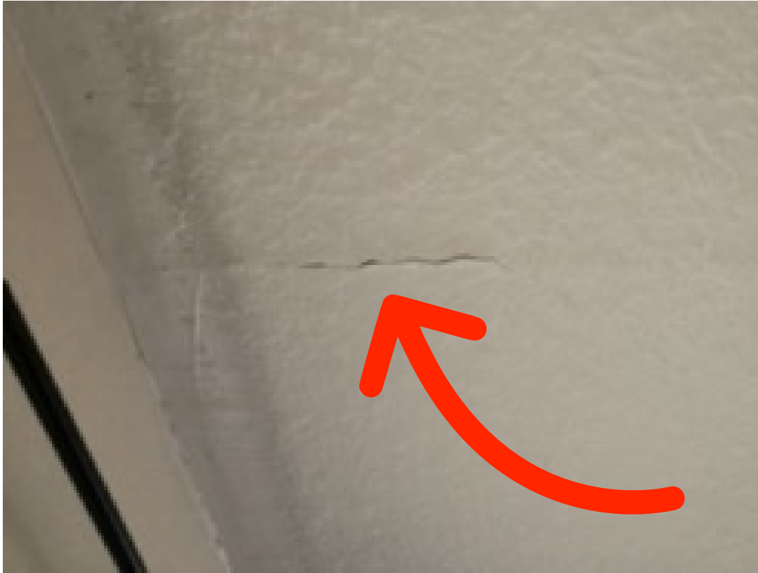
Living Room Ceiling Cracks in ceiling.
