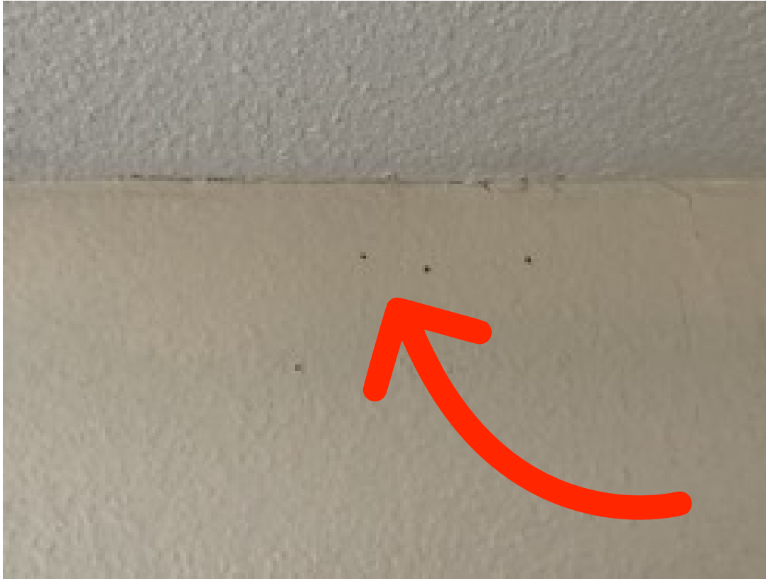
Entry Walls/Paint Holes in wall.
