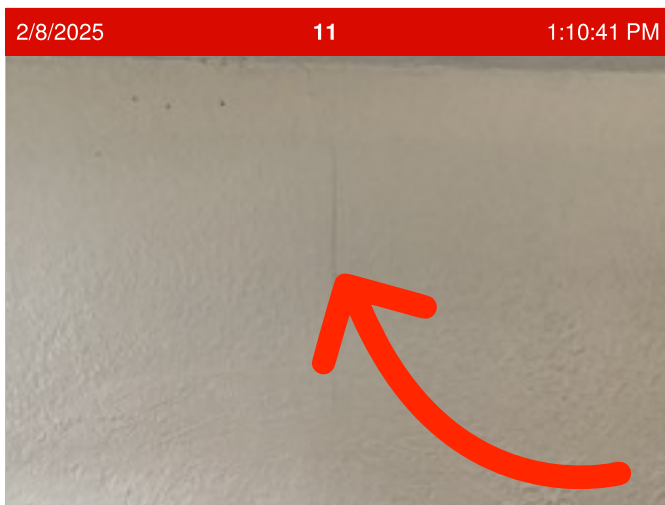
Walls/Paint | Cracks in texture
