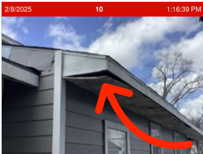
Walls/Siding/Trim | Siding warping/pulling away
