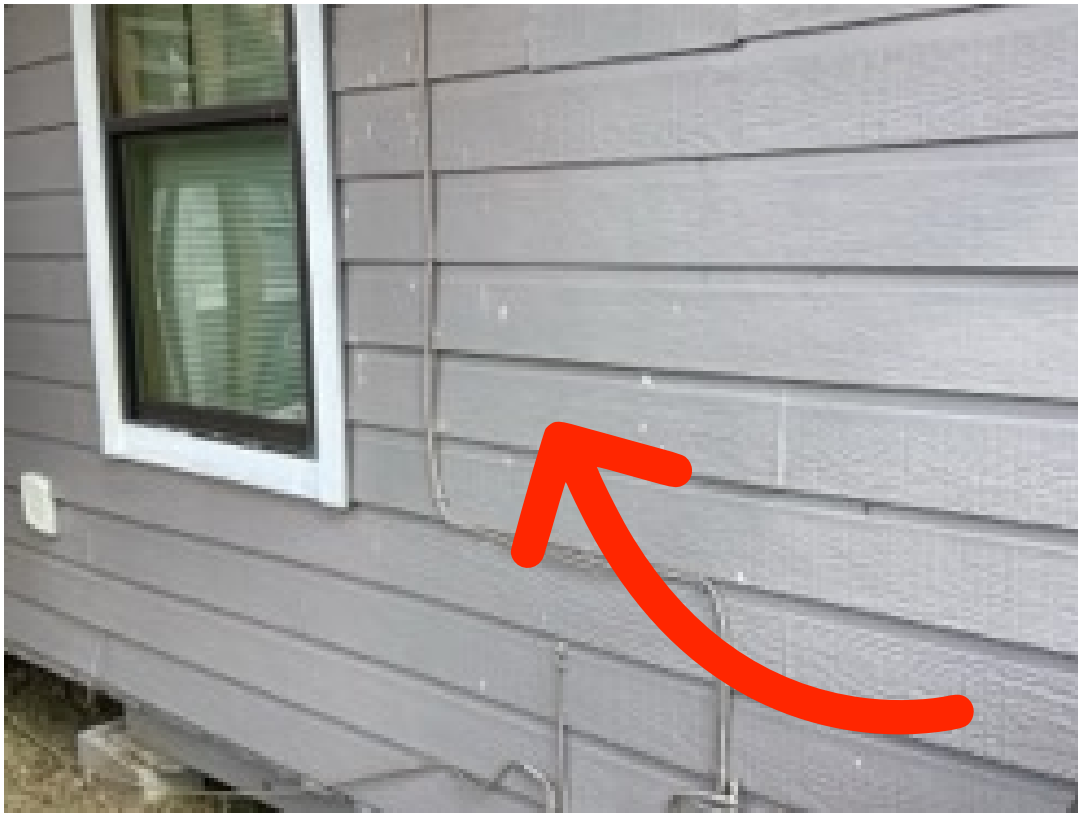
Front Exterior Walls/Siding/Trim Siding is discolored
