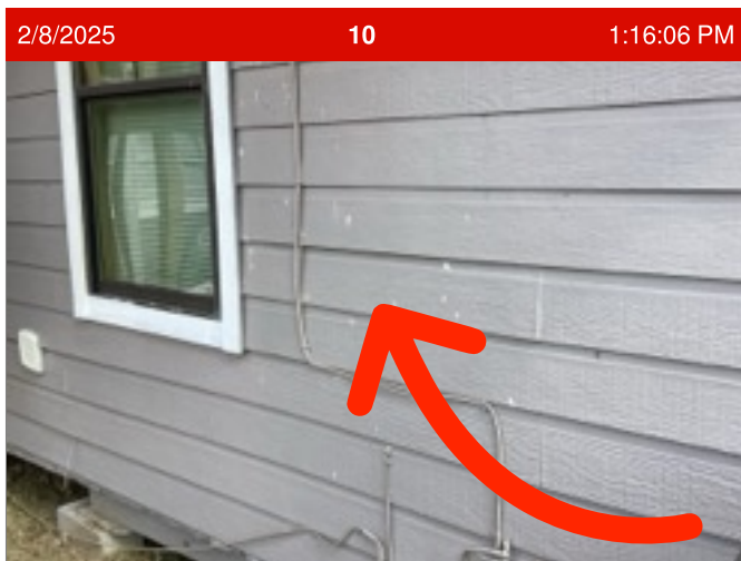
Walls/Siding/Trim | Siding is discolored
