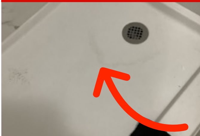
Shower/Fixture | The floor is discolored around the base of the shower pan.
