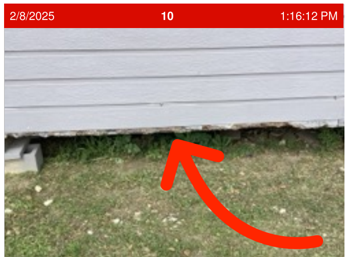
Walls/Siding/Trim | Siding is deteriorating
