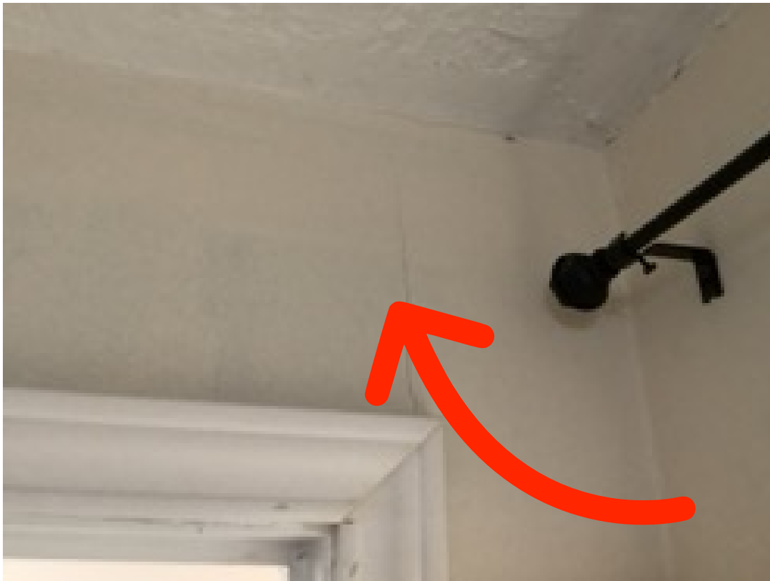
Living Room Walls/Paint Cracks in texture
