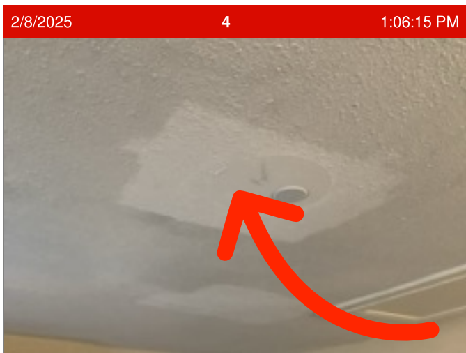
Ceiling | The ceiling is discolored.
