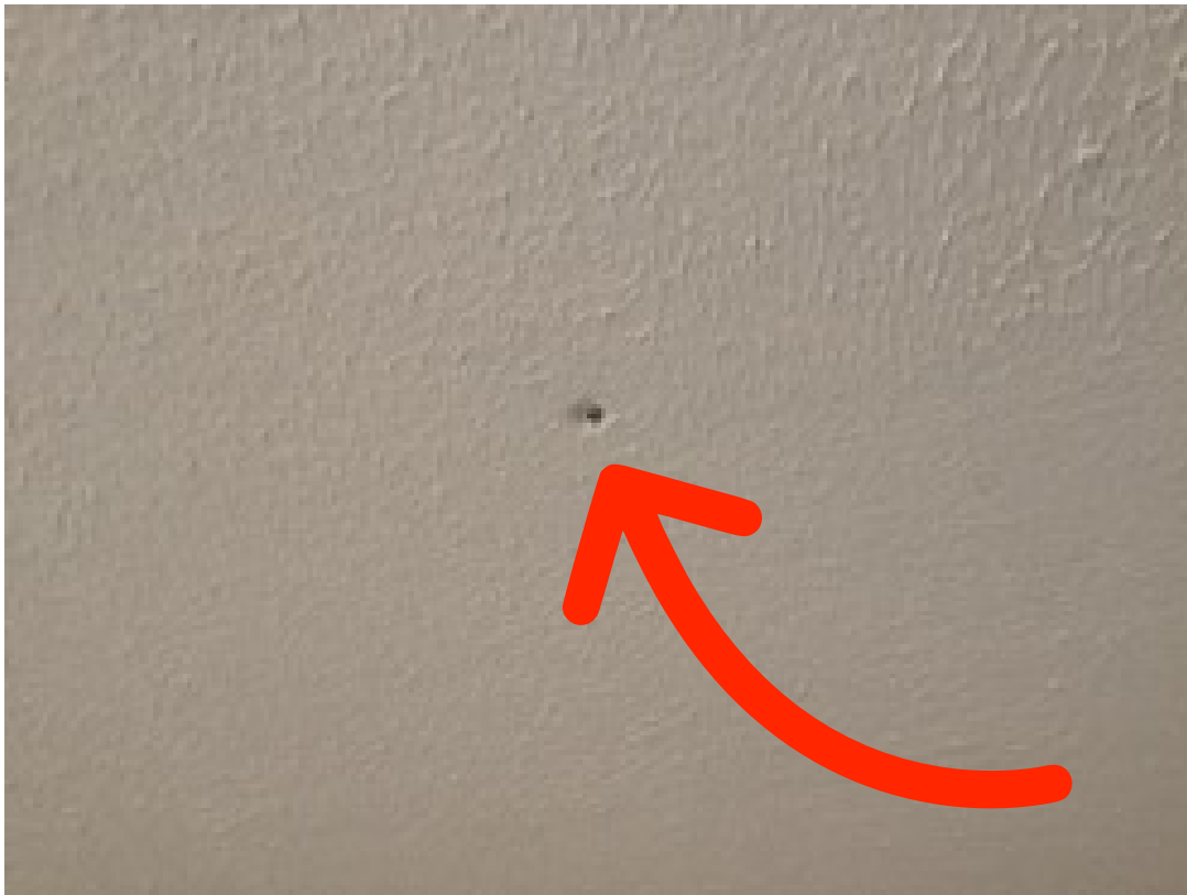
Kitchen Ceiling Nails backing out
