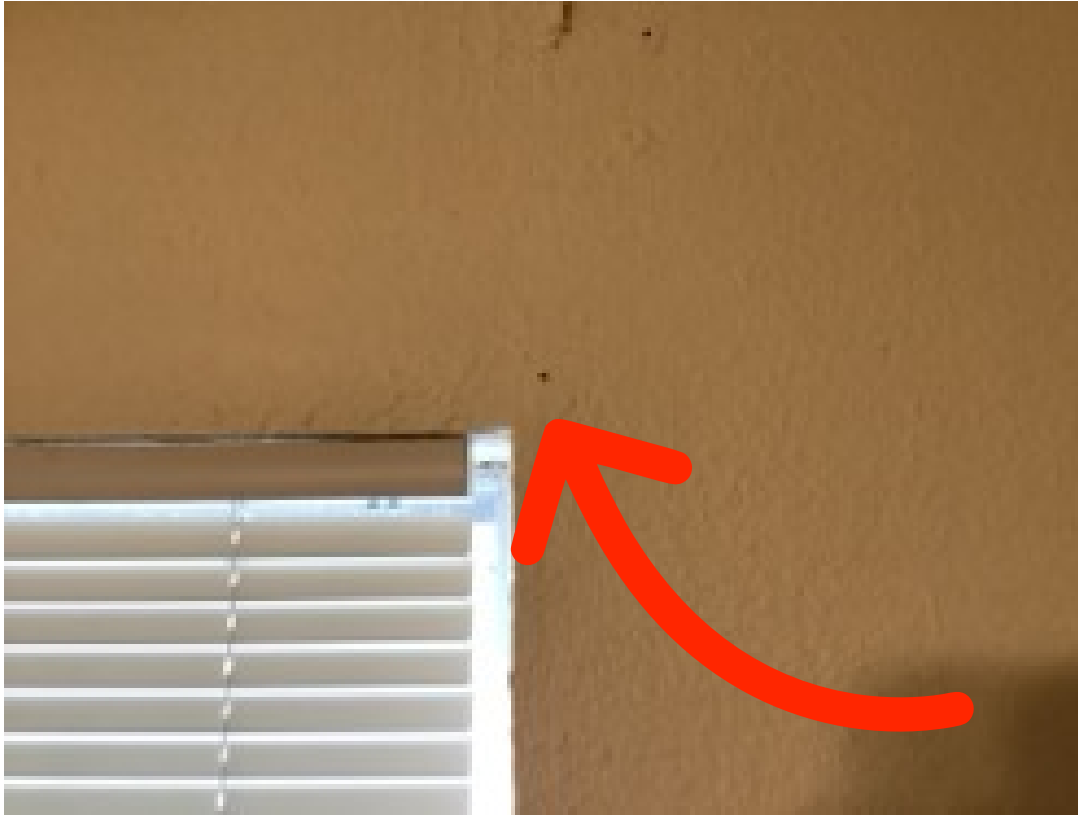
Dining Room Walls/Paint Holes in wall.
