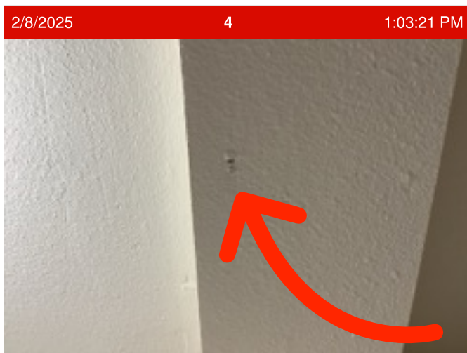
Ceiling | Holes in ceiling
