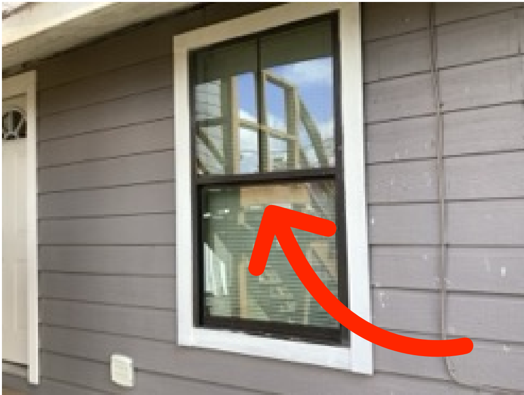
Front Exterior Window Screens Screen(s) are missing
