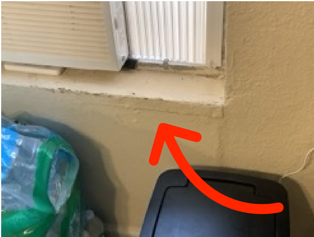
Dining Room Walls/Paint Cracks in texture
