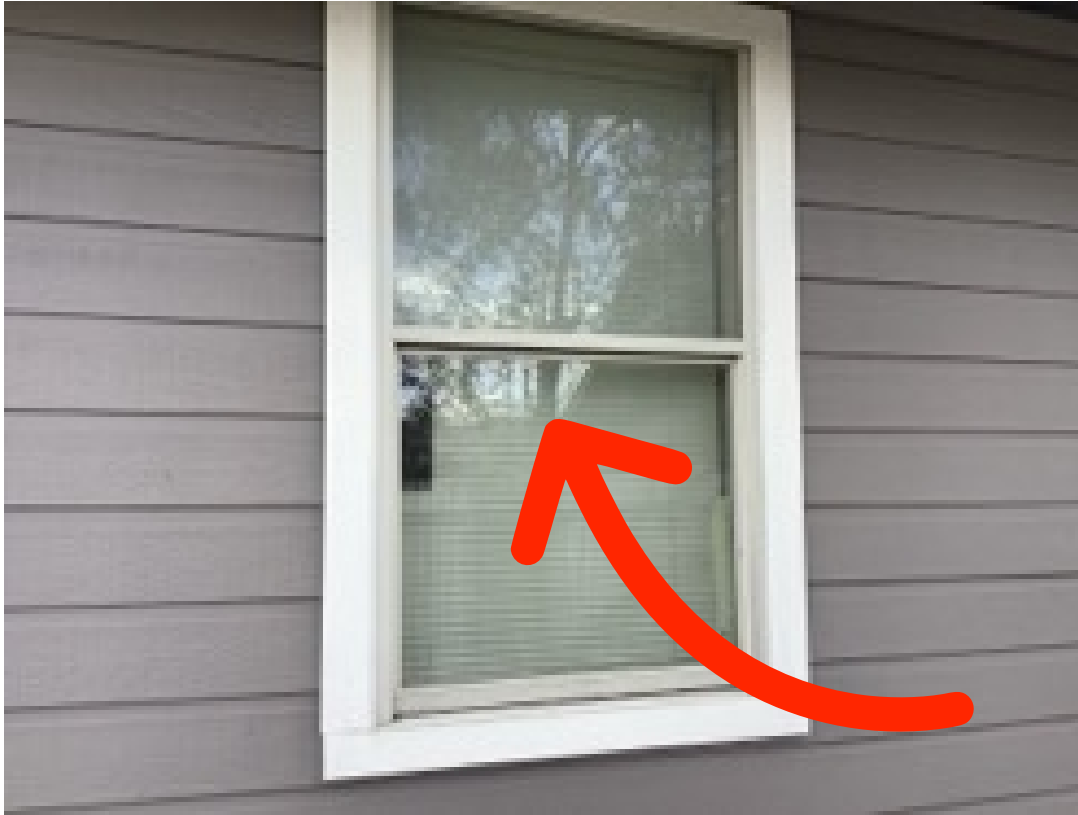
Front Exterior Window Screens Screen(s) are missing
