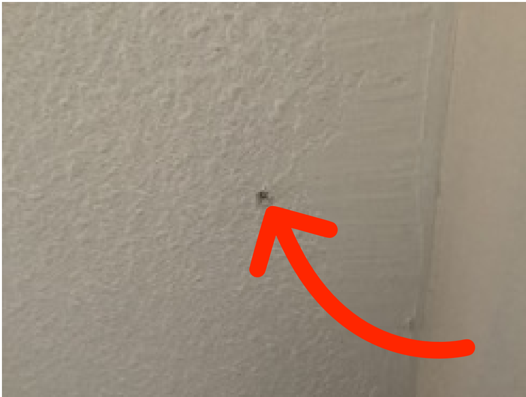
Living Room Ceiling Nails backing out
