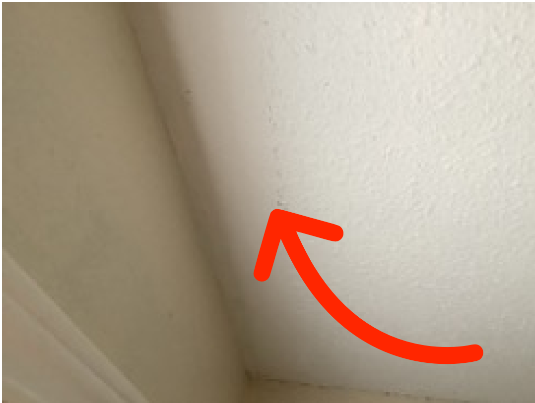
Entry Ceiling Cracks in ceiling.
