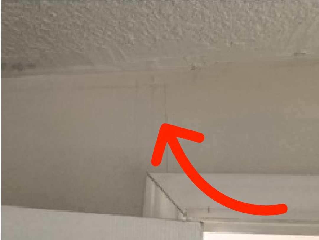
Living Room Walls/Paint Cracks in texture
