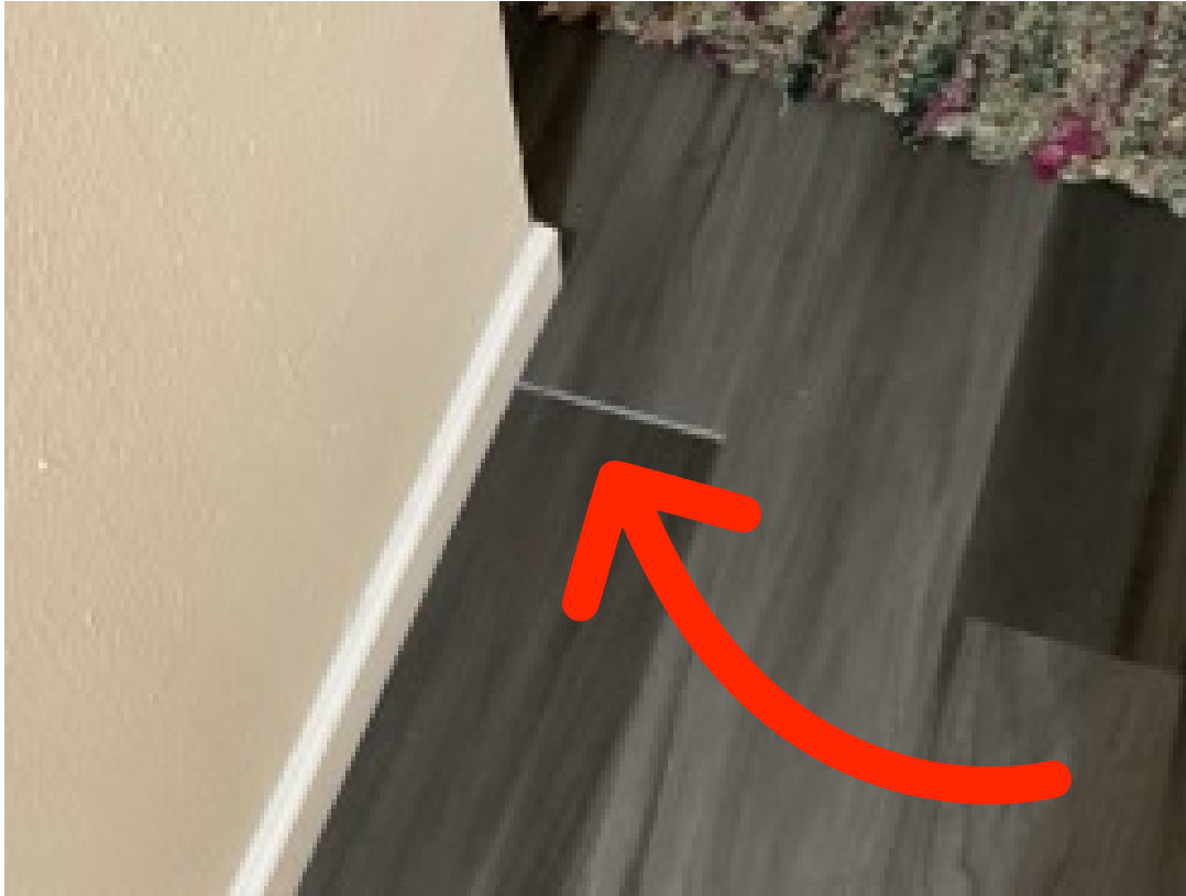
Hallway/Stairway Floors Gap in flooring.
