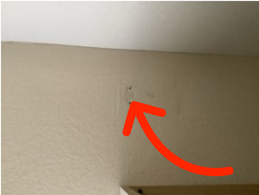
Kitchen Walls/Paint Holes in wall.
