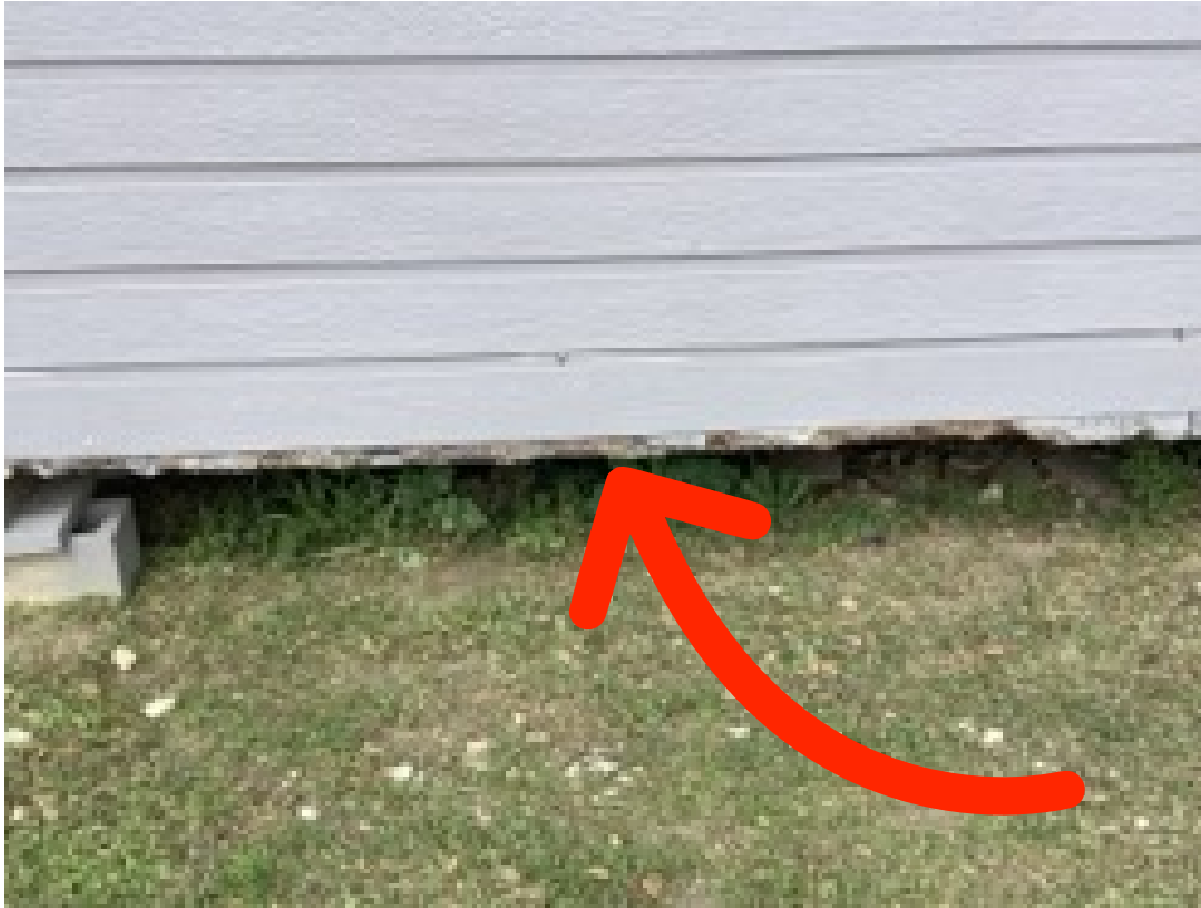
Front Exterior Walls/Siding/Trim Siding is deteriorating
