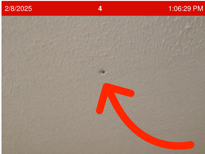
Ceiling | Nails backing out
