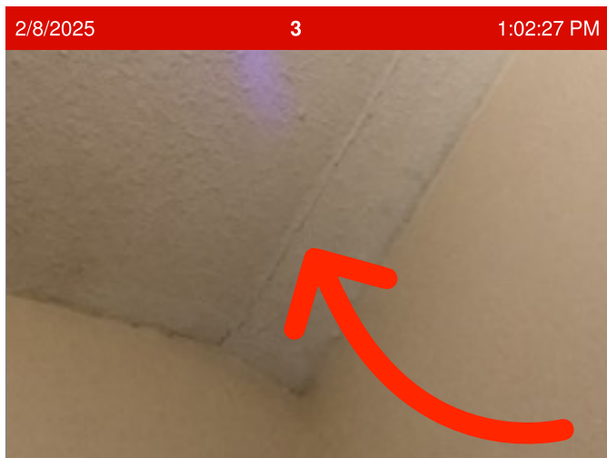
Ceiling | Cracks in ceiling.
