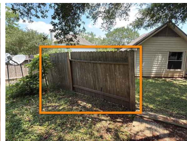
Example Rear - leaning
