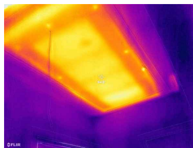
Thermal image of heat transfer at attic stairs
