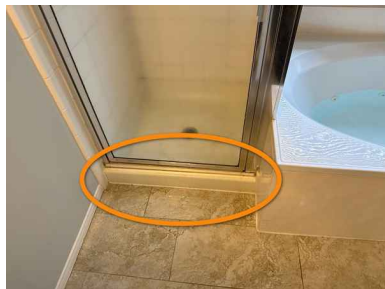
Example 1st Floor Primary Bathroom
