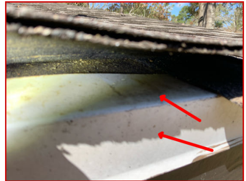
Example of improper felt overlap at drip edge
