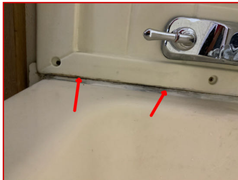
Damaged sealant where tub meets surround
