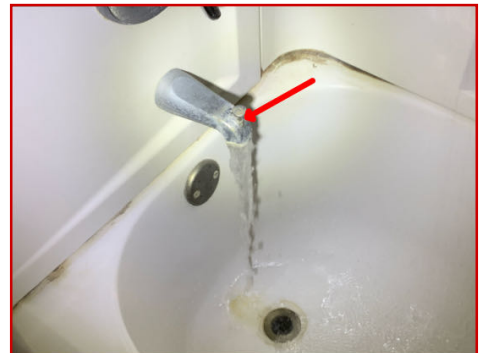
Diverter is inoperable
