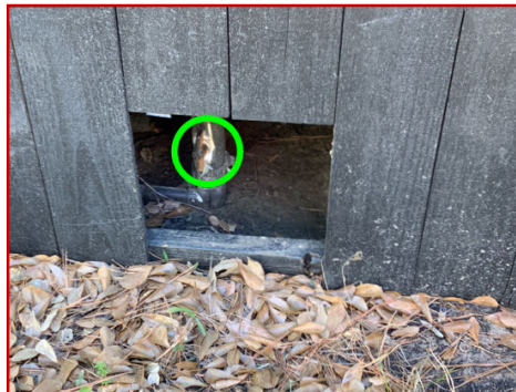
Main water shut off at rear of house
