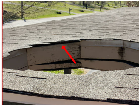
Example of missing drip edge
