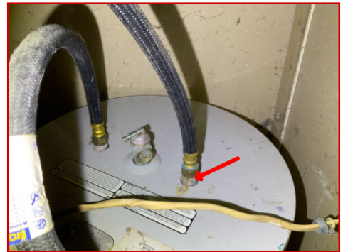
Corrosion visible at water connection
