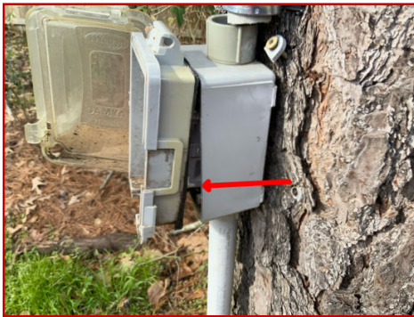
Example of loose exterior receptacle
