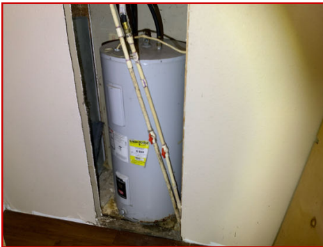
Water heater in bedroom closet
