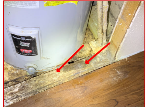
Elevated moisture levels and damage in wall by water heater
