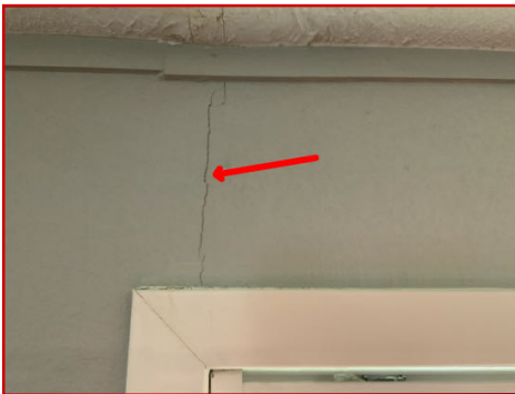
Example of wall cracks
