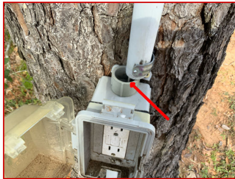
Example of damaged conduit on tree to left of house
