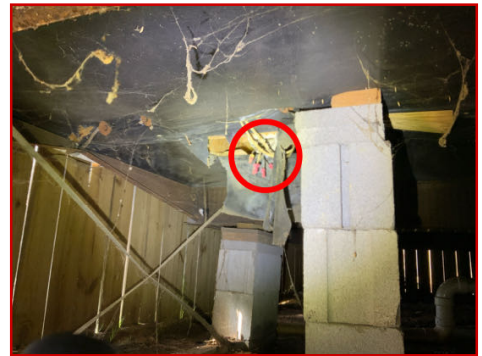
Missing junction box cover in crawlspace
