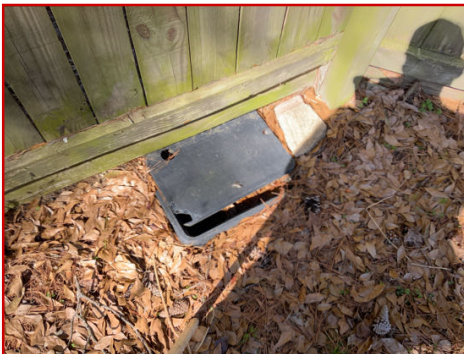
Water meter in right rear of property
