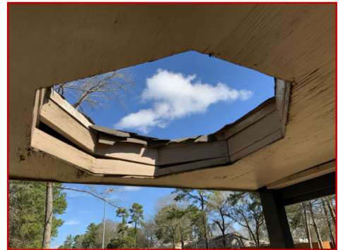
Hole in cover for tree that has been removed
