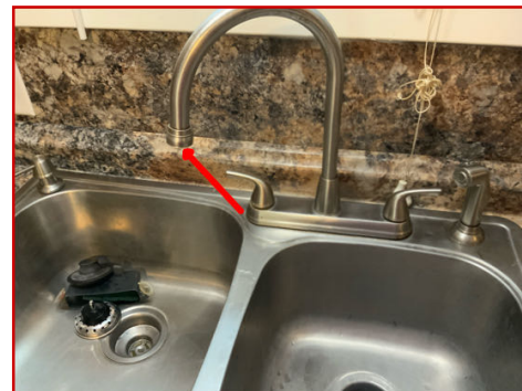
Kitchen faucet leaks when not in use
