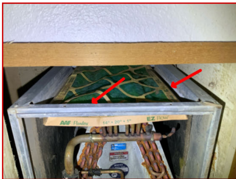
Example of damaged filter
