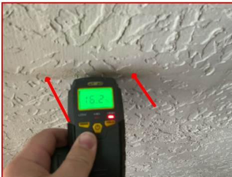
Moisture stain in living room ceiling, elevated moisture levels detected at inspection
