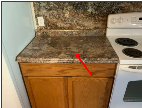
Example of loose counter top
