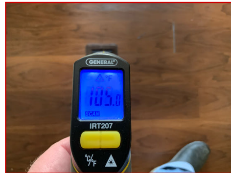
Furnace producing approximately 105° F at register
