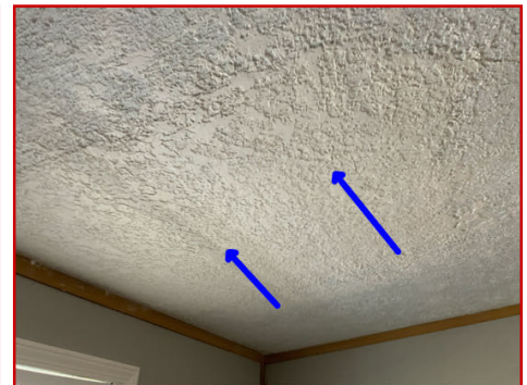
Example of ceiling patches
