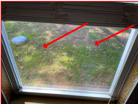
Example of missing screens
