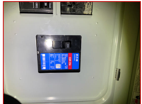
Sub panel, 200 amp main shut off
