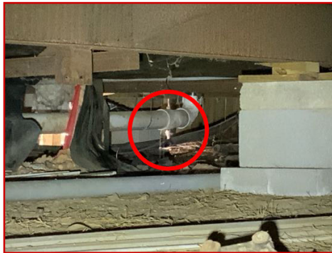
Leaking drain in crawlspace
