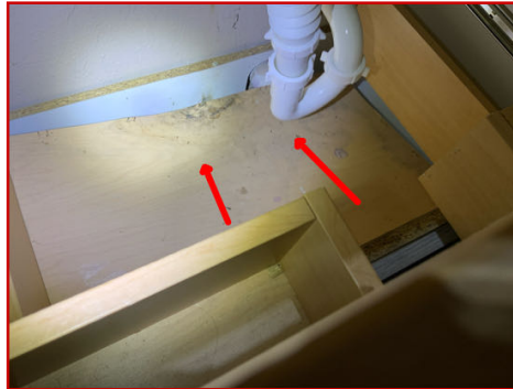
Bathroom vanity cabinet floor, past moisture damage, dry at inspection
