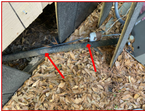
Deteriorated insulation at coolant lines
