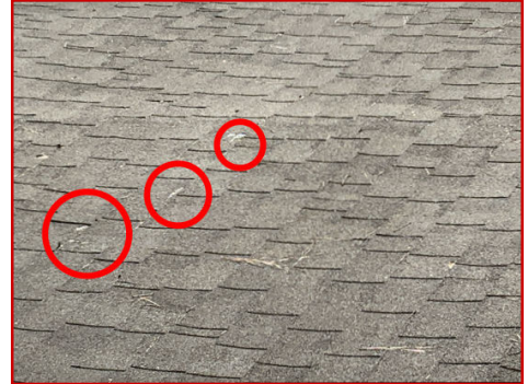
Example of fiber glass visible in shingle surface
