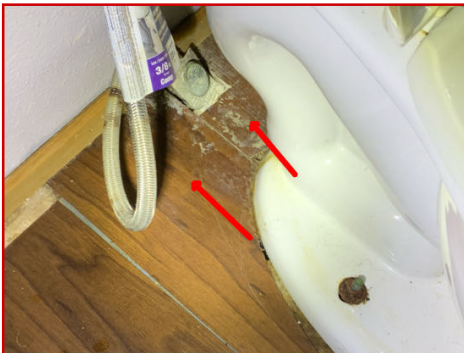
Sub floor behind toilet is completely deteriorated
