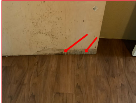
Elevated moisture levels and damage visible in water heater panel
