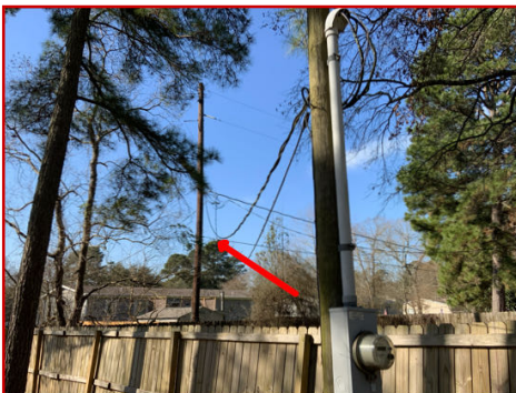
Overhead service proximity to trees, trespasses neighbor's property
