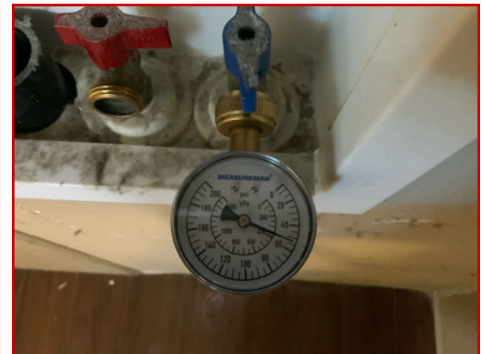
Static water pressure approximately 50 psi
