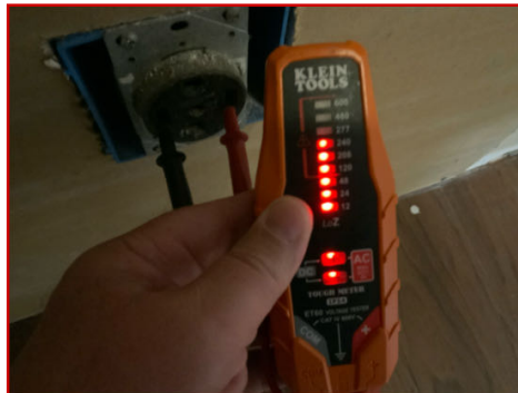
4 wire dryer receptacle is functional at inspection
