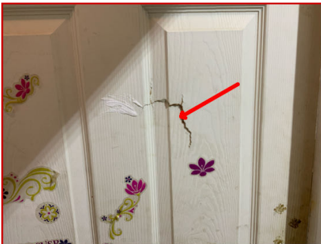
Example of damage to interior door
