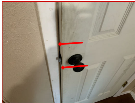
Closet door binds on jamb, will not close
