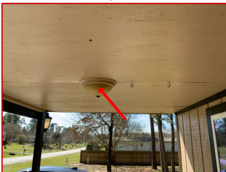
Example of inoperative exterior light
