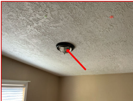
Example of missing diffuser
