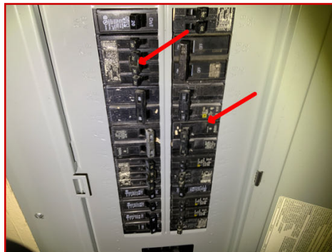
Sub panel, different brand breakers
