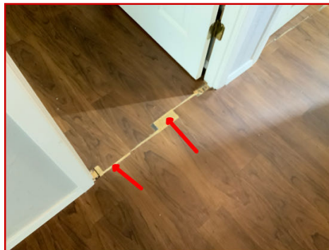
Incomplete flooring installation/exposed subfloor
