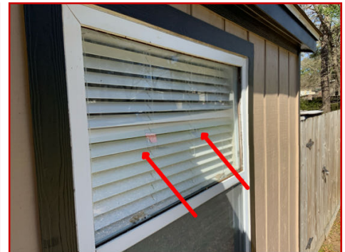
Master bedroom, broken window
