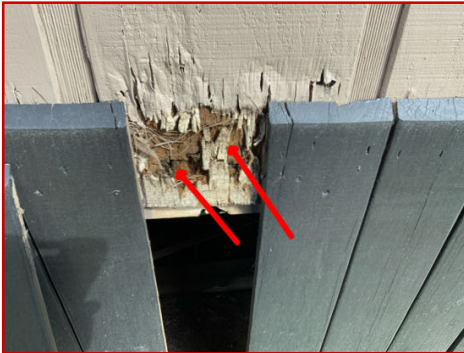
Example of damaged siding
