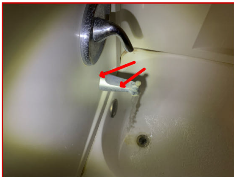
Tub spout is loose/missing sealant
