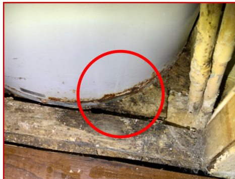
Rust and possible leak visible in water heater casing
