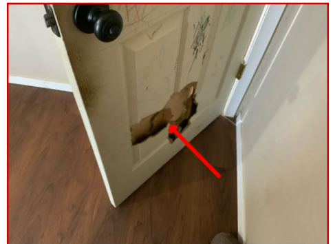
Example of interior door damage
