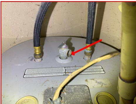
TPR valve improperly terminated
