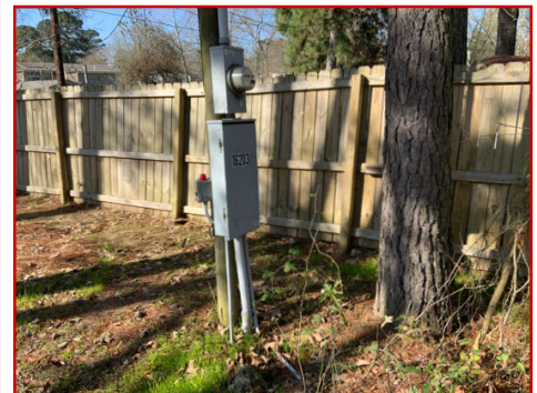
Service panel, meter and driven rod ground on pole to left of structure
