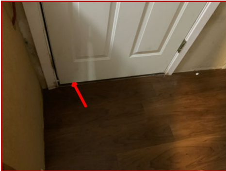
Rear entry binds on threshold
