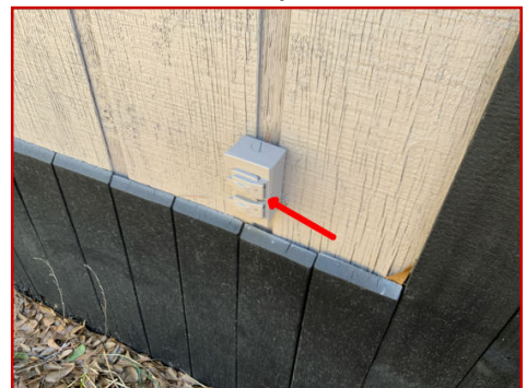
Exterior receptacle, no GFCI
