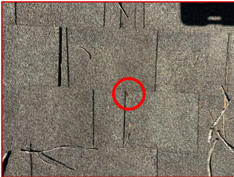
Example of exposed nail heads
