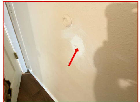
Example of door knob damage in bedroom
