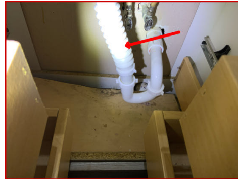
Example of accordion style drain line in bathroom
