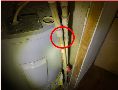
Water leak in pipes by water heater
