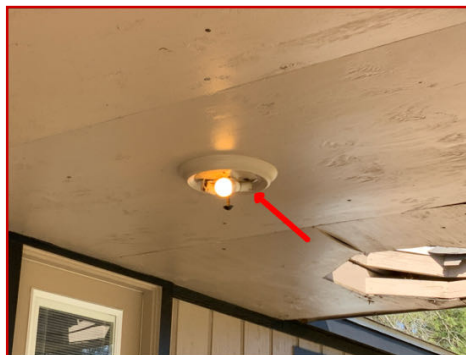
Example of missing diffuser at exterior light
