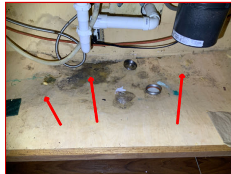
Elevated moisture levels and damage to kitchen sink cabinet
