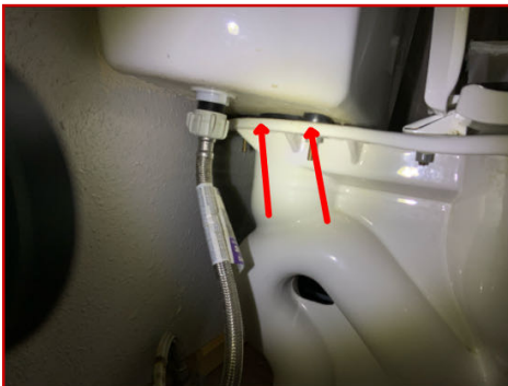
Hallway bath, leak at toilet tank
