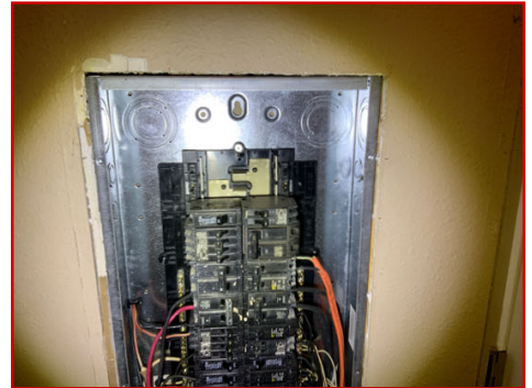
Sub panel, interior
