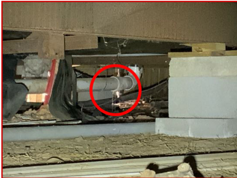
Example of leaking drain in crawlspace
