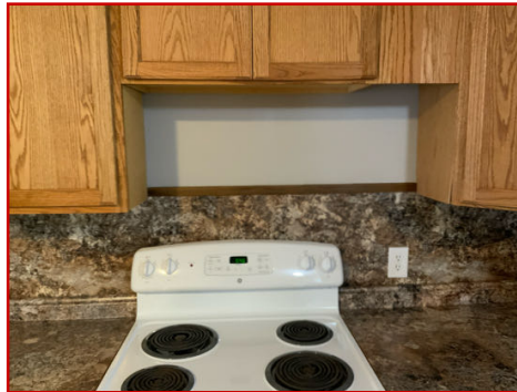
No vent hood
