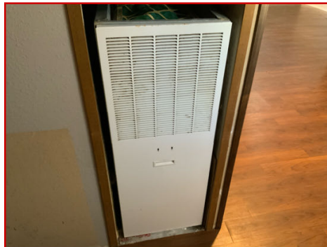
Furnace in laundry area
