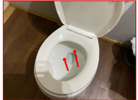
Hallway bathroom, toilet runs continuously
