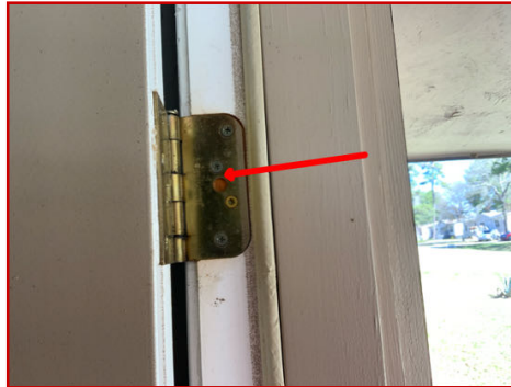
Loose hinge/stripped screws at front door
