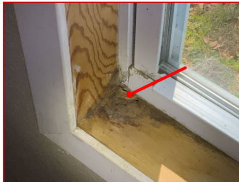
Example of deterioration at interior window sill
