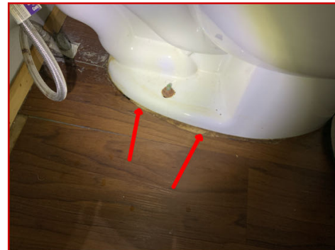
Elevated moisture levels in sub floor at toilet
