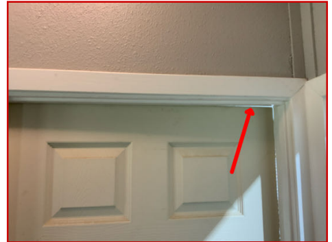
Example of uneven interior door
