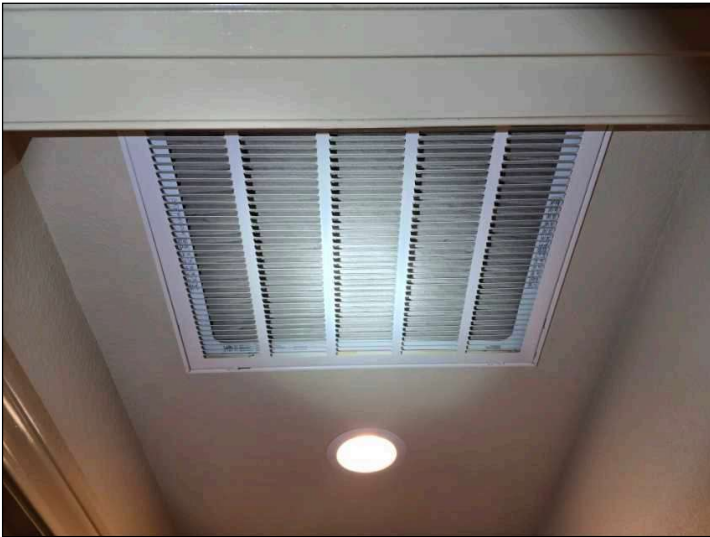
Filter is dirty
