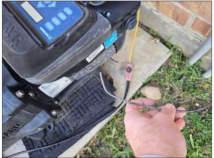
Missing bonding wire from pump to pump.
