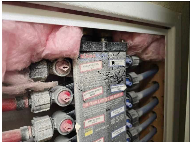
Missing PEX valve wrench
