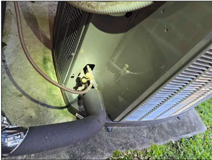
Missing locking refrigerant caps. These caps prevent tampering and possible chemical abuse.
