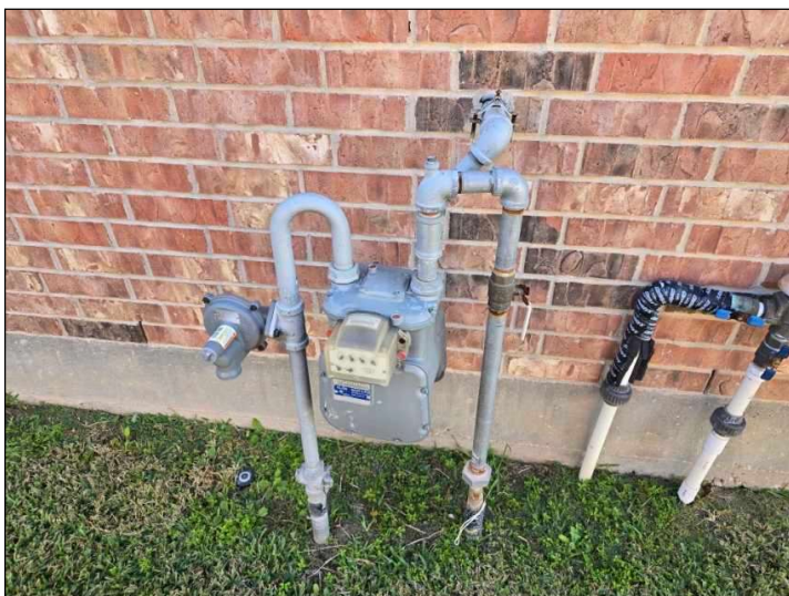
Gas Meter and Shutoff Location.
