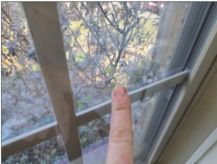
Missing / damaged screens noted.
