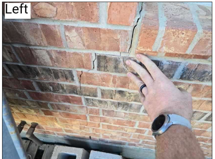
Exterior cracks in brick veneer noted. Cracks located at window corners are from settlement or uneven weight distribution.
