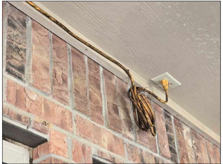
Cord outside used as permanent wiring. Noted this may be removed.
