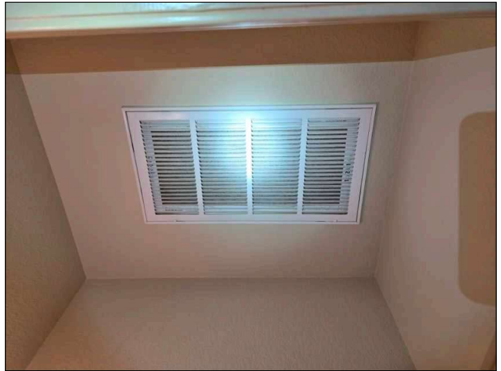
Filter is dirty
