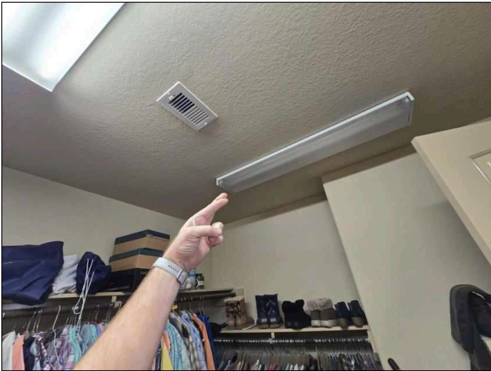
Bedroom closet light fixture does not working.
