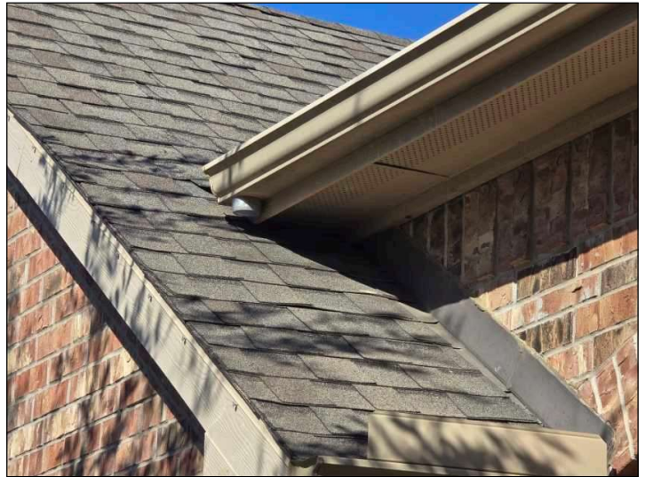
Gutters terminate on top of shingles. Gutters should extend to the ground or to another gutter. Shingles may wear faster in this area.
