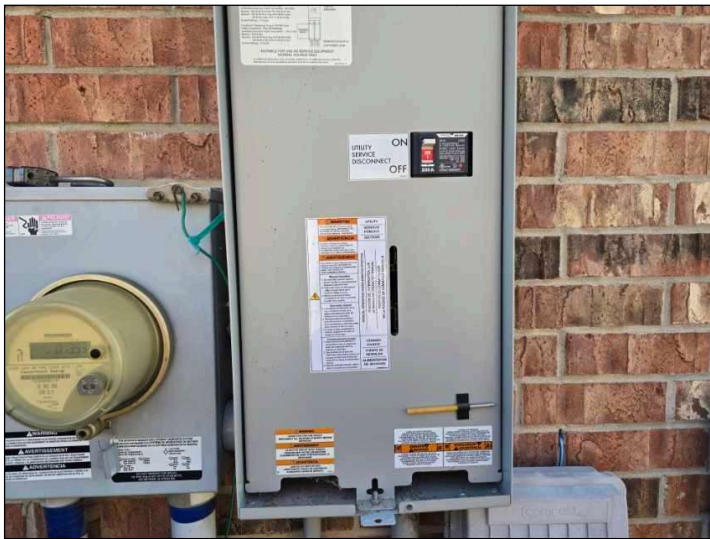
Automatic transfer switch installed. Not tested.
