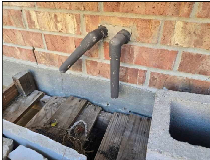
Water heater vent and drain lines. If water is seen coming from here, contact plumber for evaluation.
