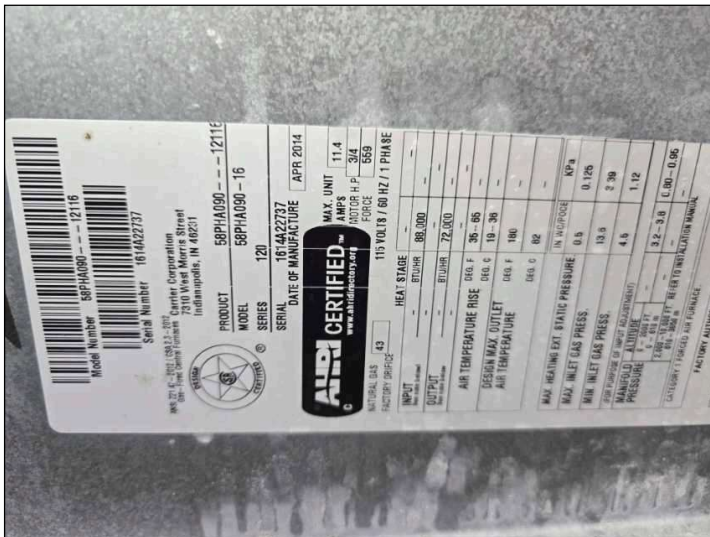
Estimated Age of Furnace :2014 88k btu gas furnace
