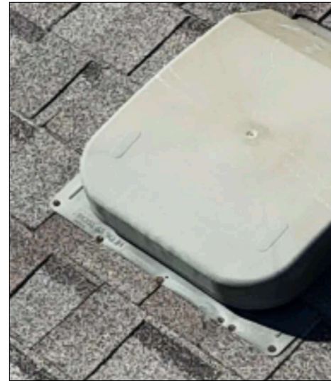
Exposed nails should be sealed over.
