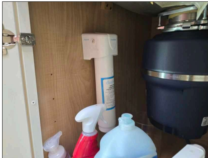
Under sink filtered water not used.
