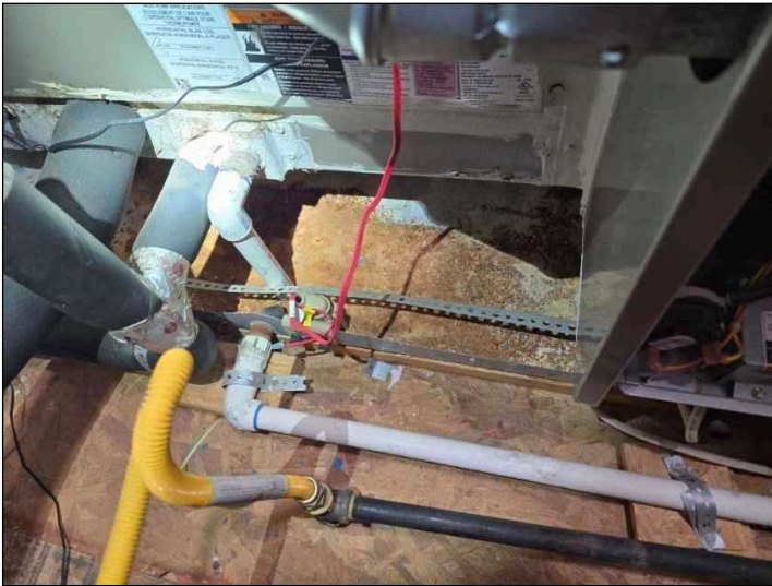
Heavy rust in overflow pan. Recommend replacement of overflow pan, as rust can cause holes to leak.
