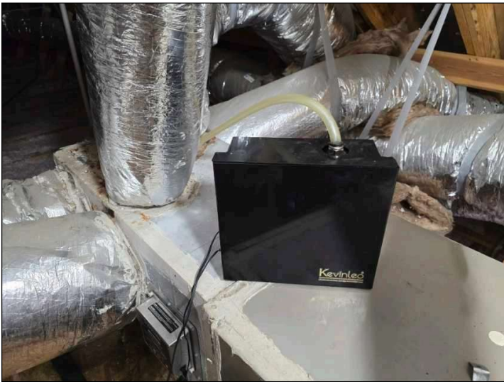
Home has a scent smelling box added to supply plenum. May add an oily substance inside insulation board that cannot be cleaned. Do not suggest using this device.
