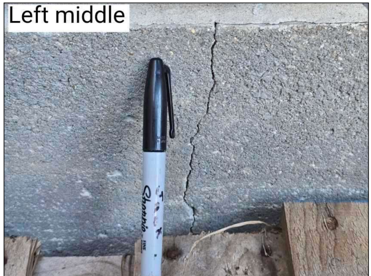
Visible crack in foundation is beginning to separate and has caused brick cracks. Left side.
