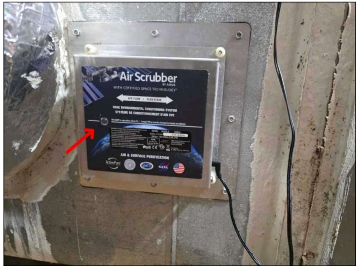
Air scrubbing UV light device is installed. Not functioning according to light.
