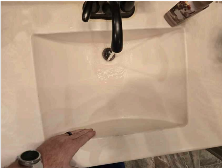
Note that lavatory does not have an overflow vent and can easily overflow. Use caution.
