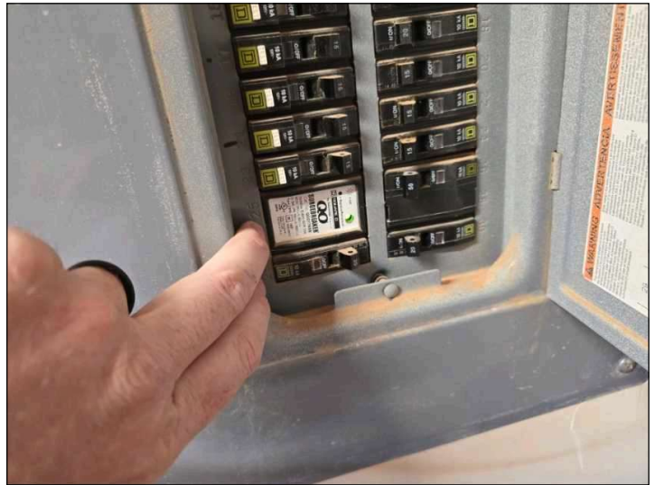
Surge protector should be closest to main disconnect in a Square D Panel.
