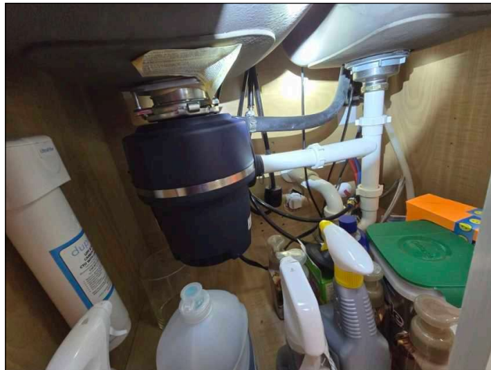
Operated - appeared functional at time of inspection.
