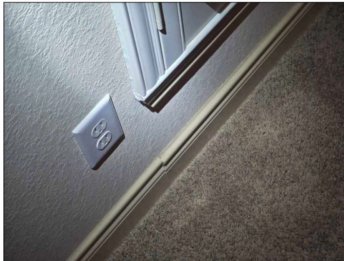
Trim separation noted in master bedroom. No moisture found.
