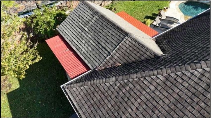
Back patio shingles were not tied into existing shingles correctly. Played over existing roof.
