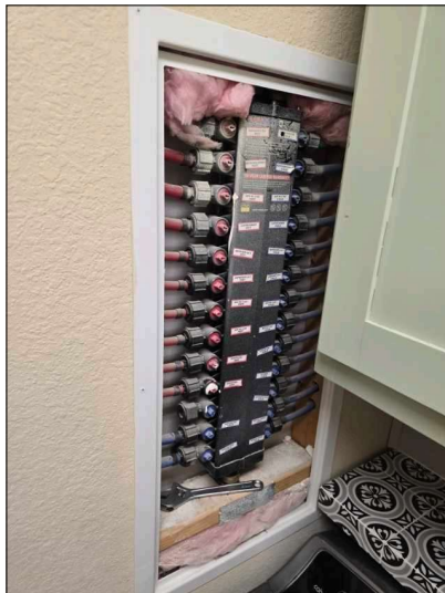
PEX manifold present inside house. Check periodically as these tend to leak. No leaks at time of inspection.
