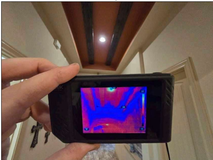
Missing insulation in some places. Noted via thermal camera.
