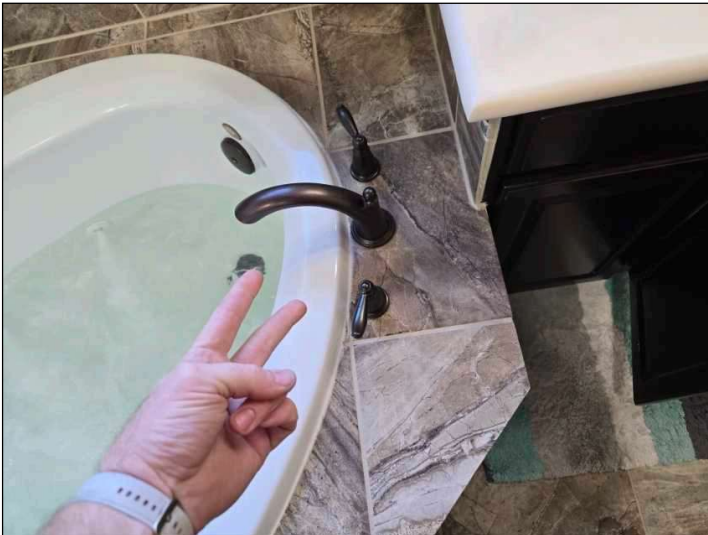
2 handle tub present without a temperature regulating mixing valve present / found. This allows for a max temperature to be preset to avoid scolding.
