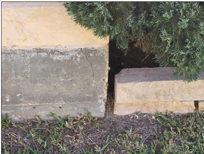
Corner pop noticed. Corner sections of the foundation are not supported as much as rest of foundation. This is not typically an issue, but take notice if cracks begin to form in bricks or mortar above corner pop.
