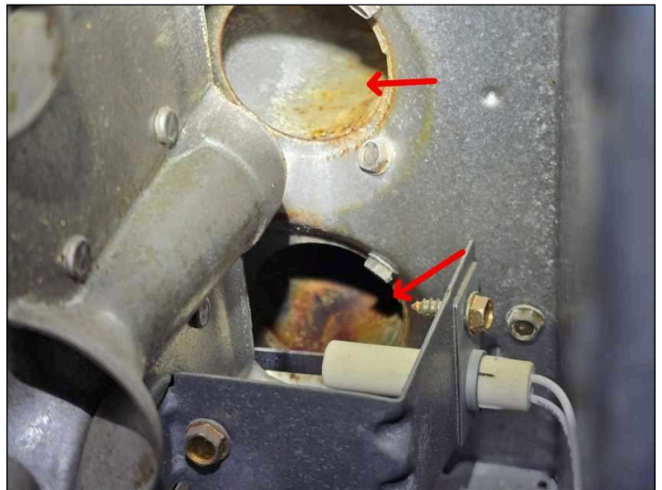
Rust / corrosion found on furnace burner tubes. Possible rust corrosion on heat exchanger. Suggest having HVAC contractor perform a maintenance inspection for CO leakage.
