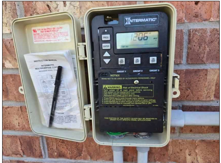
Pool previously had a time box added for various functions. This is no longer used as the motor is now a variable speed motor.
