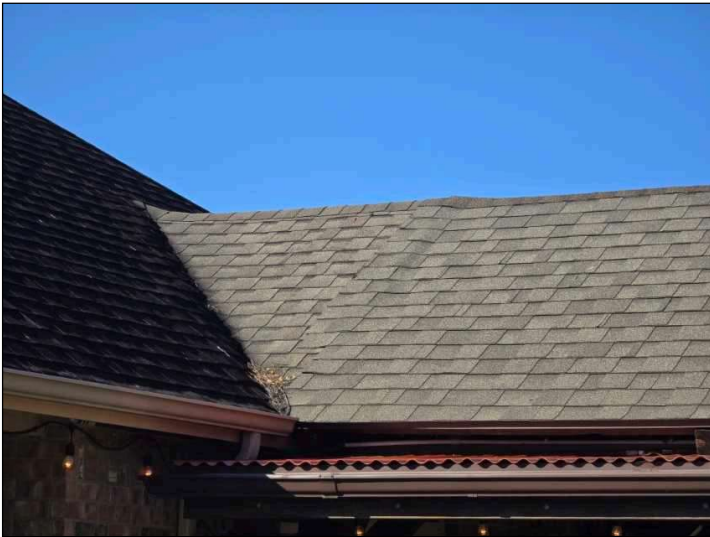
Back patio shingles were not tied into existing shingles correctly. Played over existing roof.
