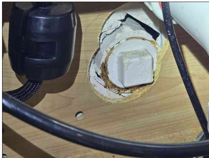
Noted that kitchen drain has some debris around threads. No signs of leaking. Monitor.
