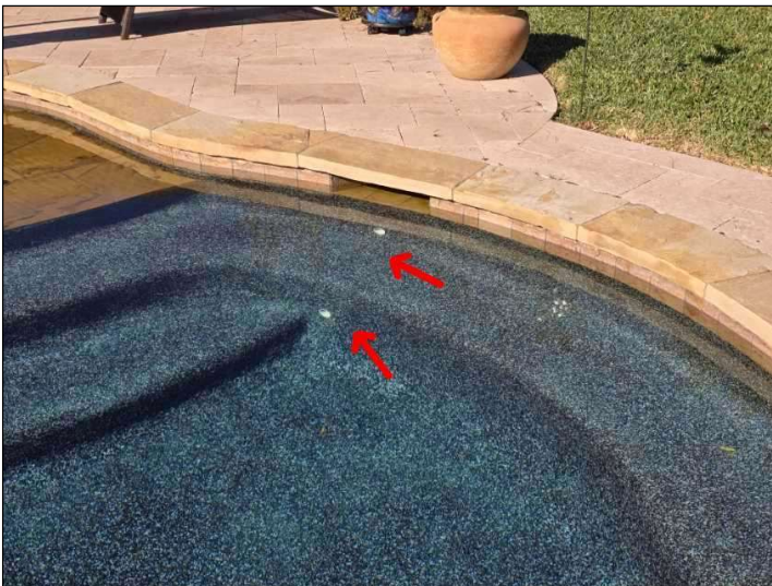
Skimmers were clean. Added cleanout ports can be plugged as desired.
