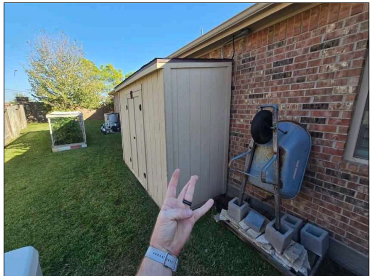
Middle bedroom window is permanently blocked by storage building. This window is no longer an egress window and limits the use of this room as a sleeping / bedroom.
