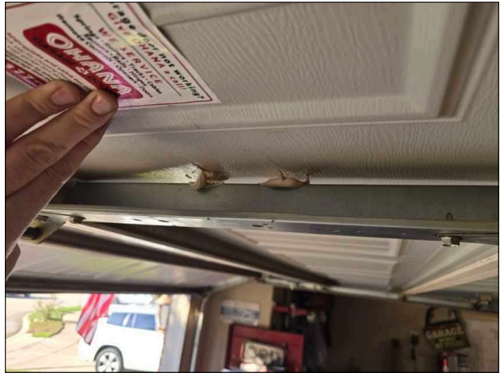
Glue from panels and frame has come loose. This glue helps secure the structure.
