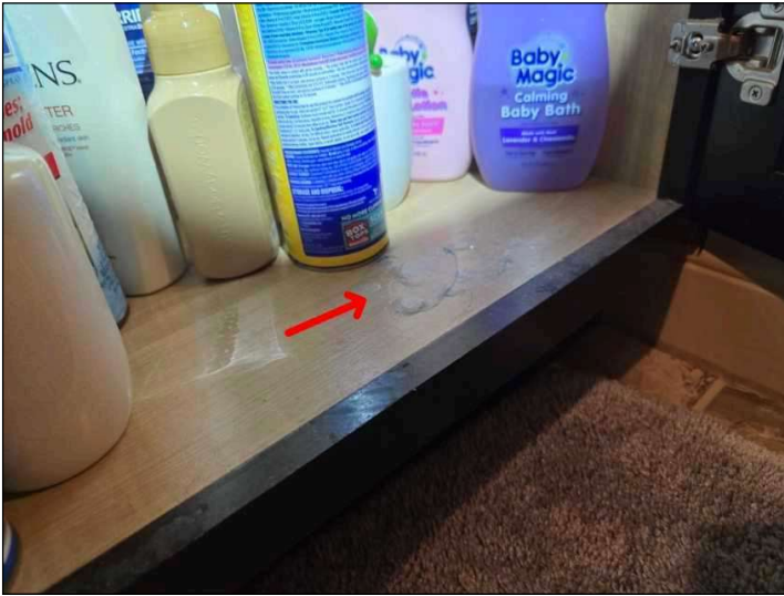
Damaged cabinets noted. Possible spill / leak could be reason.
