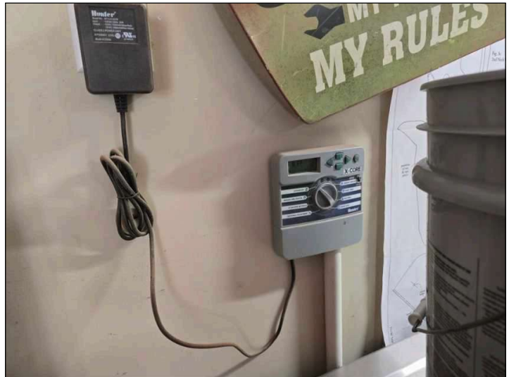
Missing labeled zones and / or irrigation installer license.
