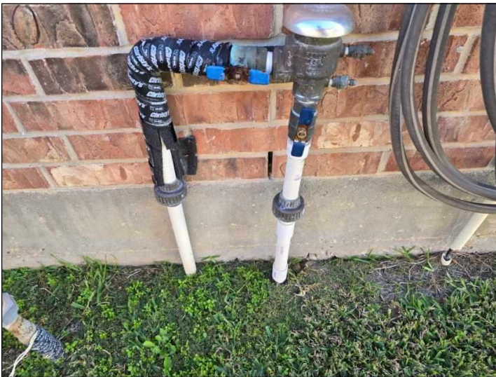
Exposed piping missing some insulation.
