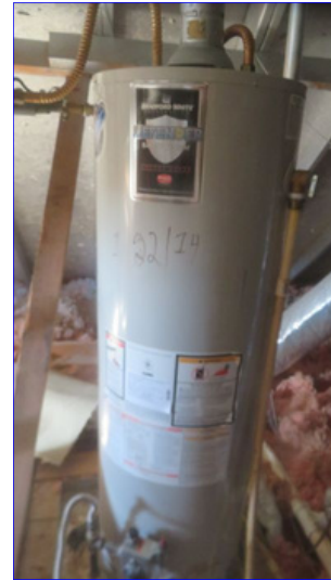
The water heater(s) appeared to be properly installed at the time of inspection.
