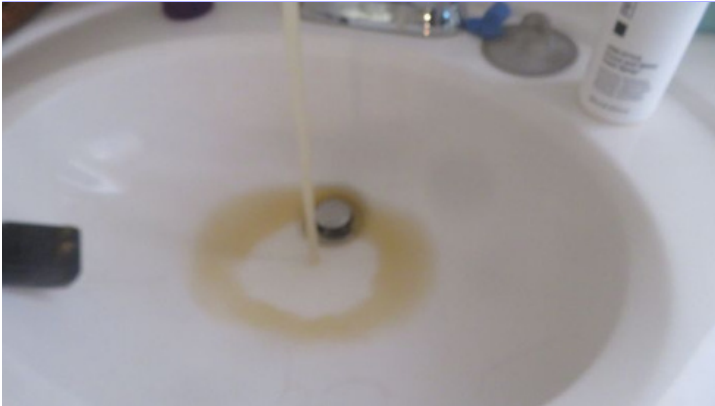
Rust colored water was observed. This is typically caused from sediment in the tank or lines. The tank/lines may need to be flushed. Recommend further evaluation.
