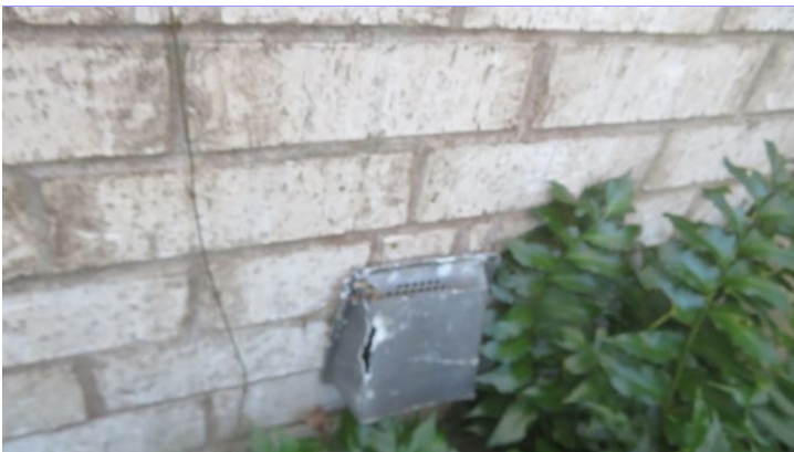
The exterior wall vent(s) appear to be damaged. Recommend repair.
