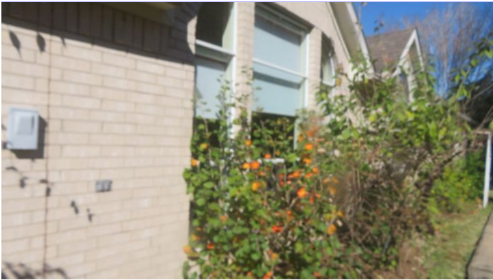
Vegetation is in contact with or has insufficient clearance of exterior walls. It is recommended vegetation be cut back at least 12-18 inches from exterior walls.
