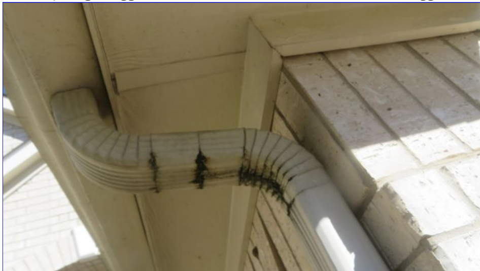
Minor leaks in the gutters should be repaired.
