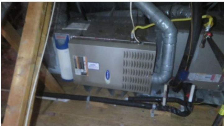
View of the Heating/ evaporator Unit.
