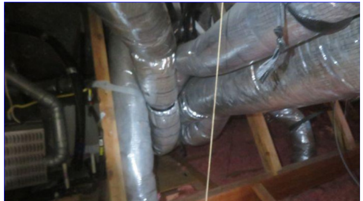
Observed "Contact" of the ductwork between other ducts/surfaces. Separation can be as simple as placing a piece of insulation between the ducts/other surfaces. Further evaluation and improvements are recommended.
