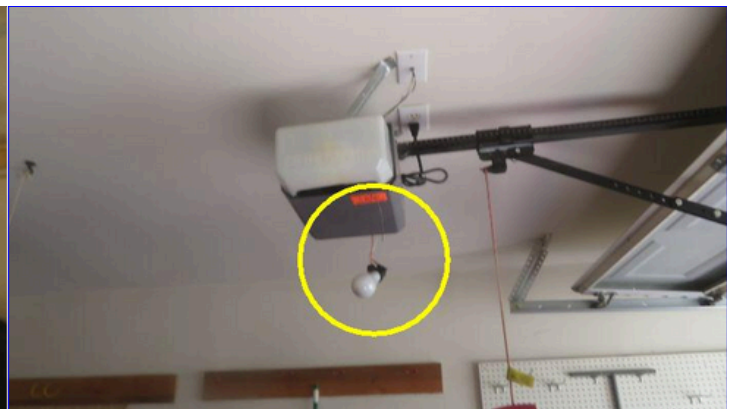
Light bulb on the garage door opener was inoperative at the time of inspection.
