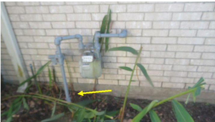
The Main gas shut-off. This is informational only.
