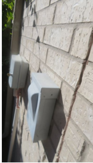
Seals around panel/service boxes/fixtures/access covers/outlets/switch boxes are incomplete/ missing. Panel/service boxes etc, should be properly sealed on top and both sides only.
