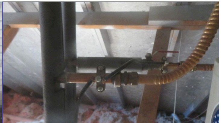
Note: Verified "Bonding" of the gas piping system. This is informational only. (see pics)
