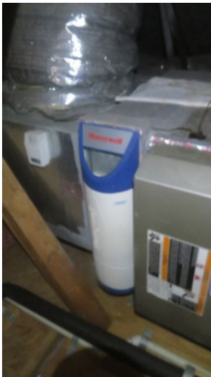
Observed a "Media Air Filtration System" as part of the HVAC system.
