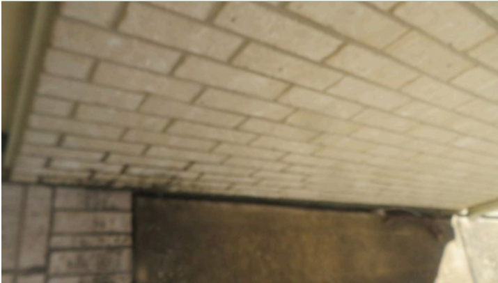
Gutters over spilling. Clogged
