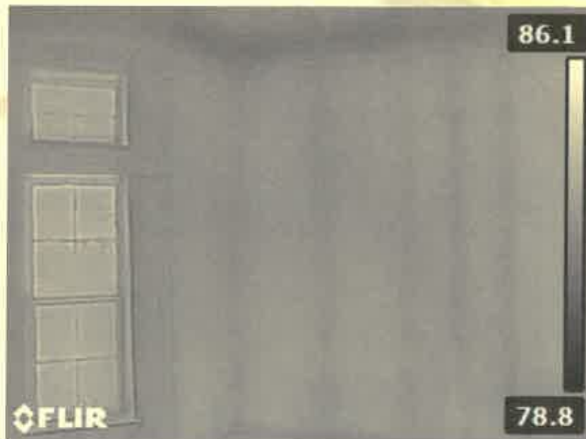
Infrared picture of your home's interior wall.
